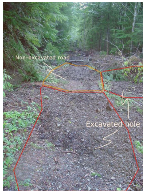
Photo C. Decom potholed road.
