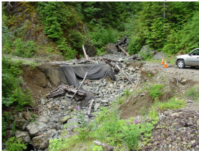
Photo S. A washed out stream crossing.
