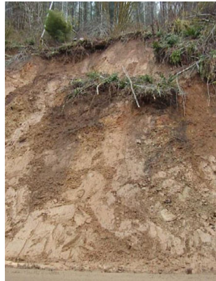
Photo G. A slumping cutslope.
