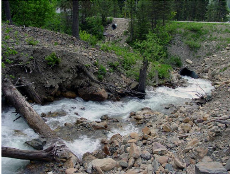
Photo T. Debris flow at a stream crossing. Notice the mass of sediment intermingled with buried logs.
