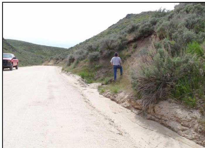
Figure 8. A scalloped cut above a ditch relief culvert.
