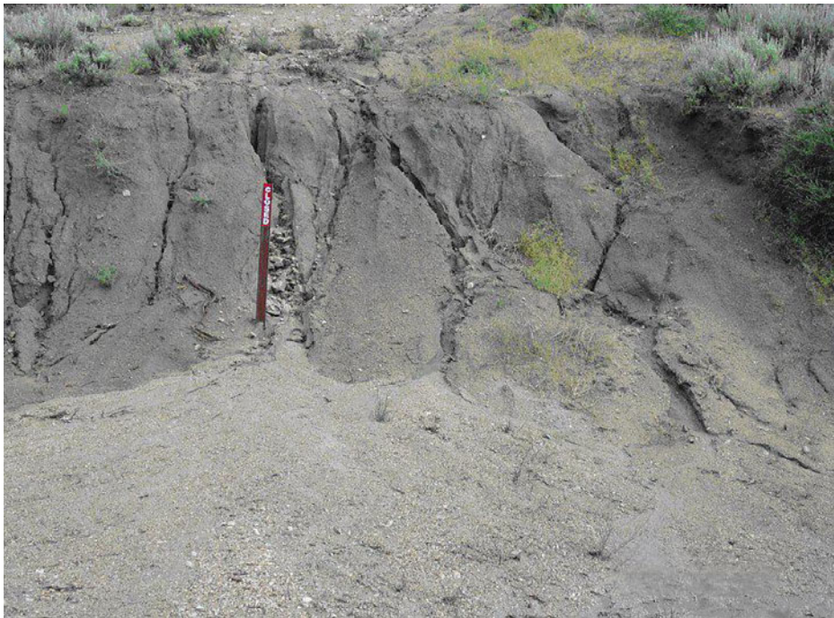
Photo E. Badly rilled cut slope following high intensity rainfall event.
