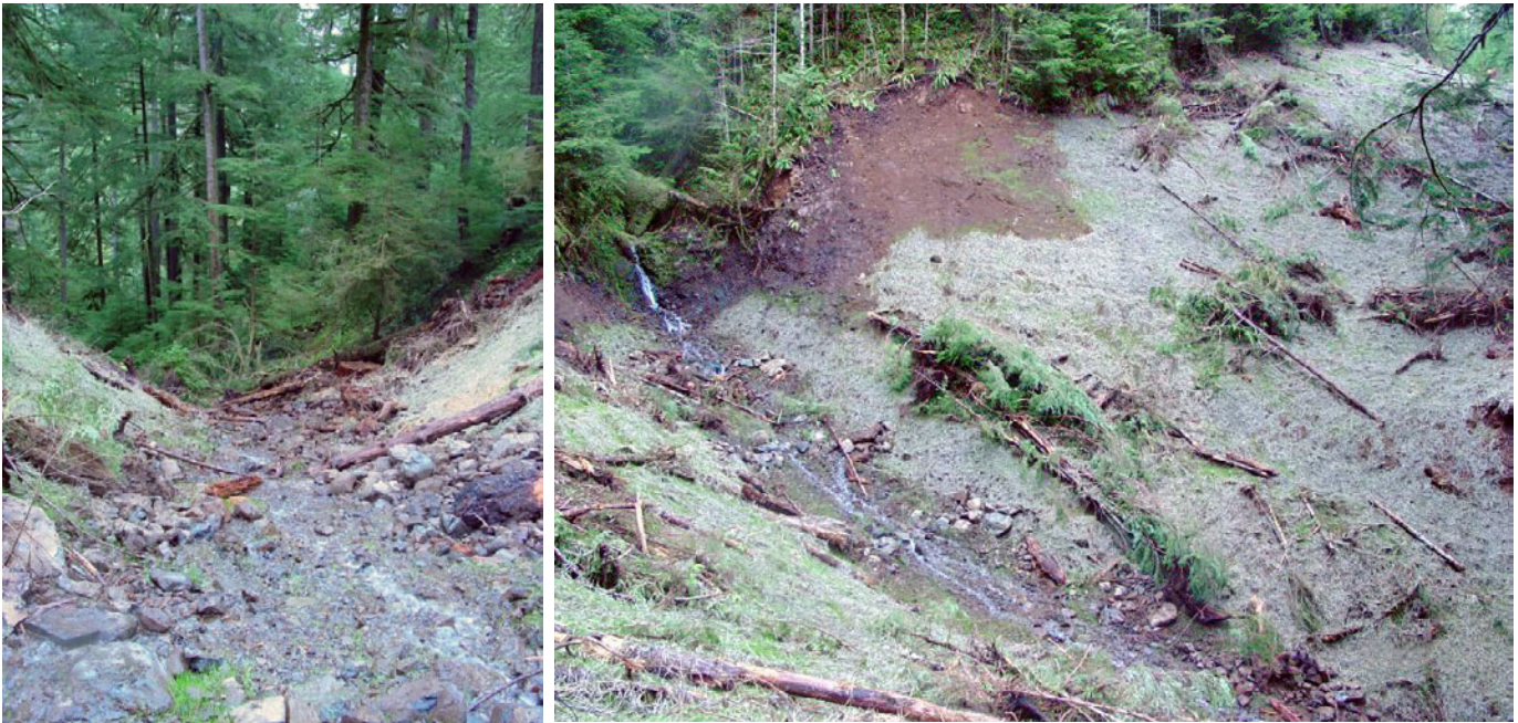
Photo N. Two views of an excavated stream crossing. Notice the straw and logs on the side slopes.
