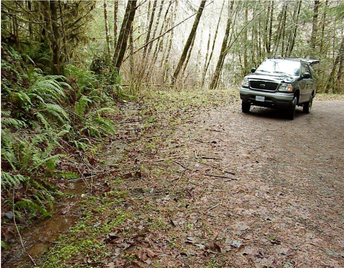
Photo P. Lead off ditch discharging to hillslope.
