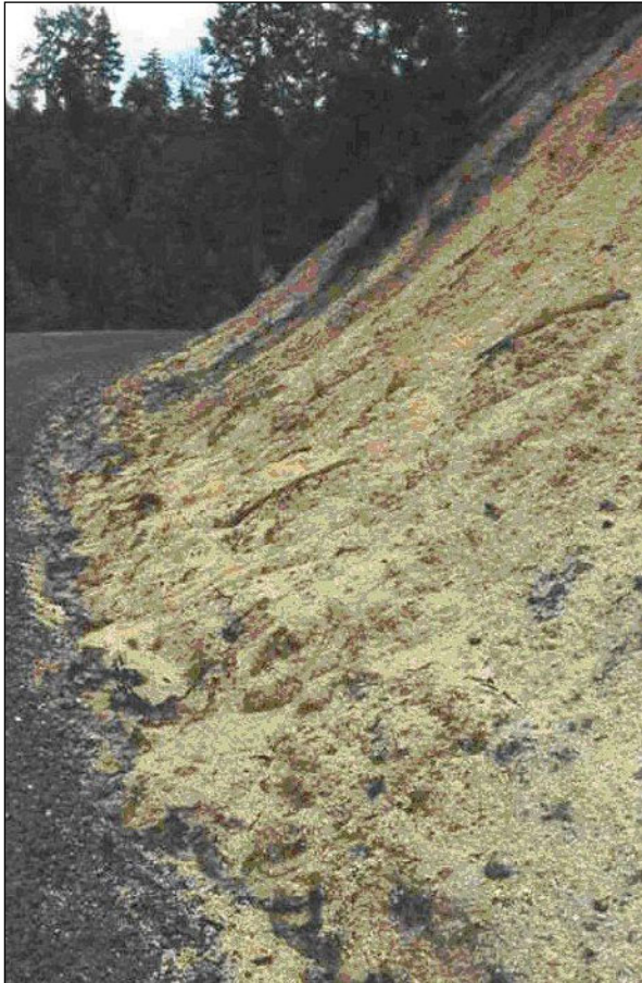
Photo F. A severely raveling cutslope in granitic saprolite. The ditch has been obscured by the accumulated apron of debris
