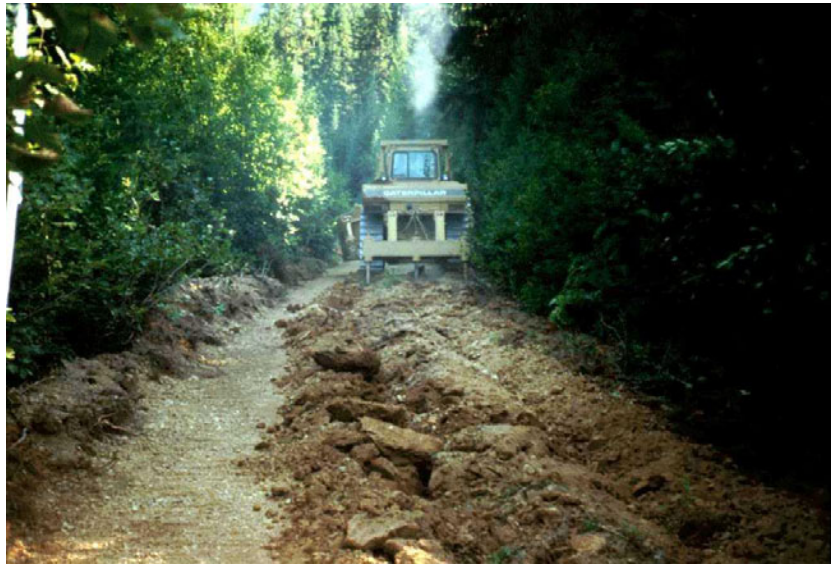
Photo A. Ripped road.
