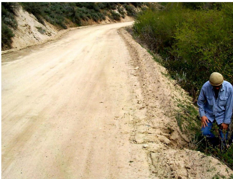
Photo Q. A non-engineered drainage at a broken berm. Water flowing along an outside berm is diverted over the fillslope. The fill erosion in this case would meet the 5 cubic foot minimum.
