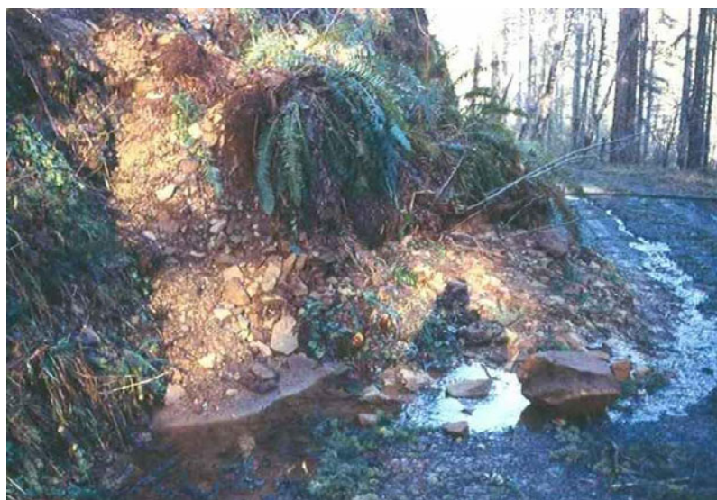
Photo DD. This road related landslide resulted from an over steepened cutslope that failed during an intense rainfall event.
