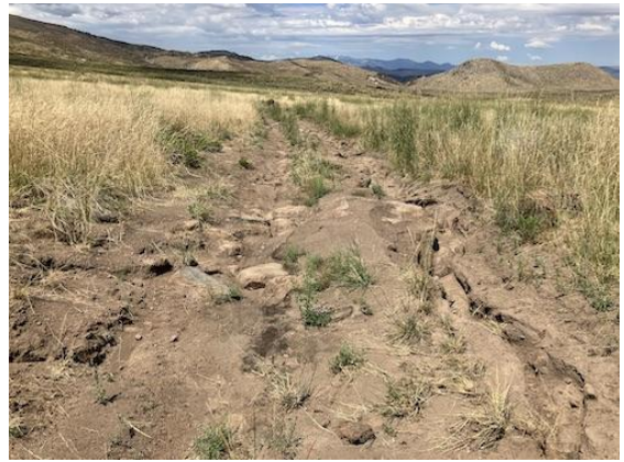
The road was then washed out.
