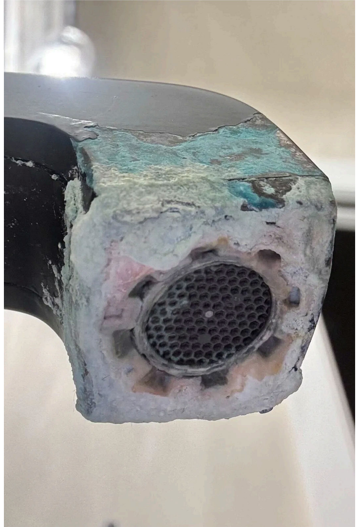
The Boarmans' water corroded their faucet. Courtesy of Tammy Boarman
