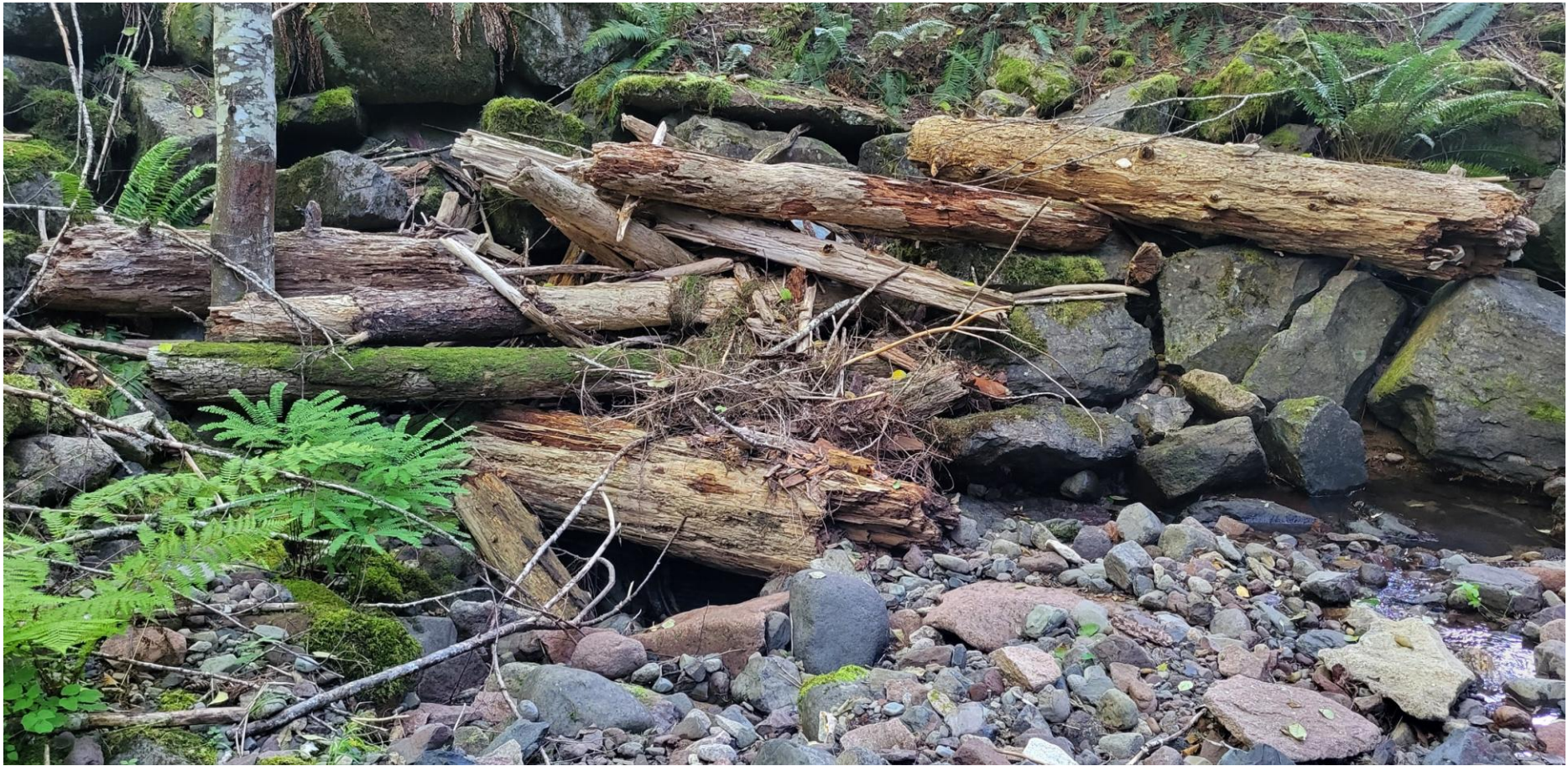
Culvert inlet where the 93 road crosses Platinum Creek. I removed some of the woody debris after taking this photo but the culvert is clearly not adequate for the location.
