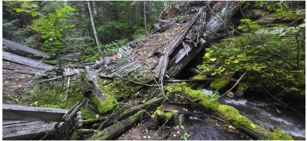
Collapsed bridge in Twin Falls Creek
