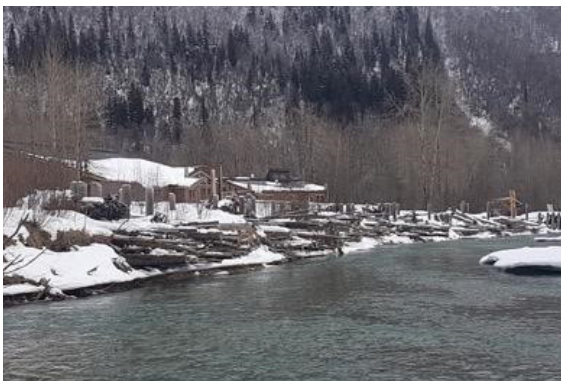
The Jilkáat main channel runs back along the riverbank immediately downstream of Tlákw Aan, in front of the Jilkaat Kwaan Cultural Heritage Center. Engineered log jams are visibly installed along the riverbank. Photo: Feb 2020.
