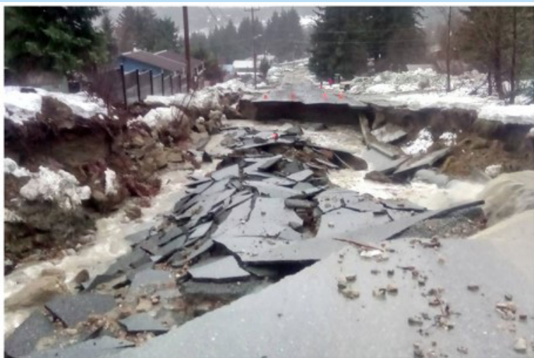
Many roads have been heavily damaged in Haines after heavy rain and flooding. Dec 2, 2020. (Photo provided by Darwin Feakes)
