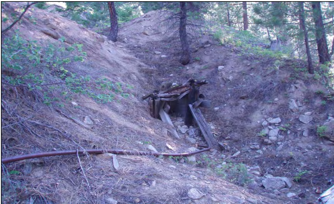
Photo No. 7: View of collapsed workings with hydraulic piping in middle portion of hillside (looking east). Possibly correlates to Blackbird No. 4 adit in historical records.
