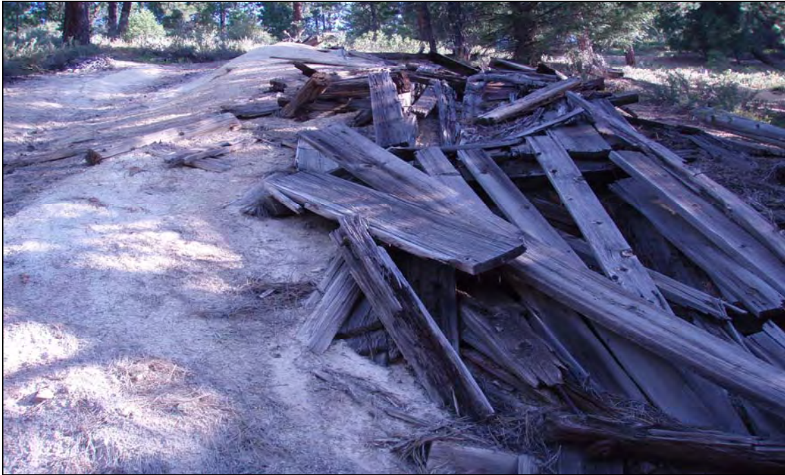
Photo No. 8: View of collapsed portal and waste dump located above the road on the western portion of the site (looking up to the north).
