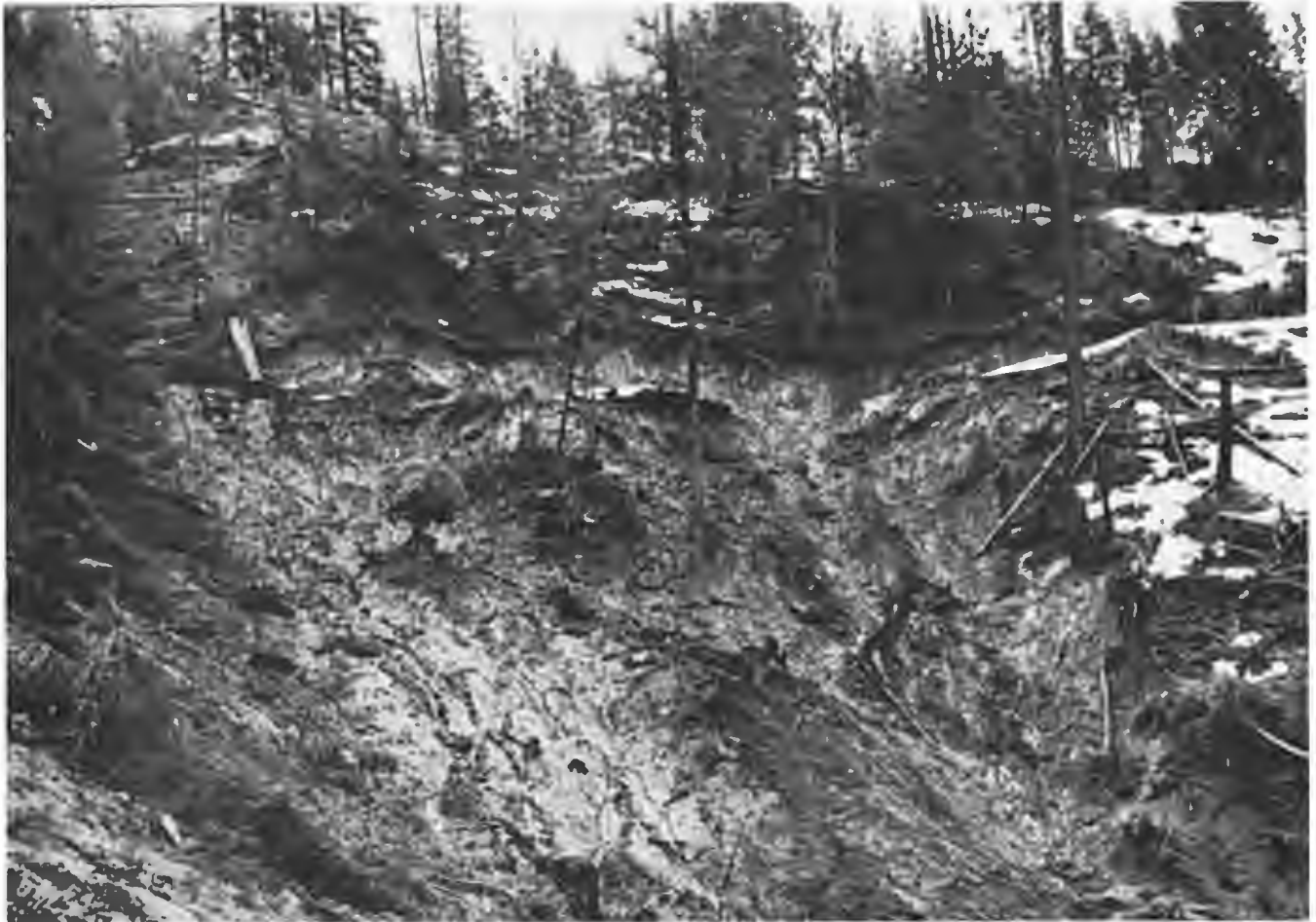
Fig. 4. Mass erosion on a jammer road in the Deep Creek study area due to poor road location and construction practices.
