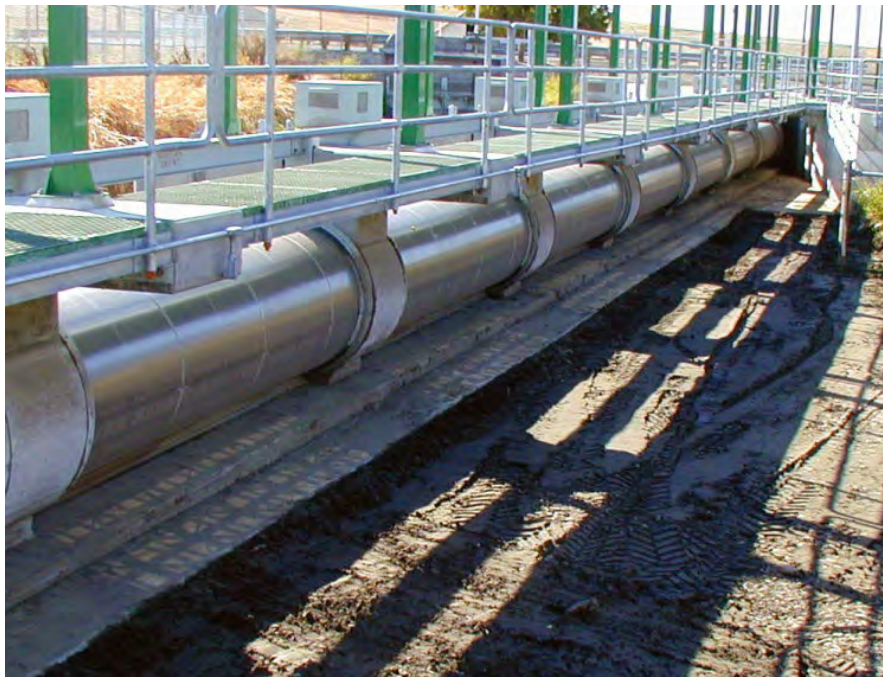
Figure 8-8 Medium-sized rotary drum screen at the Burlingame Diversion located on the Walla Walla River near Walla Walla, Washington
