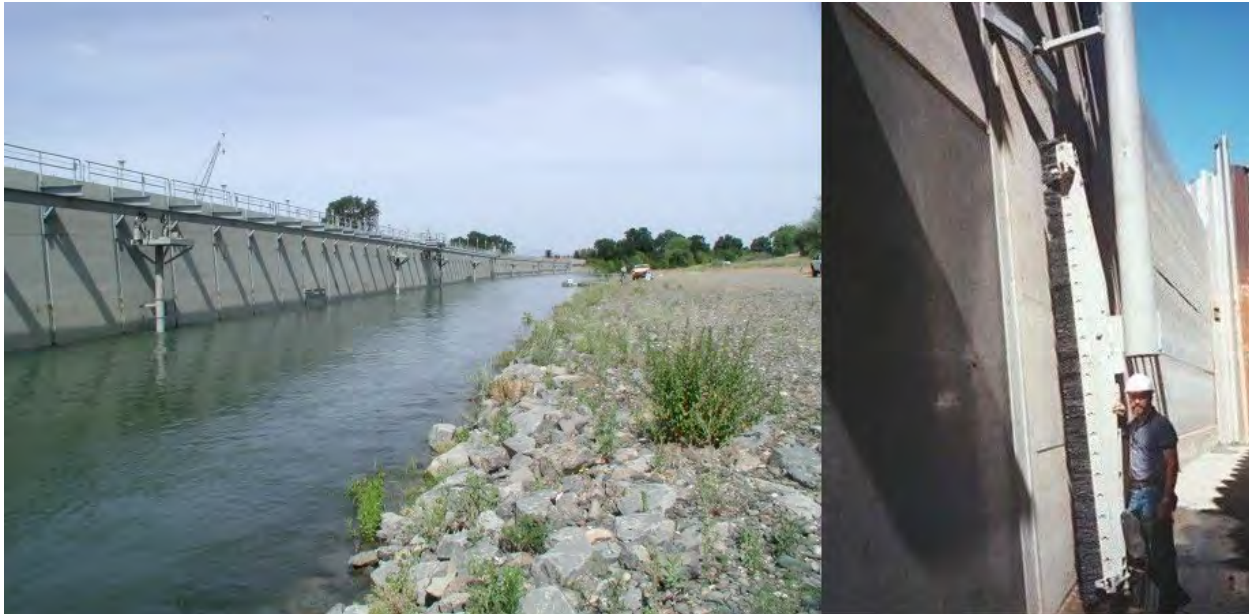
Figure 8-3 Bankline vertical flat plate fish screen sized for 3,000 ft 3 /s (Glenn-Colusa Irrigation District) along the Sacramento River in California (Note: the screen is shown in operation (left) and during construction (right).)
