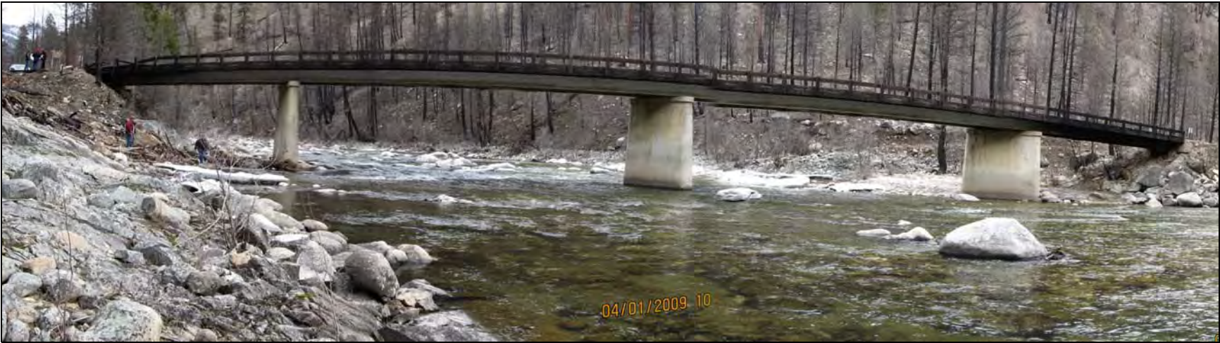
Figure 1. —Composite picture of entire span from the west side (left) to the east (picture was stitched from four separate images, the discontinuity in the center is from improper image alignment).
