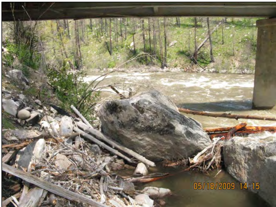
Figure 16. —Large rocks on the McCall side of the bridge to be left in place.
