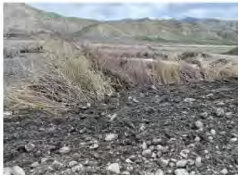
STAGE 3: TRENCH BACKFILLED WITH NATIVE ALLUVIUM AND ORGANIC TOP LAYER BEING PLACED.
