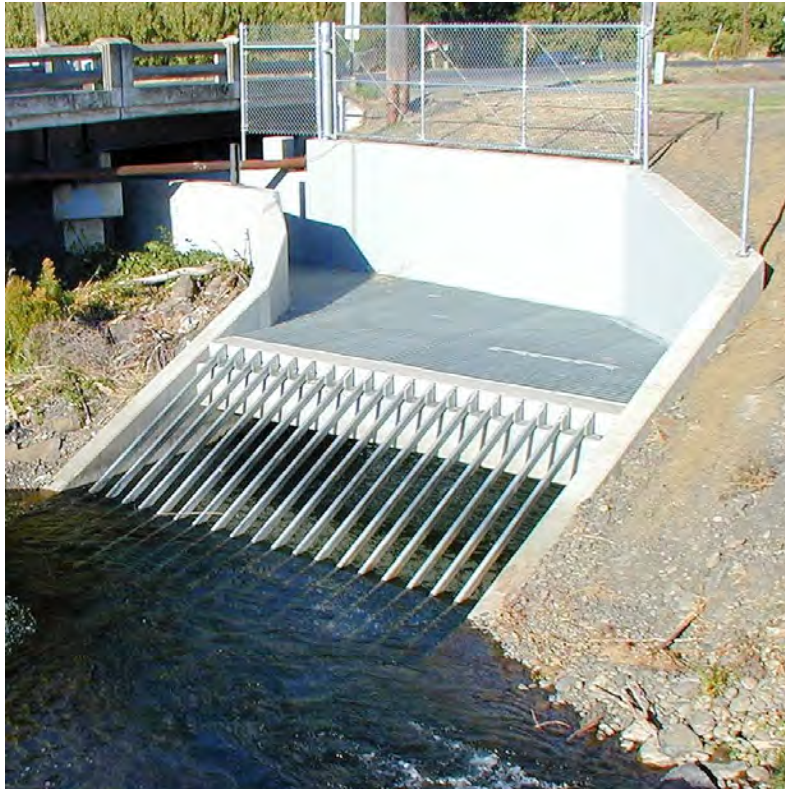
Figure 5-11. Sloping coarse trash rack on a fishway exit channel
