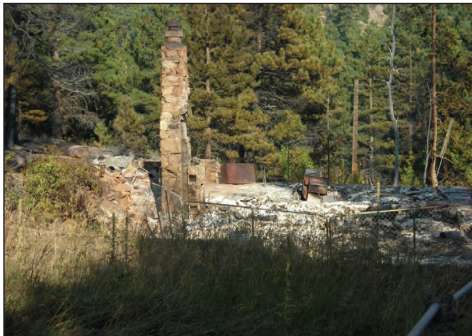
Figure 53. An example of total home destruction surrounded by unconsumed vegetation indicates the ignition was associated with a low intensity fire exposure (photo: Boulder County Sherriff Office).
