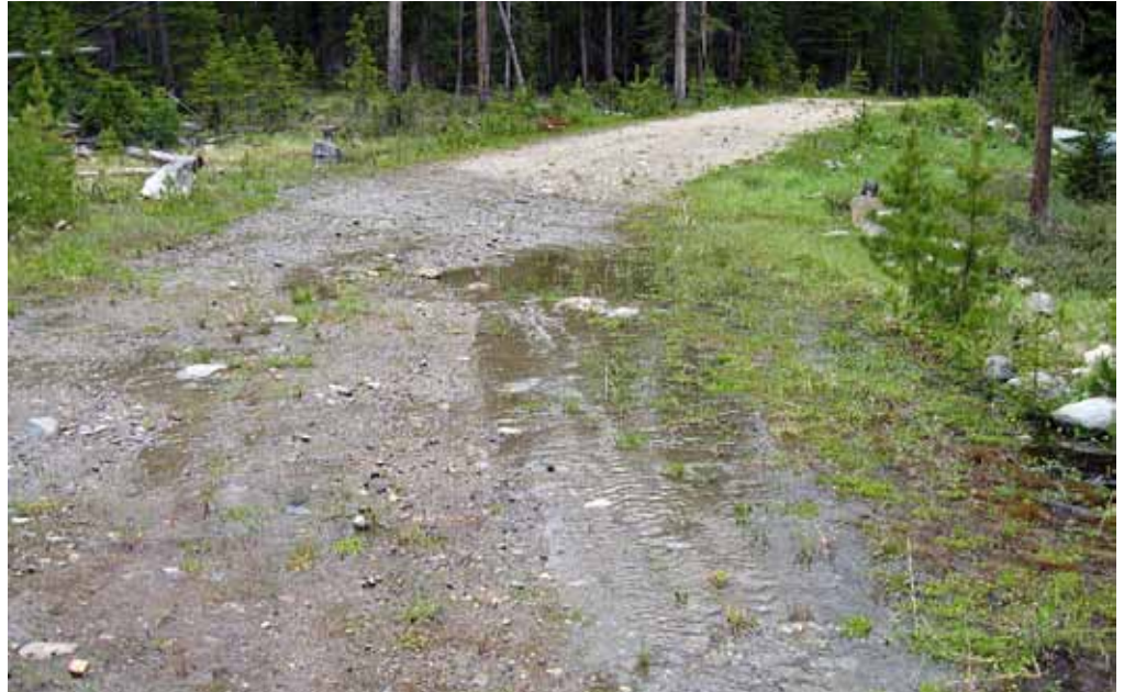
A non-functional culvert diverts water away from the creek and down a road. Photo by Adam Switalski.
