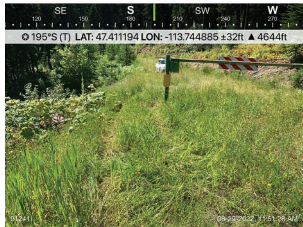
Fig. 19: Gate driven around by ATV on road 91241.
