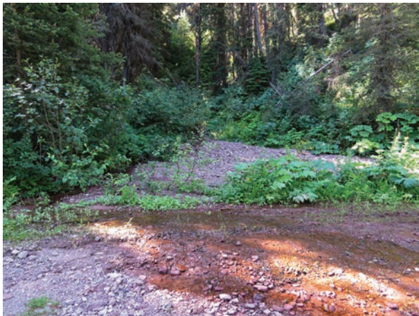
Road 1673 looking upstream at plugged catchment.
