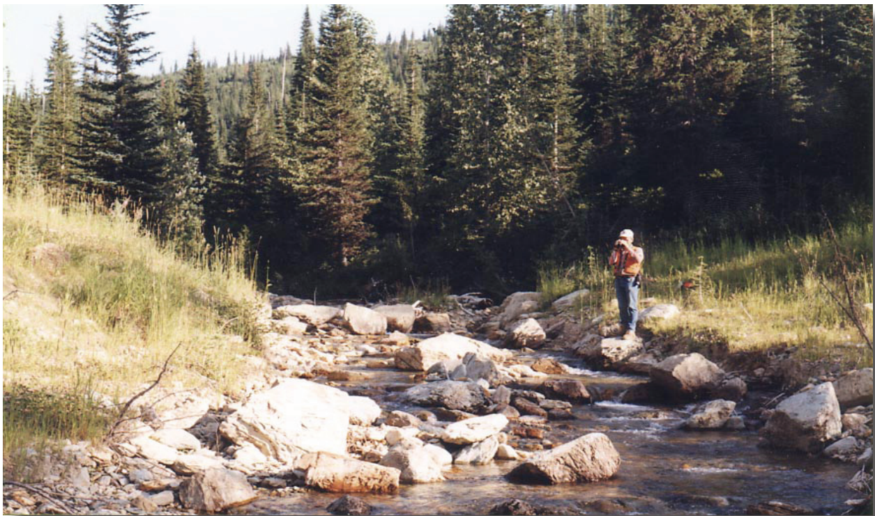
Reclamation of 60 miles of road in the Big Creek watershed removed culverts and restored native stream channels, like this reclaimed crossing. This resulted in Big Creek being the first watershed in Montana restored and removed from its list of watersheds "impaired" by logging and road-building. (Forest Service photo)
