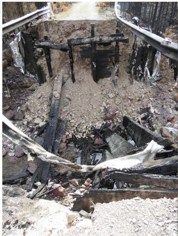
Wildfire burned this Road 549 bridge over Bunker Creek in 2015, stranding 3 bridges and 30 culverts beyond!
