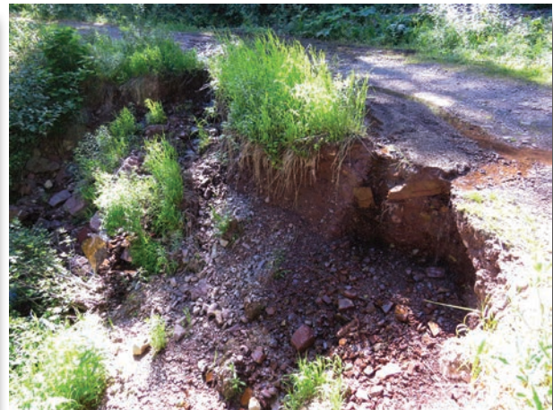
Road 1673 looking downstream at road-fill erosion.
