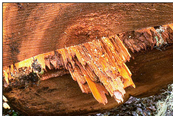
Figure 7 —Laminate decay in western redcedar caused by Obba rivulosa .
