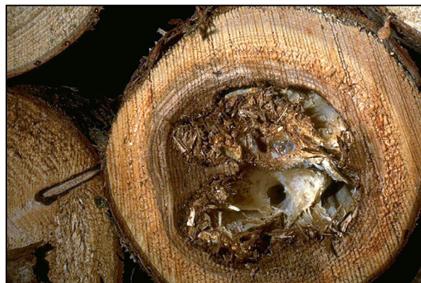
Figure 8 —Advanced decay in western redcedar caused by Perenniporia subacida .
