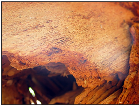
Figure 3 —Pitted and laminar decay of western redcedar wood caused by a white rot fungus.
