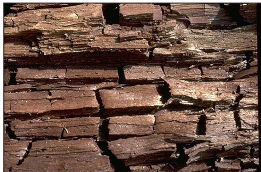
Figure 4 —Brown cubical decay of western redcedar wood caused by a brown rot fungus.
