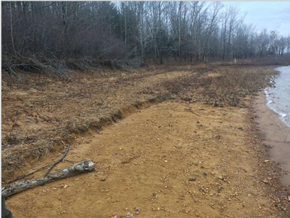
Figure 8: Photo of Monroe Lake Shoreline Erosion
