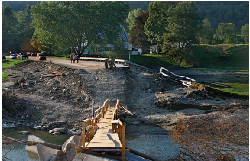
Top: Floodwaters caused by Tropical Storm Irene washed out this bridge in Brattleboro, Vermont.
