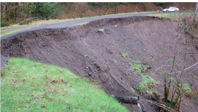
Bottom: A road blowout and landslide on the Olympic National Forest. The results include loss of public access, damage to fish habitat, and substantial water treatment facility costs to downstream communities.
