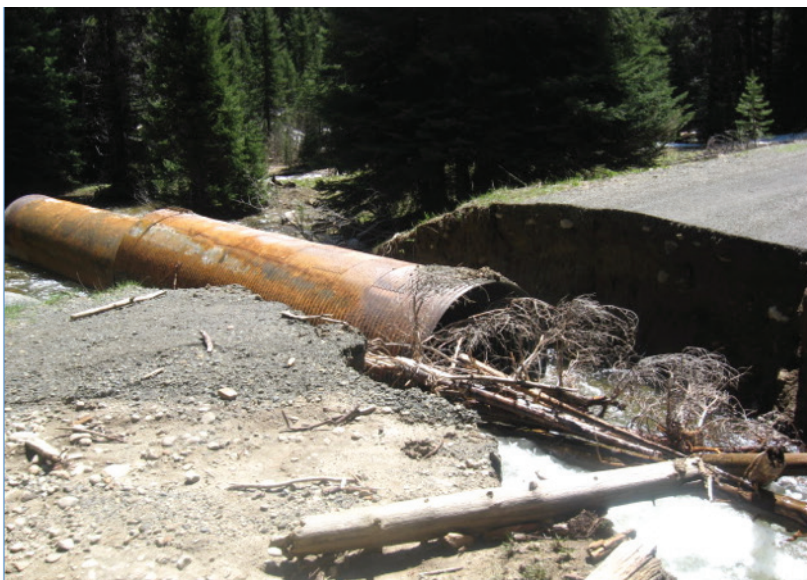
A road blowout at the Fawn Creek culvert on the Boise National Forest.
