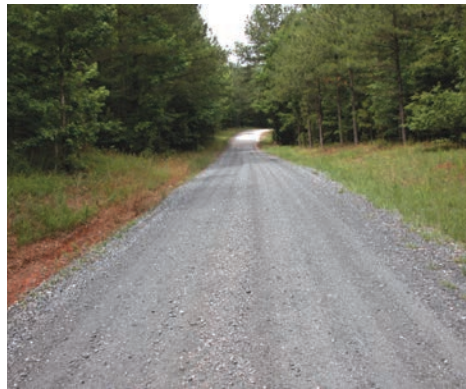
This is a Maintenance Level 4 road. ML3 and ML4 roads are often gravel roads designed for regular passenger vehicles, while ML5 refers to ordinary paved roads. 10
