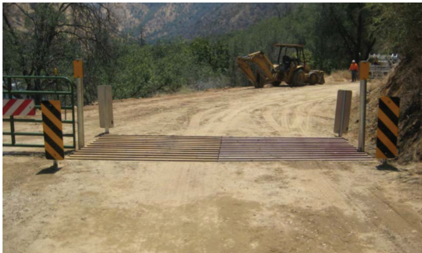
This Sequoia National Forest project made significant improvements to a nearly 11-mile stretch of deteriorated forest road.
