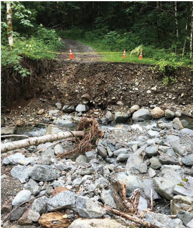
This road on the Mt. Baker-Snoqualmie National Forest blew out when a culvert plugged during a storm, eliminating access to popular trails.
