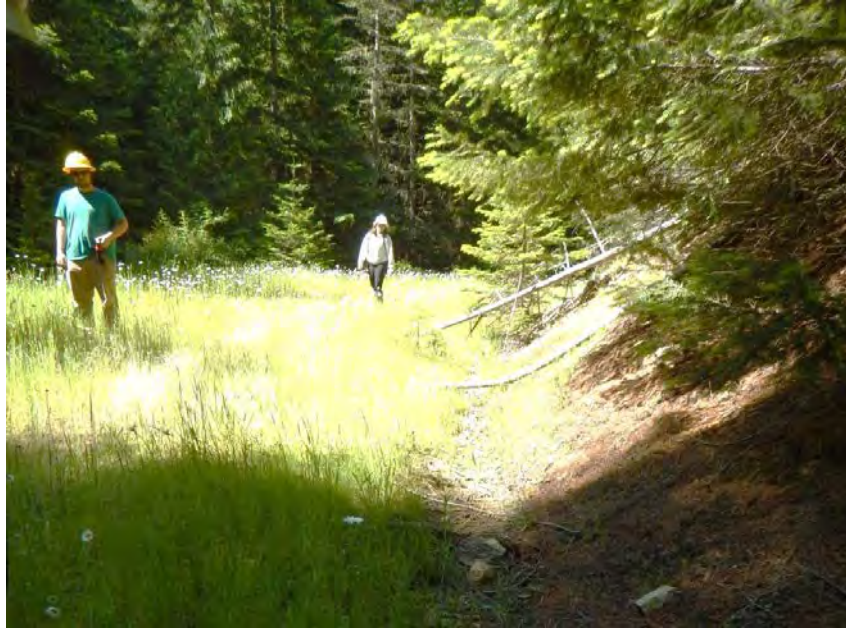
Figure 8. Typical vegetated cover on road north of site 1. Note some evidence of ditch erosion. Similar grass cover was observed at location 3 (Figure 7).
