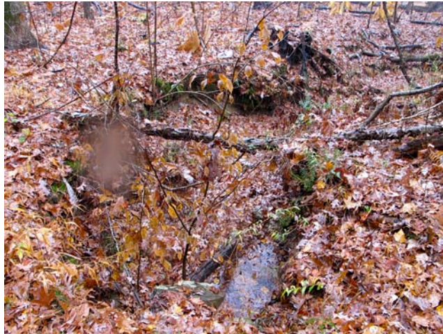
Scour, downstream of partially blocked culvert
