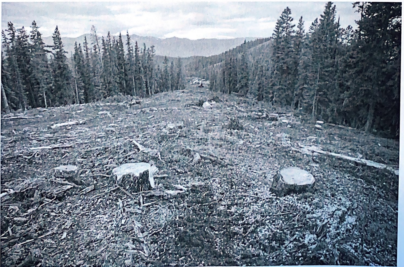
Construction crews have cleared trees at Keystone ski area as part of an expansion into the resort's Bergman Bowl, seen on July 28. (Hugh Carey, The Colorado Sun)
