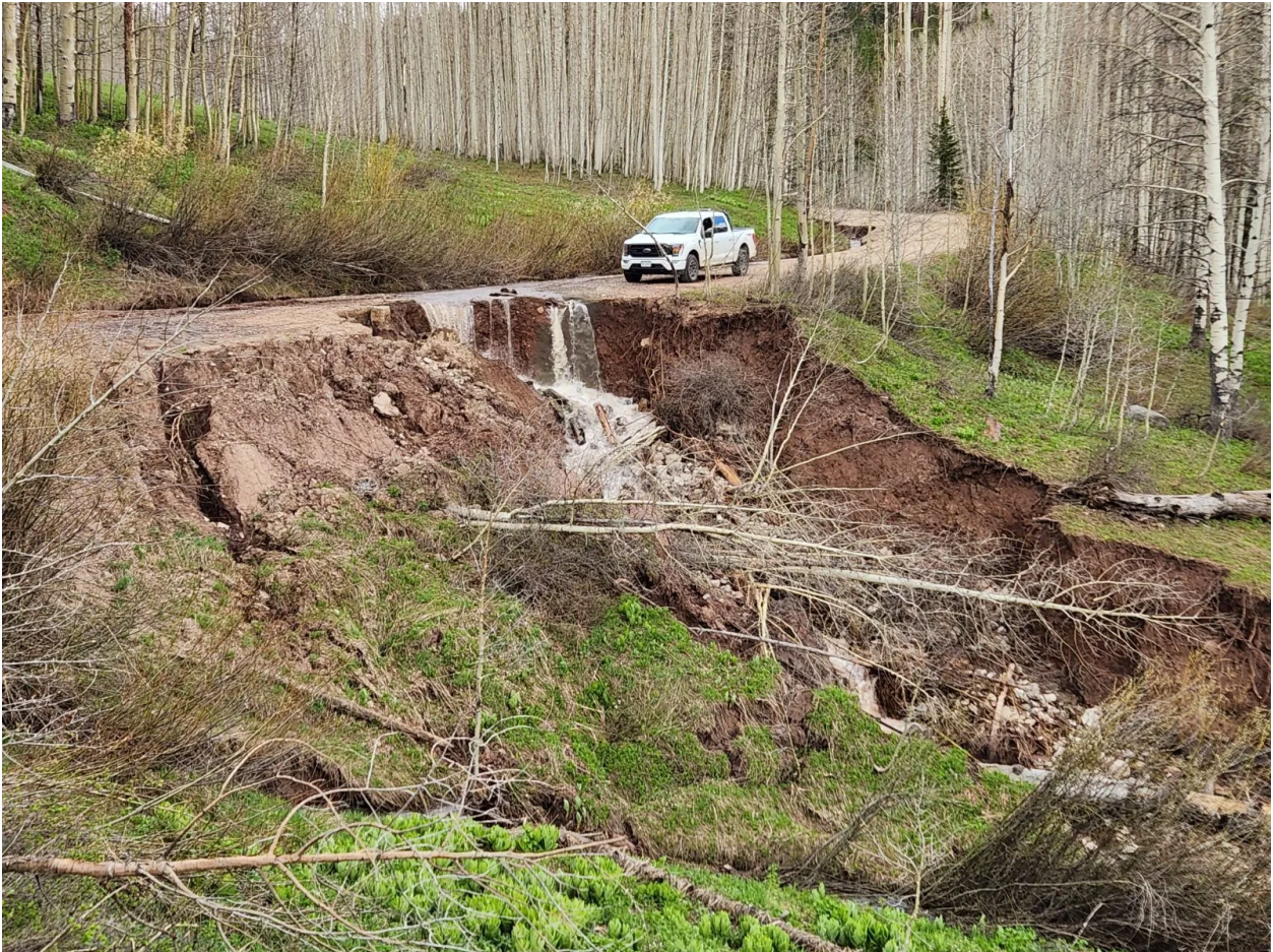
Photo courtesy of Gunnison County. Kebler Pass washout.
