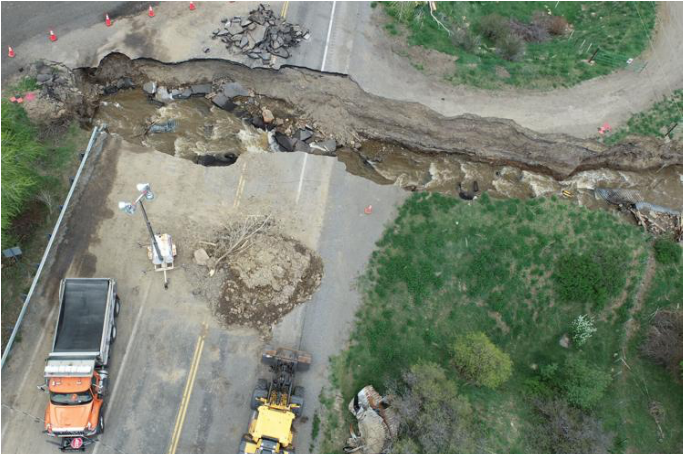
Photo courtesy of Colorado Department of Transportation. The photo above shows road damage on Colorado Highway 133. Photo taken Monday, May 15.
