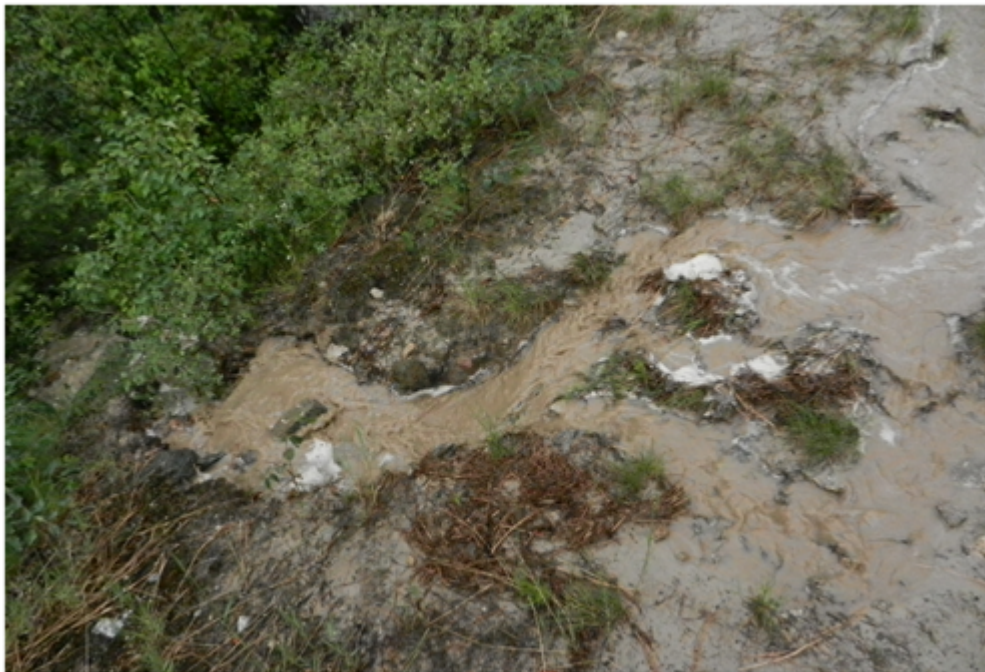
The second photo (above) shows this “stream” at the beginning of its flow off of the road at the location of the discharge of a small culvert (the culvert is not visible in the photo).
