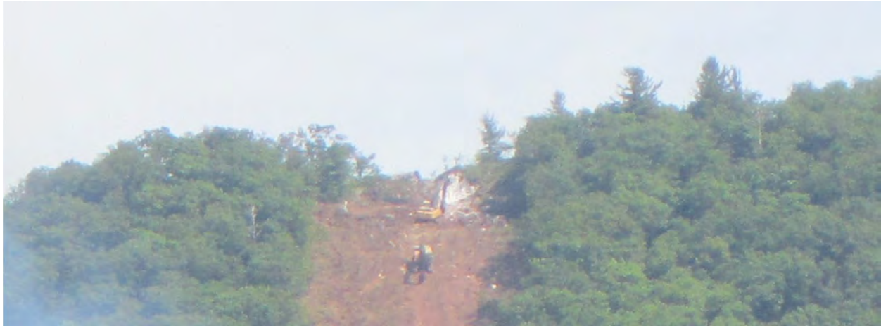
Figure 4. Photo of the pipeline corridor at the top of Sinking Creek Mountain, 16 June 2018. It appears that explosives have been used to fracture the rock formerly constituting the mountaintop. The photo was taken from a non-JNF location in Craig County but the JNF boundary runs across the top of Sinking Creek Mountain at the photo location. Hence, it is clear that surface geologic structure within the JNF has been affected similarly. 124
