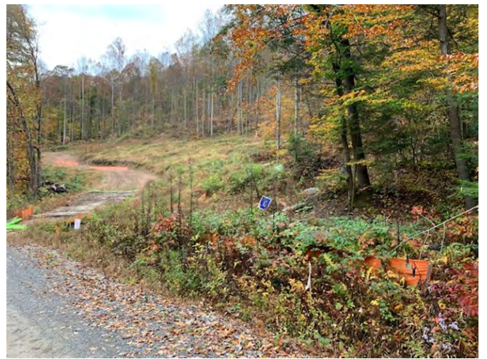
Spread C – The installed erosion control devices at County Route 7 (Elk River Road) were in good condition and have functioned well. The vegetation was in good condition and no signs of erosion were observed (December 31, 2020) – MP 87.6 – Acceptable
