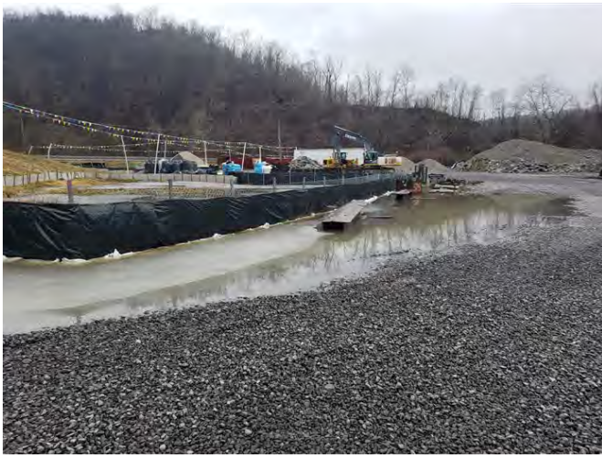
Laydown Yard – MVP-LY-001 – The sediment barriers at the sensitive resources have been properly maintained and were functioning as designed (January 1, 2021) – MP 0.0 – Acceptable
