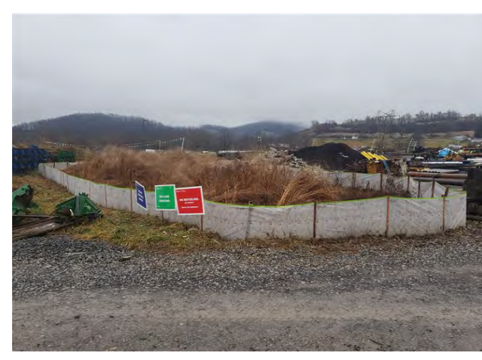
Laydown Yard – MVP-LY-051 – Resource signage was clearly visible and the sediment barriers have been properly maintained (January 2, 2021) – MP 0.0 – Acceptable
