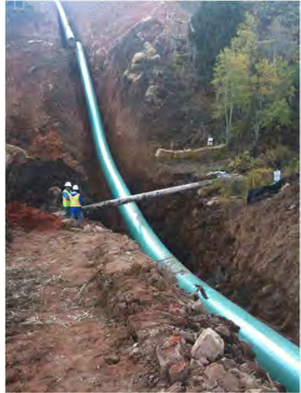
Figure 5. Typical flumed stream crossing. This figure is available in colour online at wileyonlinelibrary.com/journal/rra
