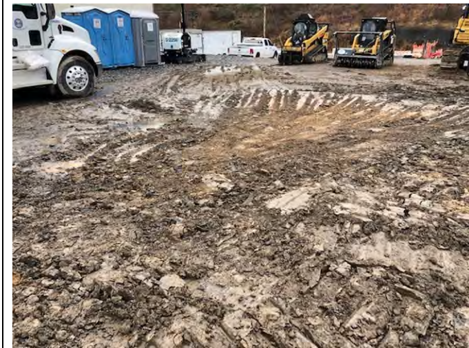
Laydown Yard – MVP-LY-068 – All of the spill was properly cleaned up, removed, and disposed (December 31, 2020) – MP 0.0 – Acceptable
