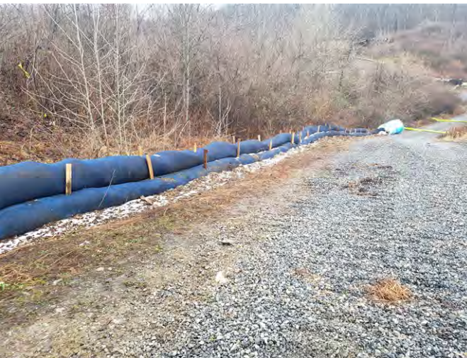
Laydown Yard – MVP-LY-002 – The sediment barriers have been properly maintained and were functioning as designed (January 2, 2021) – MP 0.0 – Acceptable
