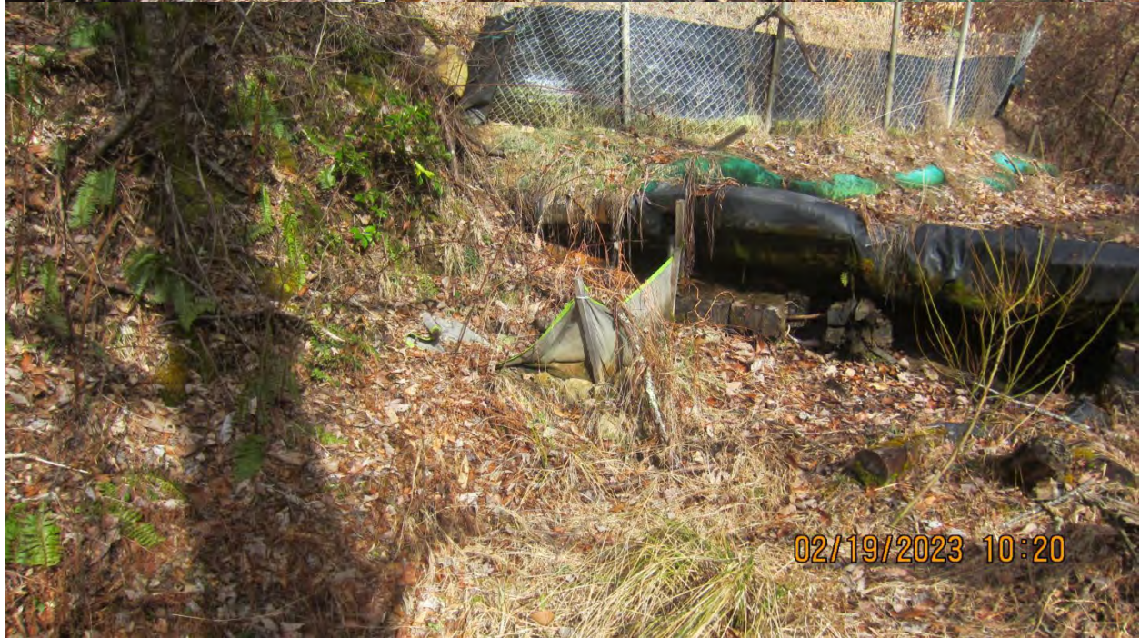
ABOVE: The silt fences at the base of the bridge is in disrepair.
