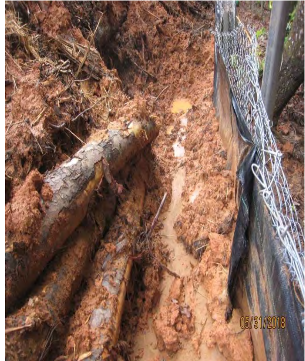
Sediment located on north side of SF
