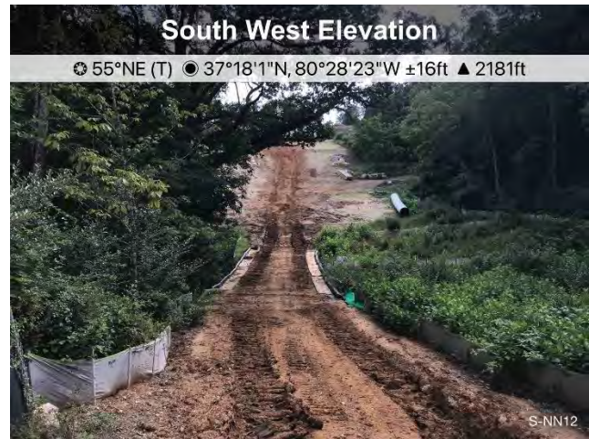
Figure 2: Designated crossing S-NN12
