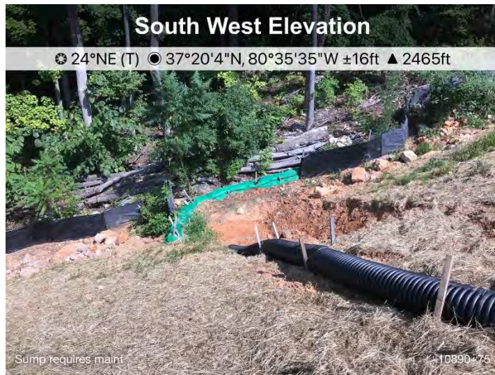
Figure 3: St 10890+75 sump requires maintenance
