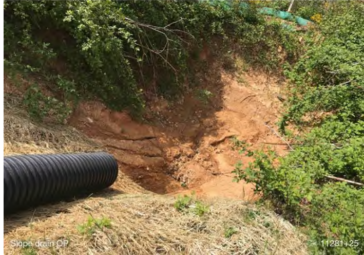
Figure 5: STA 11281+25 – Slope drain does not have outlet protection. BRG: 122°SE (T) LAT: 37.295792 LON: -80.485271 ±16ft ALT: 2273ft
