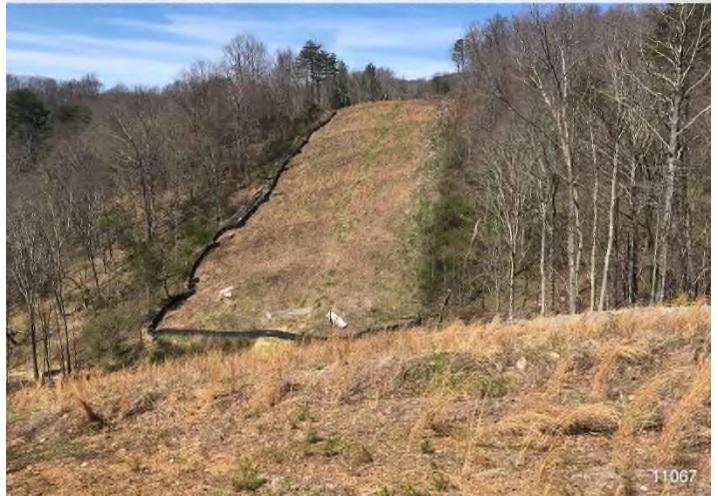
Figure 4: STA 11067+00 – Controls in place and functioning properly. BRG: 92°E (T) LAT: 37.306213 LON: -80.508641 ±13639ft ALT: 2168ft
