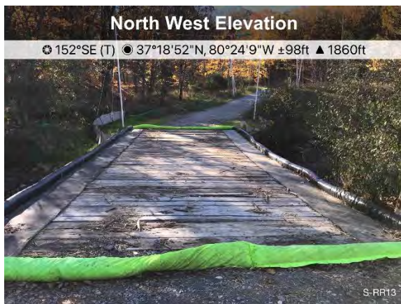
Figure 3: Designated crossing S-RR13, ECD's are in place.
