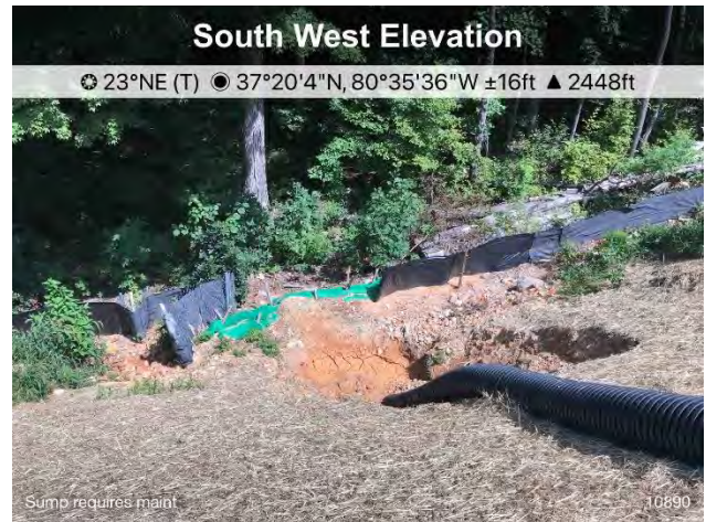
Figure 2: St 10890 sump requires maintenance
