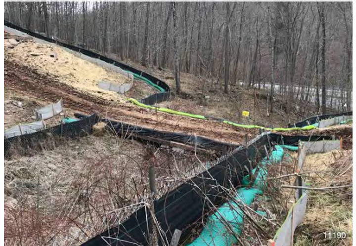
Figure 4: STA 11190+00 – Controls in place and functioning properly. BRG: 169°S (T) LAT: 37.306290 LON: -80.509893 ±32ft ALT: 1947ft
