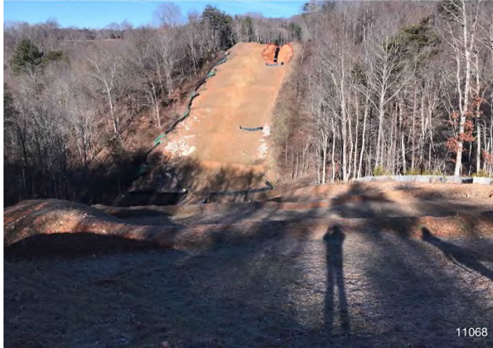
Figure 1: STA 11068+00 – Controls in place and functioning properly. BRG: 307°NW (T) LAT: 37.267910 LON: -80.471223 ±16535ft ALT: 2192ft
