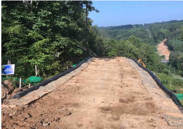
Figure 1: Stream S-Z14 – Controls in place and functioning properly. BRG: 281°W (T) LAT: 37.336314 LON: -80.677131 ±25695ft ALT: 2361ft
