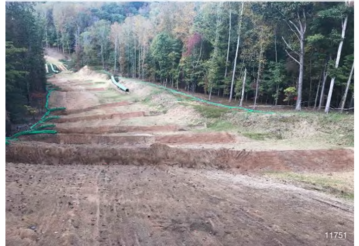
Figure 4: STA 11751+00 – Controls in place and functioning properly. Area stabilized with straw. BRG: 288°W (T) LAT: 37.288736 LON: -80.373423 ±16092ft ALT: 2037ft
