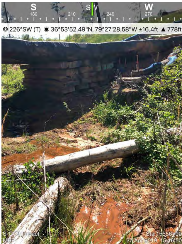
Figure 47 - Sediment deposited in UT to Cherrystone Creek, Action Item ID 2646, Source: MBP
