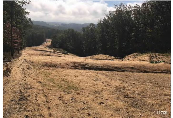
Figure 2: STA 11709+00 – Controls in place and functioning properly. Area stabilized with straw. BRG: 111°E (T) LAT: 37.296546 LON: -80.384996 ±32ft ALT: 2379ft
