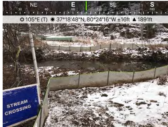
Figure 2: Designated crossing S-006 ECD's are in place.
