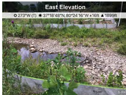
Figure 3: Designated crossing S-006, ECD's are in place.
