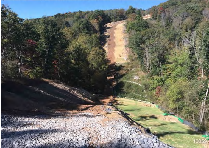
Figure 1: STA 10859+00 – Controls in place and functioning properly. Area stabilized outside of active travel lane. BRG: 291°W (T) LAT: 37.337672 LON: -80.604354 ±98ft ALT: 2288ft
