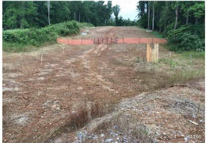
Figure 4: STA 11766+00 – Controls in place and functioning properly. BRG: 290°W (T) LAT: 37.296027 LON: -80.368025 ±16ft ALT: 1949ft
