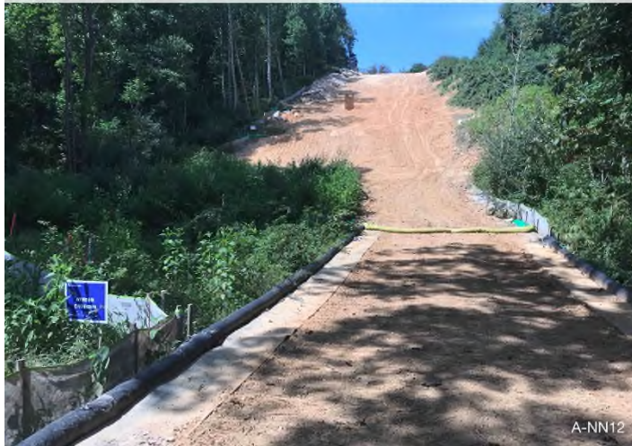
Figure 3: Stream S-NN12 – Controls in place and functioning properly along stream S-NN12. BRG: 237°SW (T) LAT: 37.300621 LON: -80.472870 ±98ft ALT: 2140ft
