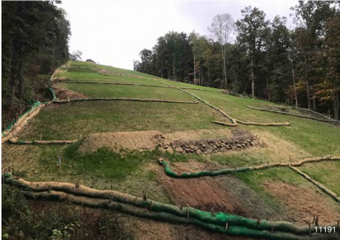
Figure 3: STA 11191+00 – Controls in place and functioning properly. BRG: 111°E (T) LAT: 37.306601 LON: -80.509923 ±98ft ALT: 1720ft
