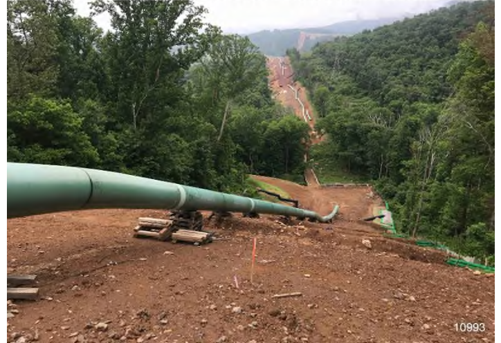
Figure 2: STA 10993+00 – Controls in place and functioning properly. BRG: 311°NW (T) LAT: 37.324776 LON: -80.562949 ±16ft ALT: 2587ft
