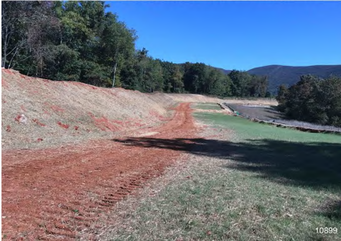
Figure 3: STA 10899+00 – Controls in place and functioning properly. Area stabilized outside of active travel lane. BRG: 11°N (T) LAT: 37.334599 LON: -80.592117 ±98ft ALT: 2540ft
