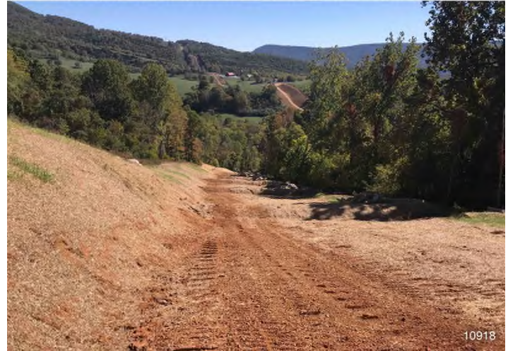
Figure 4: STA 10918+00 – Controls in place and functioning properly. Area stabilized outside of active travel lane. BRG: 131°SE (T) LAT: 37.332882 LON: -80.584734 ±213ft ALT: 2233ft
