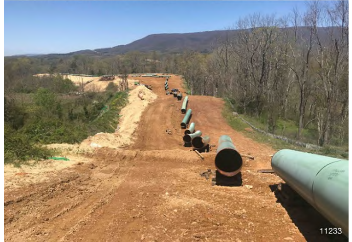
Figure 2: STA 11233+00 – Controls in place and functioning properly. BRG: 347°N (T) LAT: 37.303642 LON: -80.505547 ±13714ft ALT: 2126ft
