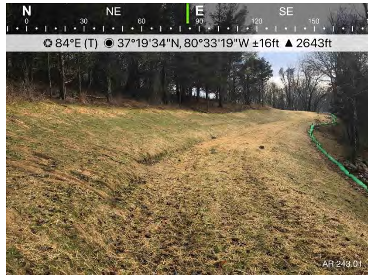
Figure 2: ESC controls were in place on AR 243.01
