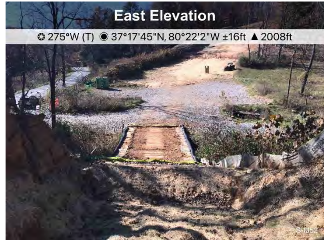
Figure 2: Designated crossing S-IJ52, ECD's are in place.
