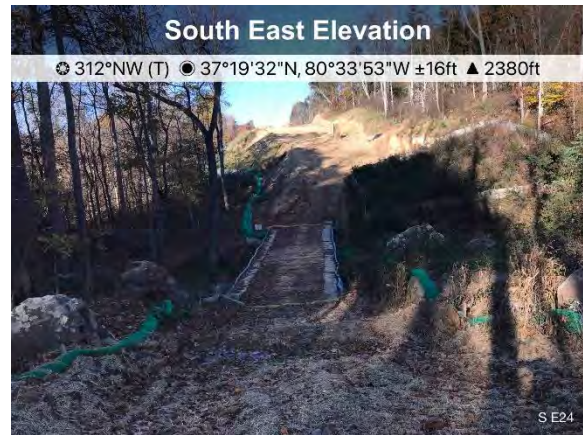
Figure 2: Designated crossing S-E24, ECD's are in place.
