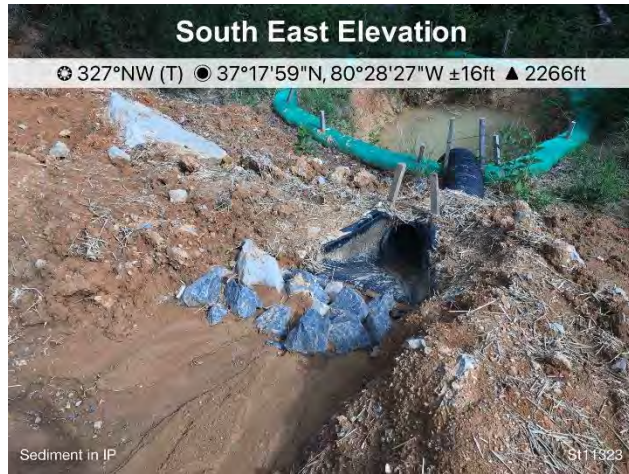
Figure 1: St11323 inlet protection requires sediment removal
