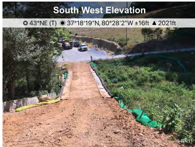
Figure 1: Designated crossing S-NN11
