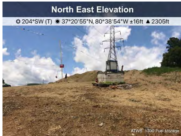
Figure 7: Fuel protected at ATWS 1390
