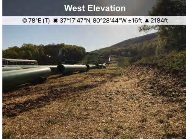
Figure 1: Near St11301+00 pipe is strung and welding crews on site, ECD's are in place.
