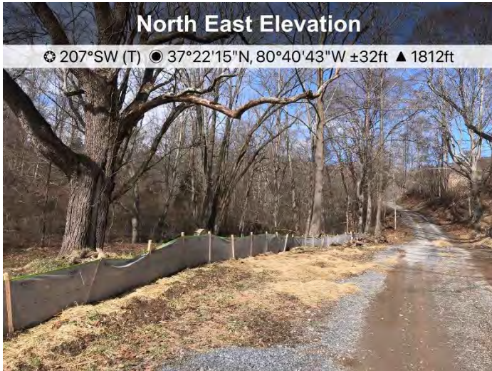
Figure 1: ECD's remain installed on AR-GI 234
