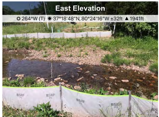
Figure 4: Designated crossing S-006, ECD's are in place.
