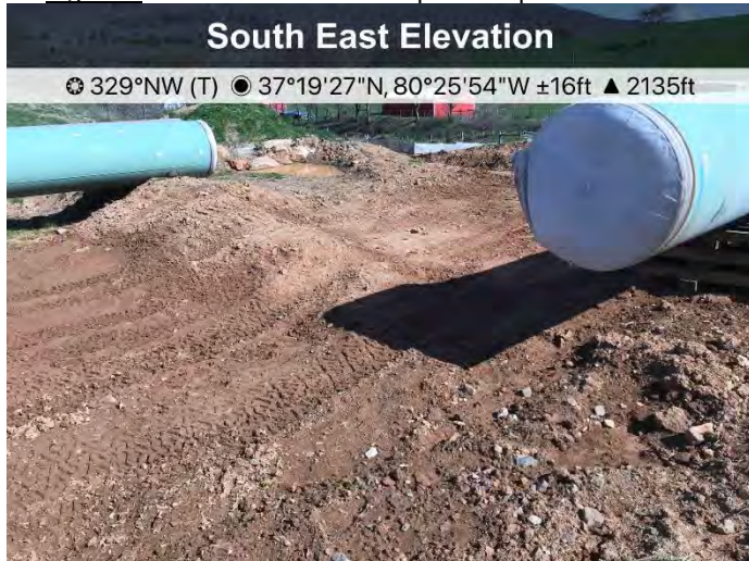
Figure 3: Waterbar not installed per the spec at St11488+00
