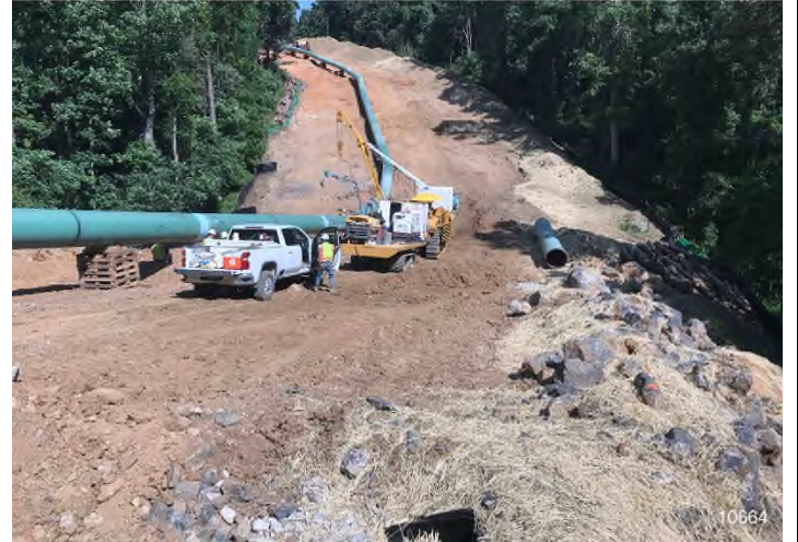
Figure 2: STA 10664+00 – Controls in place and functioning properly. BRG: 307°NW (T) LAT: 37.352778 LON: -80.661354 ±16ft ALT: 2203ft
