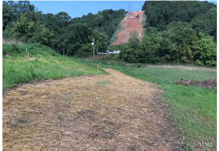
Figure 4: STA 11163+00 – Controls in place and functioning properly. BRG: 288°W (T) LAT: 37.311321 LON: -80.514494 ±16ft ALT: 1829ft
