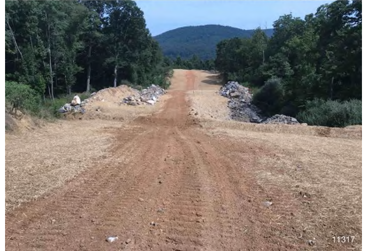
Figure 2: STA 11317+00 – Controls in place and functioning properly. BRG: 37°NE (T) LAT: 37.295694 LON: -80.476087 ±7237ft ALT: 2312ft
