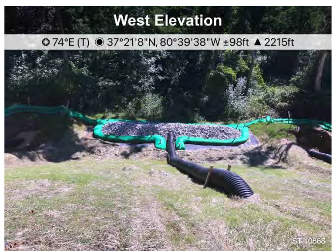
Figure 8: ECD has been installed at St10669
