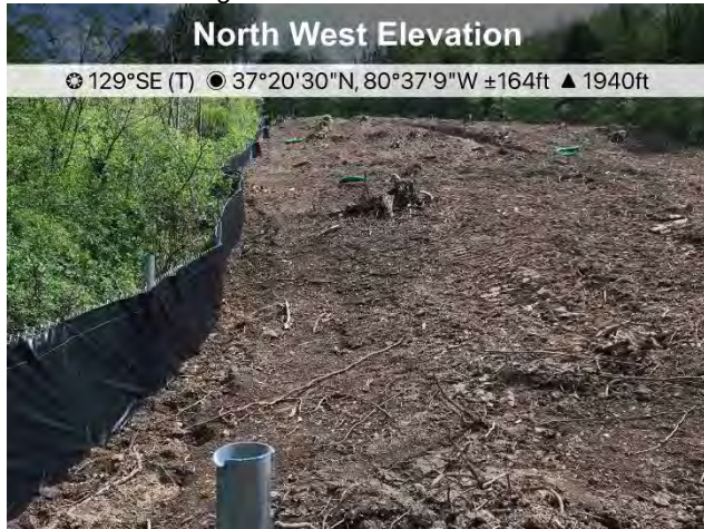
Figure 1: St10805+09 installation of waterbars uphill do not extend the full length of the ROW.
