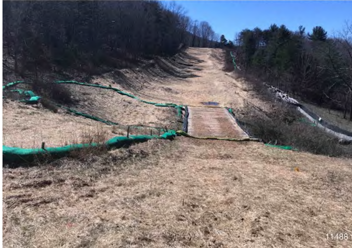
Figure 1: STA 11486+00 – Controls in place and functioning properly. BRG: 216°SW (T) LAT: 37.326721 LON: -80.426082 ±16420ft ALT: 2151ft
