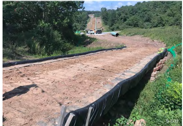
Figure 4: Stream S-G32 – Controls in place and functioning properly. BRG: 298°NW (T) LAT: 37.344473 LON: -80.663359 ±7417ft ALT: 2129ft
