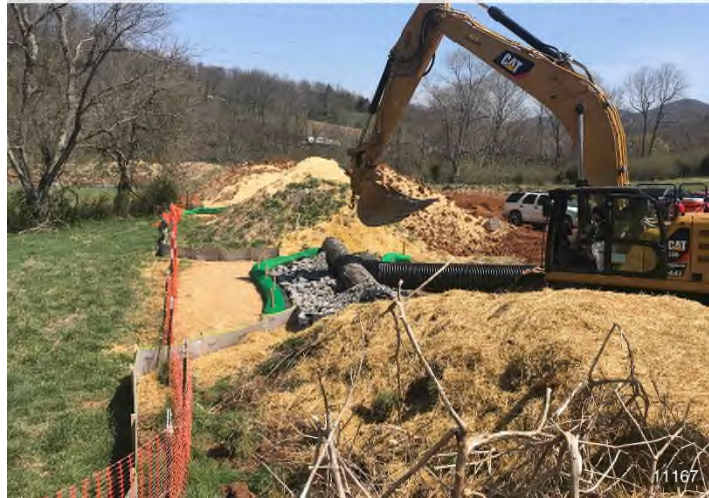
Figure 3: STA 11167+00 – PPL actively installing CWD and level spreader outlet. BRG: 48°NE (T) LAT: 37.310492 LON: -80.514443 ±16ft ALT: 1840ft
