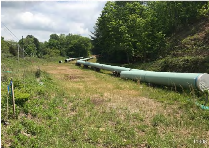
Figure 3: STA 11608+00 – Controls in place and functioning properly. BRG: 92°E (T) LAT: 37.313667 LON: -80.404540 ±32ft ALT: 1912ft
