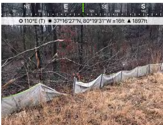
Figure 3: P1 is torn near St11960+00.
