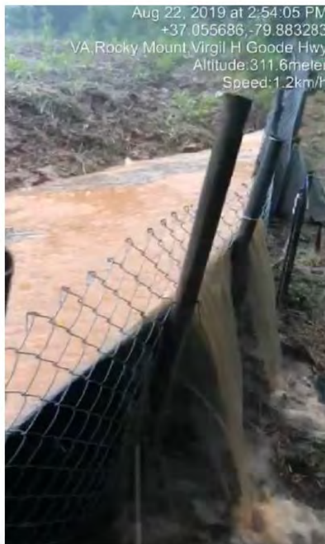
Figures 16 - 18 - August 22, 2019 Sediment-laden water flowing over, around, and through super silt fence and leaving the MVP ROW, several hundred feet upslope of the Blackwater River. Taken from a video accessible at Virginia Pipeline Violations Facebook page
