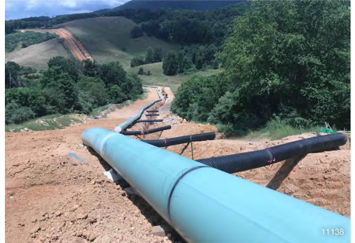
Figure 2: STA 11138+00 – Controls in place and functioning properly. BRG: 285°W (T) LAT: 37.312907 LON: -80.518180 ±15492ft ALT: 2143ft
