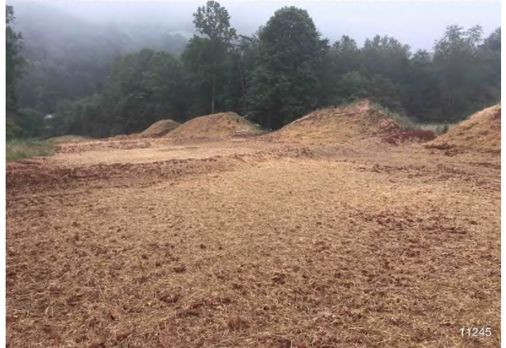
Figure 2: STA 11245+00 – Controls in place and functioning properly. BRG: 151°SE (T) LAT: 37.310473 LON: -80.506968 ±12326ft ALT: 2127ft
