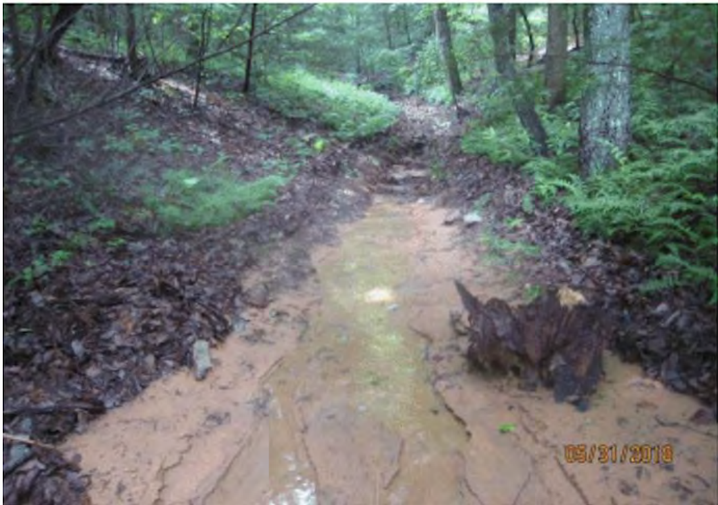
Figure 8 - Sediment deposited in UT Blackwater River, May 31, 2018, DEQ VWP inspection rpt. [sediment in streambed approx. 1,690 linear feet of stream impacted with deposits up to 5 inches deep; impacted area approx. 685 feet from ROW]
