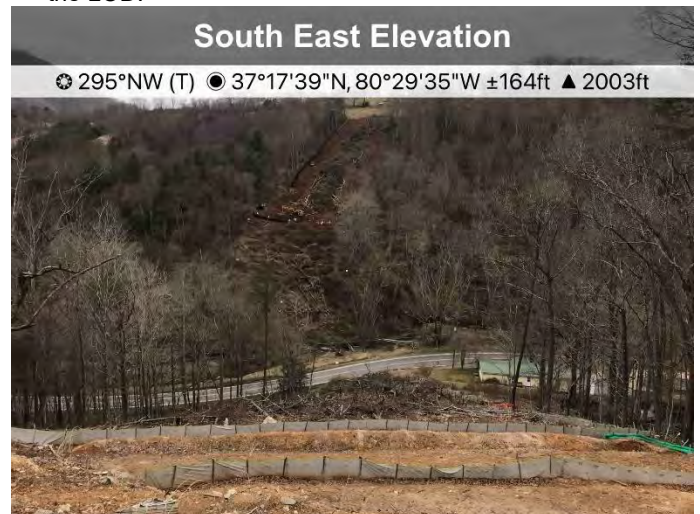
Figure 4: Near ST 11258+00 ECD's are in place at the end of the LOD.
