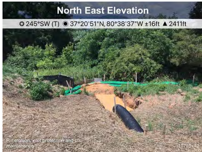
Figure 5: St 10725+42 CFS requires sediment removal
