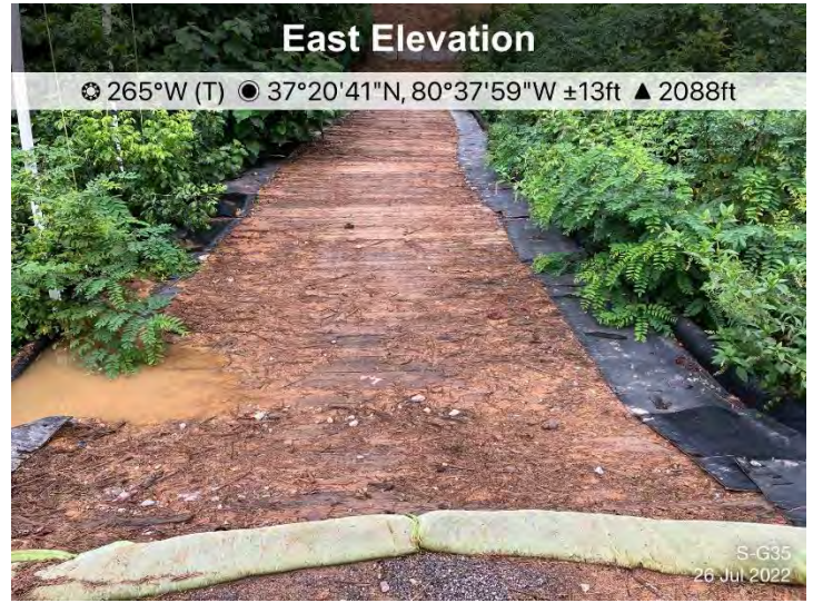
Figure 4: Designated crossing S-G35, ECD's are in place.
