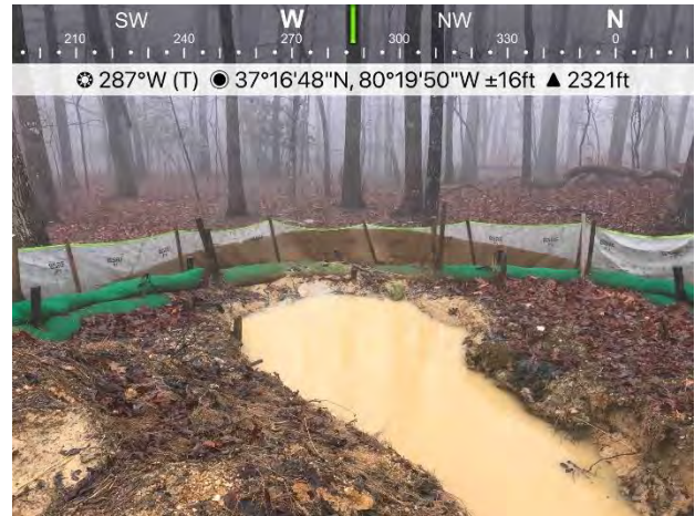
Figure 2: MVP inspectors have reported AR-MN266 sump maintenance.
