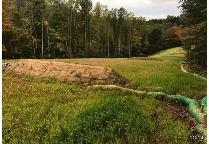
Figure 2: STA 11219+00 – Controls in place and functioning properly. BRG: 273°W (T) LAT: 37.301544 LON: -80.504047 ±16ft ALT: 2069ft
