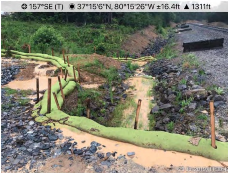
Figure 23 - Sediment-laden water undermining compost filters socks and discharging to a UT of Bradshaw Creek, July 23, 2019, DEQ Complaint inspection report, Source: DEQ
