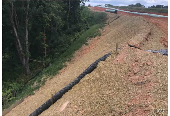
Figure 4: STA 11087+00 – Controls in place and functioning properly. BRG: 263°W (T) LAT: 37.315434 LON: -80.538351 ±16ft ALT: 2171ft
