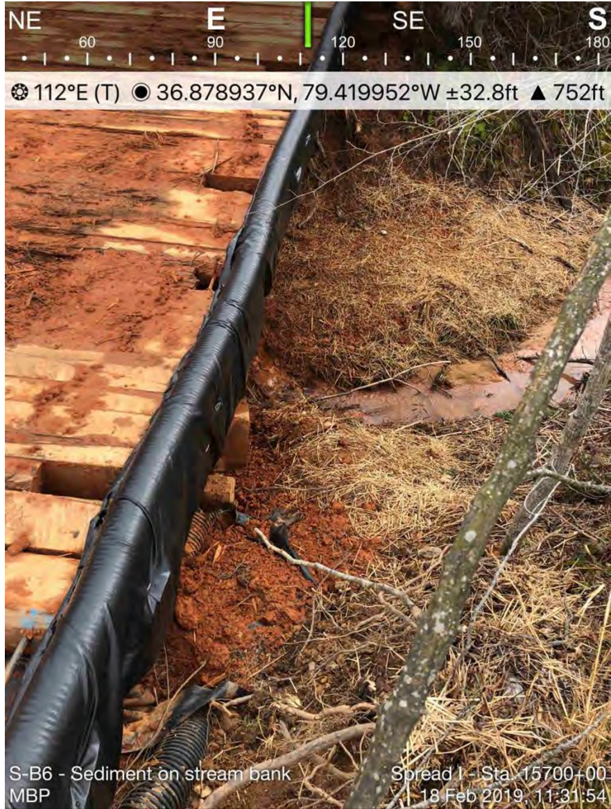
Figure 48 - Sediment deposited off ROW onto streambank at UT to Pole Bridge Branch, February 18, 2019, Action Log ID 1901, Source: MBP [deadline to remove extended "due to wet ROW," not removed until 6 days after deposited]
