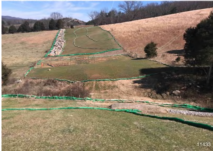
Figure 3: STA 11433+00 – Controls in place and functioning properly. BRG: 67°NE (T) LAT: 37.326364 LON: -80.448303 ±541ft ALT: 2093ft
