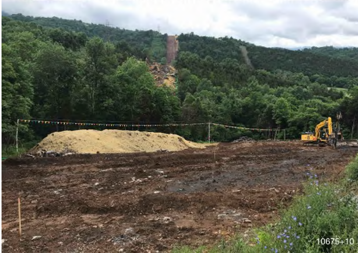
Figure 1: STA 10675+00 – Controls in place and functioning properly. BRG: 100°E (T) LAT: 37.350634 LON: -80.659512 ±16ft ALT: 2156ft
