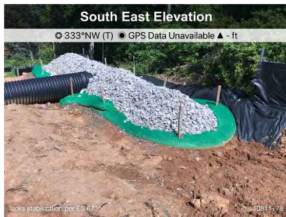
Figure 3: St10811+78 lacks stabilization per ES 67
