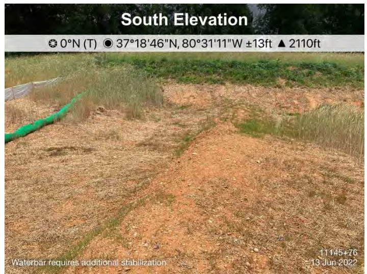
Figure 4: St 11145+67 denuded soil on waterbar requires stabilization.
