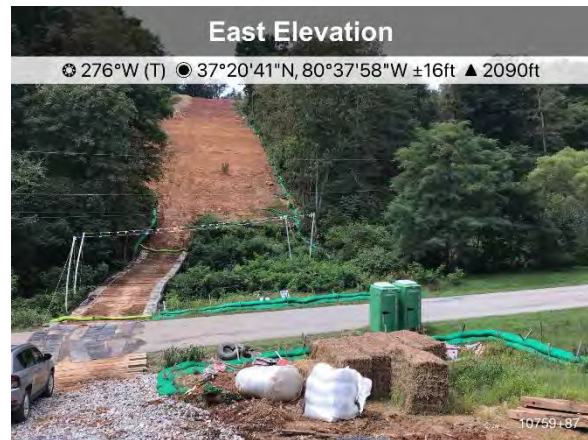
Figure 4: St 10759+87 above designated stream S-G35, ECD's are in place.
