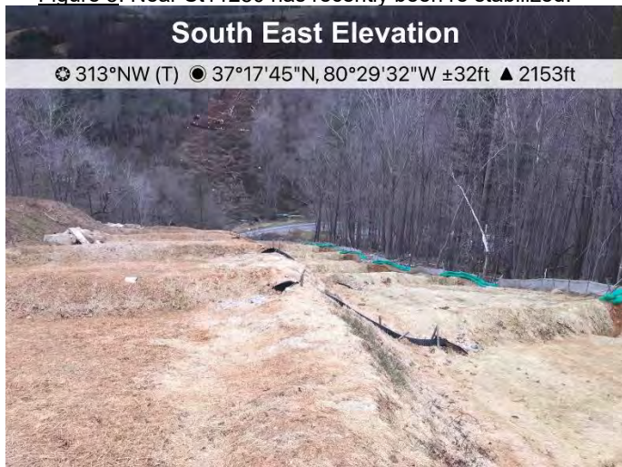
Figure 3: Near St11280 has recently been re stabilized.
