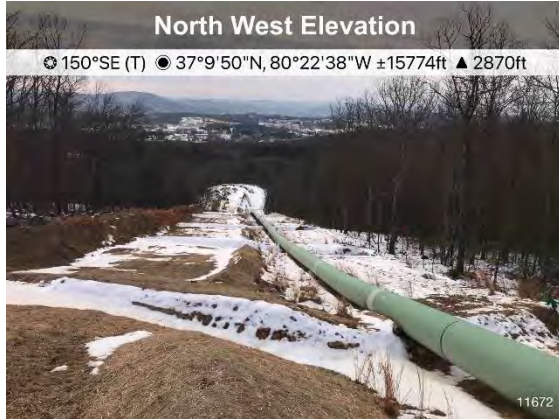
Figure 1: ESC controls were snow covered near St 11672
