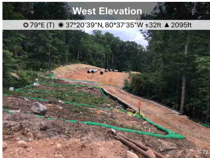
Figure 3: Designated crossing S-Z7, ECD's are in place.
