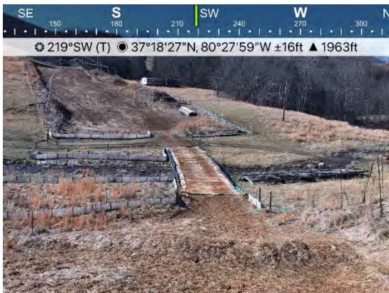
Figure 3: Designated stream S-KL43, ECD's are in place.
