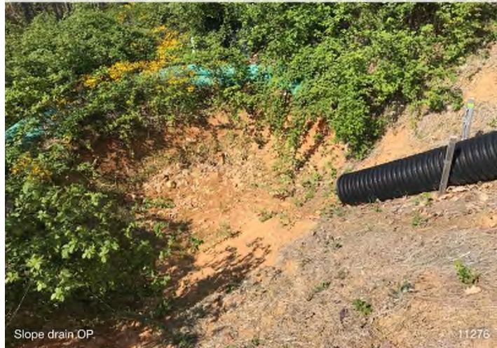
Figure 7: STA 11276+00 – Slope drain does not have outlet protection. BRG: 241°SW (T) LAT: 37.295868 LON: -80.487126 ±16ft ALT: 2281ft
