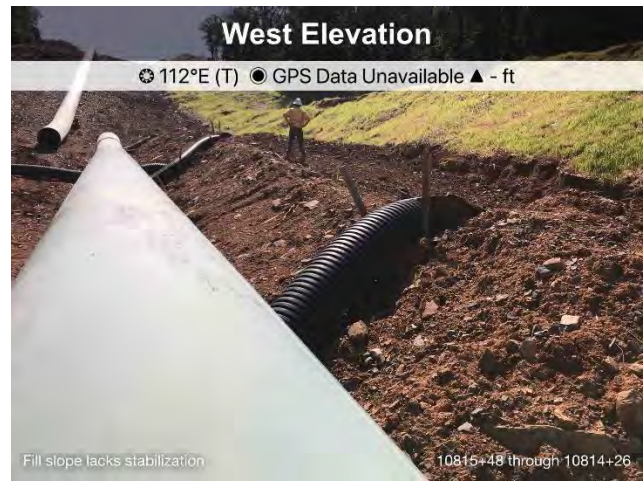
Figure 2: Two tone area lacks stabilization from 10815+45-10814+26
