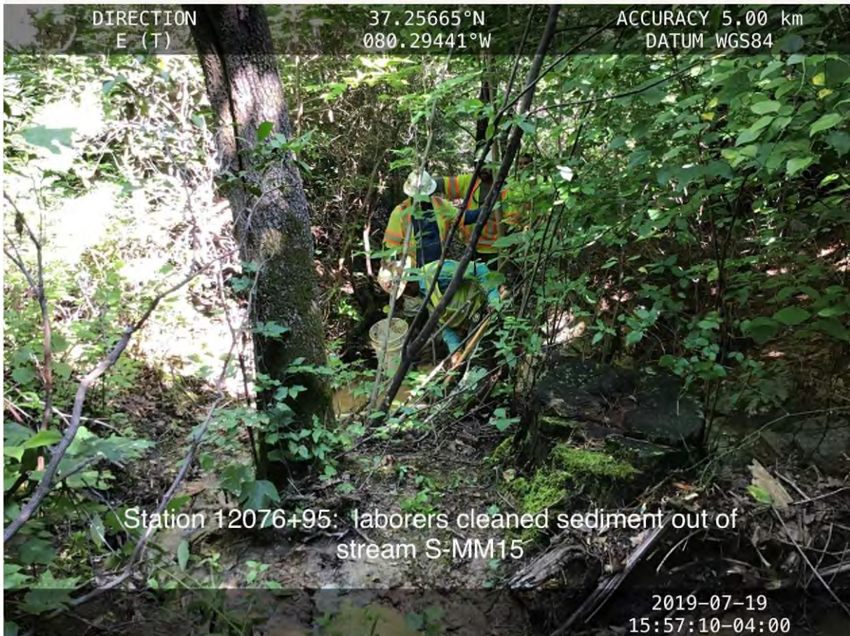
Figure 38 - Sediment deposited in UT Flatwoods Branch, July 19, 2019, Action Item Log ID 3248, Source: MBP [This is an example of what inspectors often term "remediation" through physical removal of sediments from the stream.]
