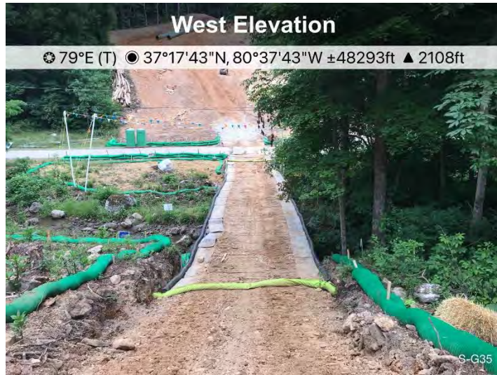
Figure 1: Designated crossing S-G35 ECD's are in place.
