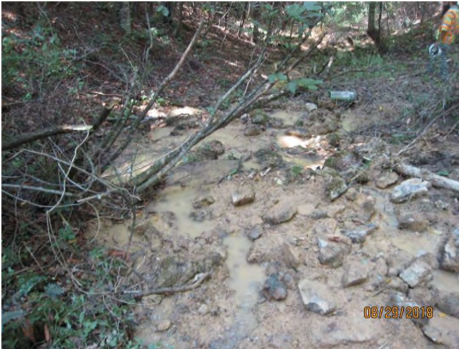
Figure 2 - Sediment deposited in UT Sinking Creek, August 29, 2018, DEQ VWP inspection, Source: DEQ [notes that sediment shown approx, 300 ft. downstream from ROW]
