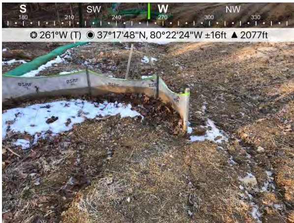
Figure 3: St11749+50 P1 requires sediment removal.
