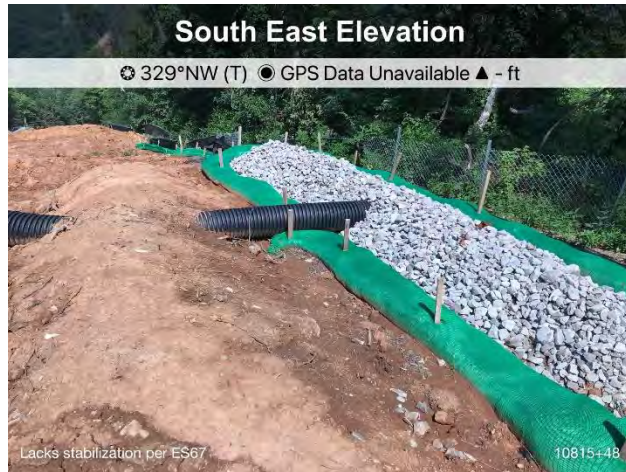
Figure 1: St10815+45 lacks stabilization per ES 67
