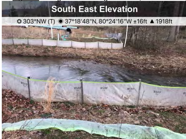
Figure 3: Designated crossing S-RR006, ECD's are in place.
