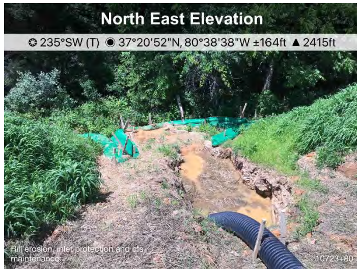
Figure 3: St10723+80 CFS requires sediment removal
