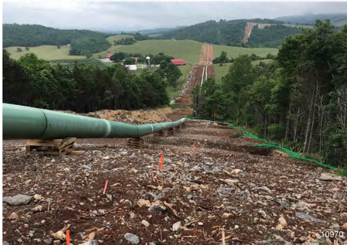
Figure 3: STA 10970+00 – Controls in place and functioning properly. BRG: 277°W (T) LAT: 37.327311 LON: -80.570350 ±16ft ALT: 2433ft
