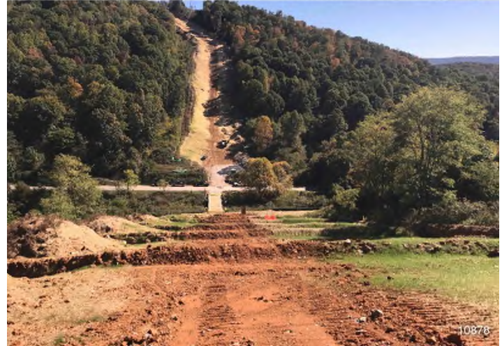
Figure 2: STA 10878+00 – Controls in place and functioning properly. Area stabilized outside of active travel lane. BRG: 89°E (T) LAT: 37.335681 LON: -80.598313 ±16ft ALT: 2296ft
