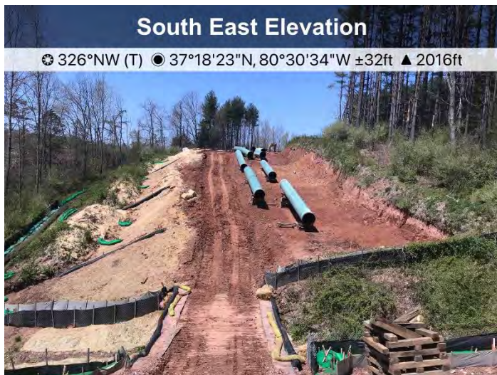
Figure 3: Near St11190, pipe has been strung and ECD's are in place for active construction.
