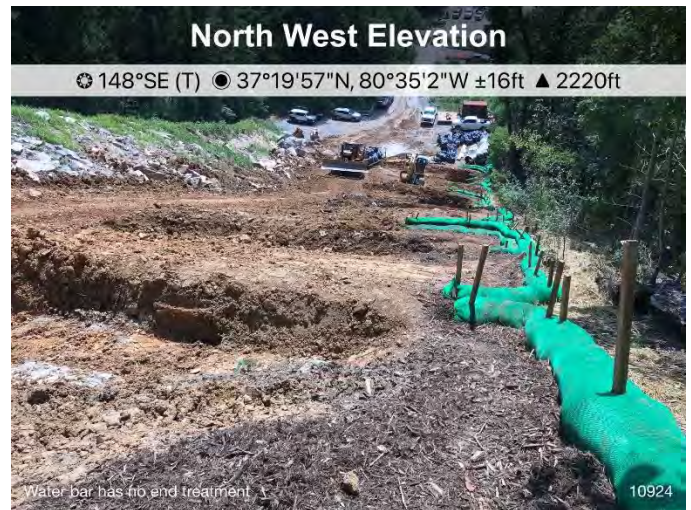
Figure 4: St 10924 waterbar has no end treatment
