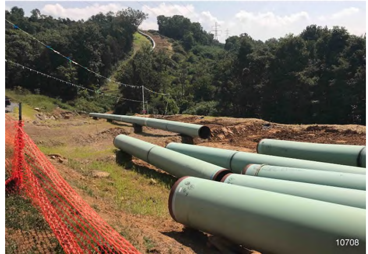
Figure 2: STA 10708+00 – Controls in place and functioning properly. BRG: 94°E (T) LAT: 37.348477 LON: -80.648721 ±32ft ALT: 2207ft
