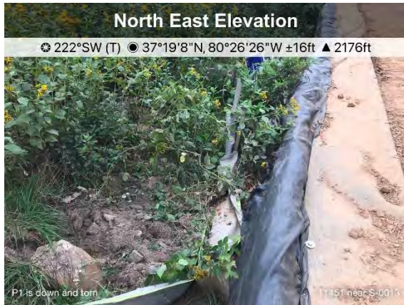
Figure 1: P1 is down and torn at near St 11451.
