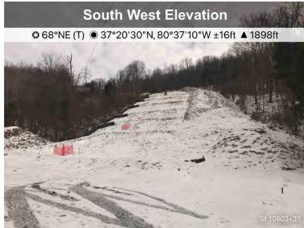
Figure 1: ESC controls were snow covered near St 10803+35
