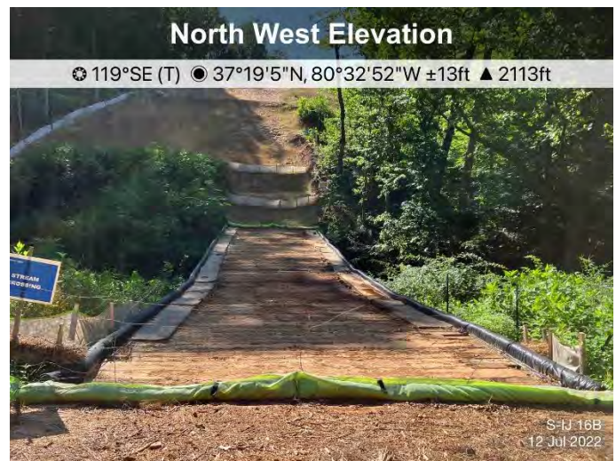
Figure 4: Designated crossing S-IJ16B, ECD's are in place.
