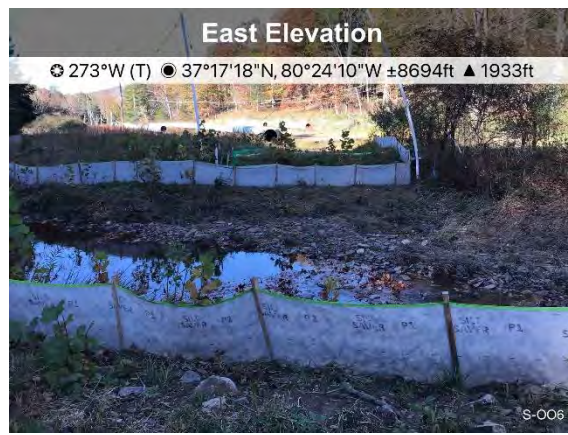
Figure 4: Designated crossing S-006, ECD's are in place.
