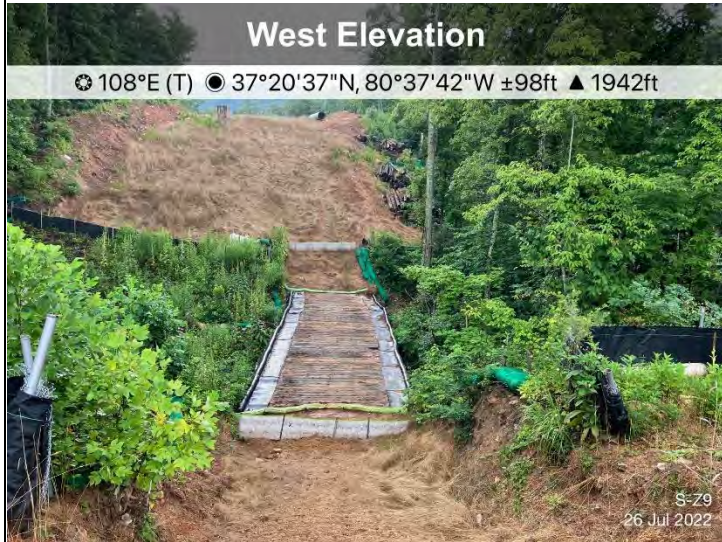
Figure 3: Designated crossing S-Z9, ECD's are in place.
