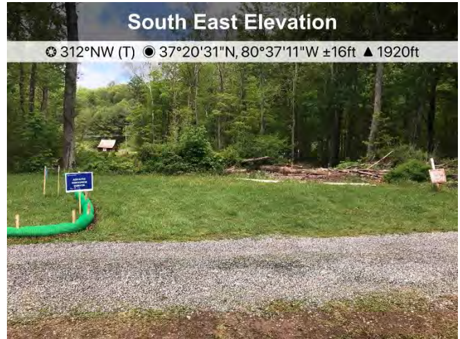
Figure 2: Designated crossing S-Z14, ECD's are in place.
