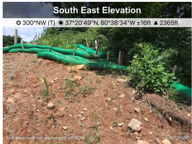
Figure 6: St 10728+87 end treatment is not allowing water off the ROW
