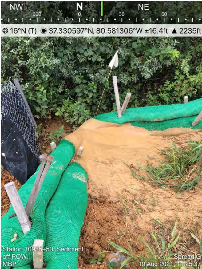
Figure 30 - Sediment overflowing compost filter socks, deposited off MVP ROW near UT Doe Creek, August 19, 2021, Action Log ID 5081, Source: MBP
