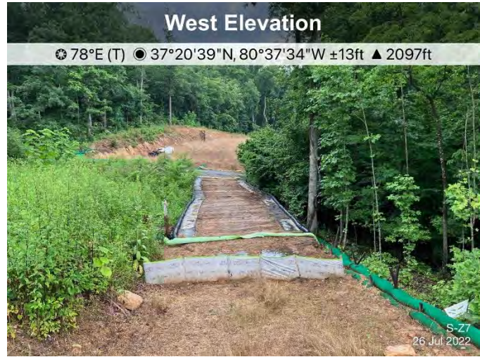
Figure 2: Designated crossing S-Z7, ECD's are in place.
