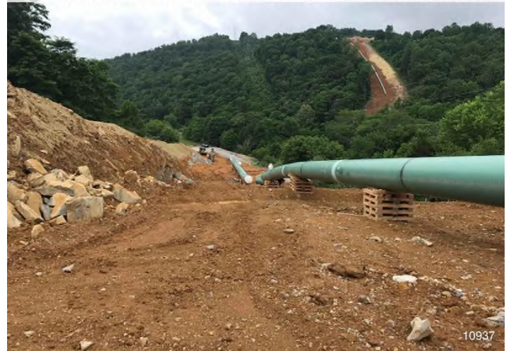
Figure 4: STA 10937+00 – Controls in place and functioning properly. BRG: 291°W (T) LAT: 37.330321 LON: -80.580914 ±16ft ALT: 2283ft
