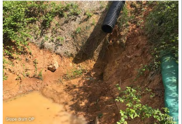
Figure 8: STA 11274+00 – Slope drain does not have outlet protection. BRG: 11°N (T) LAT: 37.295878 LON: -80.487701 ±32ft ALT: 2263ft
