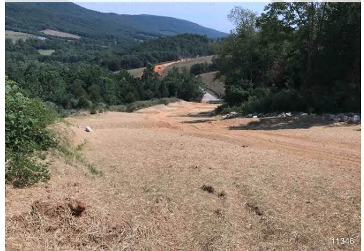
Figure 4: STA 11346+00 – Controls in place and functioning properly. BRG: 34°NE (T) LAT: 37.303949 LON: -80.468563 ±98ft ALT: 2087ft
