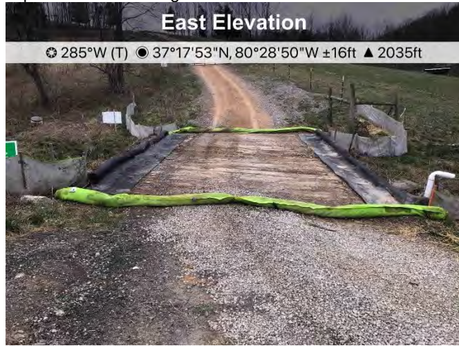
Figure 1: Designated crossings S-MM17 and W-MM10, ECD's are in place and functioning.
