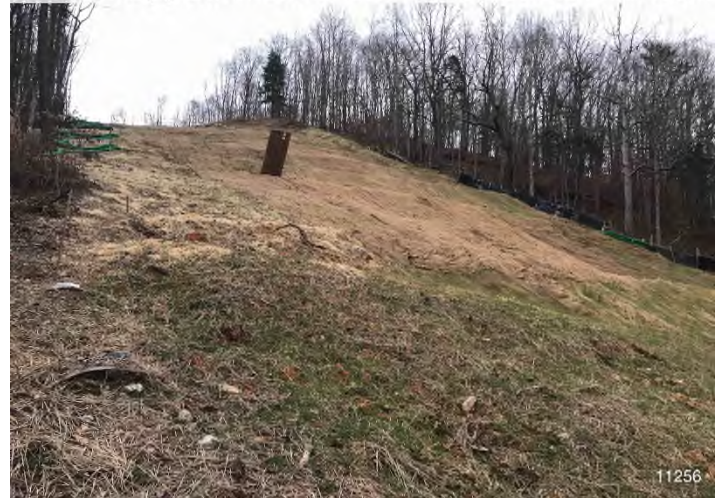
Figure 4: STA 11256+00 – Controls in place and functioning properly. Area stabilized with straw BRG: 122°SE (T) LAT: 37.296724 LON: -80.493480 ±32ft ALT: 1961ft
