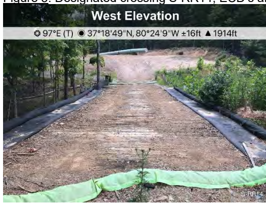
Figure 3: Designated crossing S-RR14, ECD's are in place.
