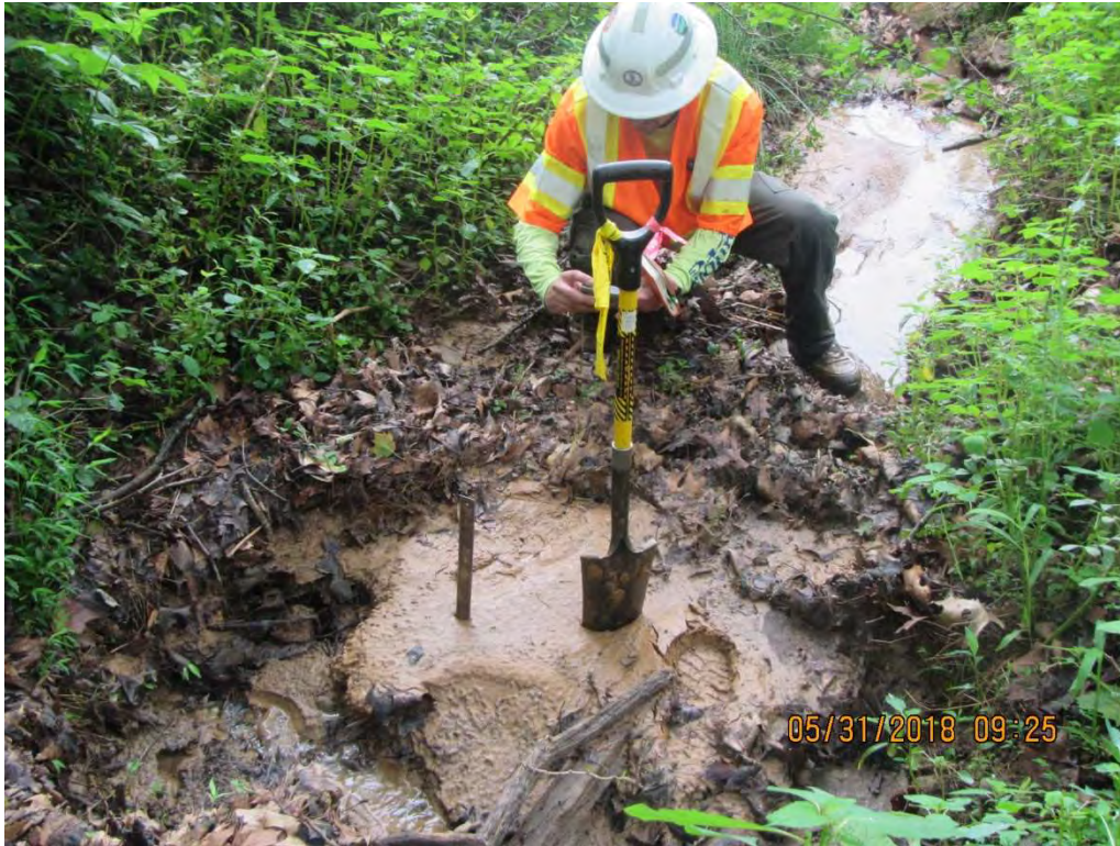
Sediment in channel near treeline ~1,000-feet from MVP LOD Channel 3-feet wide; Sediment depth 6.5-inches
