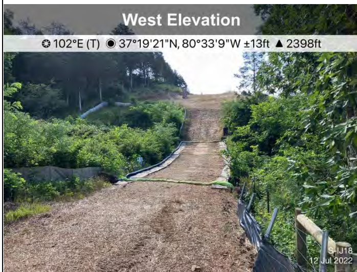
Figure 3: Designated crossing S-IJ18, ECD's are in place.
