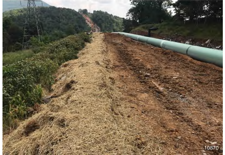
Figure 2: STA 10870+00 – Controls in place and functioning properly. BRG: 114°SE (T) LAT: 37.336352 LON: -80.601044 ±32ft ALT: 2448ft
