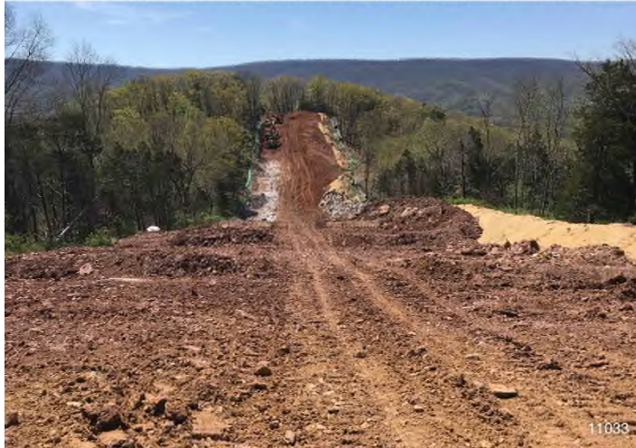
Figure 3: STA 11033+00 – Controls in place and functioning properly. BRG: 148°SE (T) LAT: 37.321152 LON: -80.550845 ±16ft ALT: 2386ft
