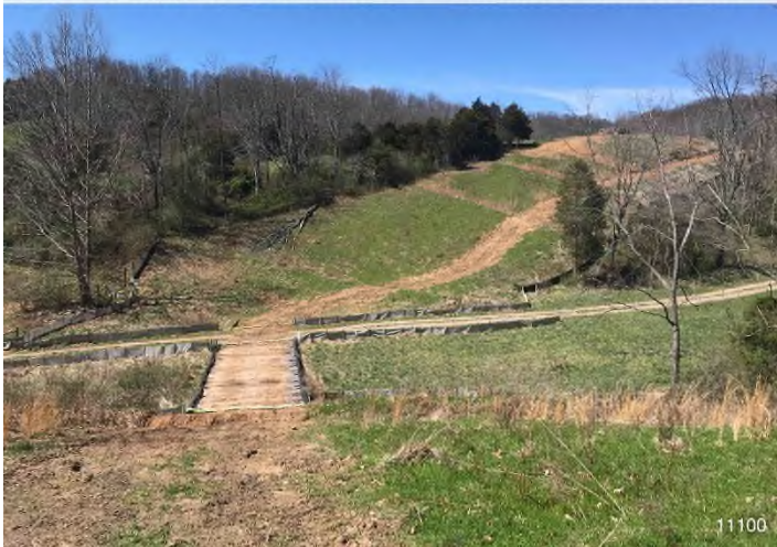
Figure 3: STA 11100+00 – Controls in place and functioning properly. BRG: 273°W (T) LAT: 37.313195 LON: -80.533283 ±32ft ALT: 1984ft
