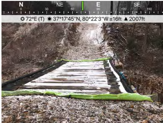
Figure 1: Designated crossing S-IJ52 ECD's are in place.
