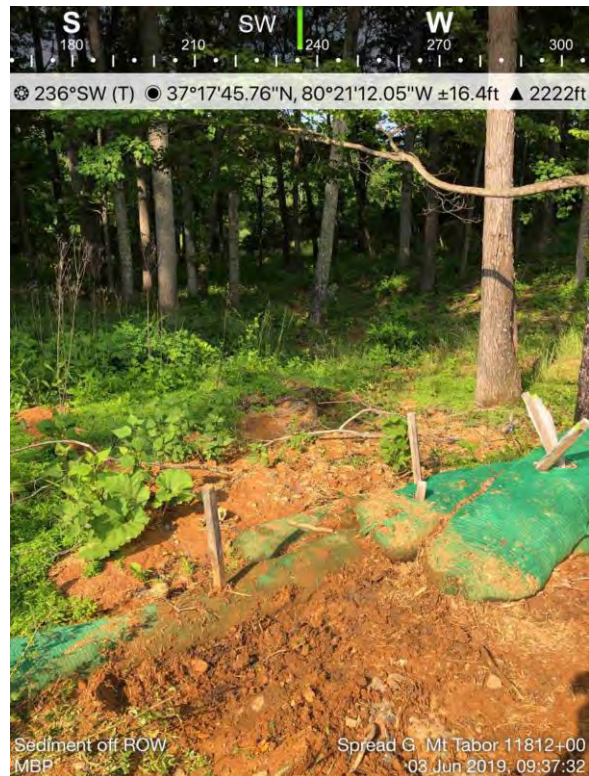
Figure 11 - Sediment deposited off ROW, June 3, 2019, Action Item ID 2844, near Dry Run, Source: MBP
