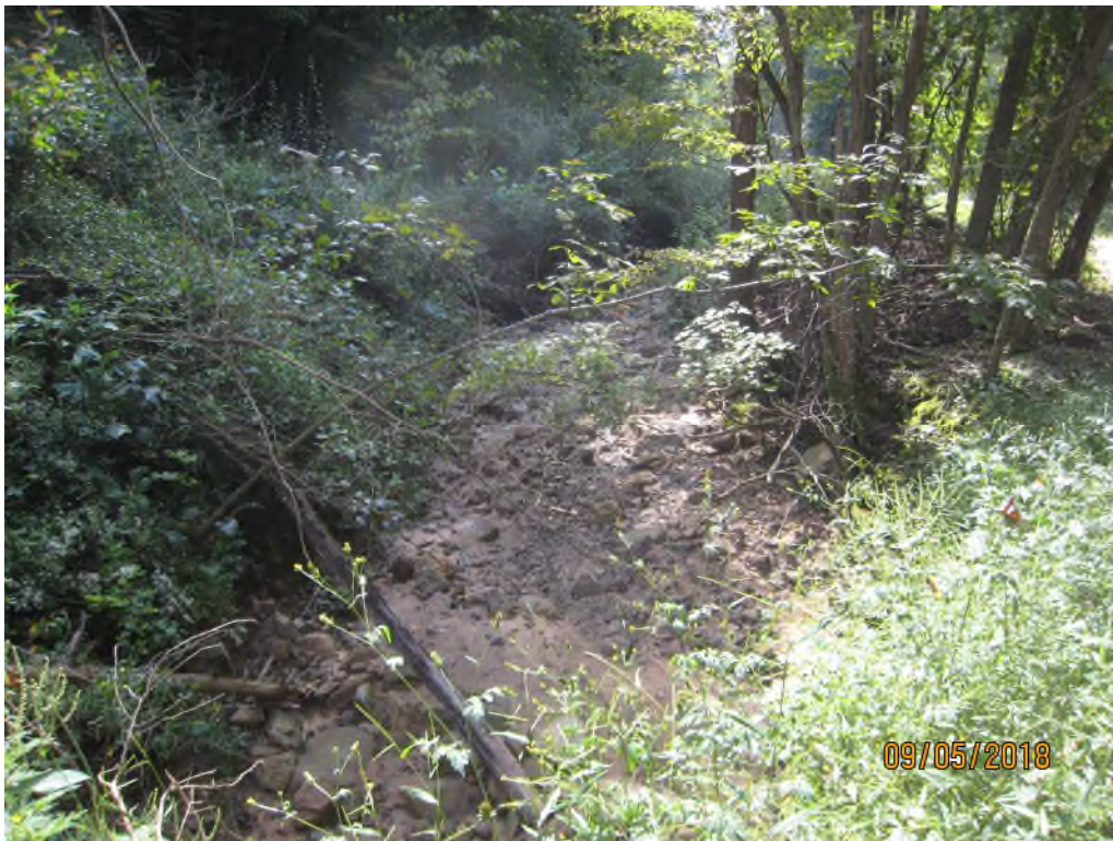
Photo 6: Sedimentation in channel downstream of Rogers Road culverts; no landowner permission Orientation: Downstream
