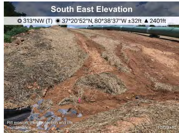
Figure 2: St10723+80 rill erosion and sediment in inlet protection
