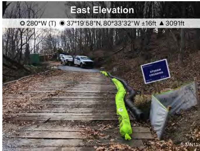
Figure 1. Designated crossing S-MN11, ECD's are in place.
