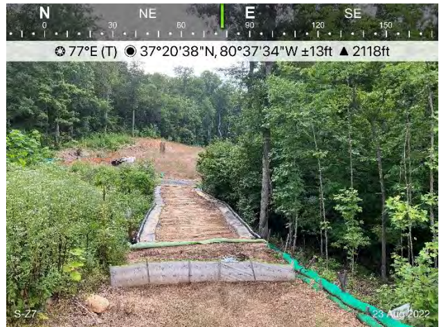
Figure 2: Designated crossing S-Z7, ECD's are in place.
