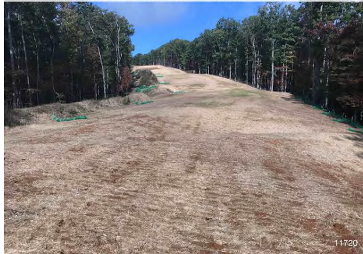
Figure 3: STA 11720+00 – Controls in place and functioning properly. Area stabilized with straw. BRG: 318°NW (T) LAT: 37.295088 LON: -80.381955 ±98ft ALT: 2250ft
