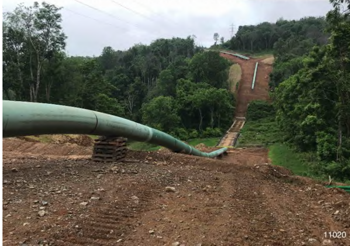
Figure 1: STA 11020+00 – Controls in place and functioning properly. BRG: 281°W (T) LAT: 37.323307 LON: -80.554028 ±16ft ALT: 2458ft
