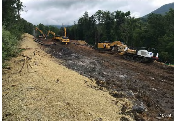
Figure 2: STA 10669+00 – Controls in place and functioning properly. BRG: 22°NE (T) LAT: 37.345776 LON: -80.673701 ±42813ft ALT: 2272ft
