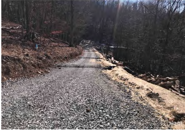
Figure 1: MVP-GI-242.01 – Controls in place and functioning properly along access road. BRG: 140°SE (T) LAT: 37.332773 LON: -80.560607 ±16ft ALT: 3018ft
