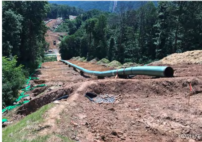
Figure 3: STA 10751+77 – Controls in place and functioning properly. BRG: 102°E (T) LAT: 37.344677 LON: -80.635558 ±98ft ALT: 2229ft
