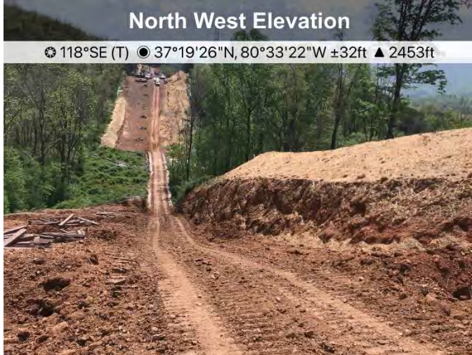
Figure 1: Above designated crossing S-RR5/ PA07, ECD's are in place for active construction.
