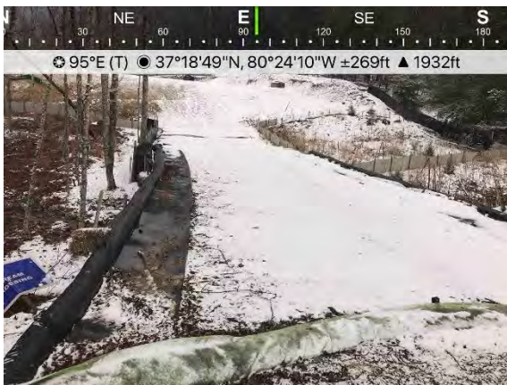
Figure 3: Designated crossing S-RR14 ECD's are in place.
