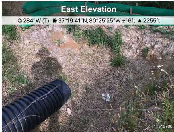
Figure 1: St 11515+30 sump lacks stone.
