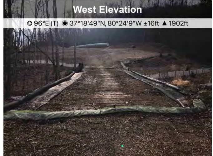
Figure 2: Designated crossing S-RR14, ECD's are in place.
