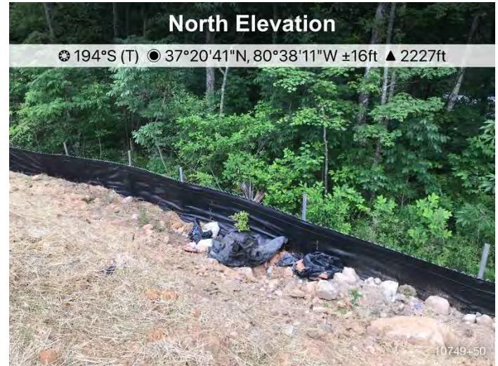
Figure 2: Uncontained trash at St10749+50
