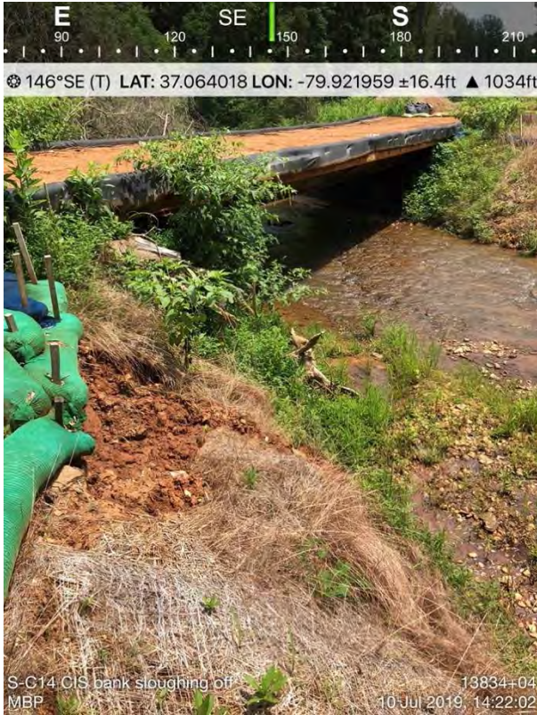
Figure 42 - Stream bank eroded at MVP site, Teels Creek, July 10, 2019, Action Log ID 3187, Source: MBP
