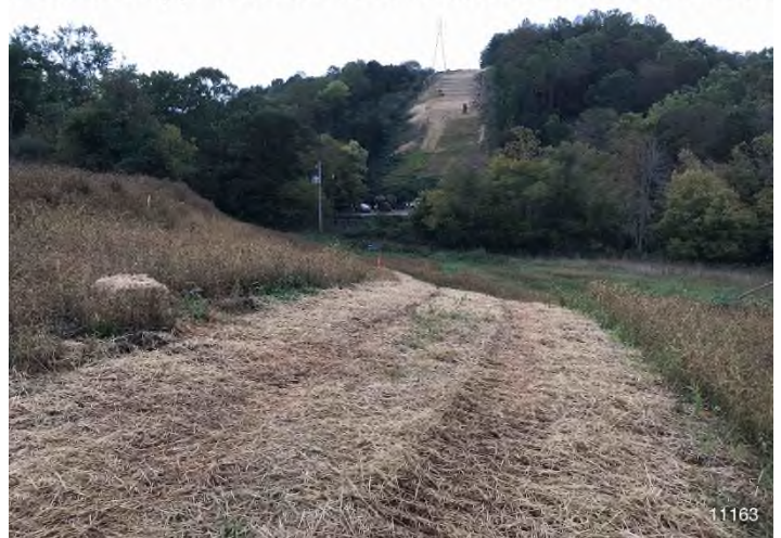
Figure 4: STA 11163+00 – Controls in place and functioning properly. BRG: 288°W (T) LAT: 37.311478 LON: -80.514426 ±98ft ALT: 1862ft
