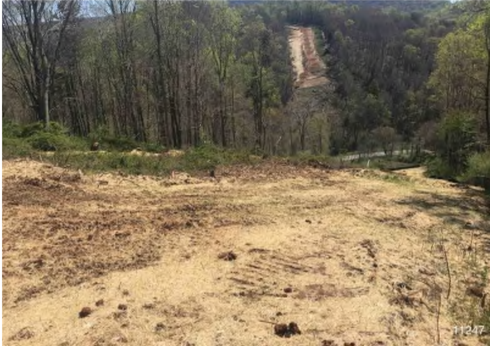
Figure 1: STA 11247+00 – Controls in place and functioning properly. BRG: 106°E (T) LAT: 37.302043 LON: -80.505112 ±12986ft ALT: 2229ft
