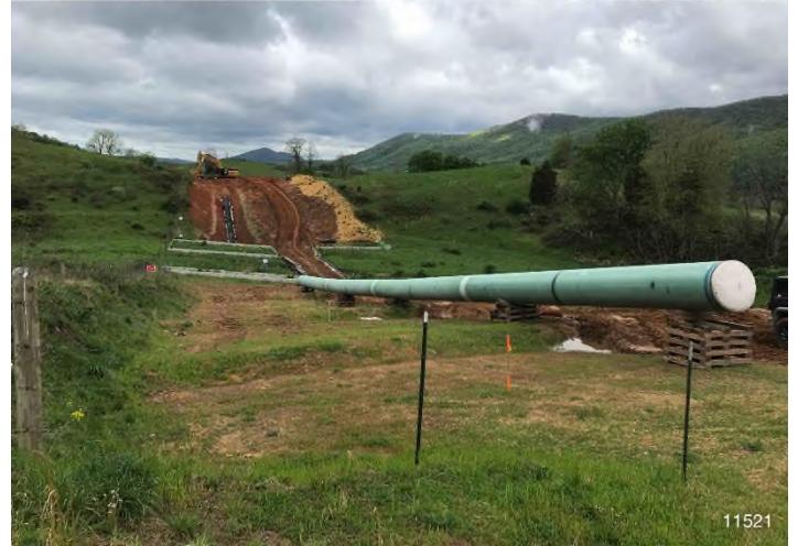
Figure 2: STA 11521+00 – Controls in place and functioning properly. BRG: 263°W (T) LAT: 37.328683 LON: -80.421833 ±16ft ALT: 2248ft
