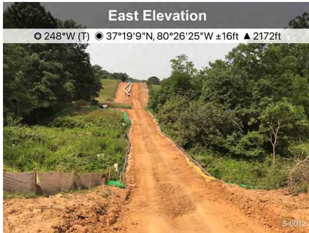
Figure 1: Designated crossing S-0012
