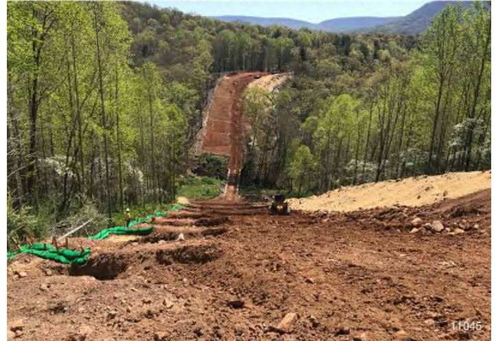
Figure 4: STA 11045+00 – Controls in place and functioning properly. BRG: 112°E (T) LAT: 37.326534 LON: -80.550608 ±9564ft ALT: 2346ft
