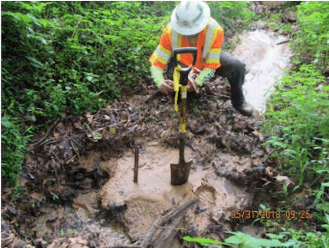
Figure 9 - Sediment deposited in UT Blackwater River, May 31, 2018, DEQ VWP inspection report, Source: DEQ [sediment covered approx. 1,110 linear feet of streambed, up to 7 inches deep]
