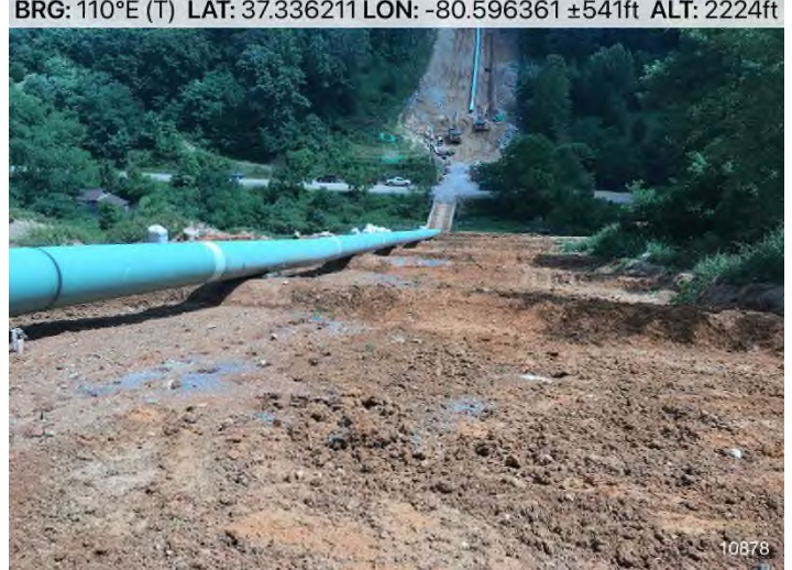
Figure 4: STA 10878+00 – Controls in place and functioning properly. BRG: 110°E (T) LAT: 37.336211 LON: -80.596361 ±541ft ALT: 2224ft
