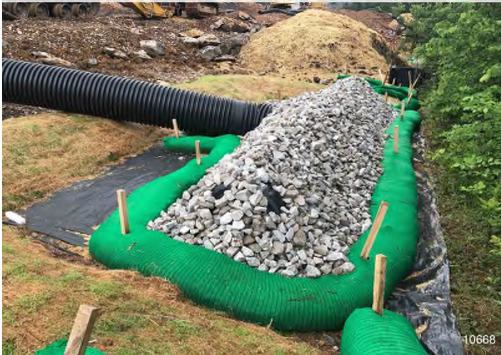
Figure 3: STA 10668+00 – Controls in place and functioning properly. BRG: 316°NW (T) LAT: 37.351774 LON: -80.660598 ±16ft ALT: 2224ft
