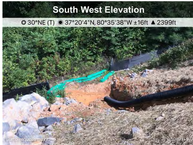
Figure 1: St 10891+97 sump requires maintenance
