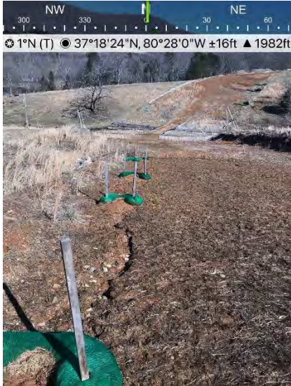
Figure 1: Near St11358 multiple CFS and rill erosion require repair.
