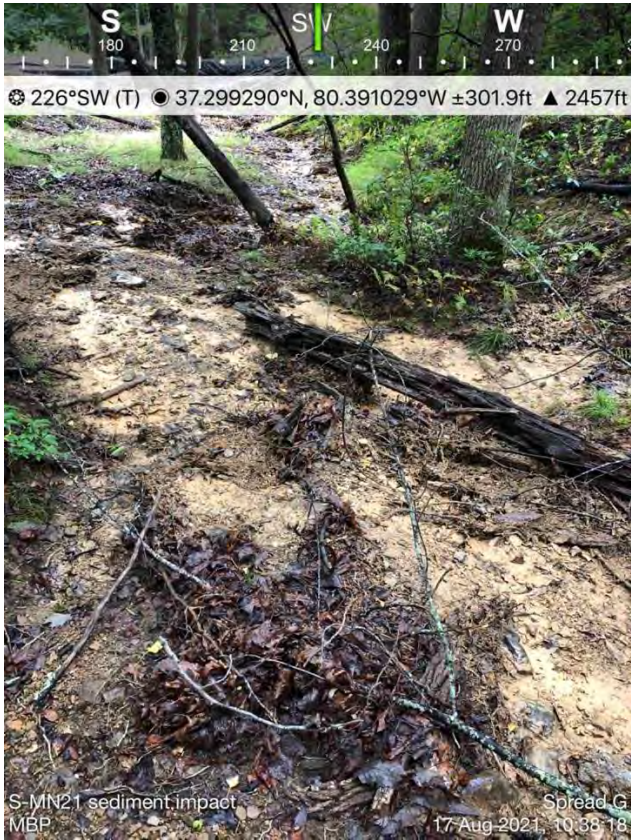
Figure 7 - Sediment deposited in UT Mill Creek and adjacent property, August 16, 2021, Action Log ID 5035, deadline to clean up extended loa [report states impacts extend approx. 75 linear feet upstream and 100 linear feet downstream; landowner denied permission to access impacted areas; approx. 3 months later, inspector reported sediment deposits no longer visible.
