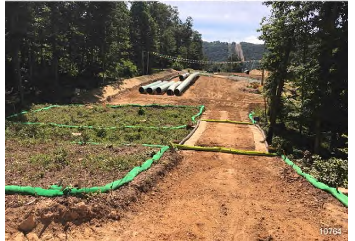
Figure 4: STA 10764+00 – Controls in place and functioning properly. BRG: 80°E (T) LAT: 37.343719 LON: -80.632378 ±1384ft ALT: 2078ft
