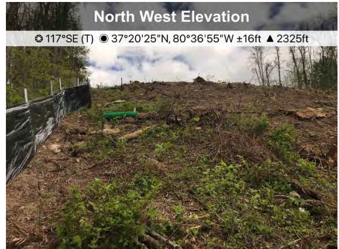
Figure 4: Near St10817+20 WB does not extend the full length of the ROW.
