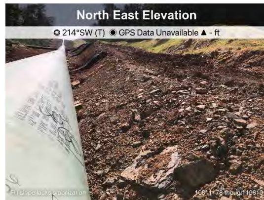
Figure 3: St10811+78 to10810 two tone area lacks stabilization
