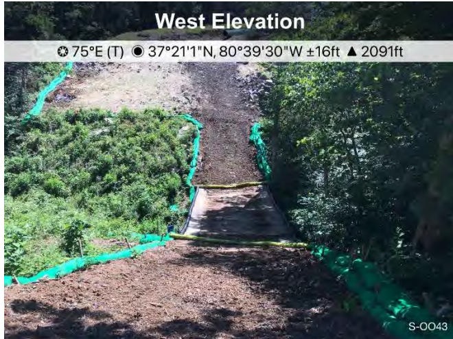
Figure 5: Designated crossing S-0043, ECD's are in place.
