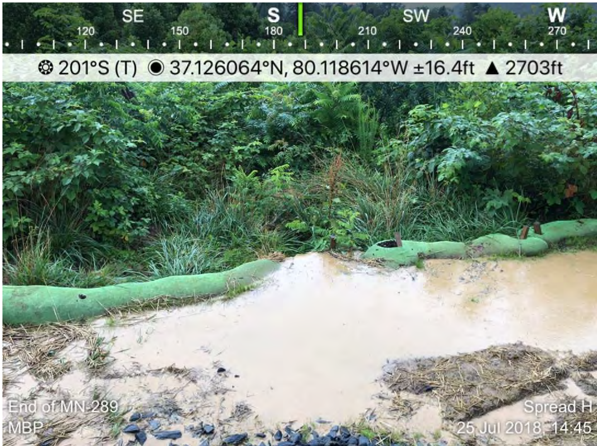
Figure 45 - Sediment-laden water overtopping perimeter control, July 25, 2018, Action Log ID 458, Source: MBP [an additional compost filter sock was added 10 days after this situation was observed]
