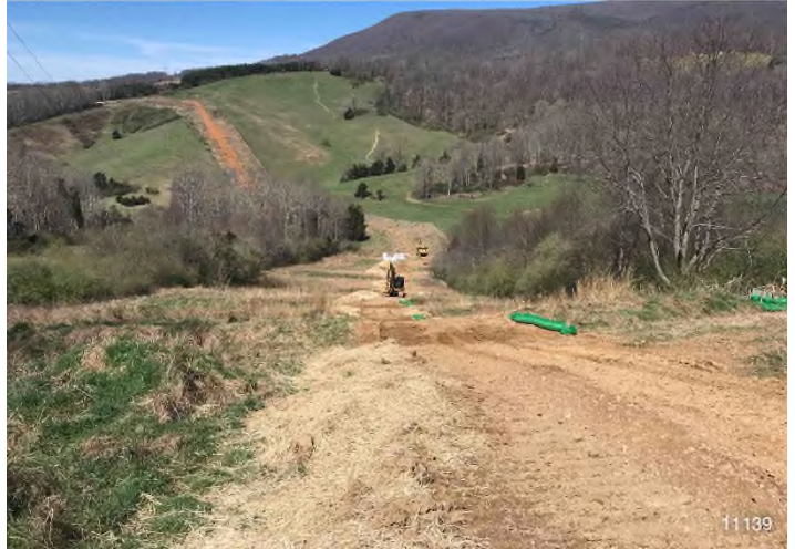
Figure 2: STA 11139+00 – Controls in place and functioning properly. BRG: 305°NW (T) LAT: 37.313599 LON: -80.522308 ±16ft ALT: 2149ft
