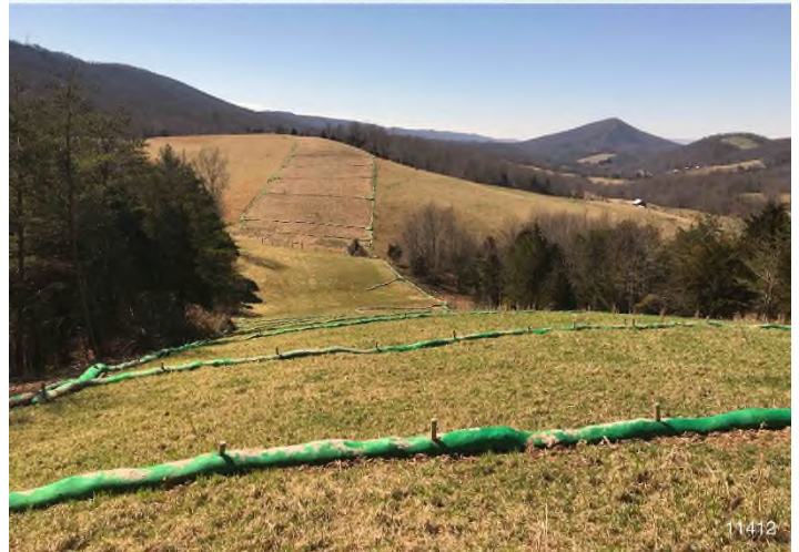
Figure 4: STA 11412+00 – Controls in place and functioning properly. BRG: 238°SW (T) LAT: 37.317810 LON: -80.446642 ±20216ft ALT: 2115ft
