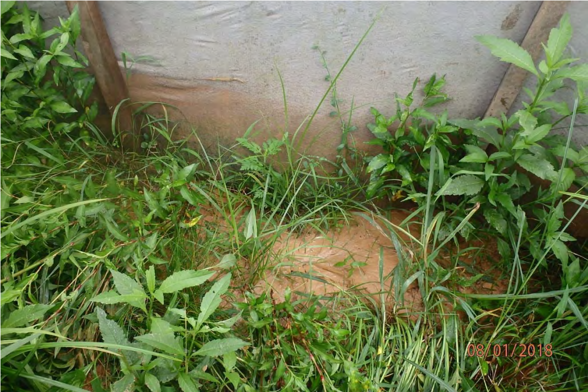
Perimeter controls adjacent to Goose Run that are undermined and allowing sediment laden water to leave the site. Deficiencies in site evaluation item numbers 1, 6, 19, 20 & 21 pictured.
