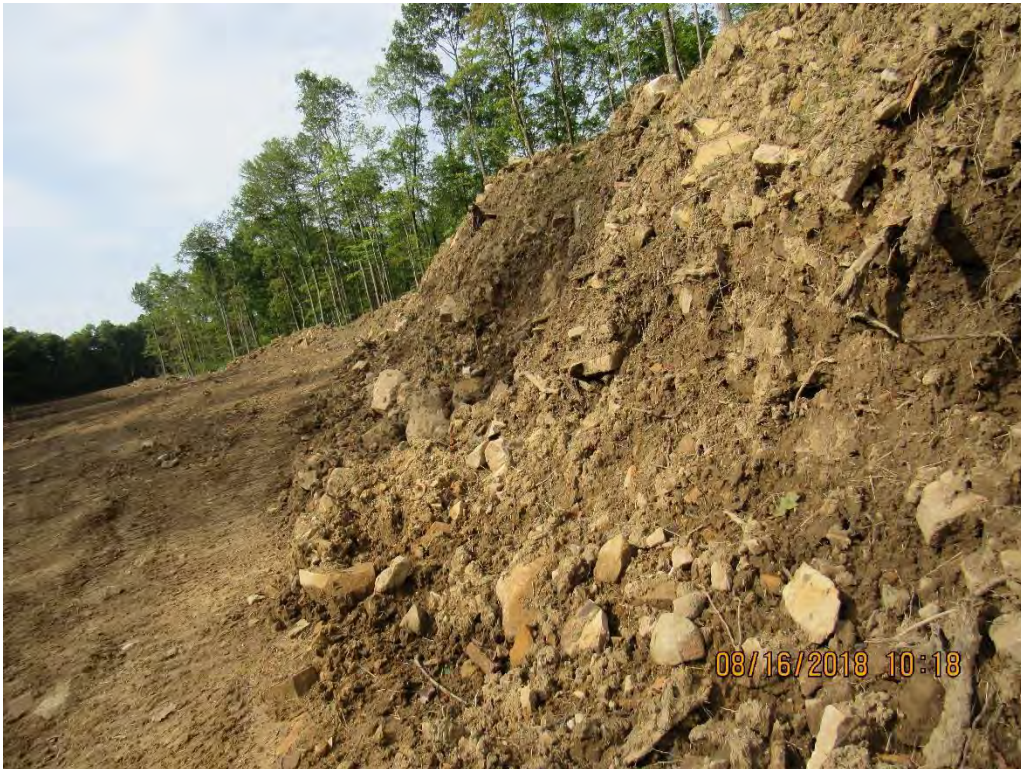
Photo 20: Southern view of waste pile with inadequate stabilization. (Photo taken near Bingham Road station 7450+00)
