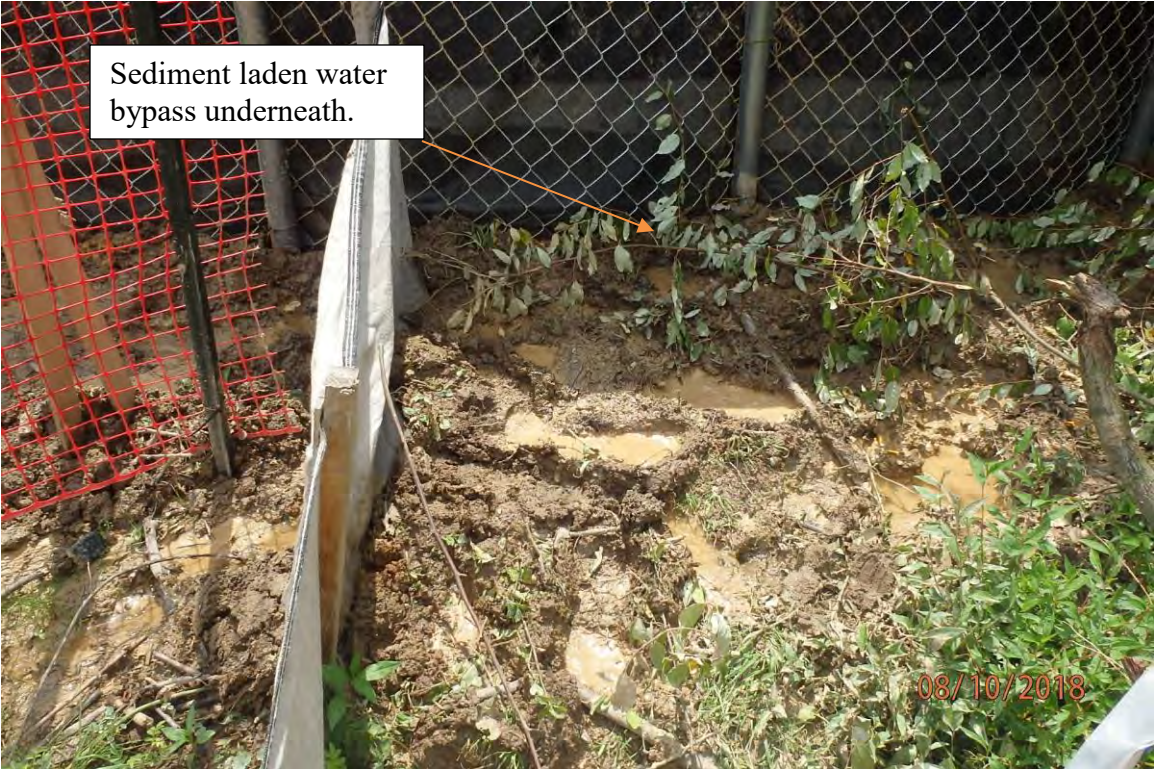
Water bar terminus BMP that was improperly operated and allowed sediment laden water to leave the site. This caused CNA deposits in wetland UNT Left Fork of Freemans Creek (W-B47) (39° 04.744' X 80° 34.904). Deficiencies in site evaluation item numbers 6, 7, 19, 20 & 21 pictured.
