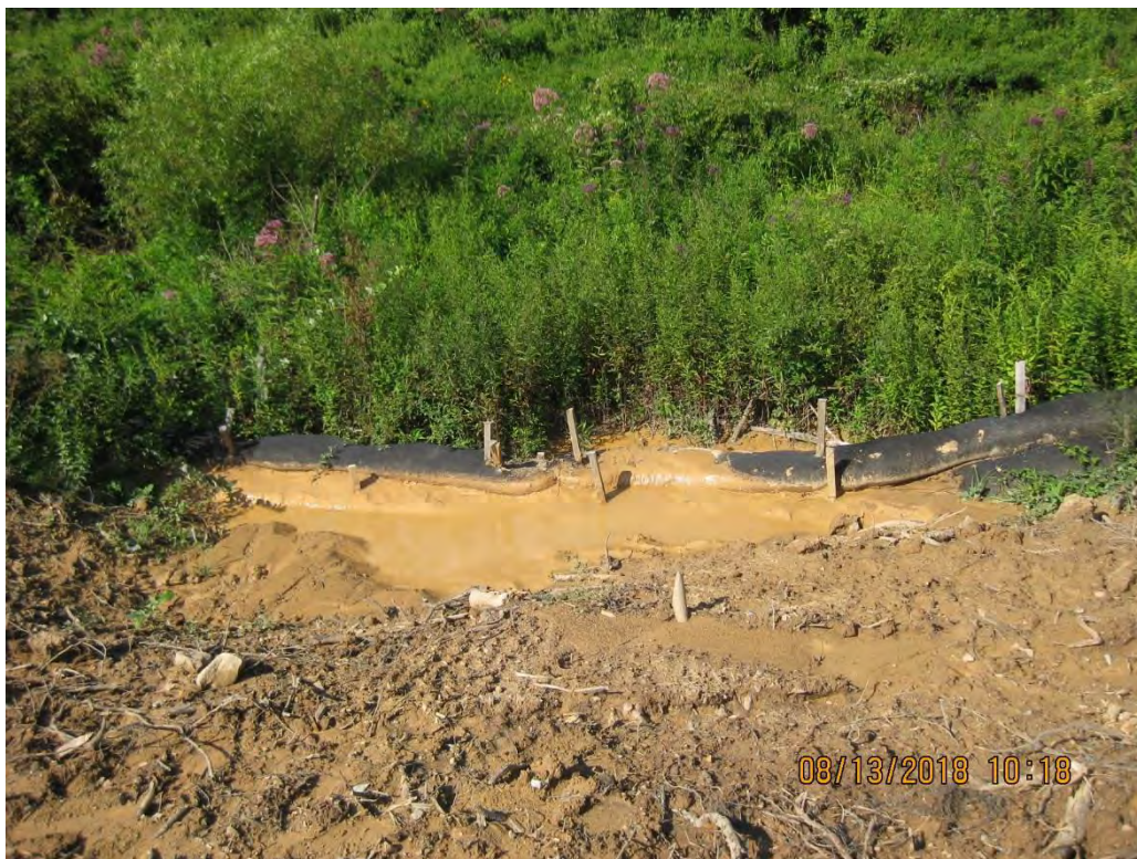
At St. 00+150 Sediment laden water left the site as a result of perimeter controls receiving concentrated flow and a lack of fill slope protection.
