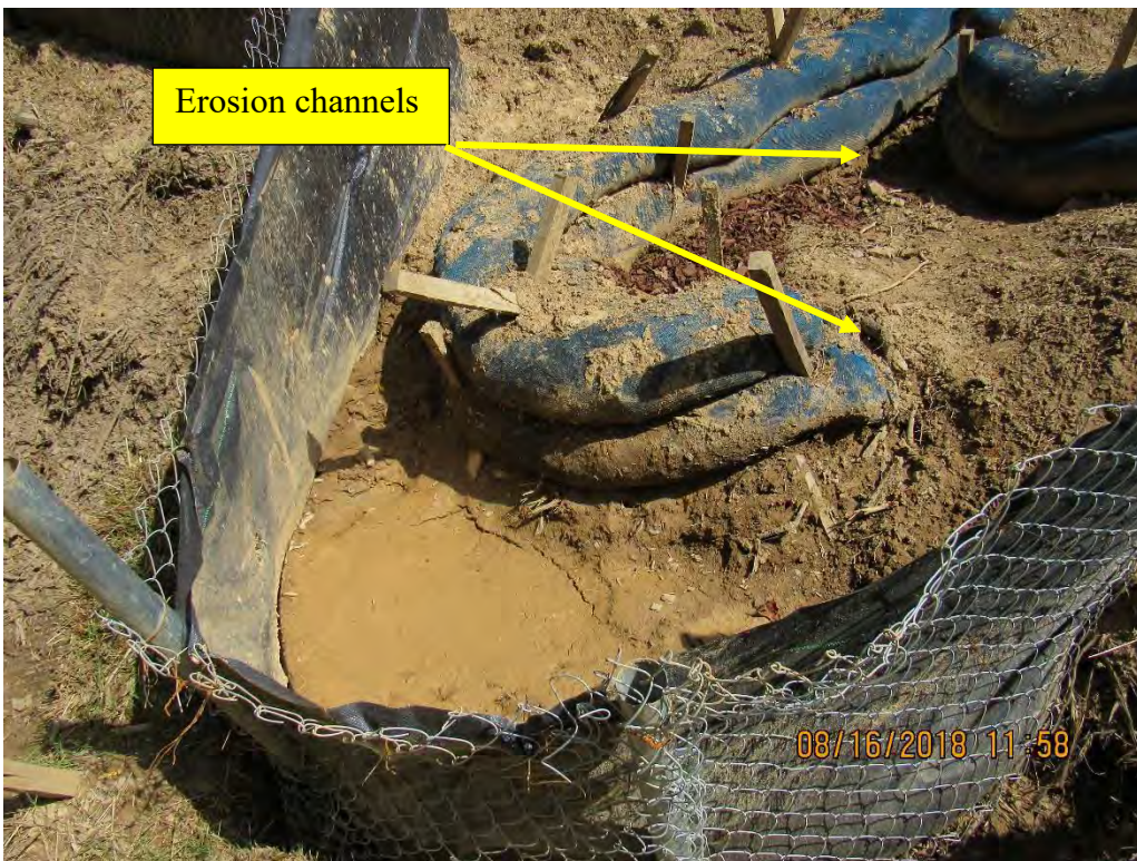
Photo 24: Water bar terminus at station 7084+00. Erosion channels observed at ends of CFS.
