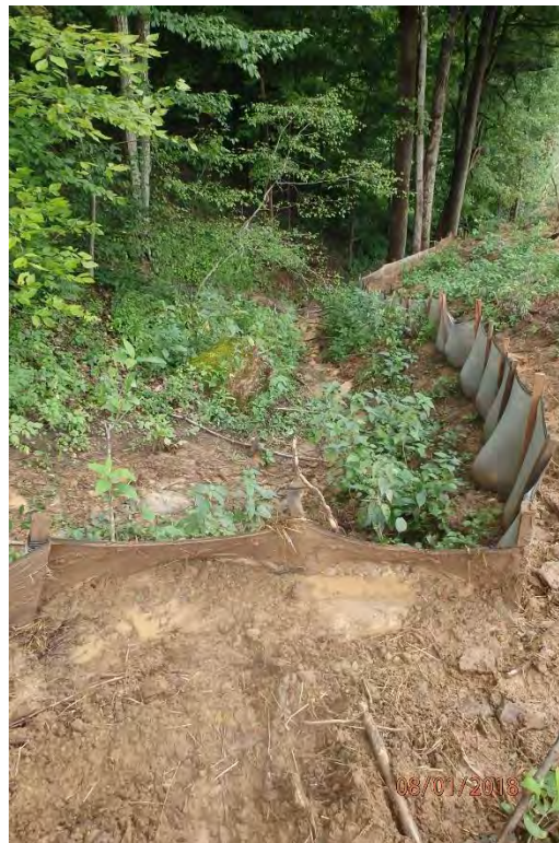
Perimeter control that has been overwhelmed due to concentrated flow from improperly installed water bars in the Goose Run watershed. Deficiencies in site evaluation item numbers 1, 6, 7, 14, 19, 20 & 21 pictured.
