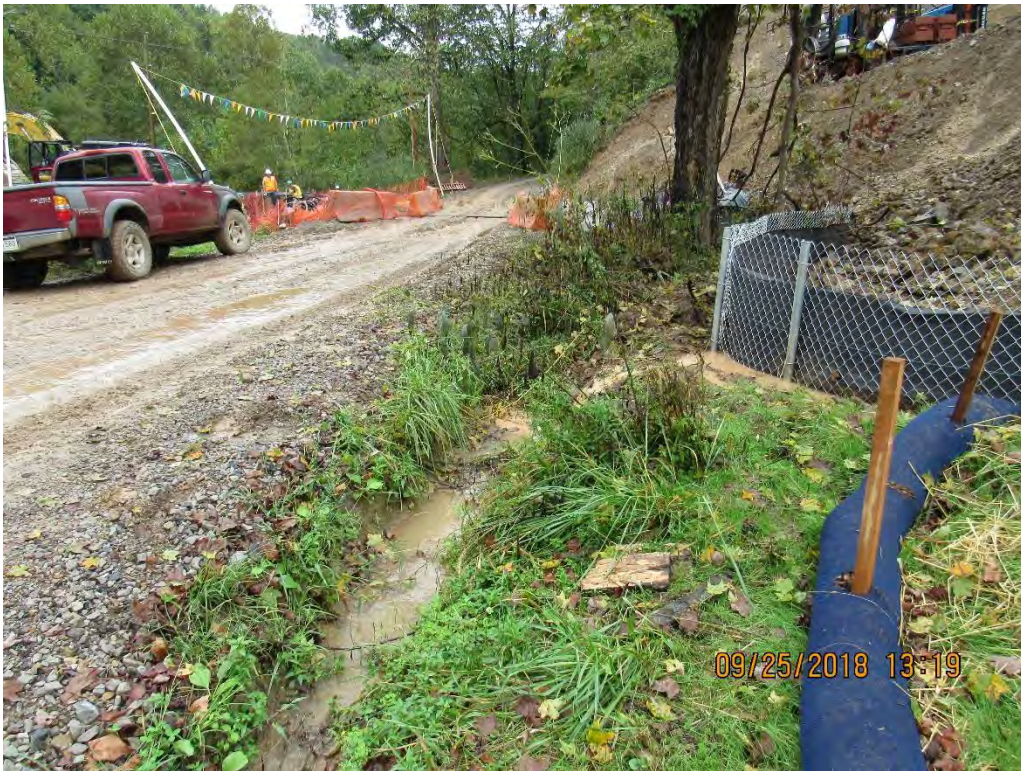
Photo 5: Sediment laden water entering UNT of Knowls Creek near station 3634+00 from failed perimeter controls.
