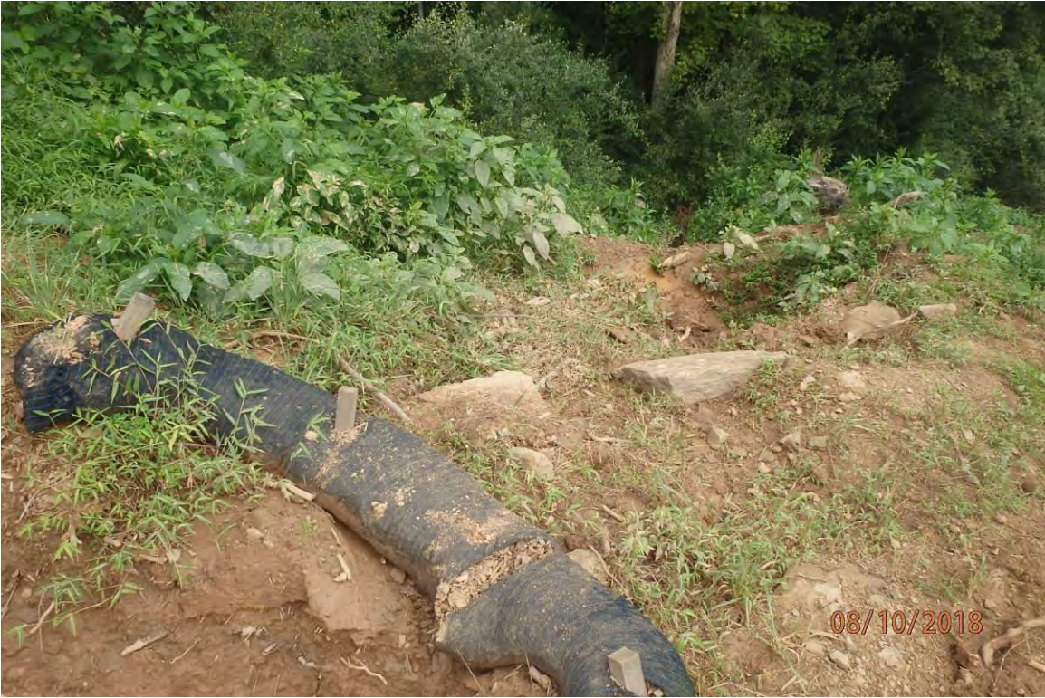
Water bar outlet indicated in above picture that allowed sediment laden water to leave the site and cause CNA in UNT Kincheloe Creek (39° 10.006' X 80° 34.736'). Deficiencies in site evaluation item numbers 2, 6, 7, 8, 14, 19, 20 & 21 pictured.
