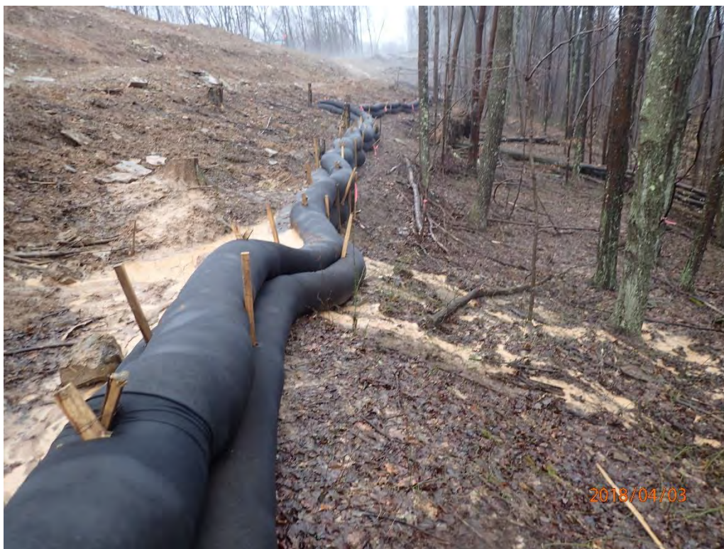
Second site of sediment laden water leaving site at Bradshaw Compressor Station.
