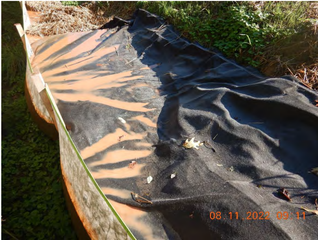
Photo # DSCN2180 – Trench de-watering filter bag located within Mountain Valley Pipeline’s permitted limits of disturbance. Sediment laden water can be seen on top of the filter bag.
