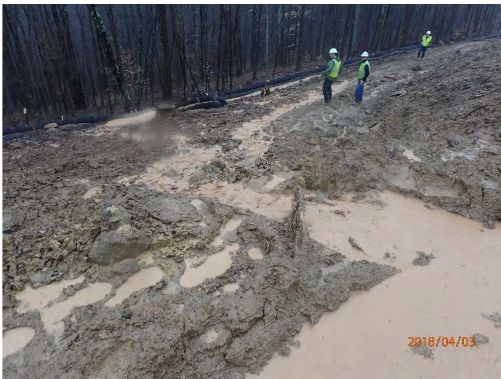
Third site of sediment laden water leaving site at Bradshaw Compressor Station.
