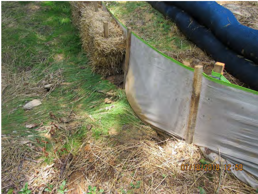
Photo 11: Down gradient of control failure from Photo 10. Photo #7 shows terminus of this control failure.
