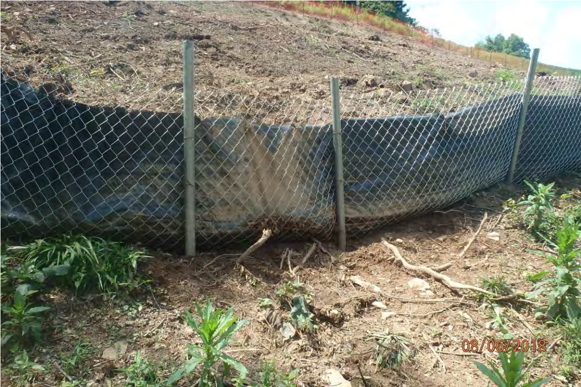
Perimeter control that was overwhelmed by concentrated flow and caused CNA deposits in Seal Run. Deficiencies in site evaluation item numbers 1, 2, 6, 7, 13, 14, 19, 20 & 21 pictured.
