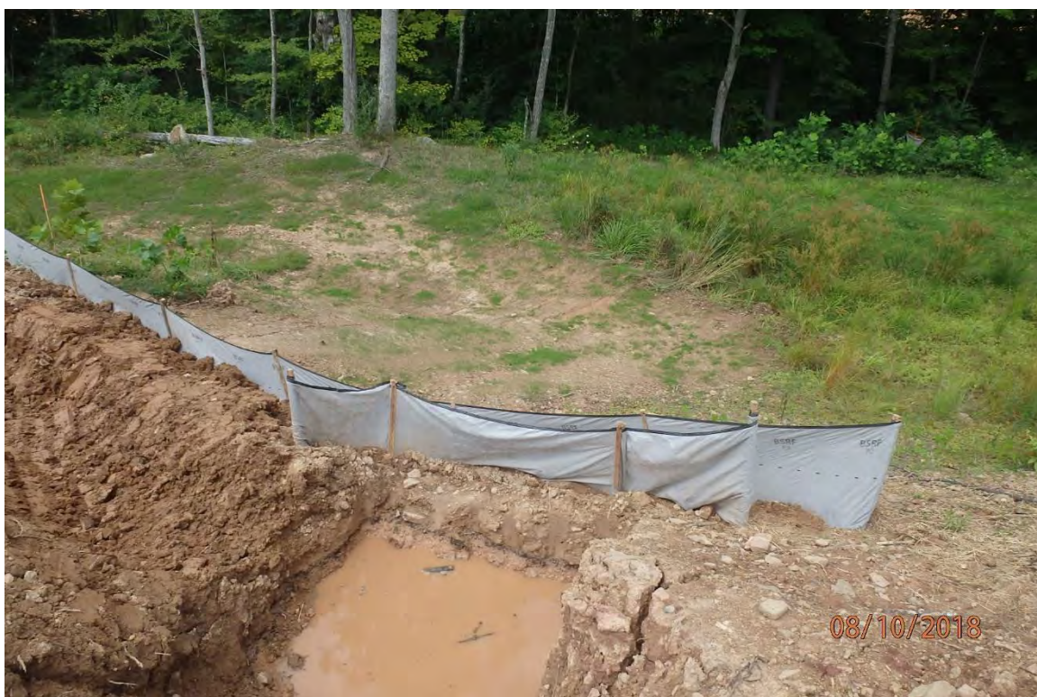
Unstable diversion that runs parallel to the slope and the associated erosion and offsite sediment deposits in the Cove Lick watershed. Deficiencies in site evaluation item numbers 2, 6, 8, 14, 19 & 21 pictured.
