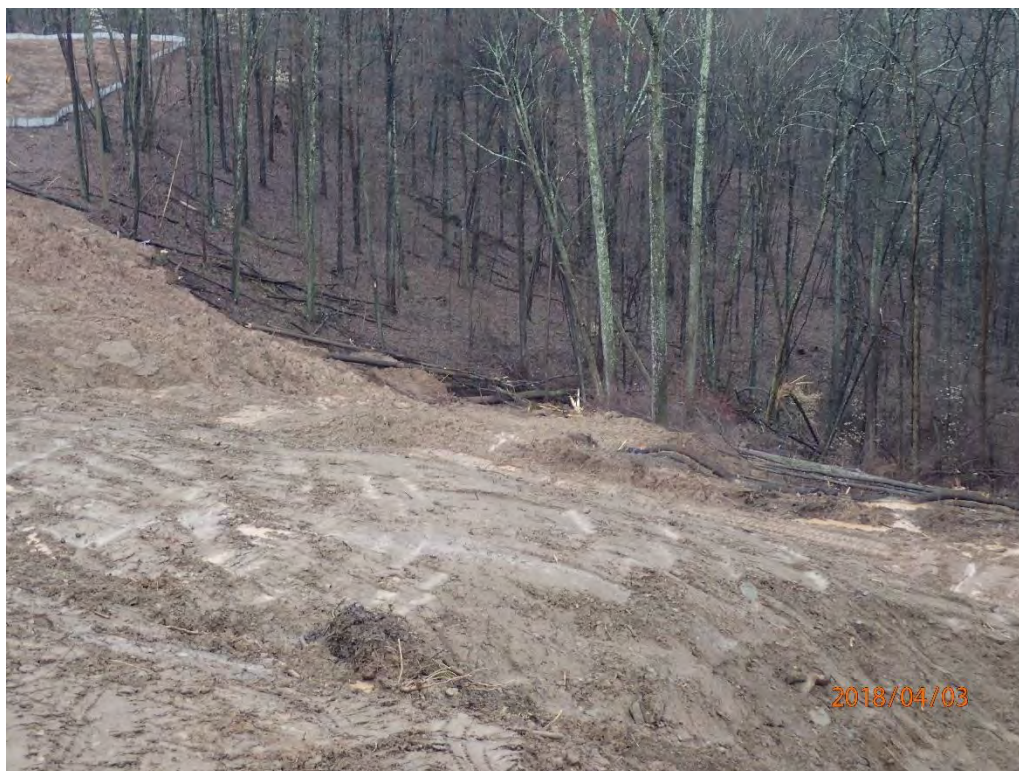
Slope above slip area.
