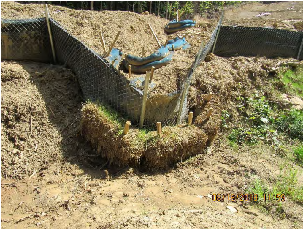
Photo 25: Controls and sediment deposits in road side ditch at water bar terminus at station 7084+00.
