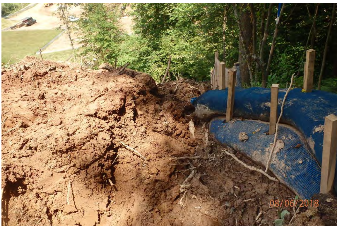
Water bar in Grass Run watershed that is improperly installed and led to CNA deposits in the stream. Deficiencies in site evaluation item numbers 1, 2, 6, 7, 8, 14, 19, 20 & 21 pictured.
