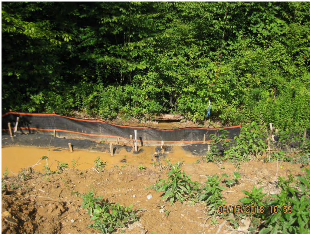
At St. 00+650 Sump/CFS/Priority 1 SF for terminus of upper diversion has not been maintained, sediment laden water left the site as a result.
