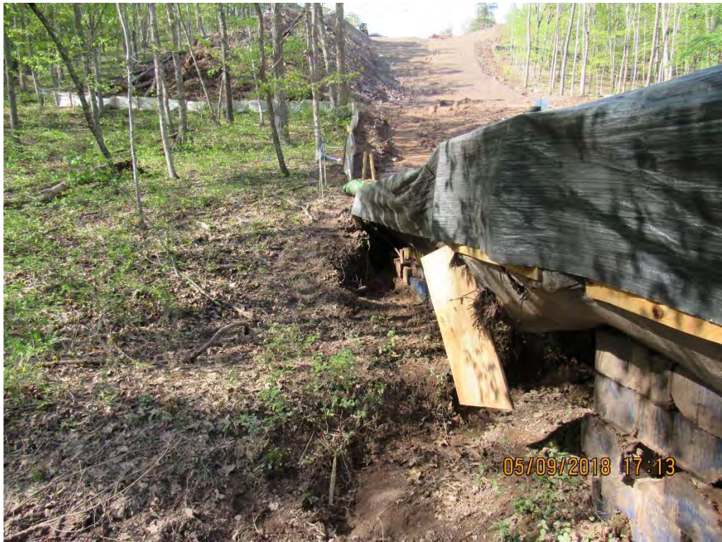
Photo 5: Stream crossing where sediment laden water left site after controls failed at stream S-IJ65 (view north). Additional controls added prior to re-building of bridge.
