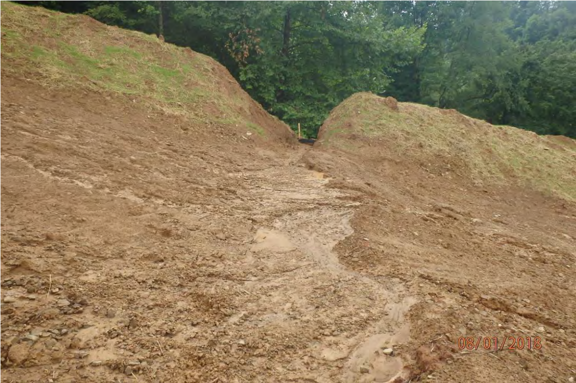
Improperly installed and poorly maintained water bars in the Goose Run watershed. Deficiencies in site evaluation item numbers 6, 7, 14, 19, 20 & 21 pictured.
