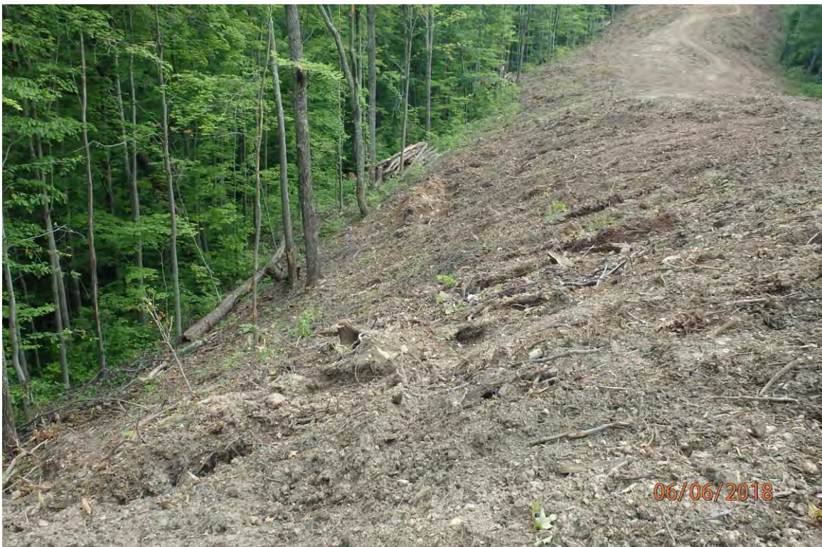
Areas of the project that have been cleared to mineral soil and BMPs are not in place as indicated in the SWPPP. Deficiencies in site evaluation item numbers 1, 7, 8, 13, 15, 19 & 21 pictured.
