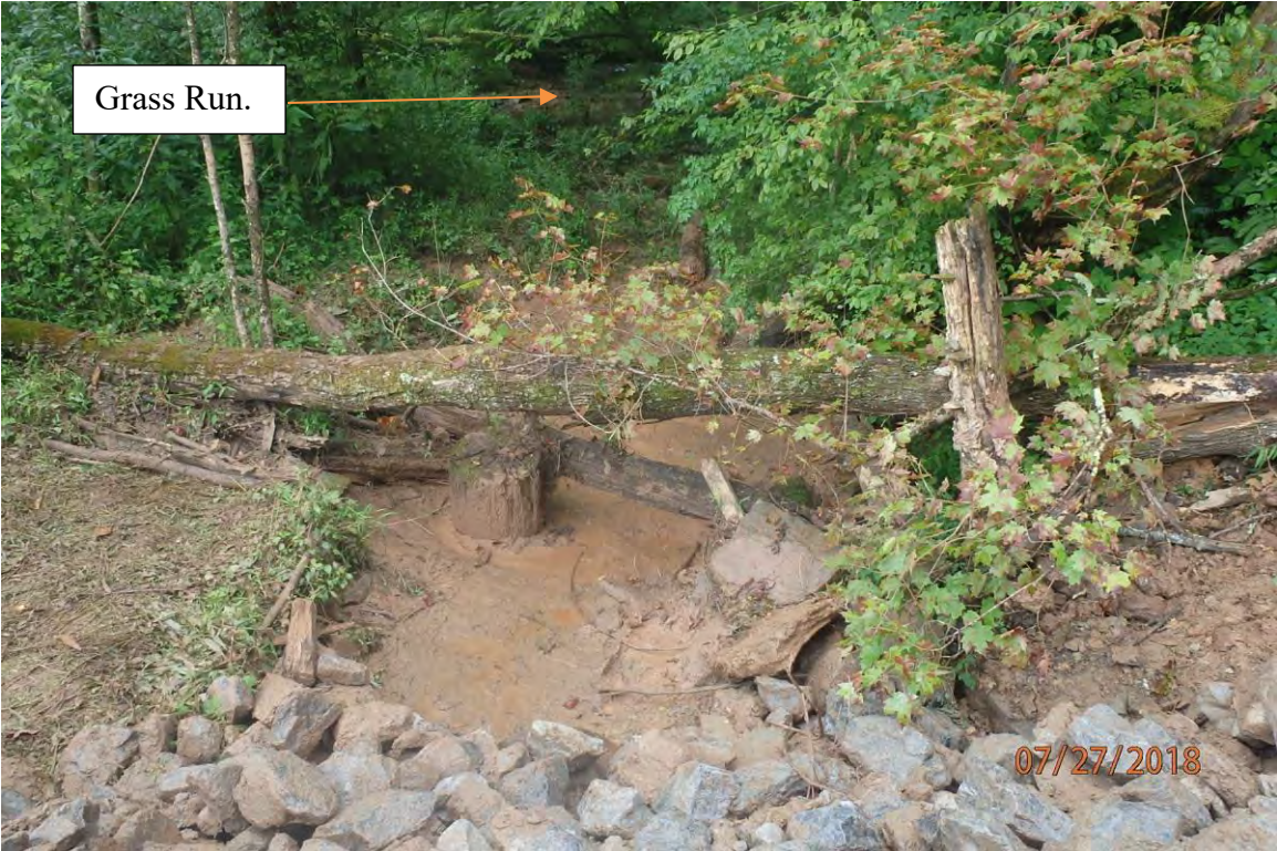
Point where sediment leaves the site. Deficiencies in site evaluation item numbers 15, 19, 20 & 21 pictured.
