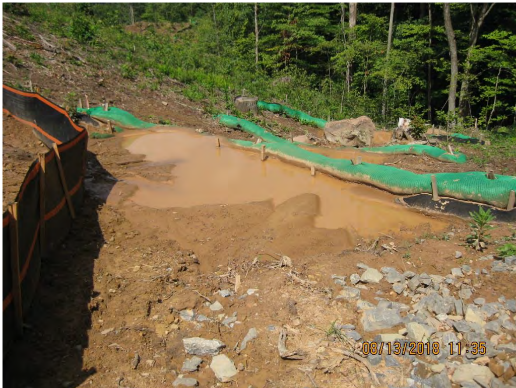
At St. 00+220 a series of perimeter controls used in a concentrated flow area had failed allowing sediment laden water to leave the site.
