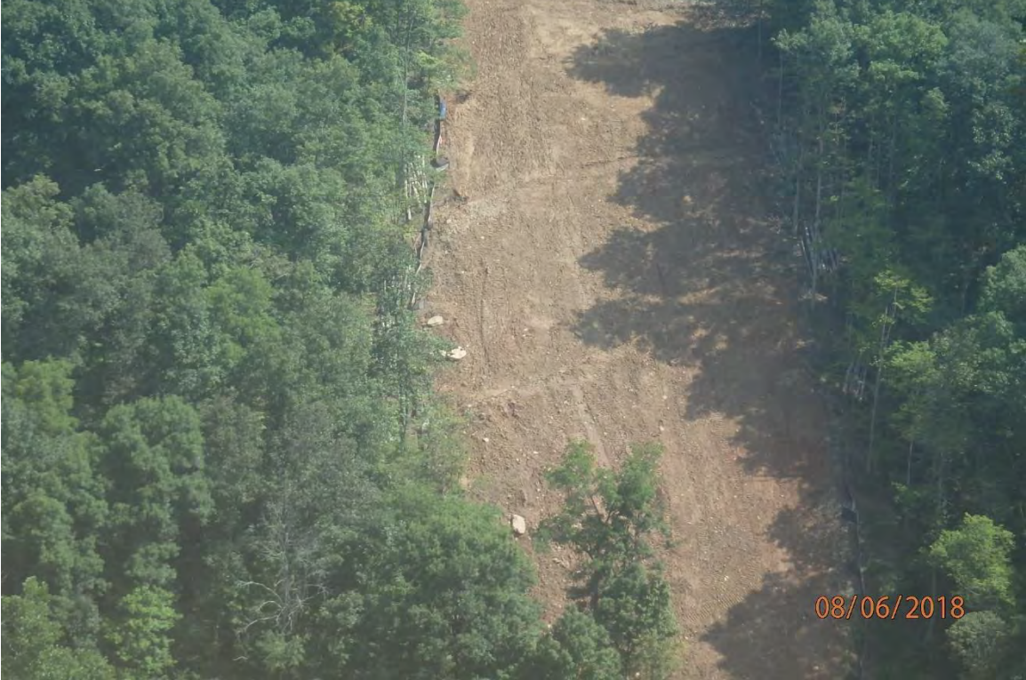
Improperly installed water bars and associated fill slope erosion in the Little Rockcamp Run watershed. Deficiencies in site evaluation item numbers 1, 6, 7, 13, 14, 19 & 21 pictured.
