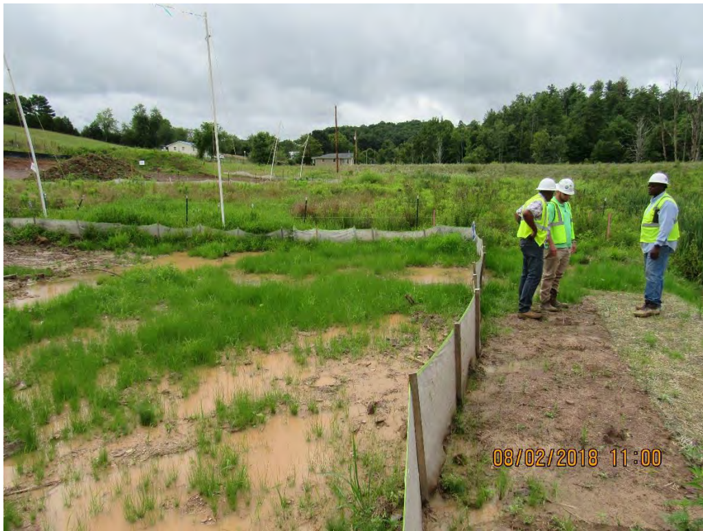
Photo 10: Installed silt fence is retaining sediment laden water
