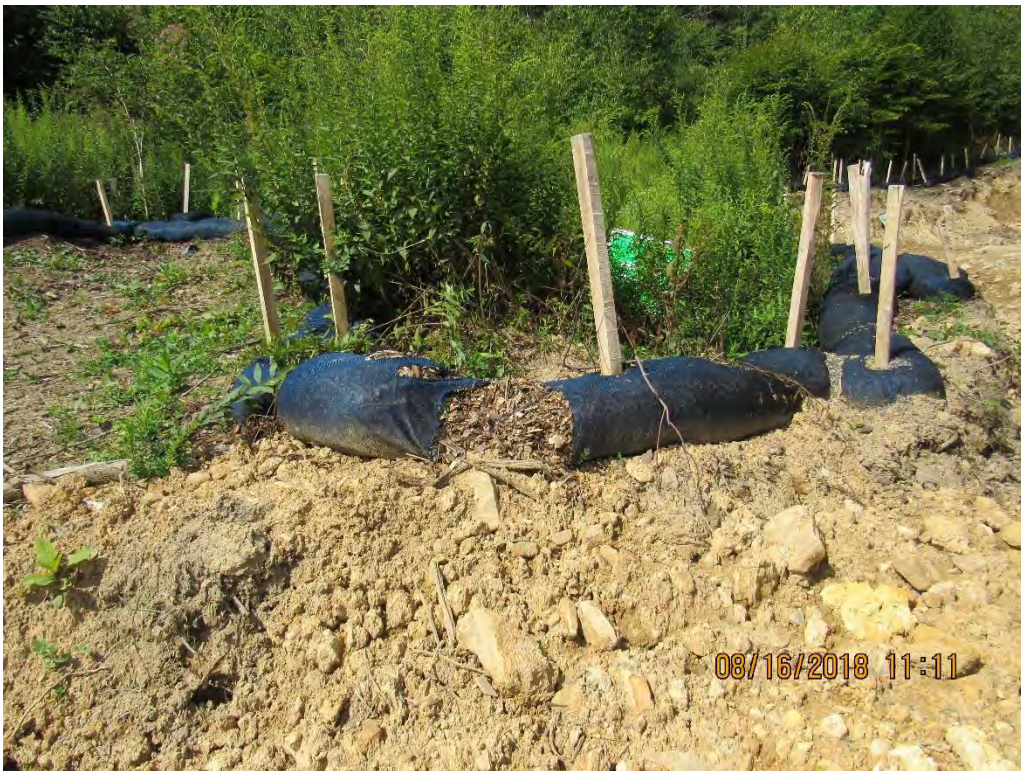
Photo 14: CFS needs maintenance near station 73232+00.
