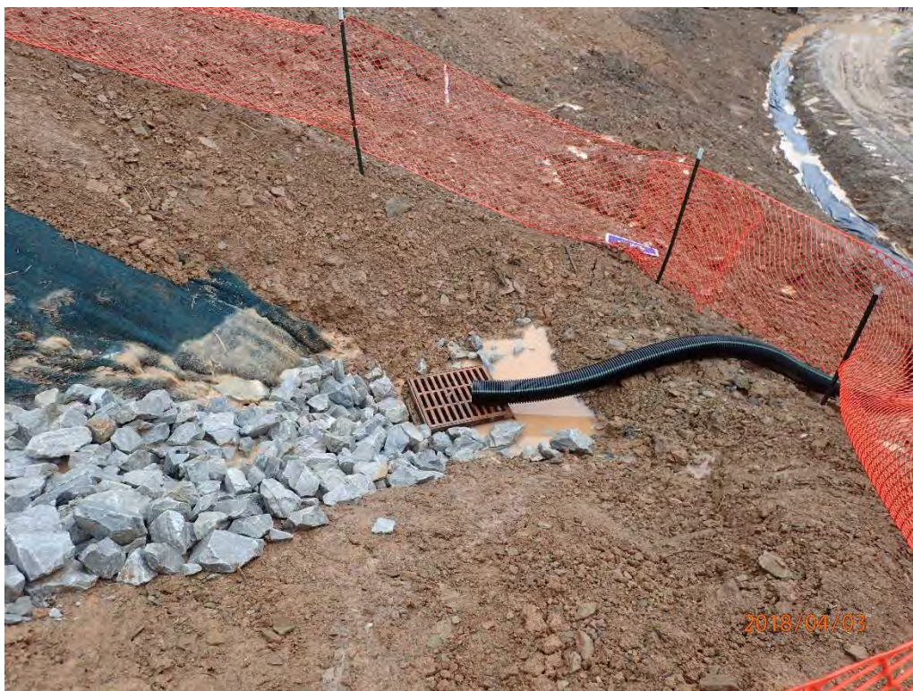
Unprotected drop inlet at Mobley Compressor Station.
