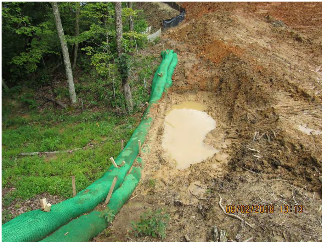
Photo 32: Location of previous failure near station 9961+00.
