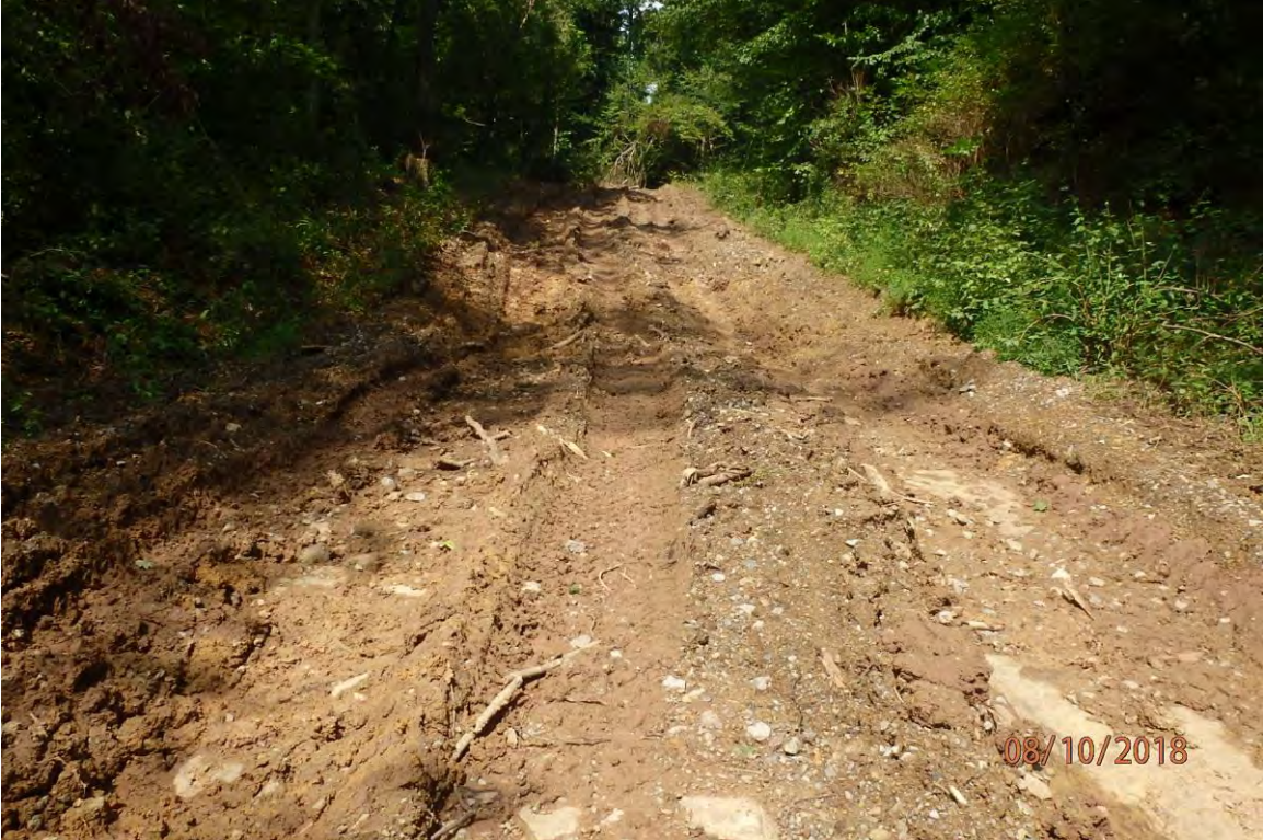
Water bar on access road LE-73.01 in the Sand Fork watershed that has been damaged by the clearing crew (Inactive since FERC permit suspension) and is in need of maintenance. Deficiencies in site evaluation item numbers 6, 7, 8 & 14 pictured.
