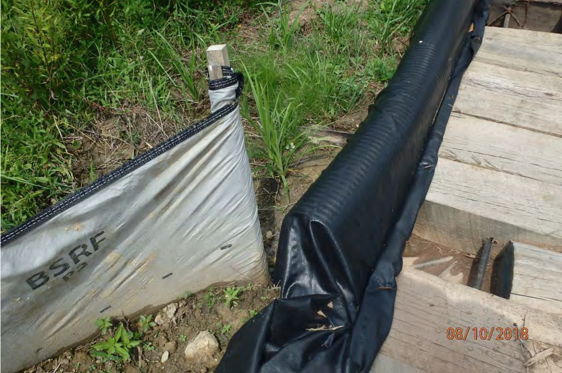
Wetland UNT Left Fork Freemans Creek (W-K31) crossing showing perimeter control not properly tied in to timber mat crossing.
