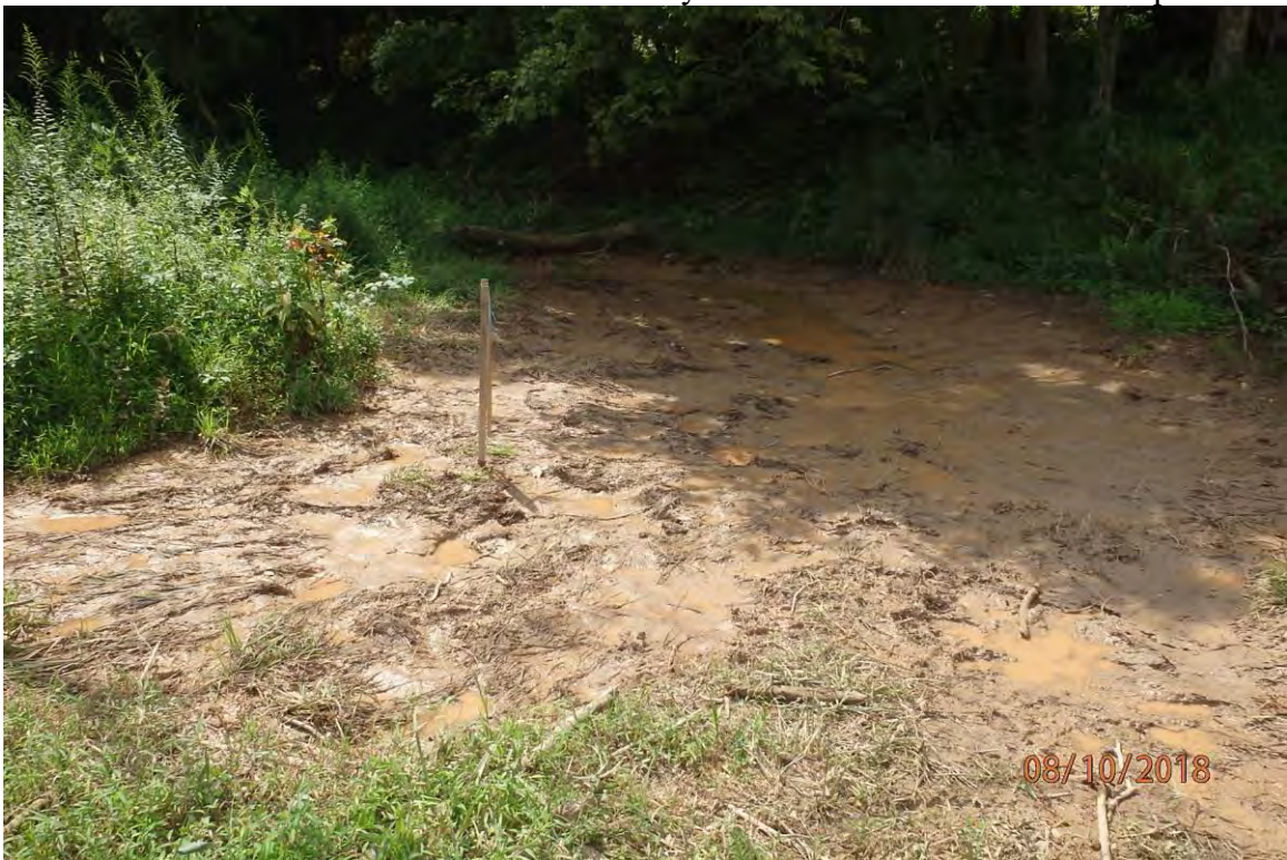
CNA deposits in wetland UNT Smoke Camp Run (W-I26) (39° 08.208' X 80° 34.610') that originate from site. Deficiencies in site evaluation item numbers 6, 7, 8, 14, 19, 20 & 21 pictured.
