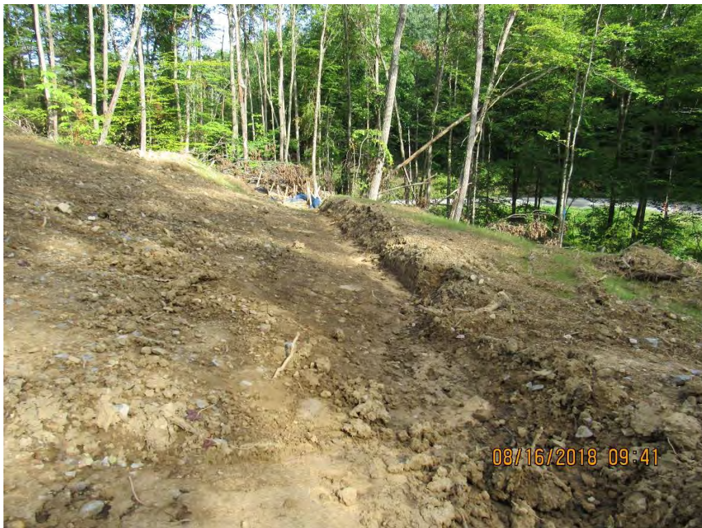
Photo 2: Western view of one of several incorrectly sloped water bars in Photo 1 off Bingham Road station 7450+00.
