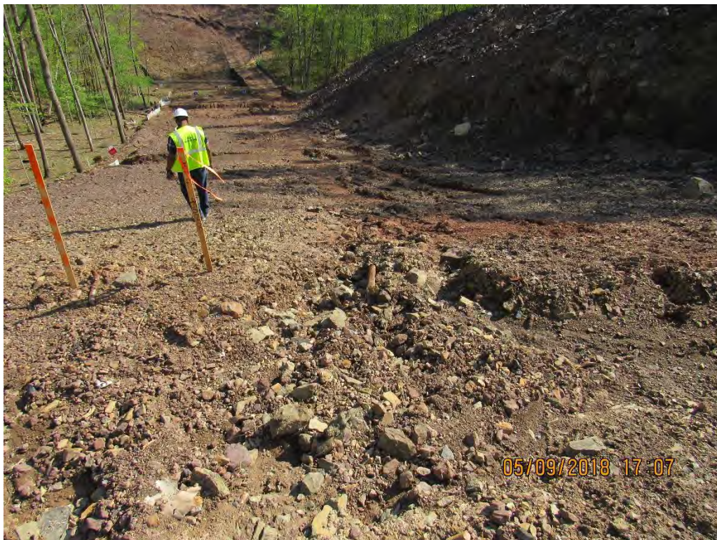
Photo 4: Downslope view of site of sediment laden water left site- erosion gullies observed on slope. (view south)
