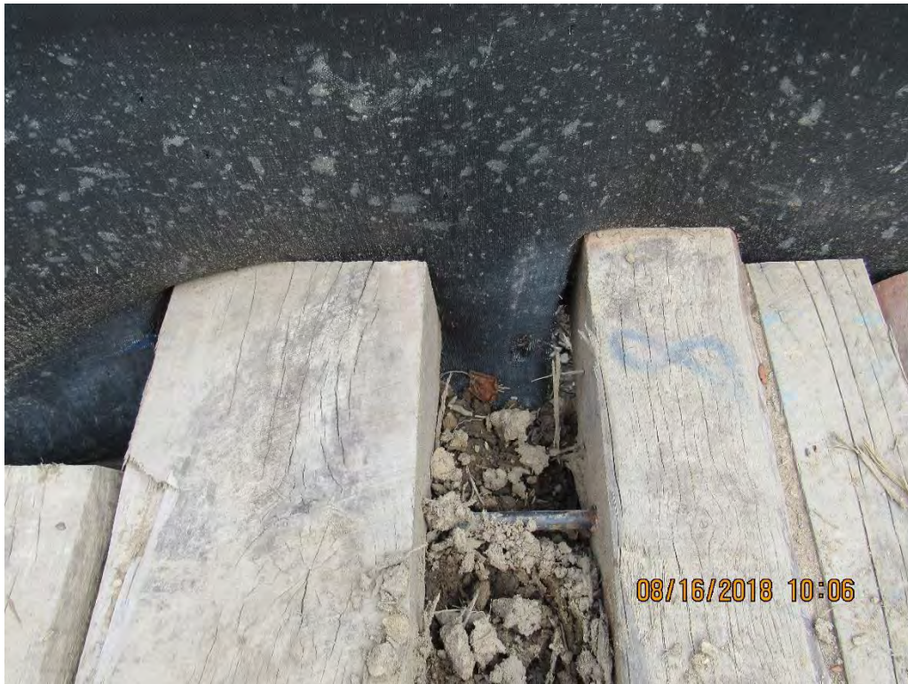
Photo 9: Timber bridge mat punctured filter fabric at station 7465+00.
