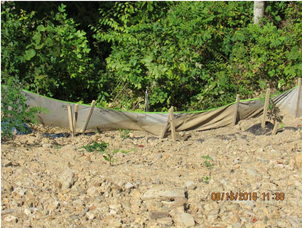
Photo 18: Close-up of inadequate controls for concentrated flow at base of fill slope near station 7158+00.
