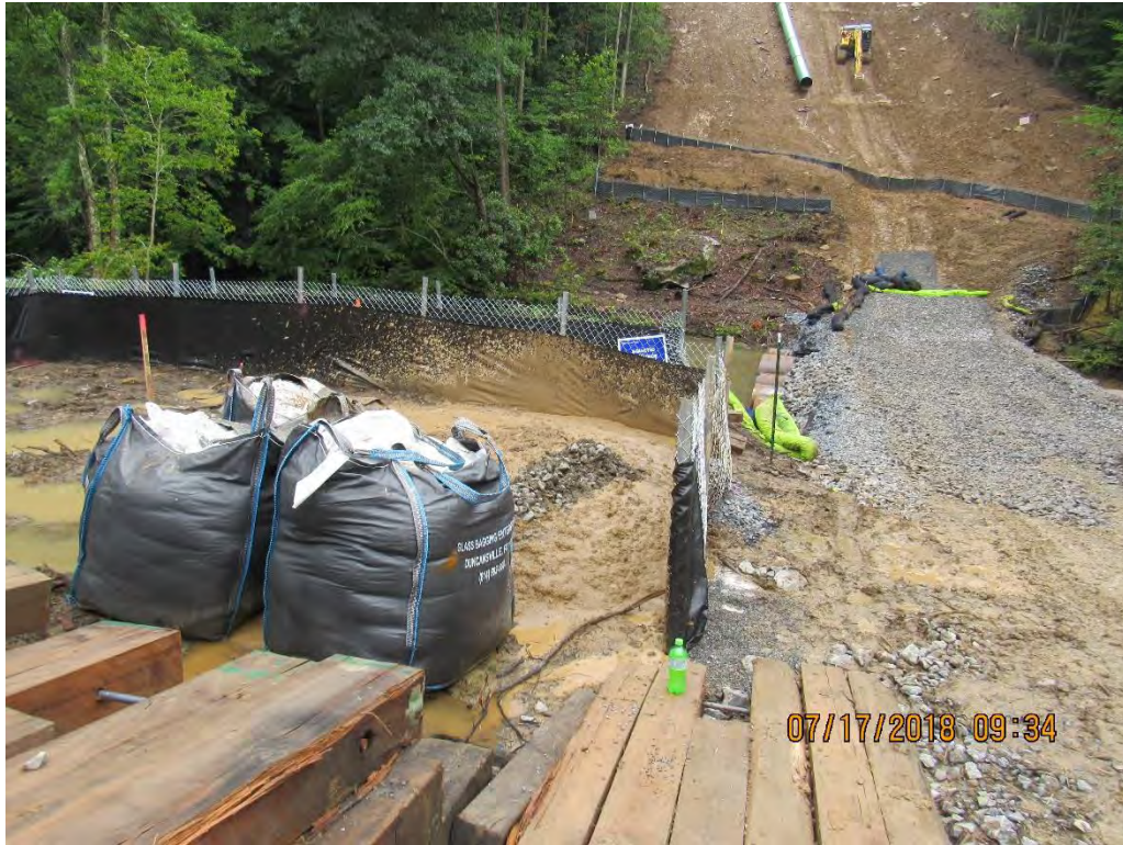
Photo 1: Sump at access road 129 needs maintenance.
