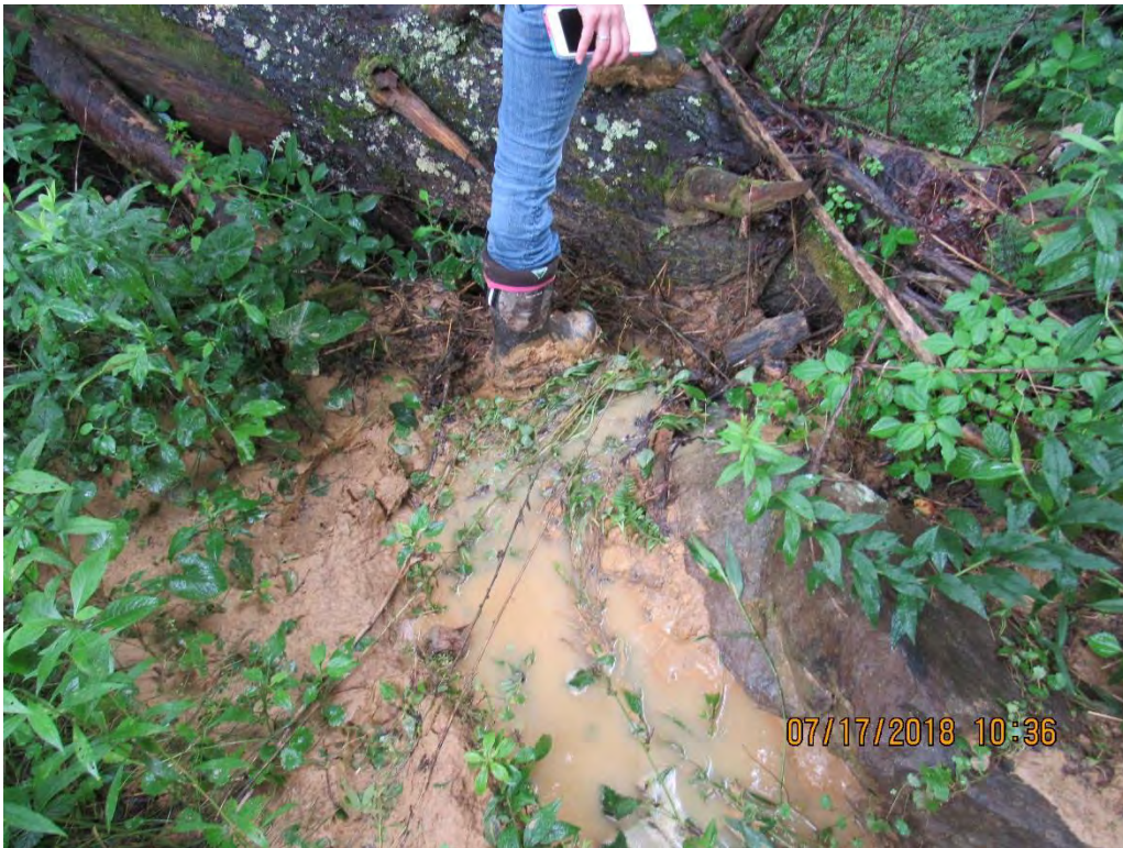
Photo 7: Sediment build up and muddy water temporarily stopped against downed tree.
