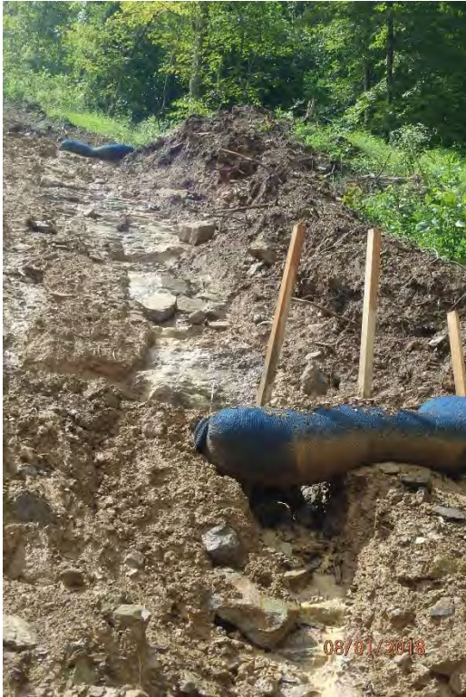
Improperly installed water bars that have caused fill slope erosion in the Big Elk Creek watershed. Deficiencies in site evaluation item numbers 6, 7, 8, 14, 19, 20 & 21 pictured.
