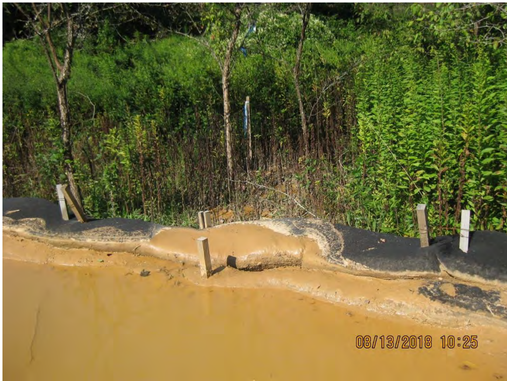
At St. 00+400 Sediment laden water left the site in three locations as a result of the lack of fill slope protection and the use of perimeter controls in an area of concentrated flow for a large drainage area that requires a sized trapping structure.
