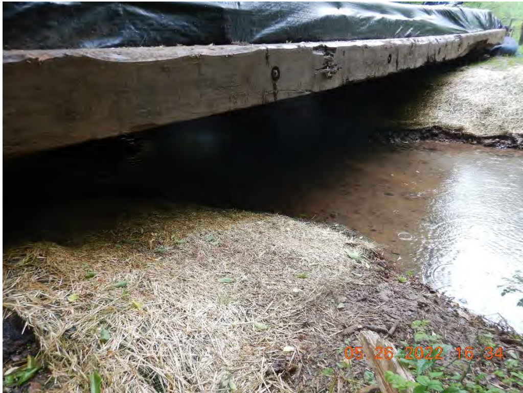
This is a photo showing the air bridge that was installed by the company. The company removed the flumes from the stream to prevent future instances of sandbags and stone from washing downstream.
