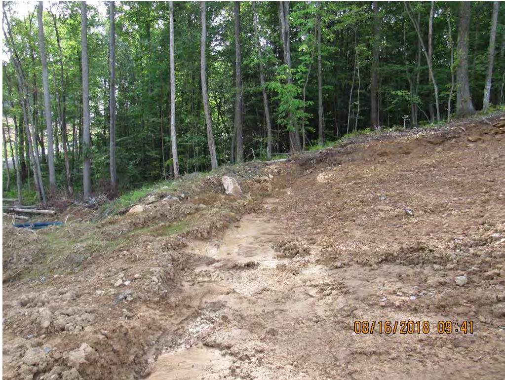
Photo 1: Eastern view of one of several incorrectly sloped water bars off Bingham Road station 7450+00.
