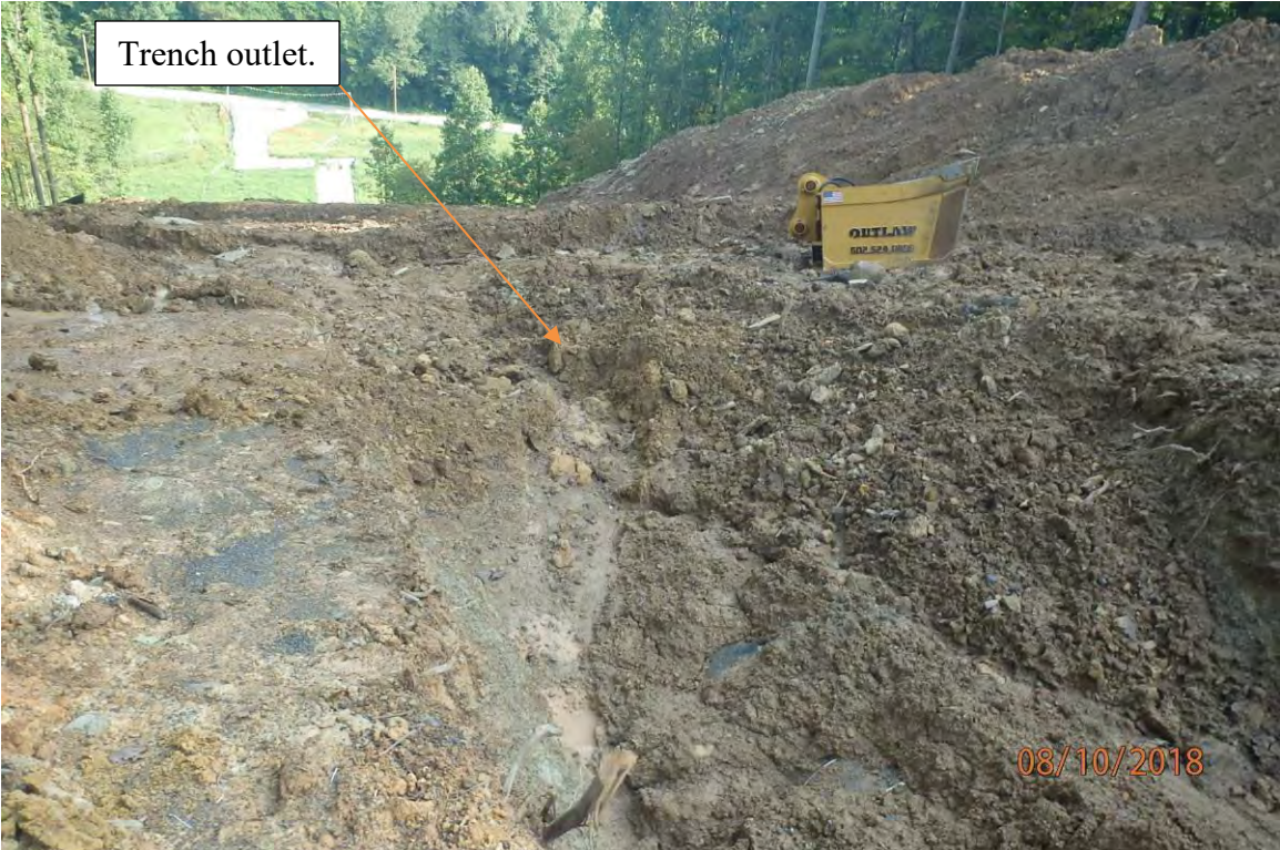
Issues with water bars that discharge into the pipe trench causing fill slope erosion. Deficiencies in site evaluation item numbers 2, 6, 8, 14, & 21 pictured.
