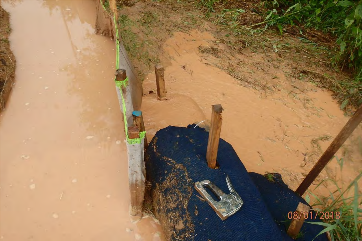
Improperly operated BMP that is causing sediment laden water to leave the site and CNA visible in Big Elk Creek. Deficiencies in site evaluation item numbers 1, 6, 19, 20 & 21 pictured.
