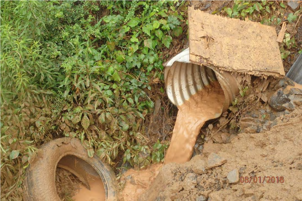
Sediment laden water that is bypassing the installed BMPs due to improper BMP operation and installation. Deficiencies in site evaluation item numbers 1, 6, 7, 13, 14, 19, 20 & 21 pictured.
