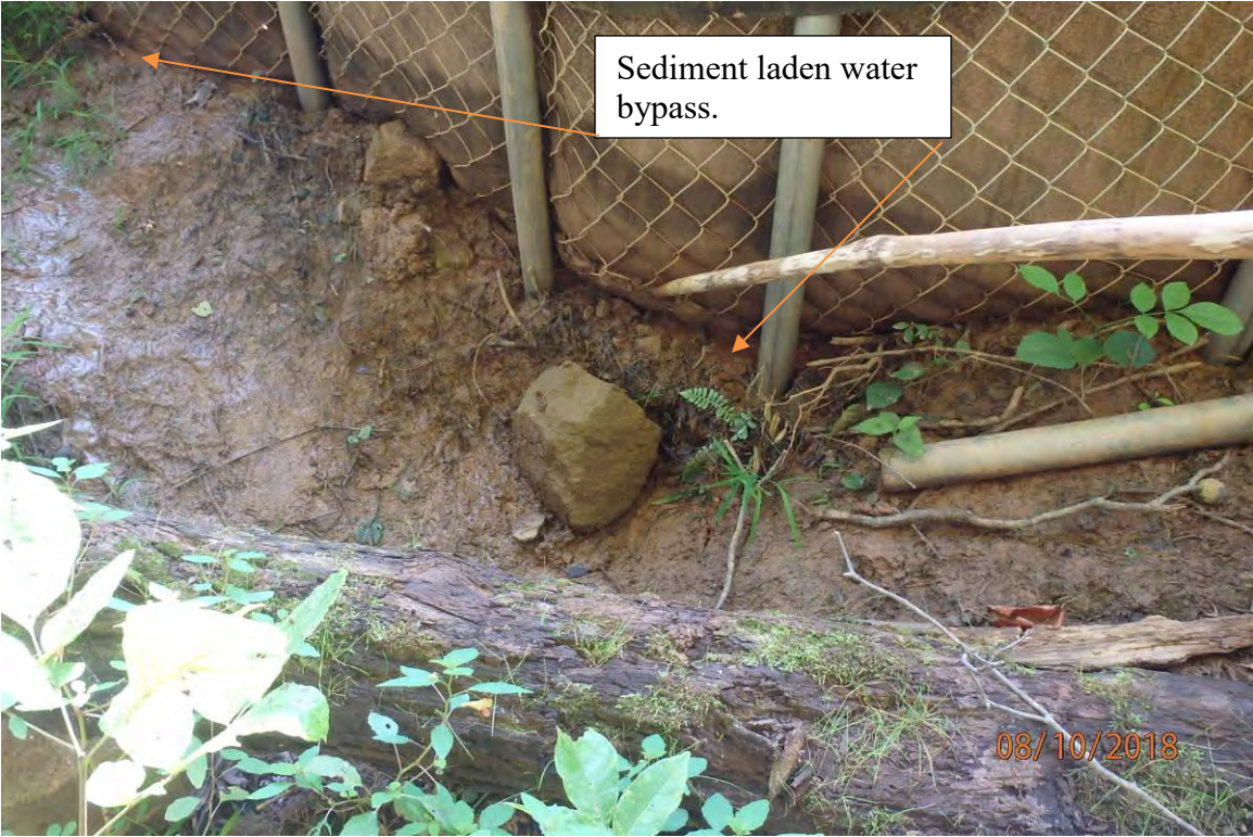
Improperly operated and maintained BMP at a water bar terminus in the Meathouse Fork watershed that led to CNA deposits and distinctly visible settleable solids in UNT Meathouse Fork (39° 11.891' X 80° 33.209'). Deficiencies in site evaluation item numbers 6, 7, 19, 20 & 21 pictured.
