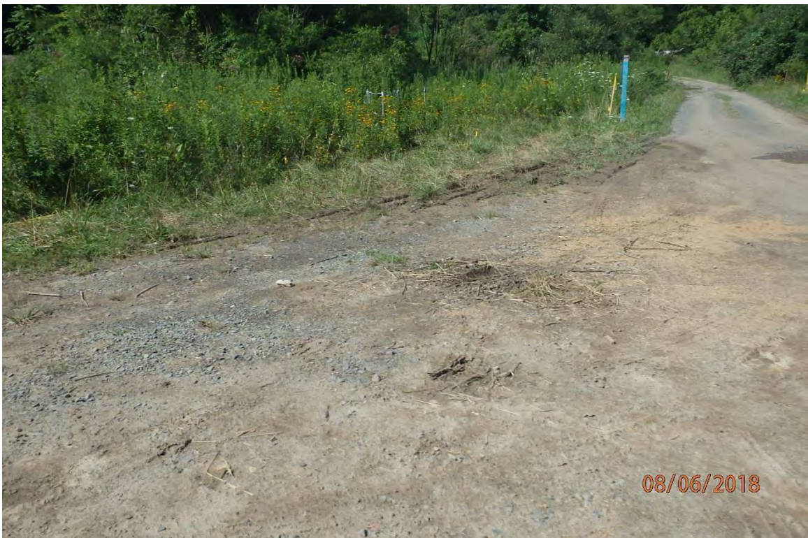
Area adjacent to wetland (W-UU1) in the Salem Fork watershed that lacks the BMPs that are indicated in the approved SWPPP. Marginal deficiencies in site evaluation item numbers 1, 13, 15, 19 & 21 pictured.
