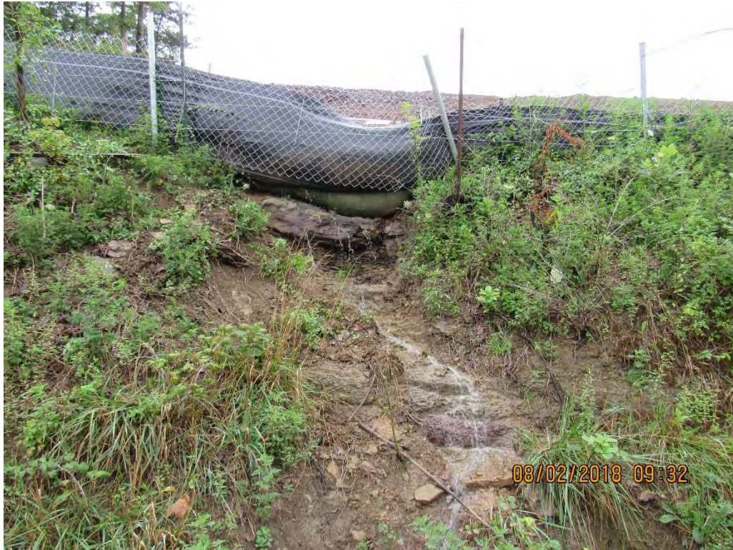
Photo 1: Clear discharge from water bar near station 9087+17.
