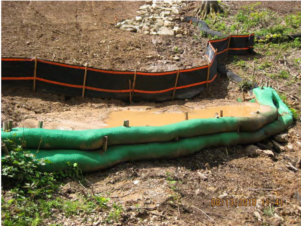
Maintenance needed north of the east wall.
