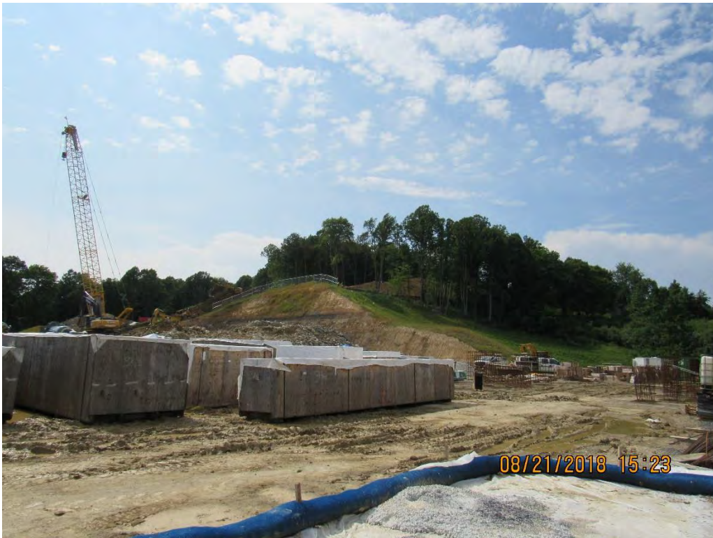
Photo 3: Slope on northwest side of site which has not been reseeded.
