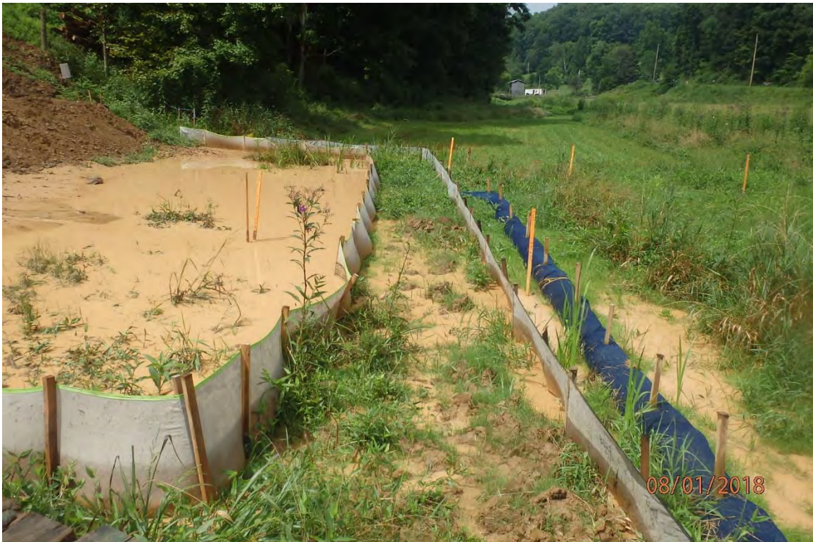
Perimeter controls adjacent to Big Elk Creek that are overwhelmed due to improperly installed water bars.
