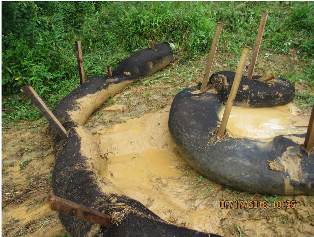
Photo 5: Next set of compost filter sock in sequence which was overtopped allowing sediment laden water to leave site.
