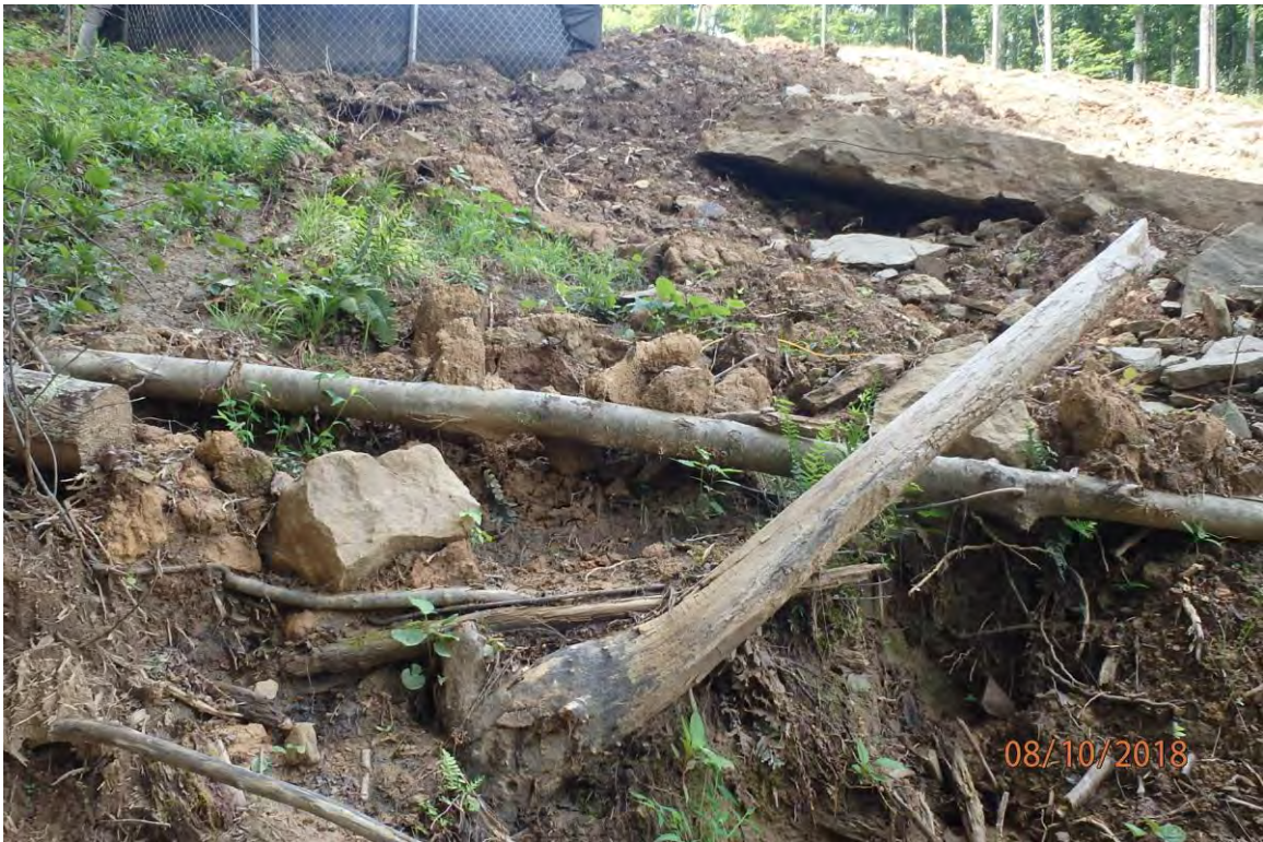
Water bar terminus BMP that was previously overwhelmed and led to CNA deposits pictured below. Water bar was altered to shed stormwater away from this area at the time of inspection.
