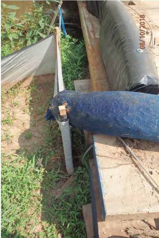
Sand Fork (S-163) crossing showing perimeter control not properly tied in to timber mat crossing. Marginal deficiencies in site evaluation item numbers 1, 19 & 21 pictured.
