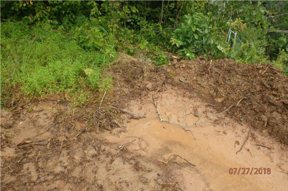
Water bar that lacked outlet protection was noted upslope of grass run adjacent to 1142+00. Marginal deficiencies in site evaluation item numbers 7, 15, 19 & 21 pictured.
