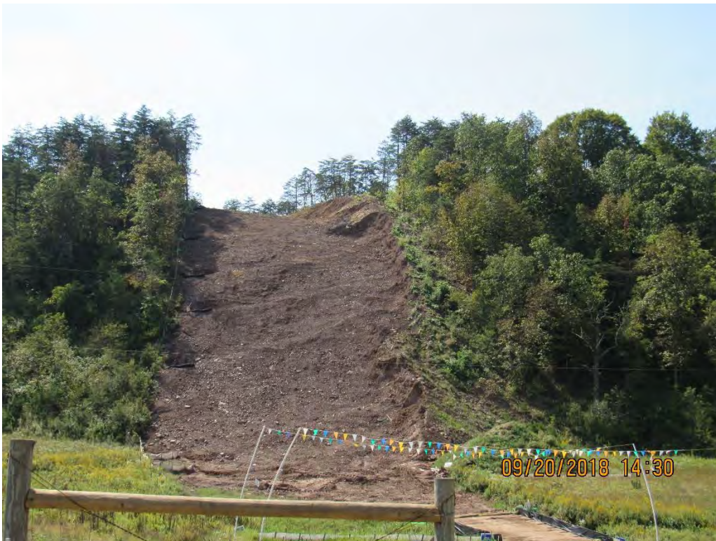
Photo 12: Wayside/Talcott near station 9466+16. Final restoration scheduled within a few weeks, weather depending.
