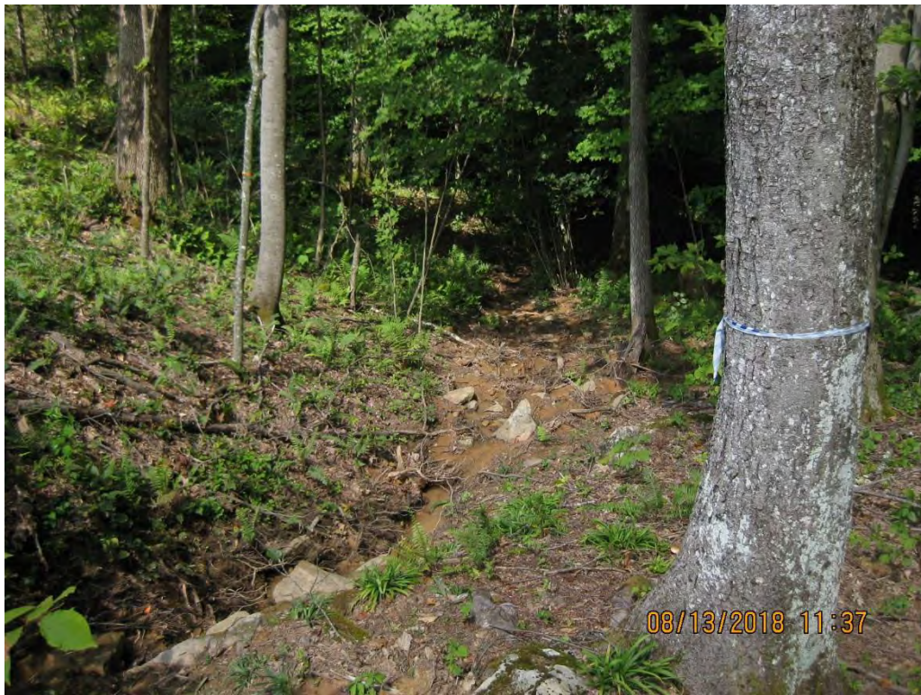
At St. 00+220 a series of perimeter controls used in a concentrated flow area had failed allowing sediment laden water to leave the site. Sediment deposits were noted in receiving stream A-104 creating Conditions Not Allowable in the Waters of the State.
