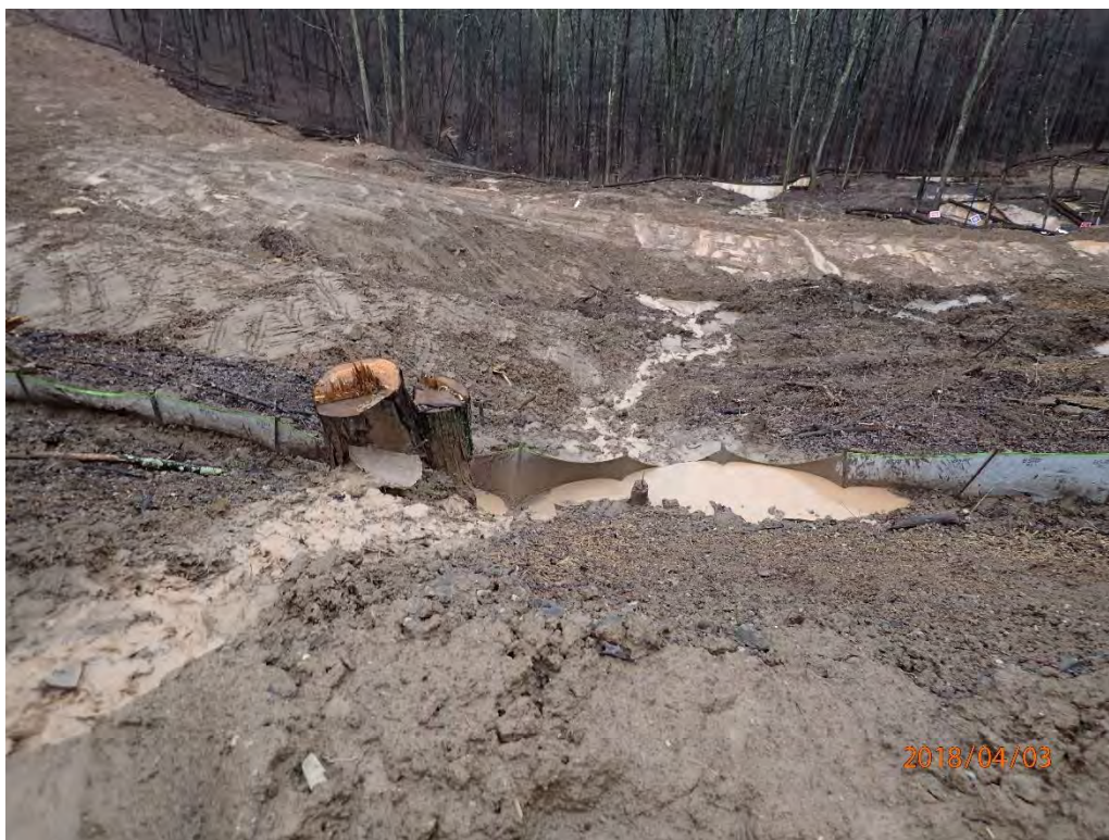
Concentrated flow eroding slope near slip.
