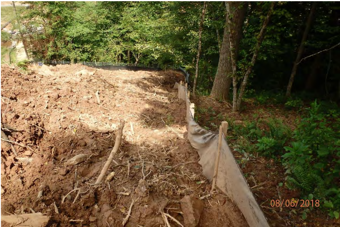
Concentrated flow being directed over fill slope into a sheet flow super silt fence from improperly installed water bars in Grass Run.
