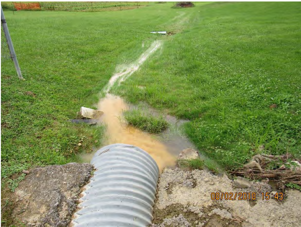
Photo 34: Sediment laden water from unknown source near Lindsie Methodist Church.
