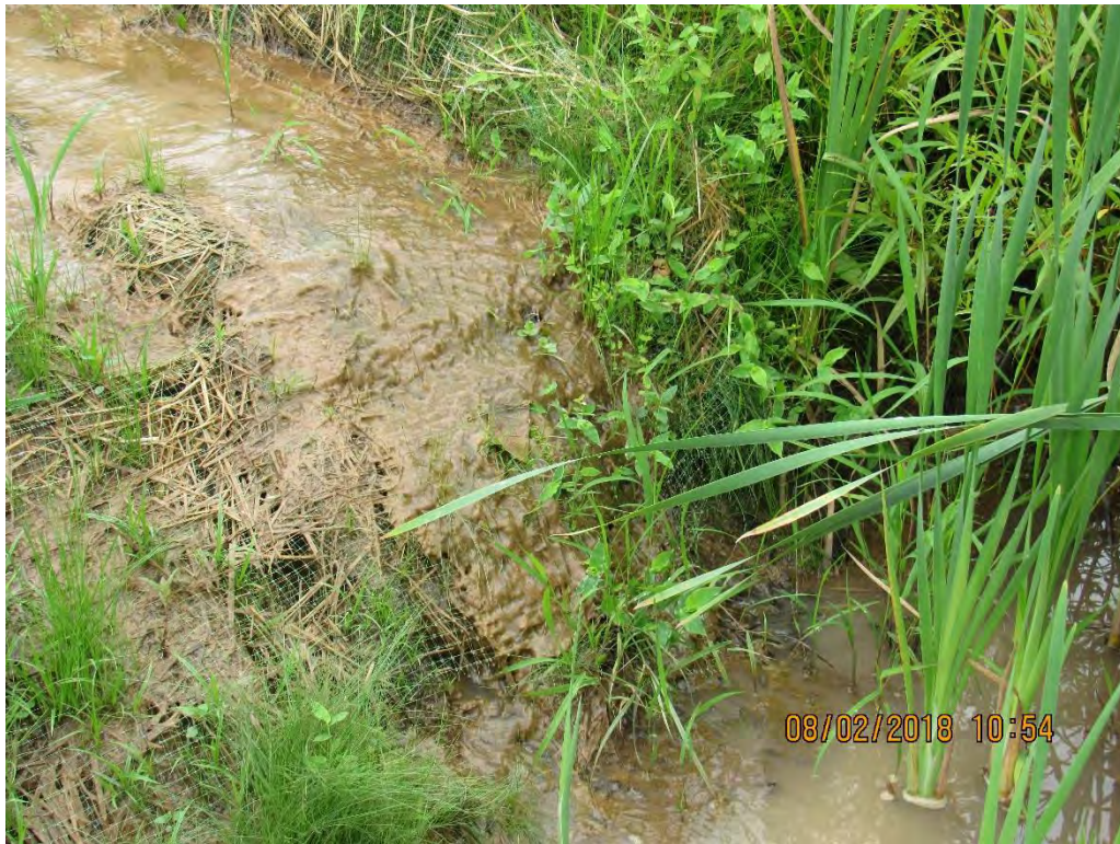
Photo 13: Sediment has been deposited on bank protection product, which is being picked back up prior to entering stream
