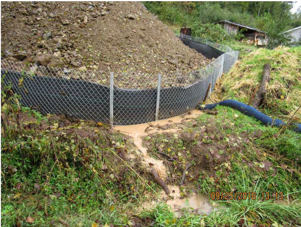
Photo 3: Failure of perimeter controls near 3634+00 allowing sediment laden water to leave site.
