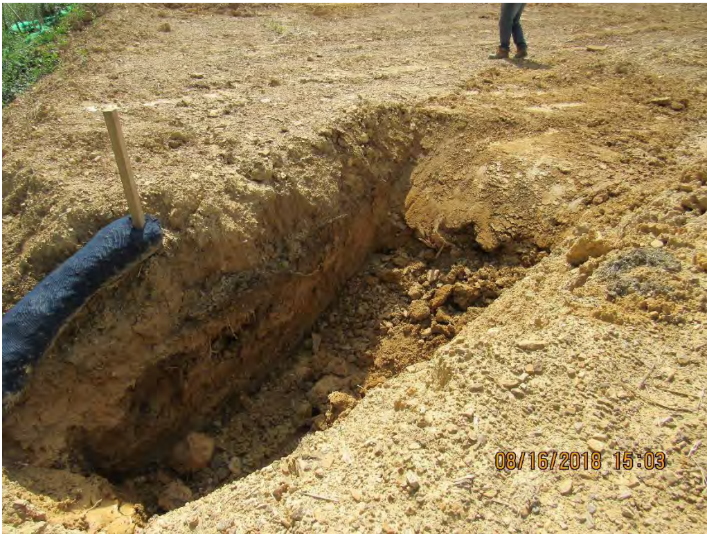
Photo 31: Sumps installed at terminus of water bars near Wahoo Road station 6781+51 which has reduced failure.
