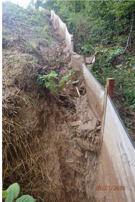
Concentrated flow being channeled along perimeter control trench due to improperly installed water bars in the Goose Run watershed.
