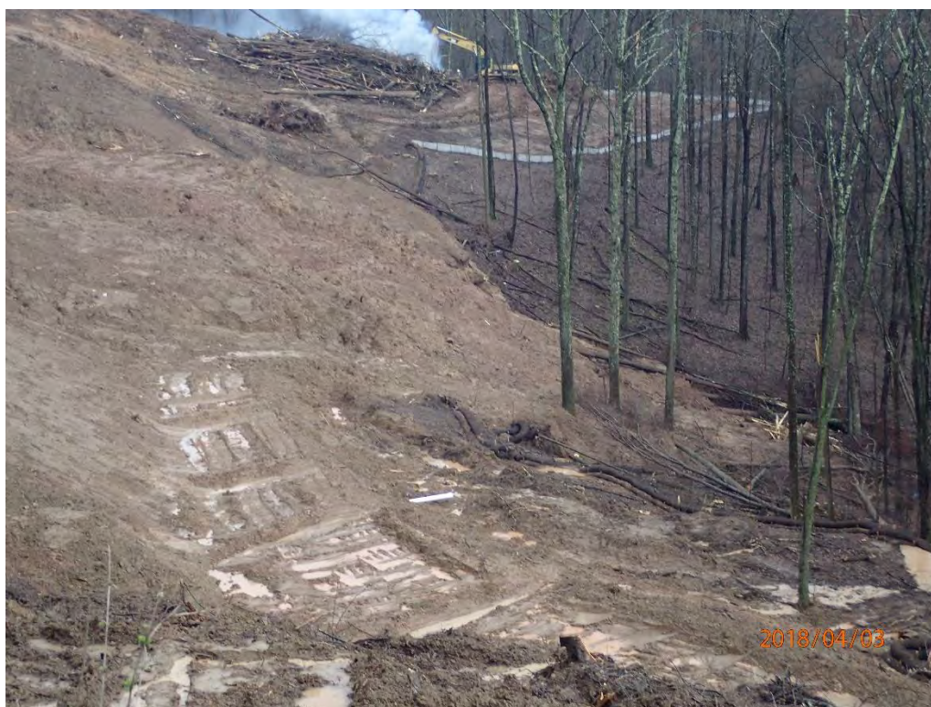
Reported slip area near Bradshaw Compressor Station.
