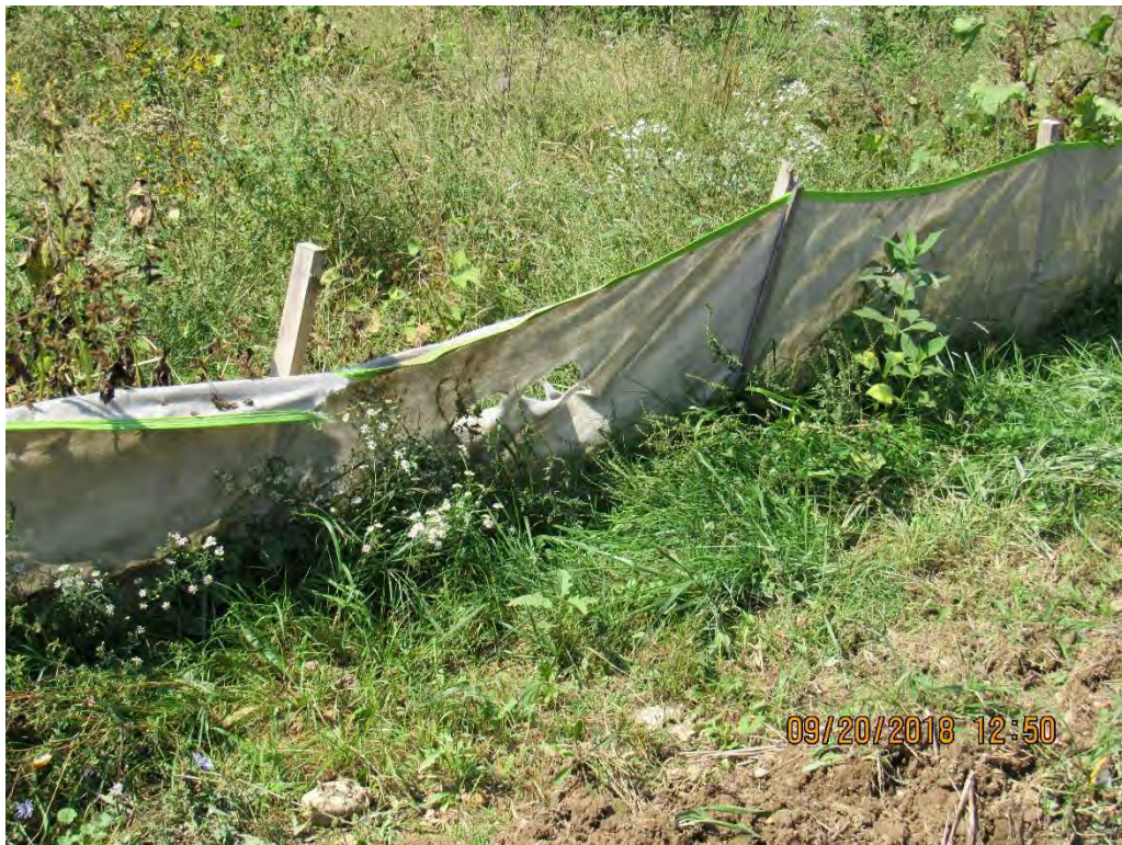
Photo 2: Silt fence needs replaced along access road 231.01 off Painters Run Road near station 10270+49.
