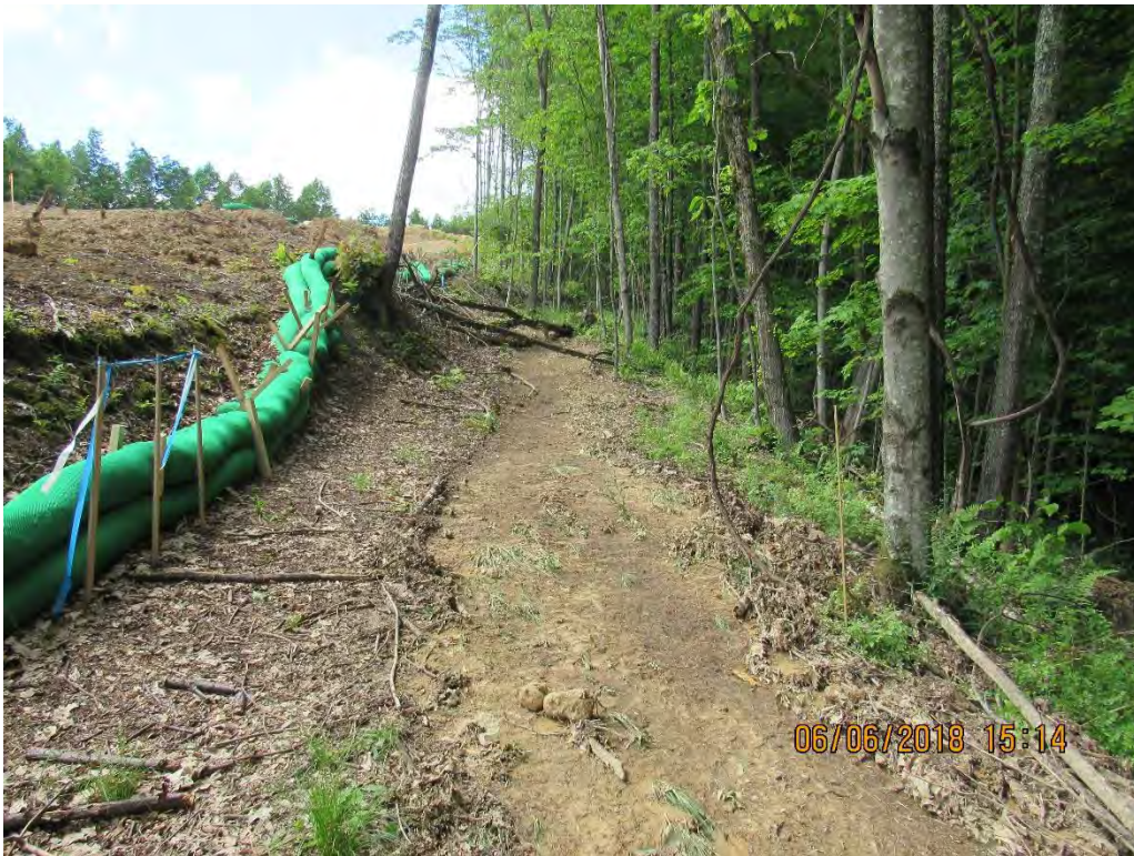
Photo 5: Scoured path from control failure at station 6812+58.
