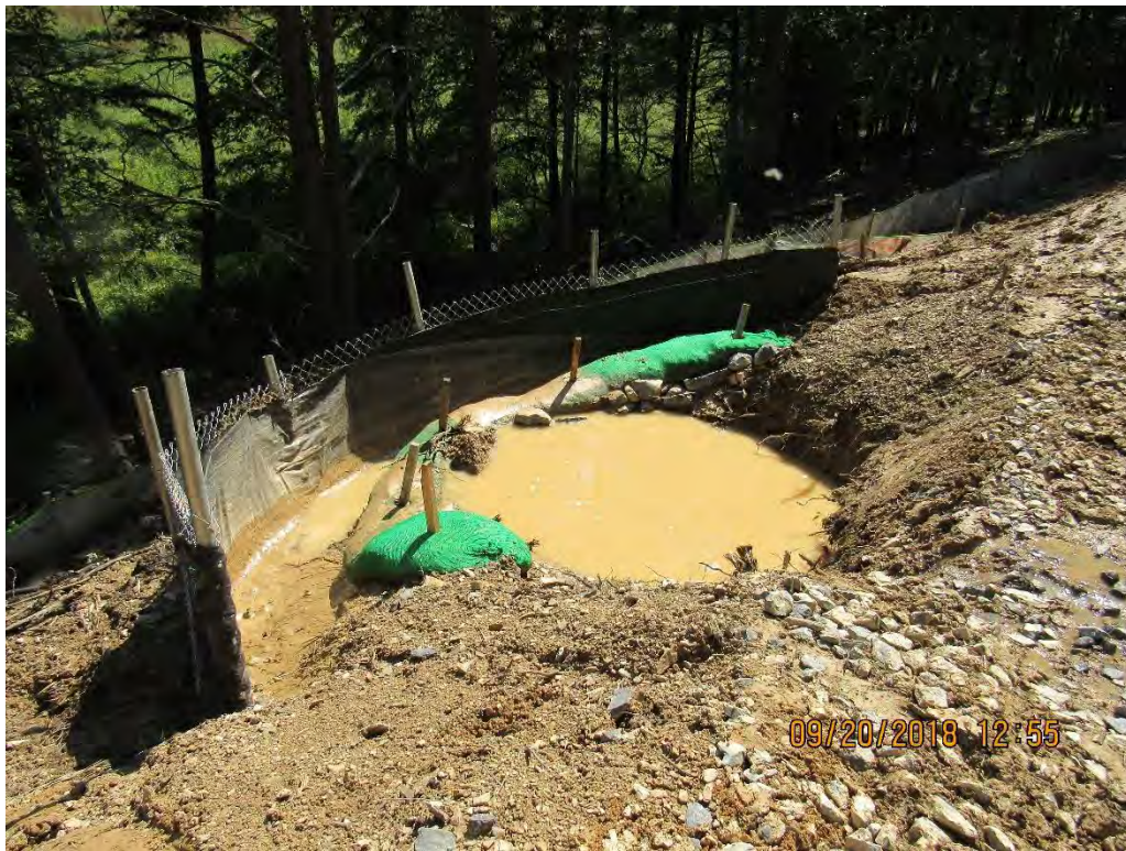
Photo 4: Sump above control failure off access road 231.01 near station 10270+49 Painters Run.
