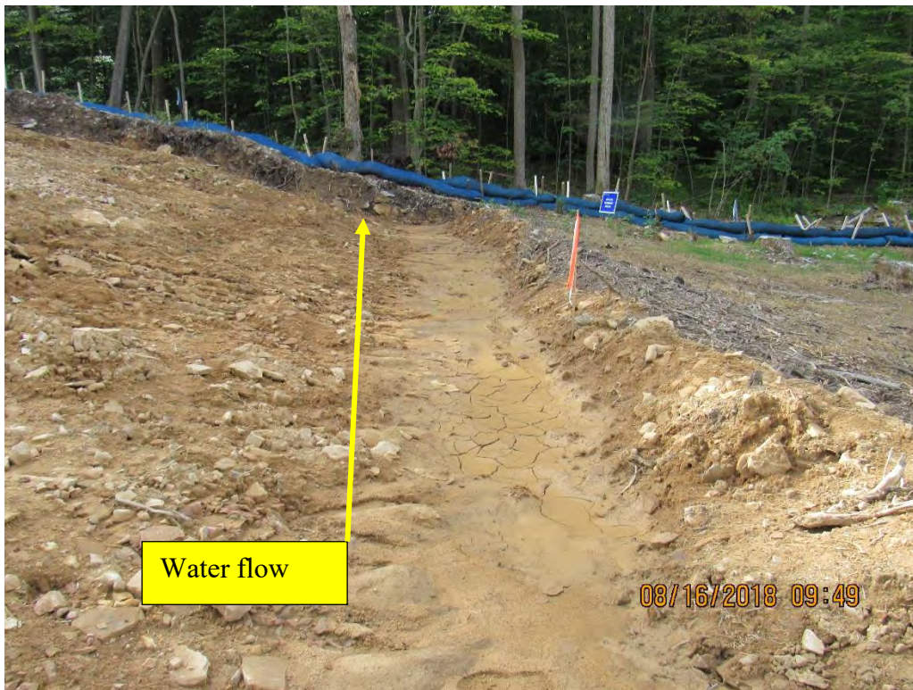
Photo 3: Incorrectly sloped water bar at Bingham Road station 7450+00- water is flowing away from outlet.
