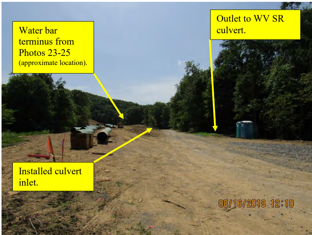
Photo 28: Relative distance of failed water bar terminus, culvert inlet and SR culvert outlet.
