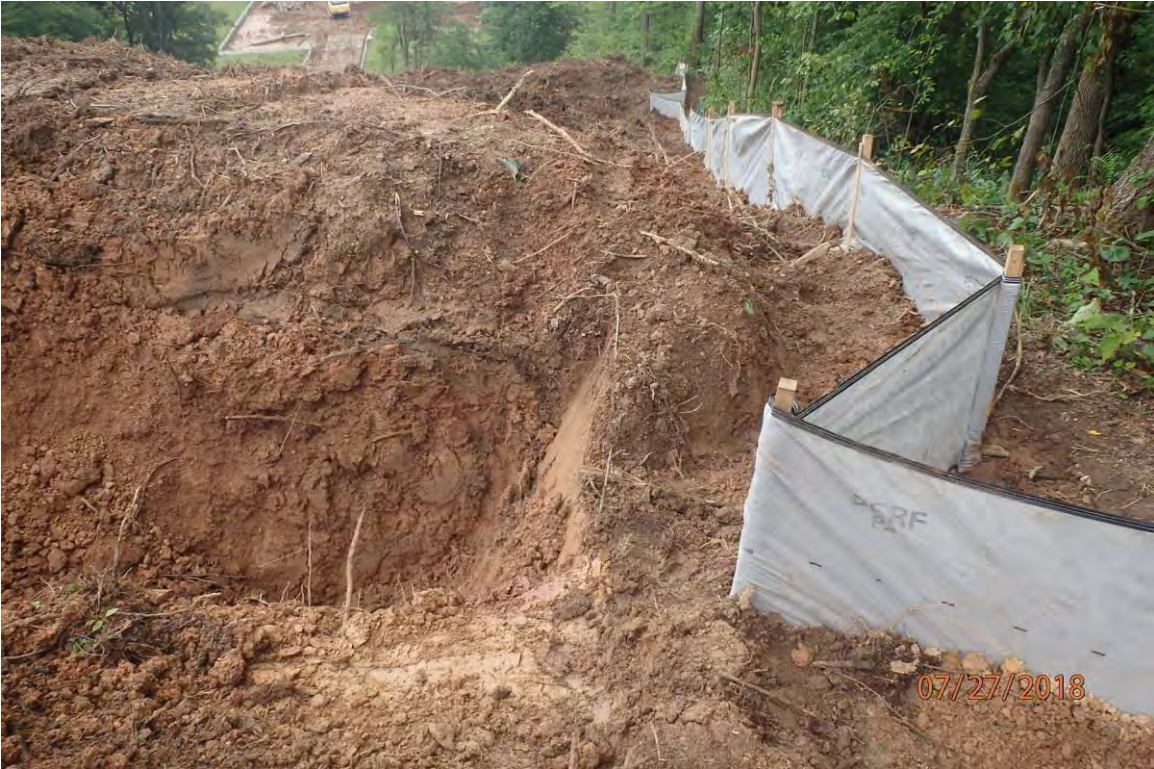
Improperly installed water bars that do not shed stormwater off site as designed. Deficiencies in site evaluation item numbers 7, 14, & 21 pictured.
