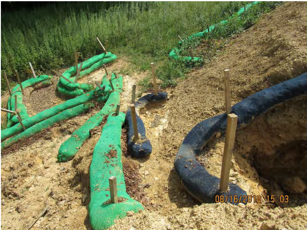
Photo 32: Site of historical water bar terminus control failure- sump installed has reduced failure.
