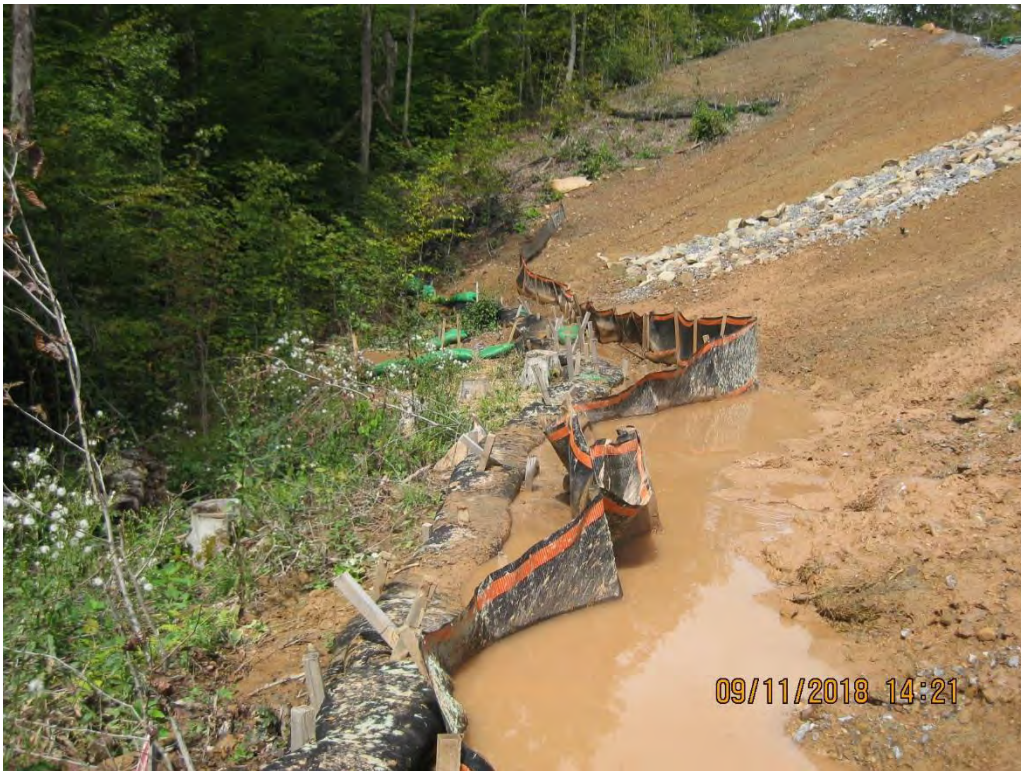
Photo 7: Station 900 (approximately) -Flow along silt fence from culvert outlet downslope to sump.
