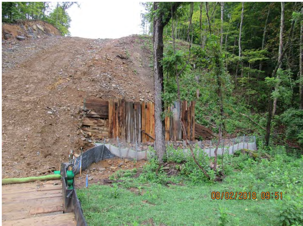
Photo 6: Large sump at end of water bar behind vertical mats.
