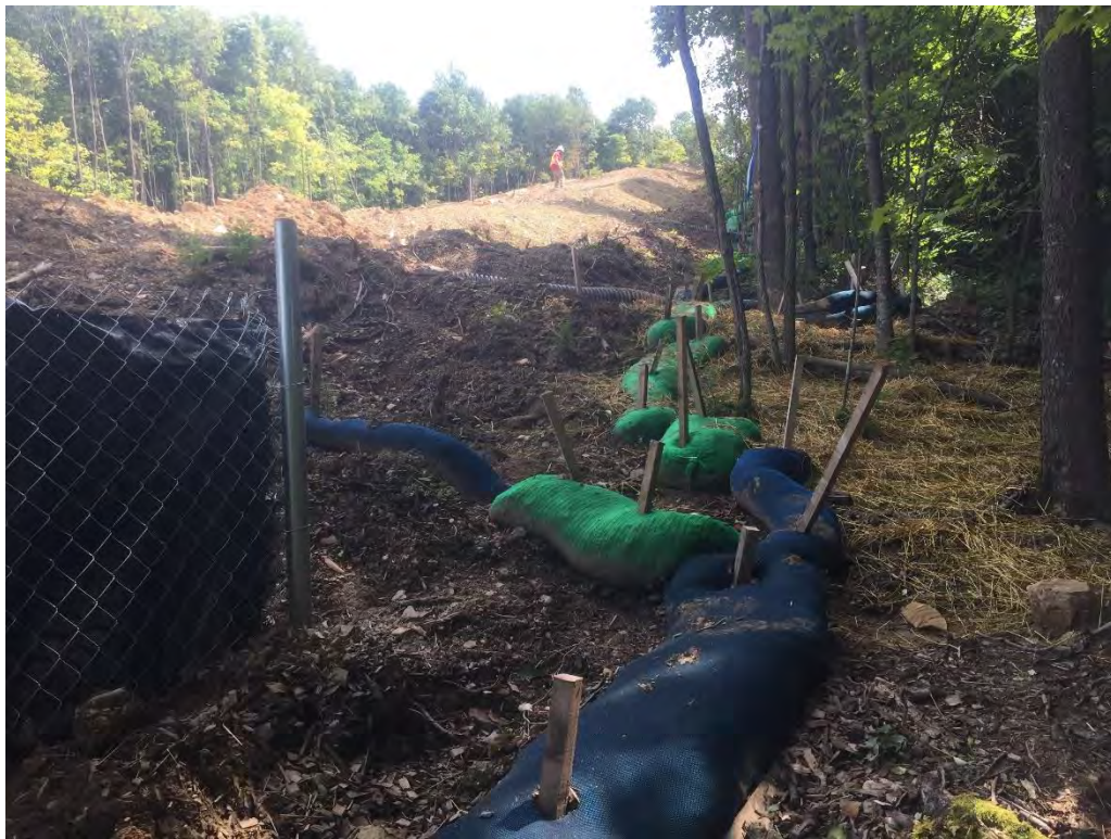
Photo 22: Failure of installed water bars between stations 7084+00 – 7093+50.
