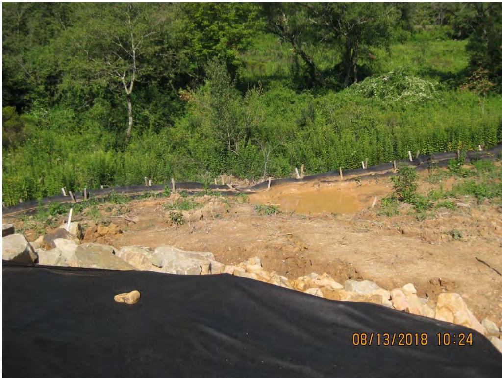
At St. 00+400 Sediment laden water left the site in three locations as a result of the lack of fill slope protection and the use of perimeter controls in an area of concentrated flow for a large drainage area that requires a sized trapping structure.
