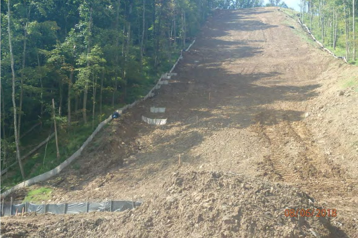
Improperly installed water bars and associated fill slope erosion in the Tenmile Creek watershed.
