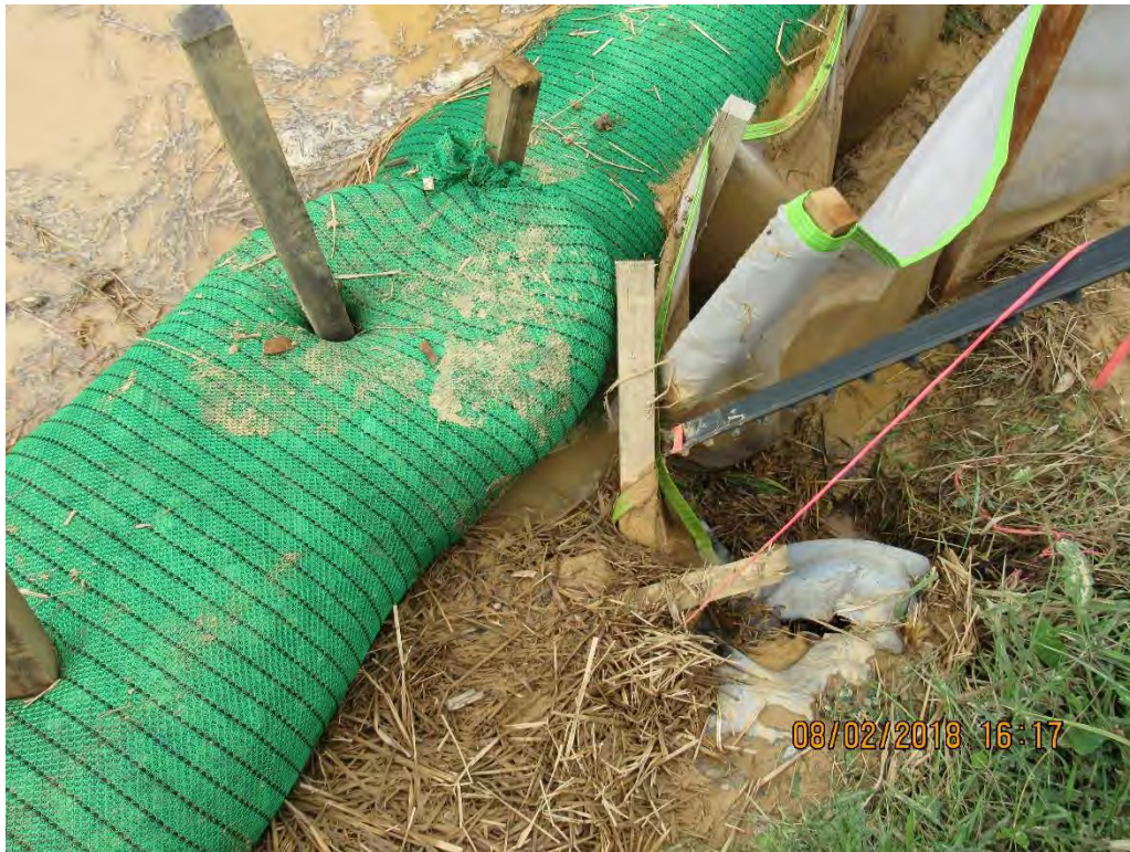
Photo 37: Sediment laden water entering culvert.
