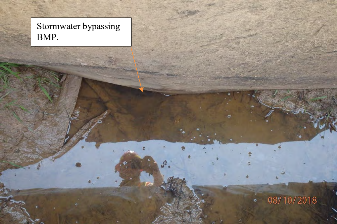
Improperly operated and maintained perimeter controls adjacent to the WJ-40 crossing led to offsite sediment deposits and CNA deposits in Wetland UNT Kincheloe Creek (WJ-40) (39° 10.060' X 80° 34.626'). Deficiencies in site evaluation item numbers 1, 6, 19, 20 & 21 pictured.
