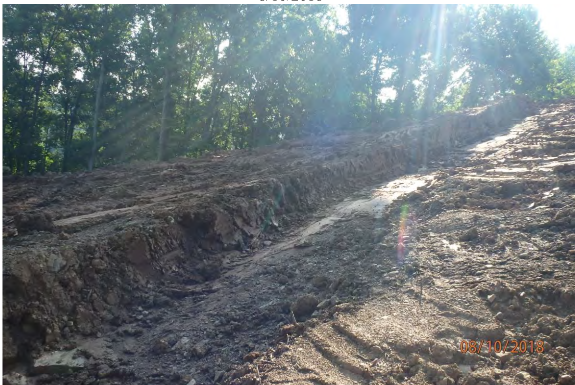
Water bar installed at a steep angle in the Meathouse Fork watershed.
