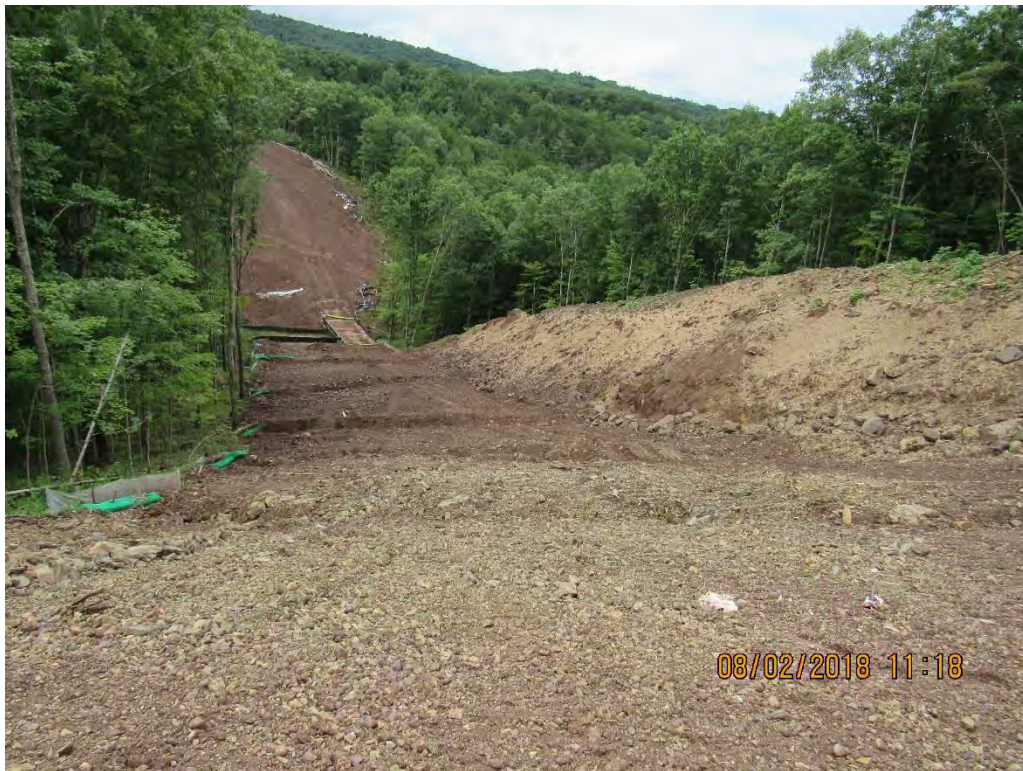
Photo 16: War Ridge Pipe installed across UNT of Little Stony Creek with restoration expected within a week. Crossing has good start on vegetation growth and controls are in good condition.
