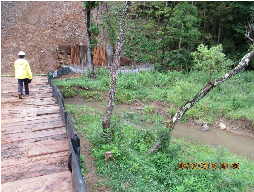
Photo 8: Downstream of installed bridge with sump behind vertical mats in back ground.
