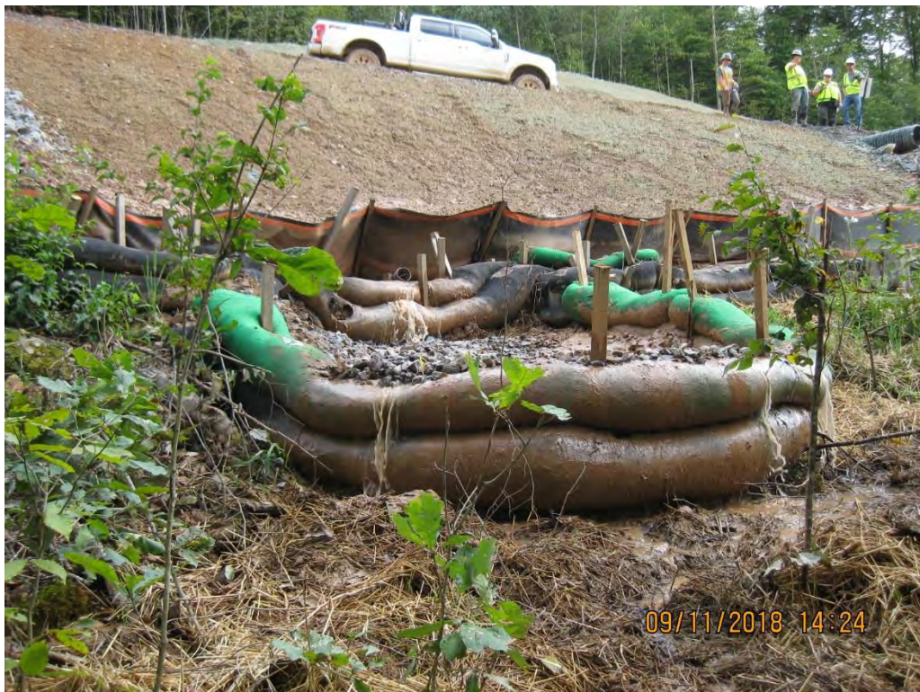
Photo 10: Station 900 (approximately)- upslope view of controls and sediment laden water leaving site.
