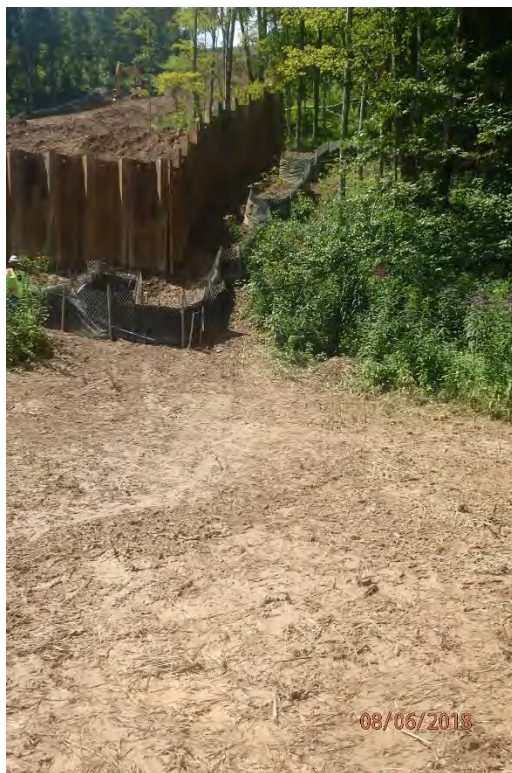
Offsite sediment deposits associated with the overwhelmed BMP at Rockcamp Run. Deficiencies in site evaluation item numbers 1, 2, 6, 7, 8, 13, 14, 19 & 21 pictured.
