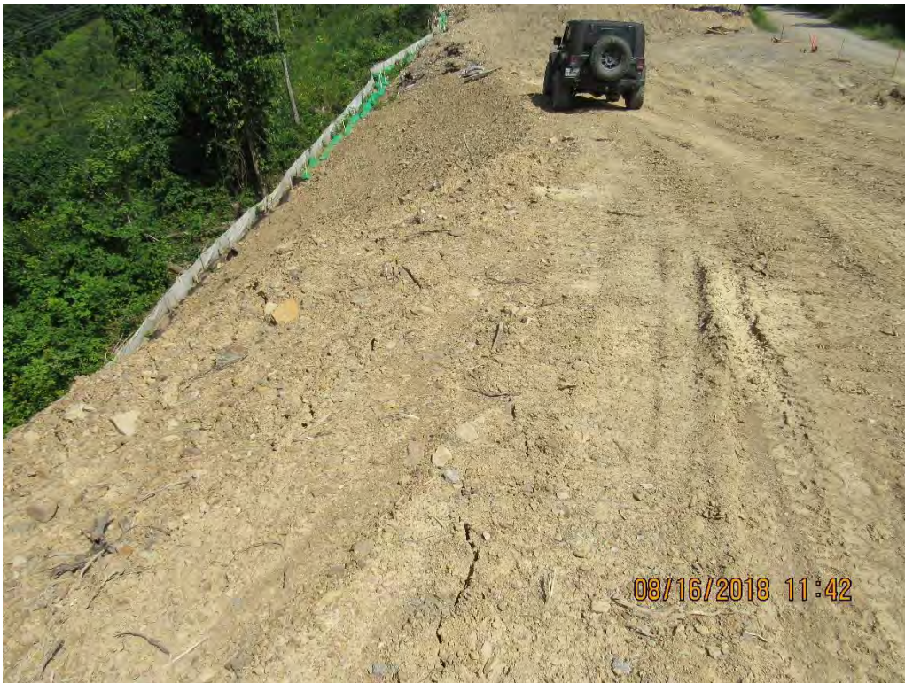
Photo 15: Northern view of Bamboo Road near Station 7158+00 without fill slope protection and temporary stabilization.
