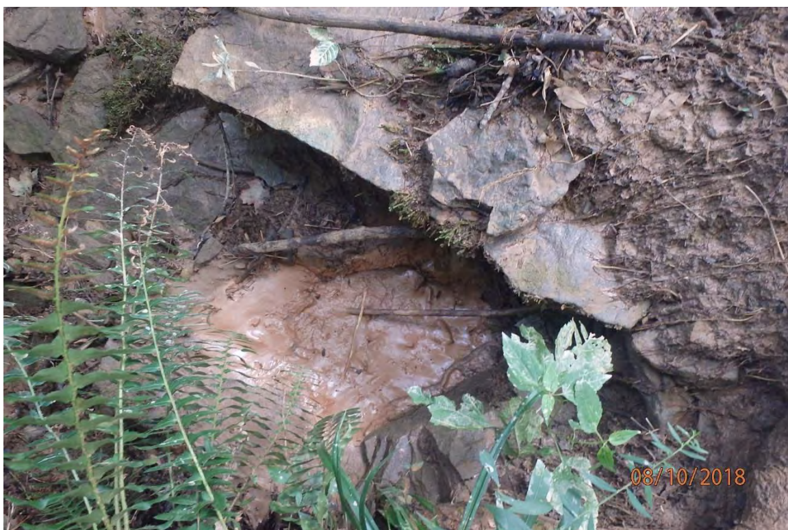
CNA deposits in UNT Kincheloe Creek (39° 10.006' X 80° 34.736') that originate from site. Deficiencies in site evaluation item numbers 2, 6, 7, 8, 14, 19, 20 & 21 pictured.
