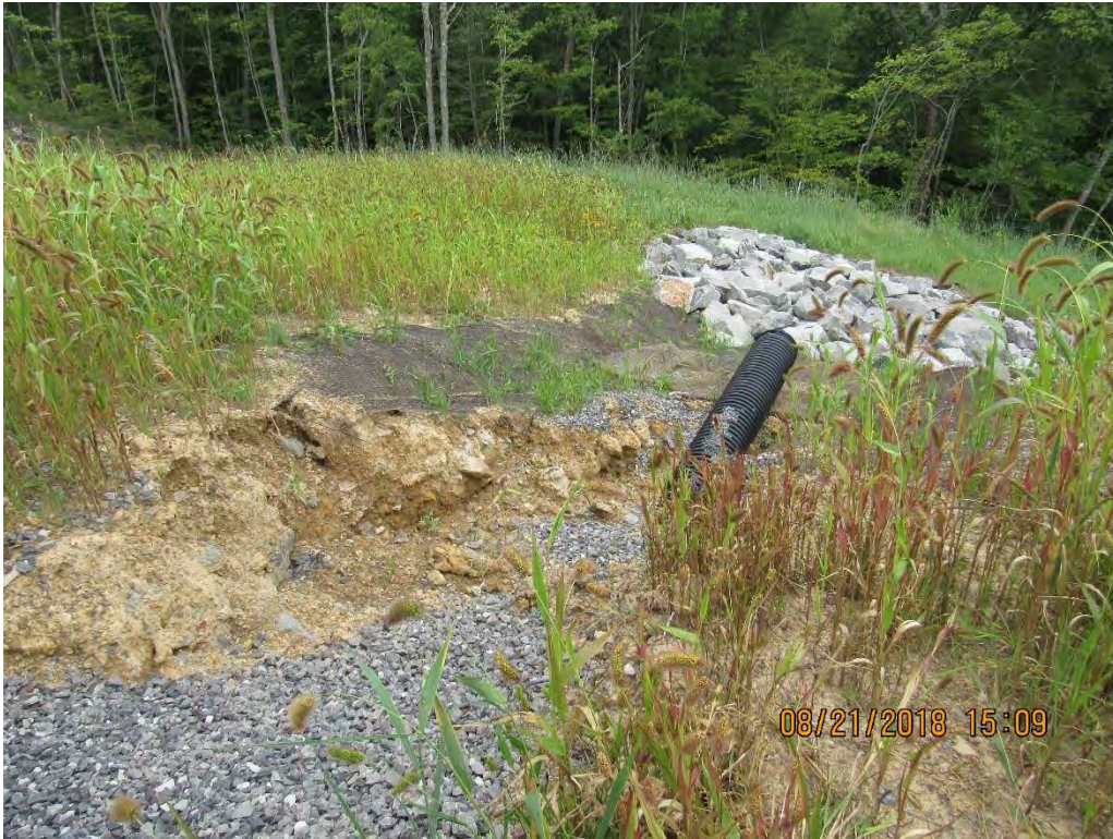
Photo 1: Unfinished underdrain installation.
