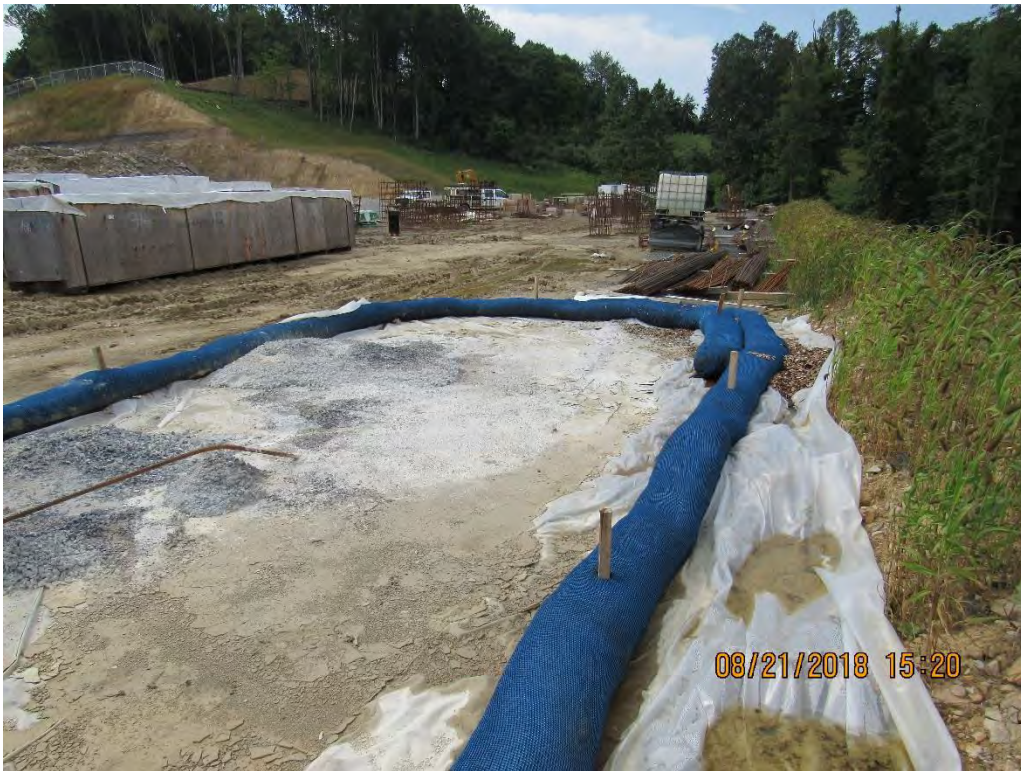
Photo 7: Improperly implemented control for concrete wash out area.
