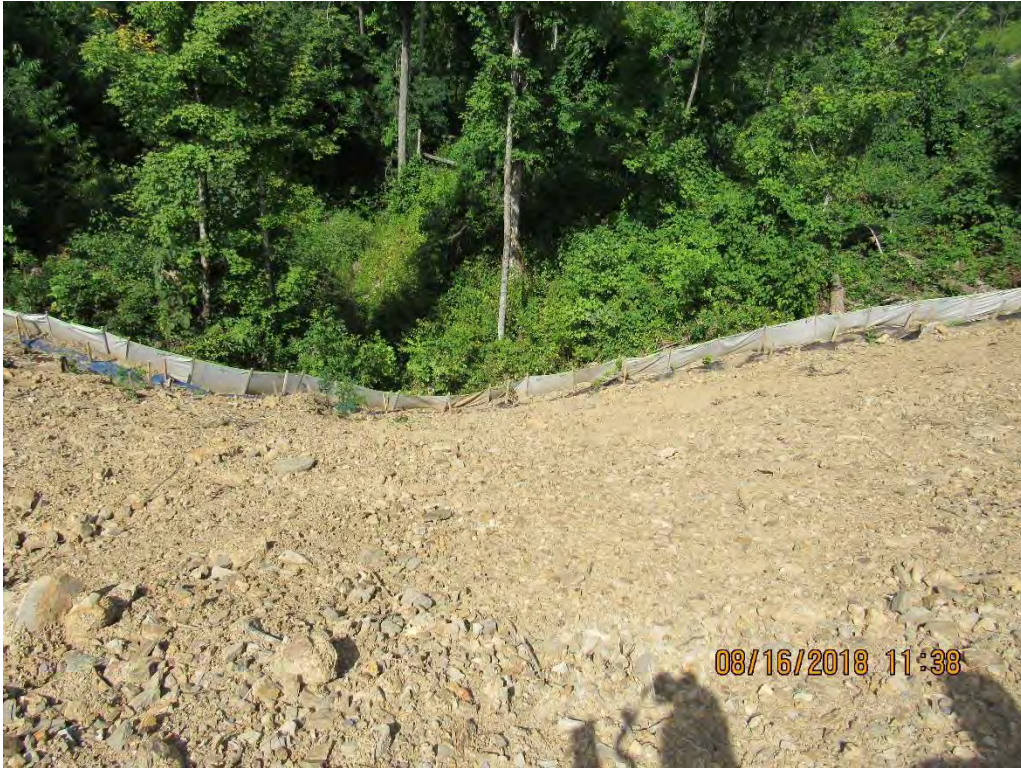
Photo 17: Inadequate controls for concentrated flow at base of fill slope near station 7158+00.
