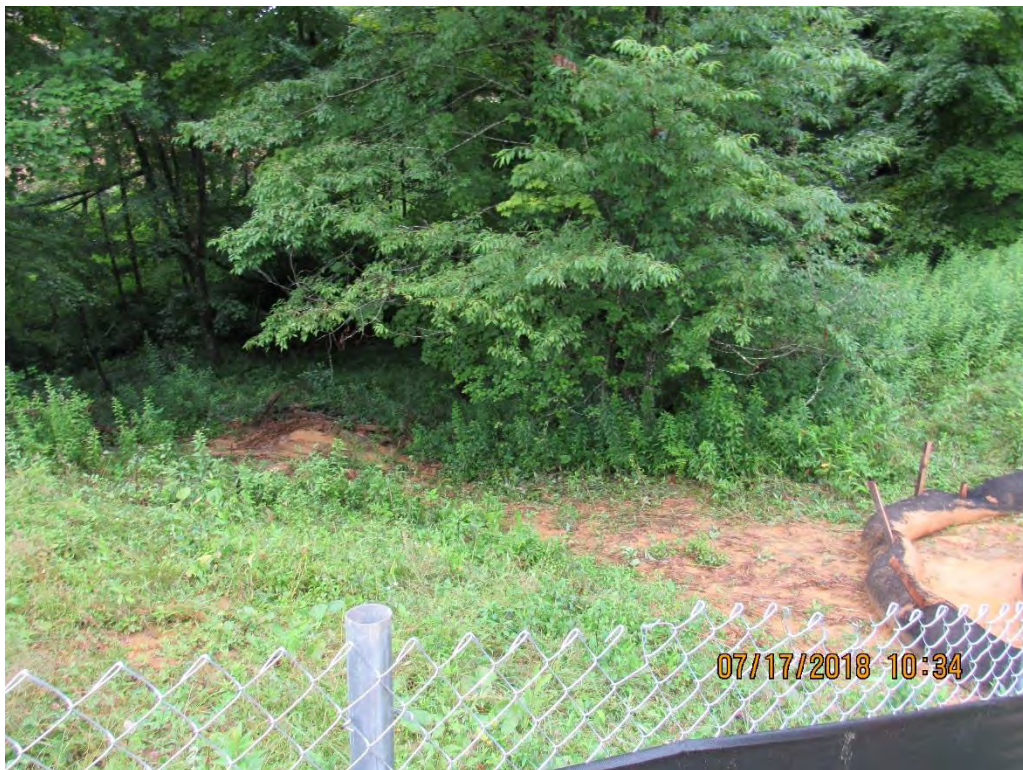
Photo 6: Last compost filter sock in sequence and path sediment laden water created leading to stream.
