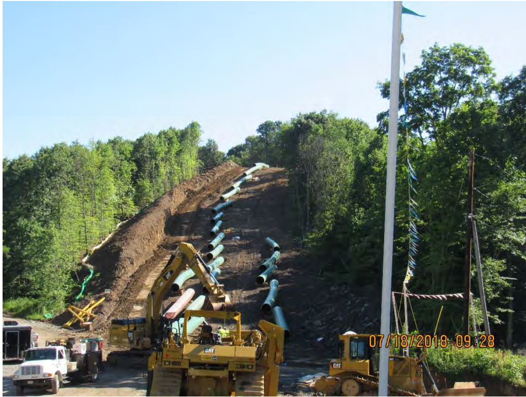
Photo 1: Station 6857+28 at access road 164 without temporary stabilization on large spoil pile. Photo is representative of project.
