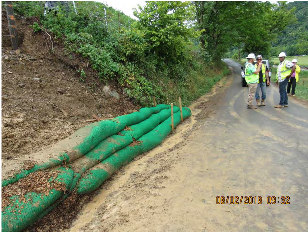
Photo 3: In process of stabilizing slope. Mud on road from crews performing maintenance.
