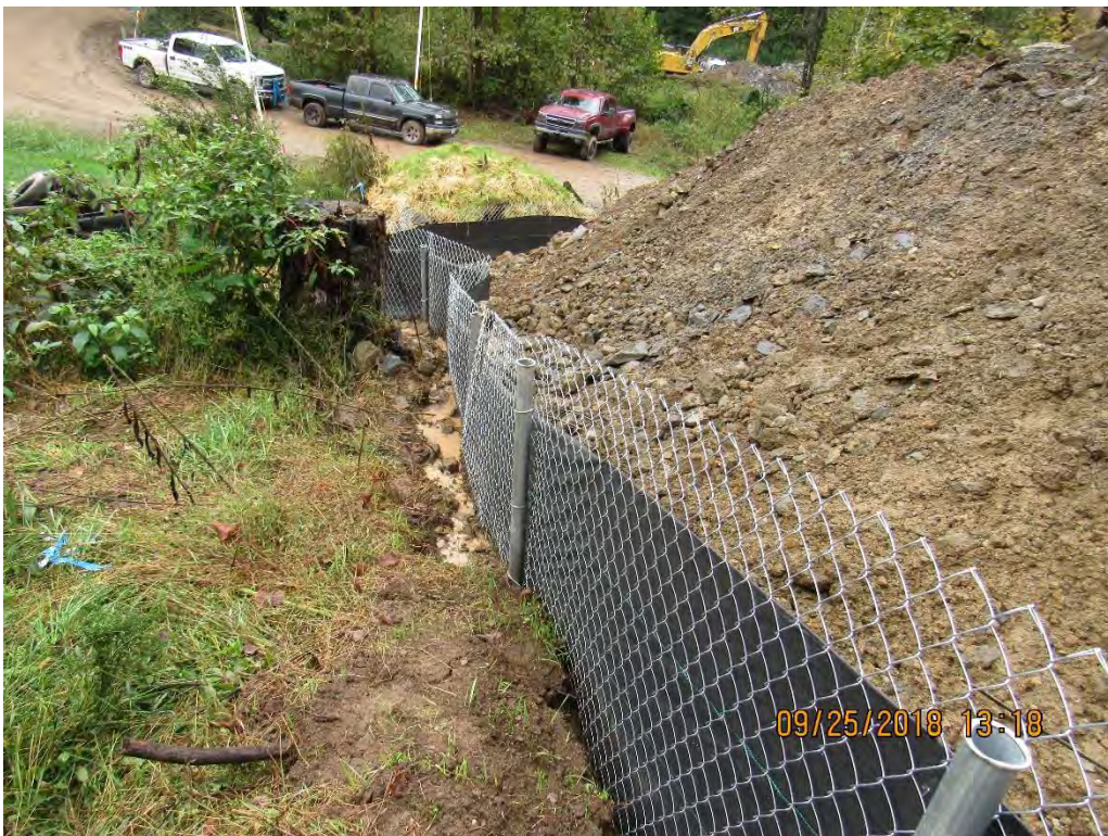
Photo 2: Undermined perimeter controls near 3634+00 which failed allowing sediment laden water to leave site.
