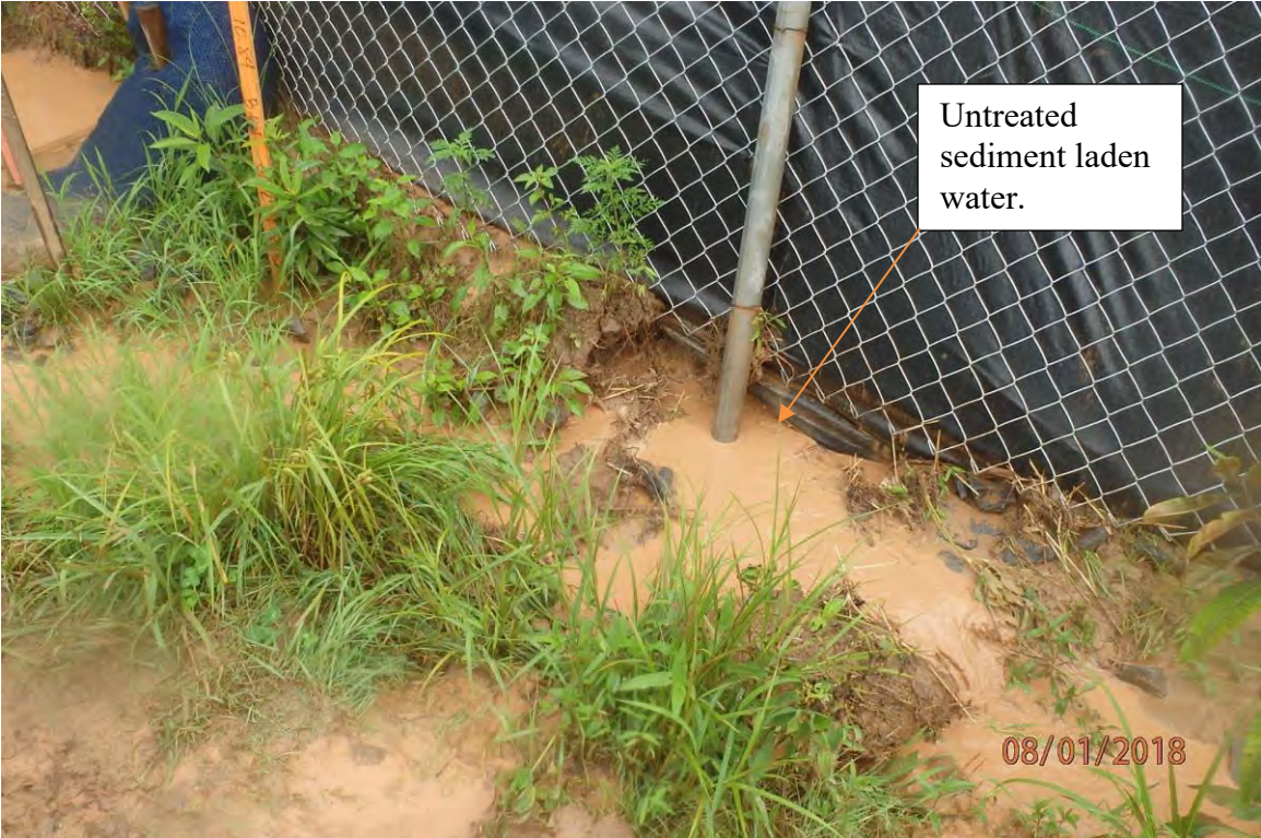
Concentrated flow from water bar outlet that is being treated by sheet flow BMP in the Big Elk Creek watershed. Deficiencies in site evaluation item numbers 1, 6, 7, 8, 13, 14, 19, 20 & 21 pictured.
