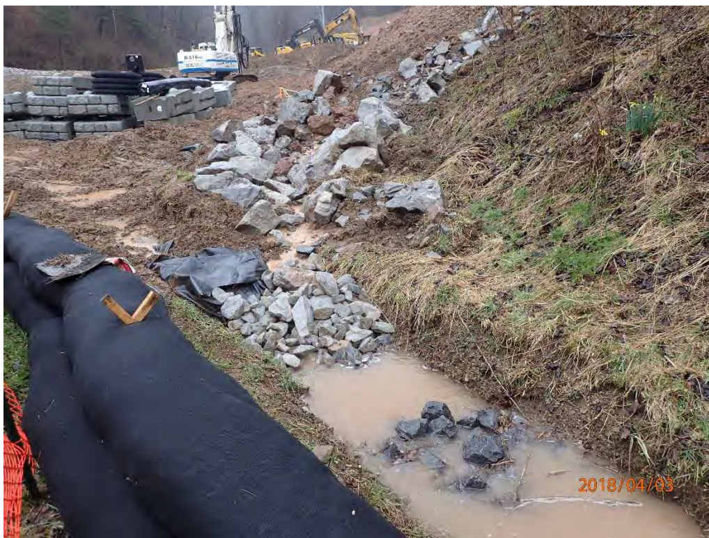
Sediment laden water leaving site through drop inlet.
