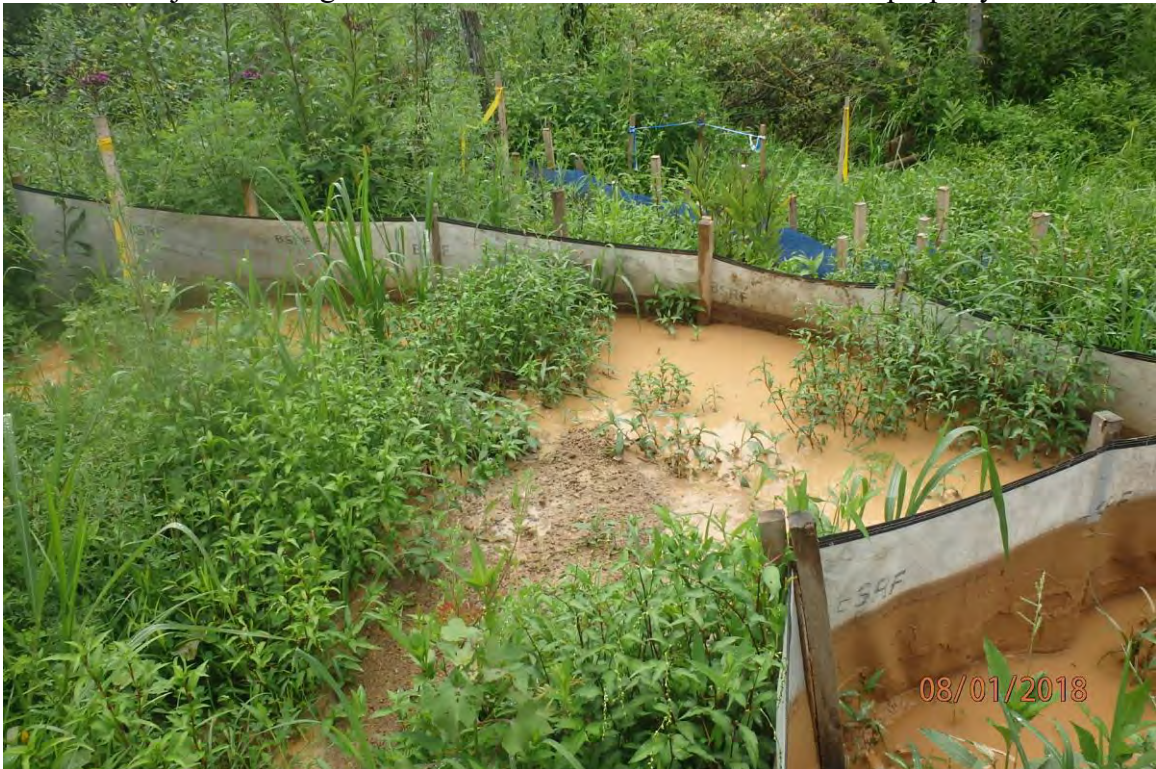
Perimeter controls adjacent to Goose Run that are overwhelmed due to improperly installed water bars.
