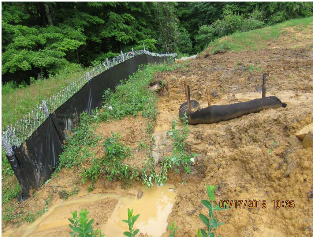
Photo 4: Station 5518+00 where water went around and undercut compost filter sock allowing sediment laden water to leave the site.
