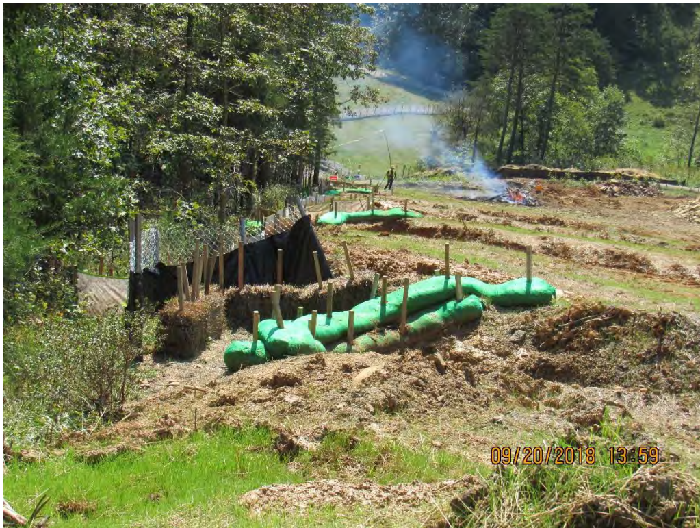
Photo 13: Ellison Ridge crossing near station 9778. Additional controls added due to historic release.
