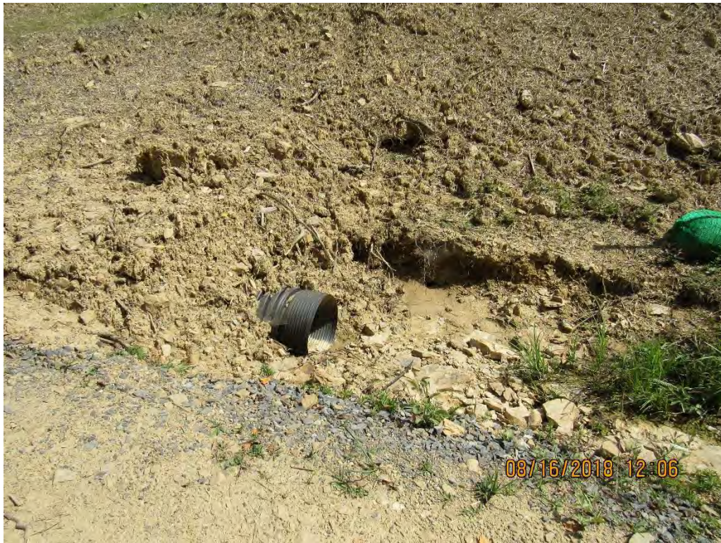
Photo 27: Installed culvert inlet near 7080+00 conveying sediment laden water from water bar terminus in photos 23-25 to SR culvert.
