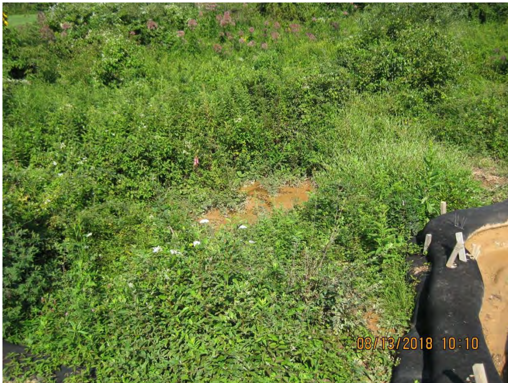
At St. 00+50 Sediment laden water had left the site via controls that had not been maintained. This control point is receiving concentrated stormwater from a large area and therefore requires an appropriately sized trapping structure.
