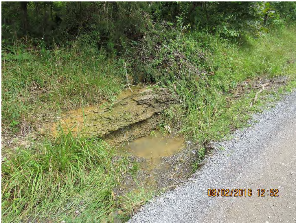
Photo 24: Entrance to UNT of Hans Creek several days after control failure on ROW- view upstream.
