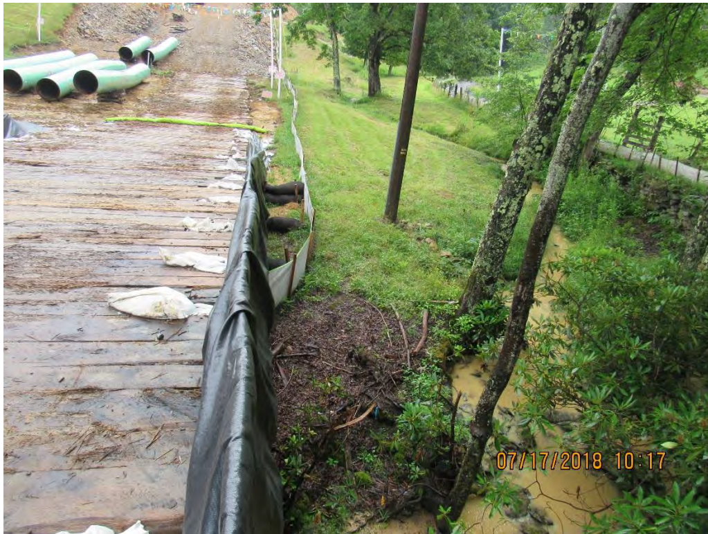
Photo 11: UNT #2 of Birch River (S-F365) at station 5548+00 where breached control upstream allowed sediment laden water in UNT #1 of Birch River (S-F34)
