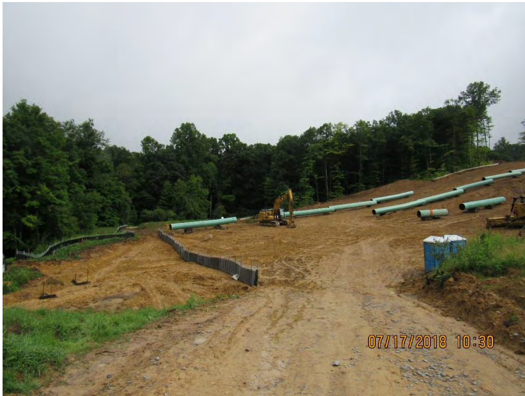
Photo 3: Drainage area where sediment laden water left site.
