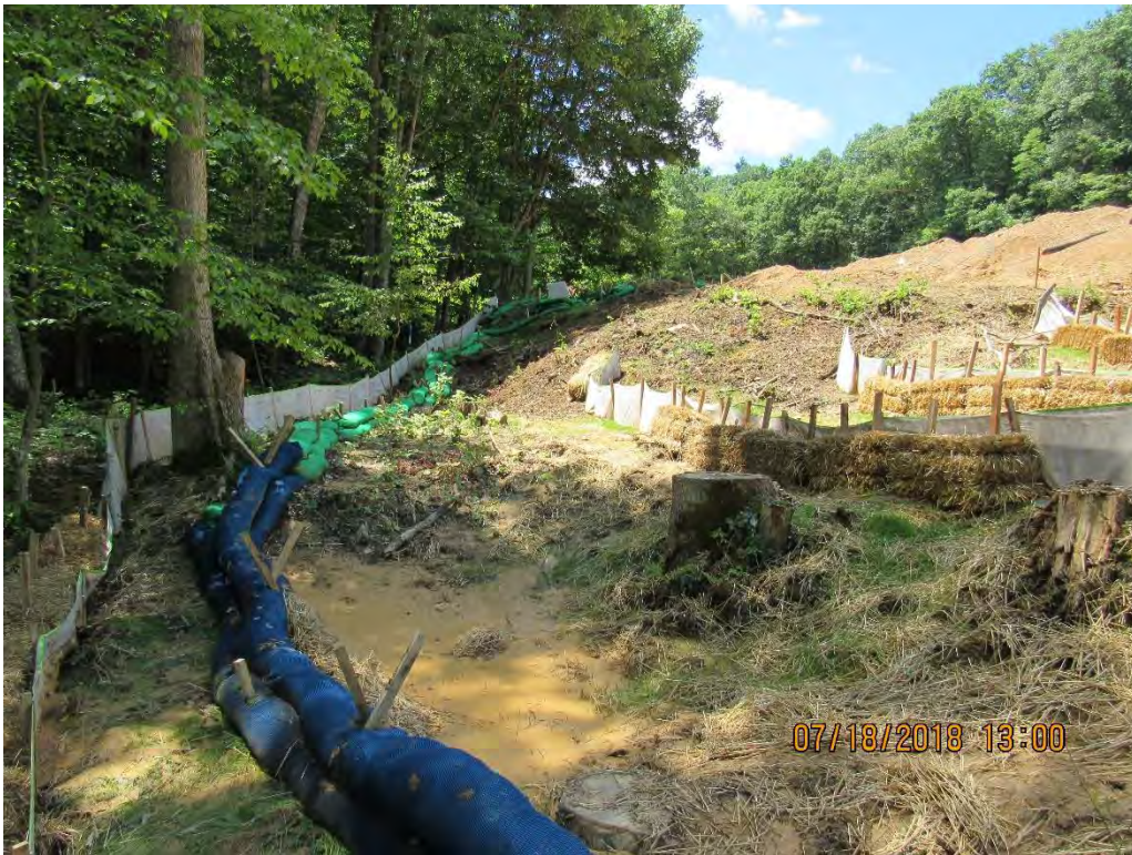
Photo 9: Control sequence near station 6781+87 with multiple control failure.
