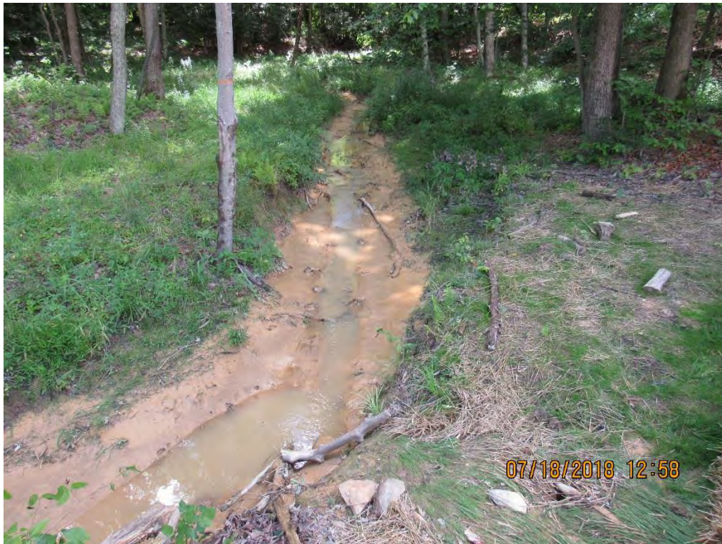
Photo 7: Sediment deposits in UNT of Harmony Creek- upstream of Photo 6. Terminus of control failure in Photos 9 & 10 (vegetation indication under date/time stamp)
