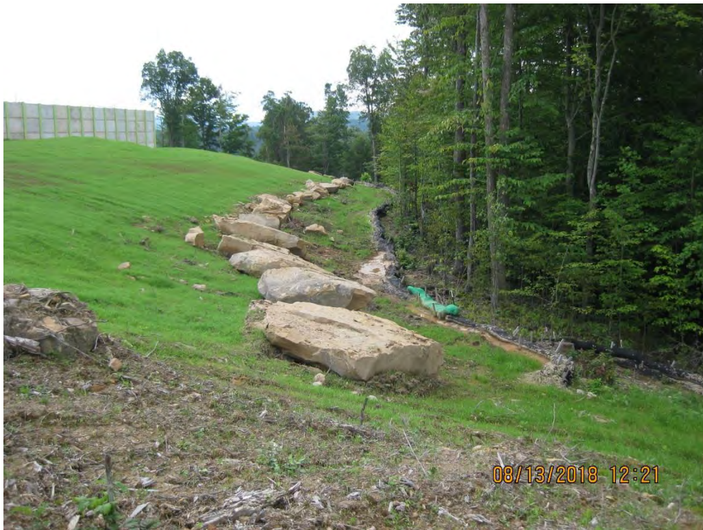
Maintenance needed for CFS at Southwest wall (marginal).
