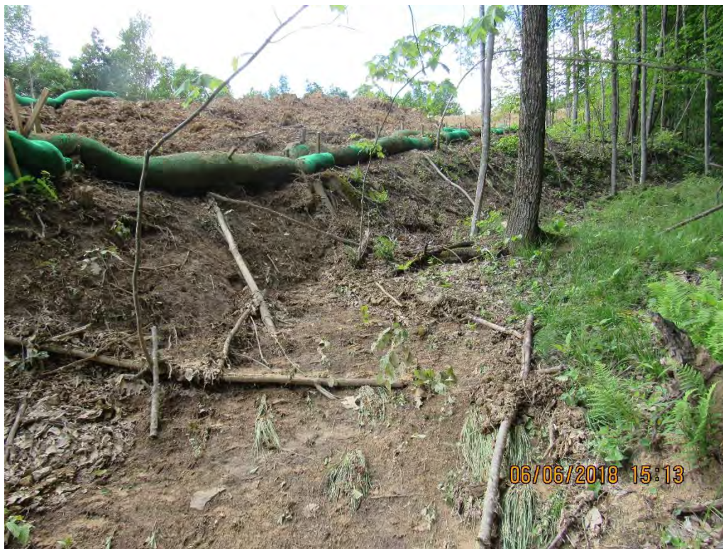
Photo 4: Control failure at station 6812+58 allowing sediment laden water to leave site.
