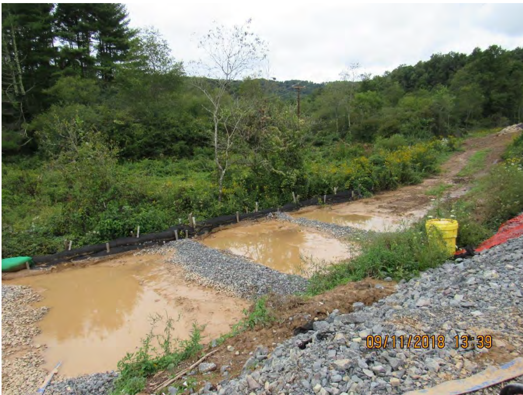
Photo 2: Station 50- New controls installed abating NOV issued 8/13/2018.
