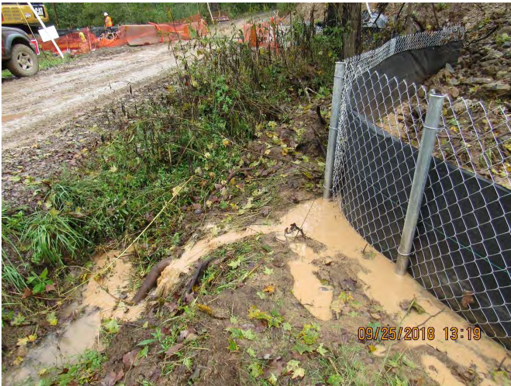
Photo 4: Close-up of failed perimeter controls near station 3634+00 where sediment laden water is entering UNT of Knawls Creek.
