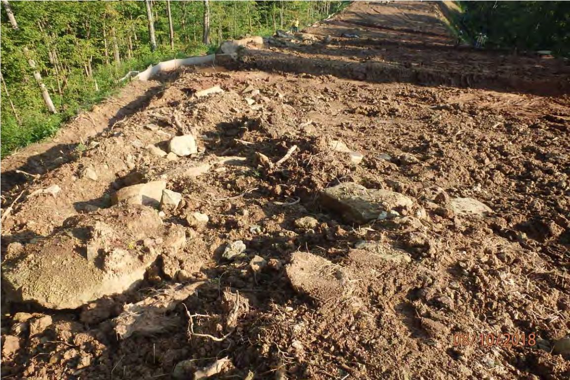
Fill slope erosion downslope of the above pictured area due to pipe trench outlet and water bar that is not installed properly in the Meathouse Fork watershed. Deficiencies in site evaluation item numbers 2, 6, 8, 14, 19 & 21 pictured.
