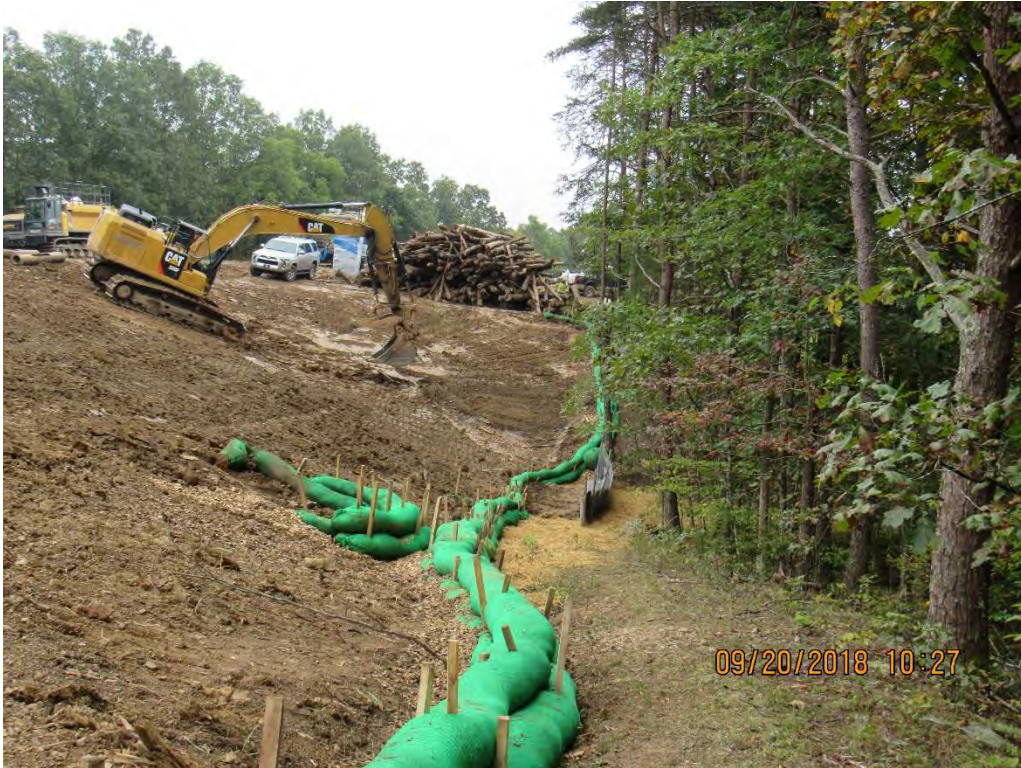
Photo 9: Source of historic release in photos 7 & 8 near station 9617+75. Final reclamation in process above Slate Run.
