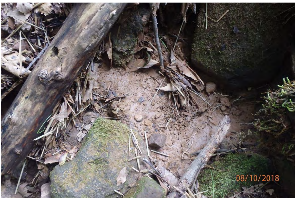
CNA deposits and associated straw mulch that originate from site in UNT Laurel Run (39° 01.133' X 80° 35.813'). Deficiencies in site evaluation item numbers 1, 13, 15, 19, 20 & 21 pictured.
