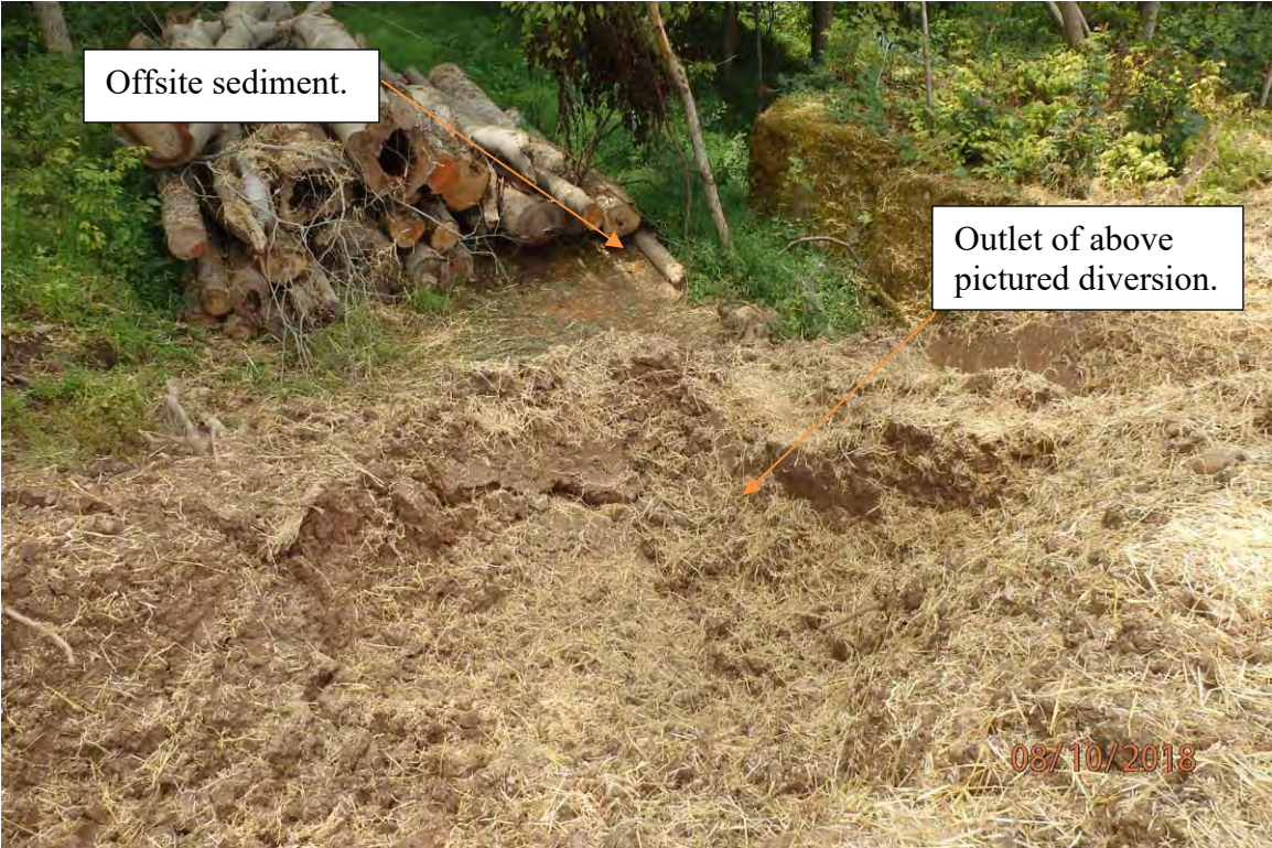
Unstable diversion that runs parallel to the slope and the associated erosion and offsite sediment deposits in the Cove Lick watershed. Deficiencies in site evaluation item numbers 2, 6, 8, 14, 19 & 21 pictured.
