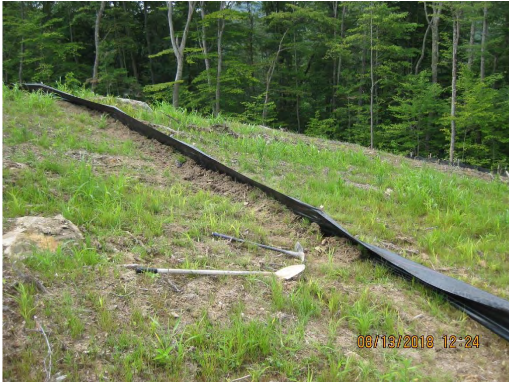
Silt fence being installed on the southern portion of the pad area was not joined or trenched in properly.
