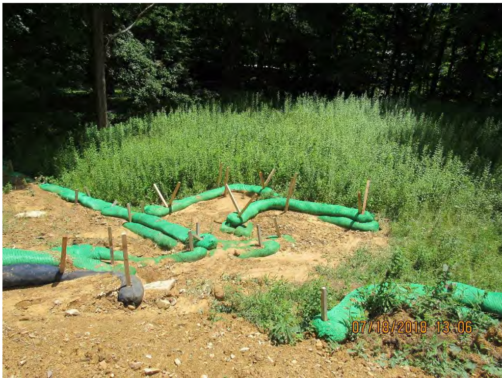
Photo 18: Installed controls at end of water bar proved inadequate and failed allowing sediment laden water to leave site.
