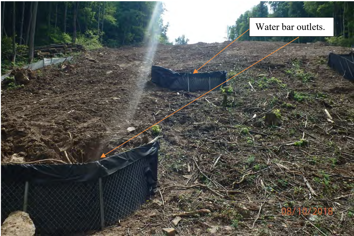
Improperly constructed water bars that do not shed stormwater off of the LOD in small quantities.
