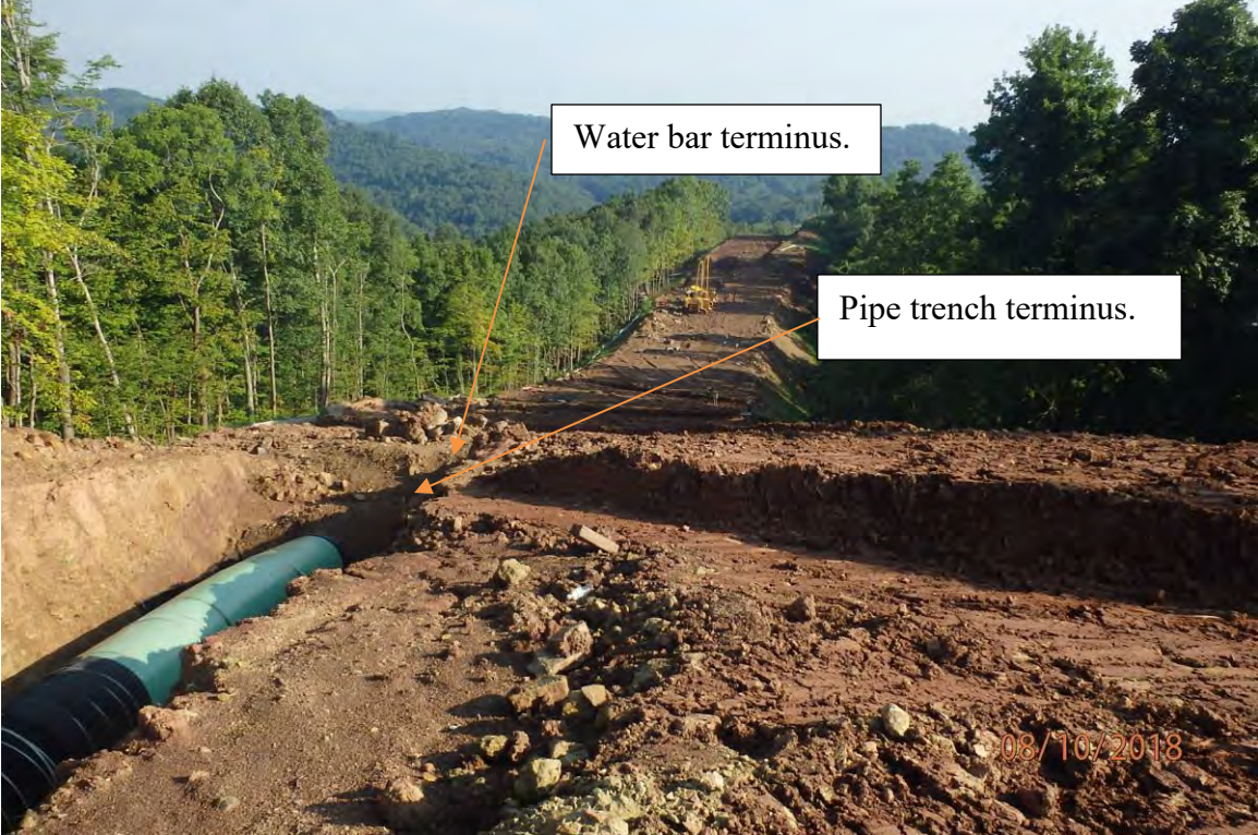
Improperly installed water bar in the Meathouse Fork watershed.
