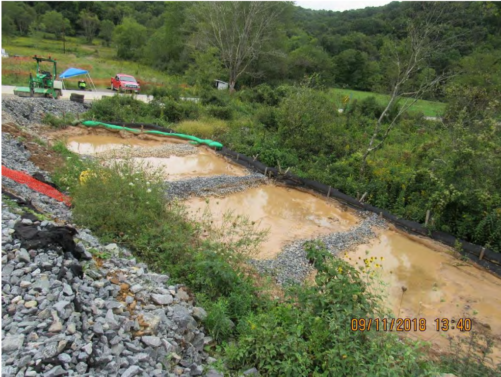
Photo 1: Station 50-New controls installed abating NOV issued 8/13/2018.
