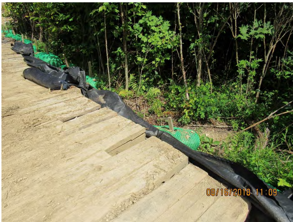
Photo 35: Recommended to add additional controls to timber mat bridge adjacent to wetland at station 7232+00.
