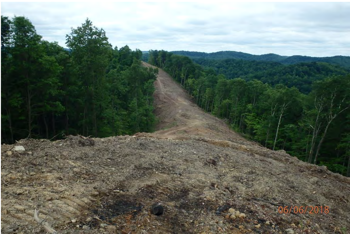
Areas of the project that have been cleared to mineral soil and BMPs are not in place as indicated in the SWPPP. Deficiencies in site evaluation item numbers 1, 7, 8, 13, 15, 19 & 21 pictured.
