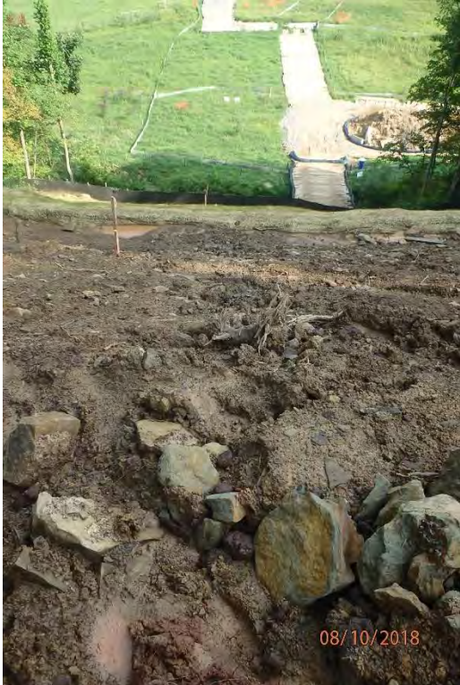
Water bar in Laurel Fork of Meathouse Fork watershed that has failed and is in need of maintenance.
