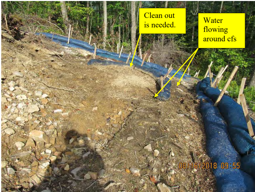
Photo 5: Water bar terminus needs maintenance at Bingham Road station 7450+00.
