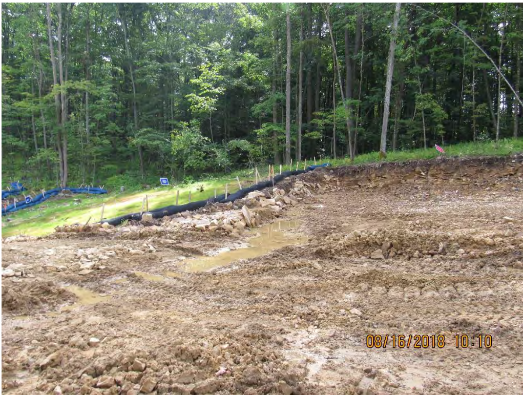
Photo 8: Eastern view of water bar without outlet near Bingham Road.
