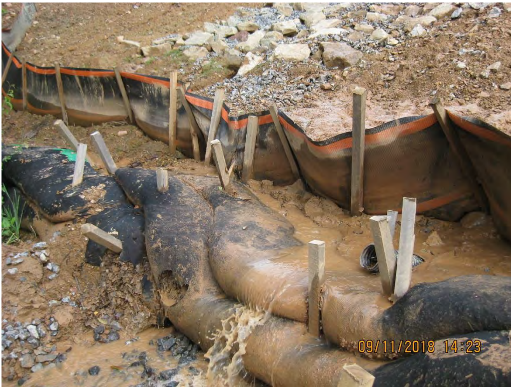
Photo 8: Station 900 (approximately)-Flow below silt fence into sump.
