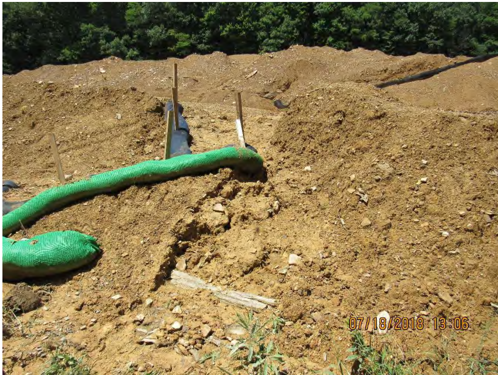
Photo 17: Erosion gullies from failed control at end of water bar near station 6785+50, which allowed sediment laden water to leave site.
