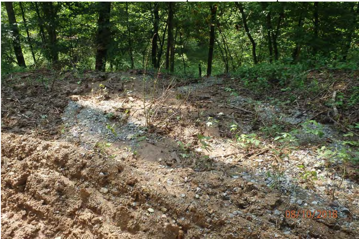
Access LE-73.01 in the Sand Fork watershed that does not have water bar terminus BMPs installed as indicated in the SWPPP. Marginal deficiencies in site evaluation item numbers 7, 13, 15, 19 & 21 pictured.
