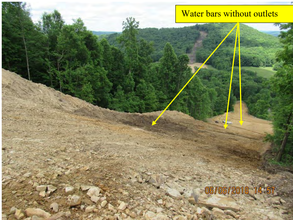
Photo 3: Water bars installed without adequate outlets near station # 6801+38 with <24^{\circ} to >30^{\circ} slope.
