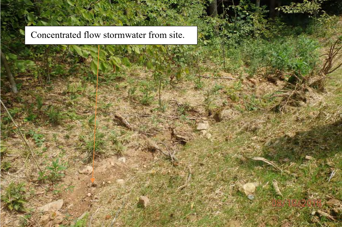
Project area adjacent to 2692+00 showing a lack of installed BMPs where sediment laden water leaves the site.
