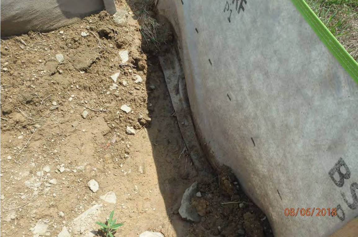
BMP in Seal Run watershed in need of maintenance that led to offsite sediment deposits.
