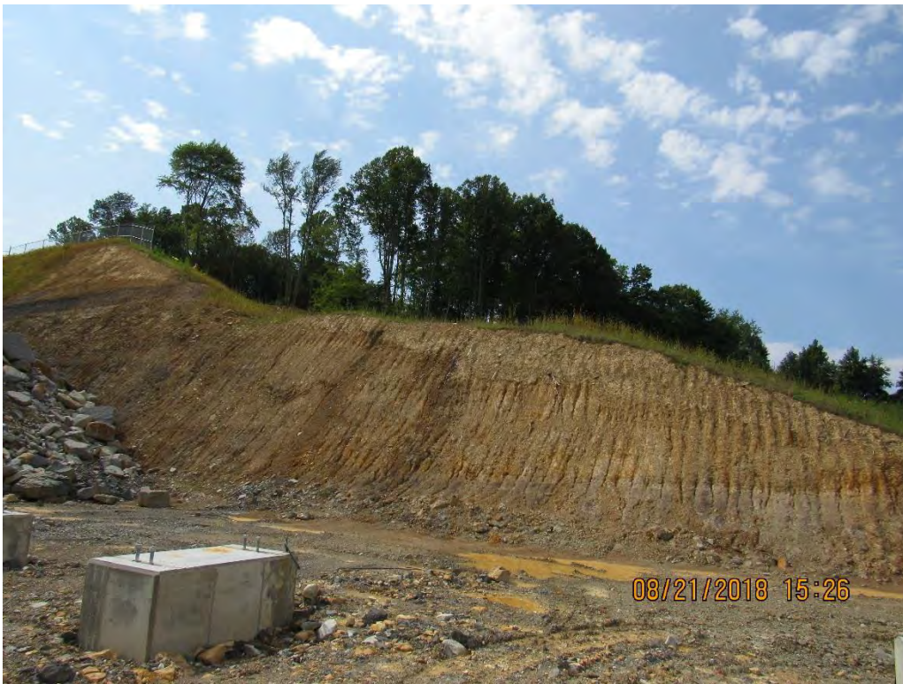
Photo 4: Slope on northwest side of site which has not been reseeded.
