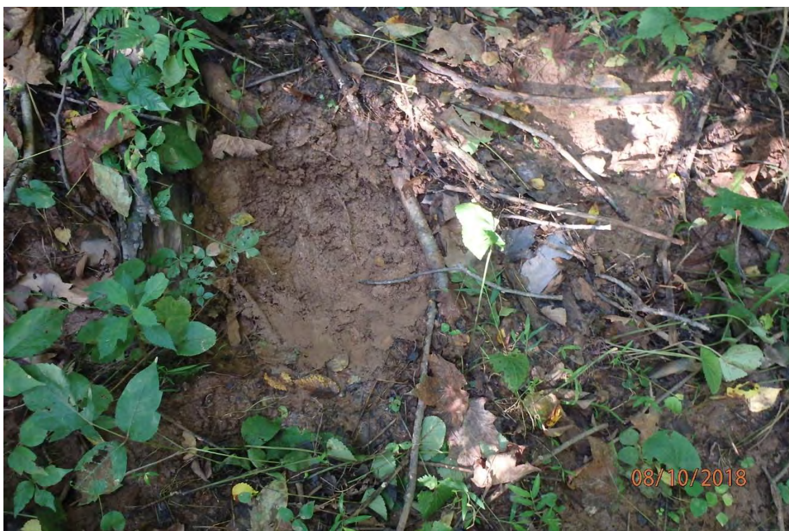
CNA deposits and distinctly visible settleable solids in UNT Meathouse Fork (39° 11.891' X 80° 33.209') that originate from site because of the previously pictured deficiencies. Deficiencies in site evaluation item numbers 6, 7, 19, 20 & 21 pictured.
