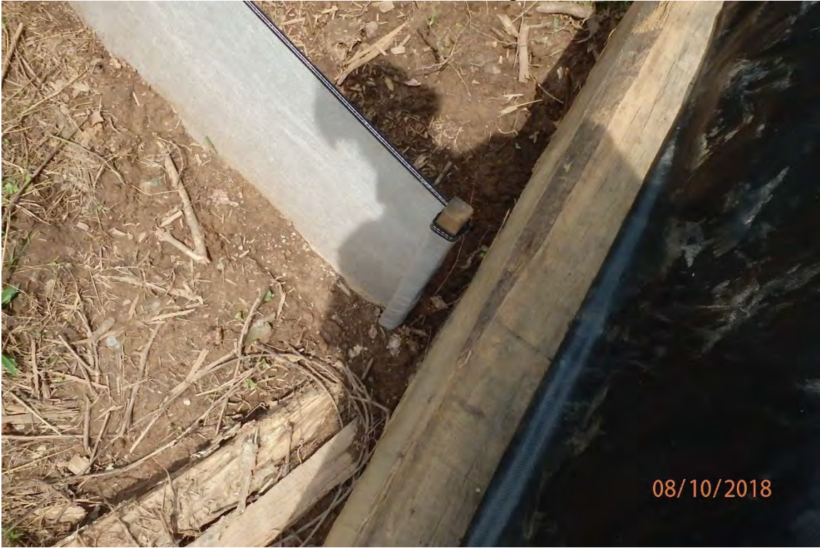
Laurel Run of Cove Lick (SKK6) crossing showing perimeter control not properly tied in to timber mat crossing. Marginal deficiencies in site evaluation item numbers 1, 19 & 21 pictured.
