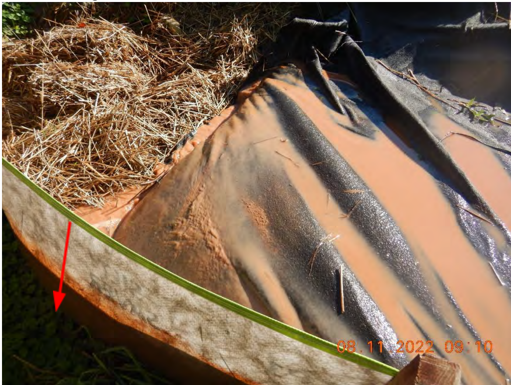
Photo # DSCN2179 – End of the de-watering filter bag opposite the end where the incoming pump water enters. The photograph shows sediment laden water flowing
