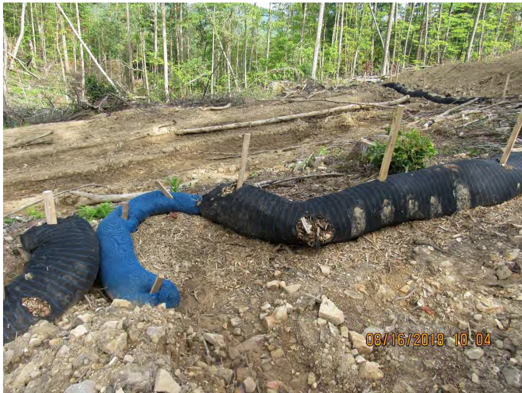
Photo 12: CFS needs maintenance near Bingham Road station 7450+00.
