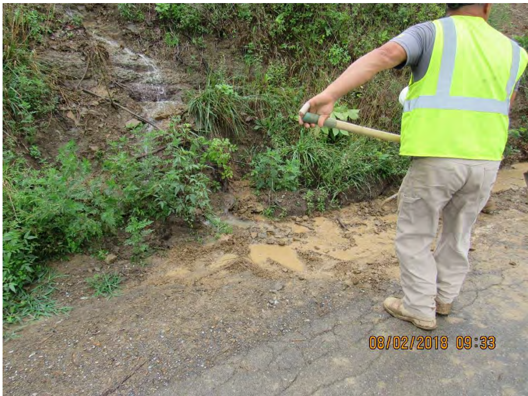
Photo 2: Water bar discharge mixing with sediment in road side ditch with crew performing maintenance.
