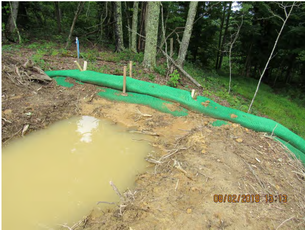
Photo 31: Water bar end altered to alleviate future failure of controls down gradient.
