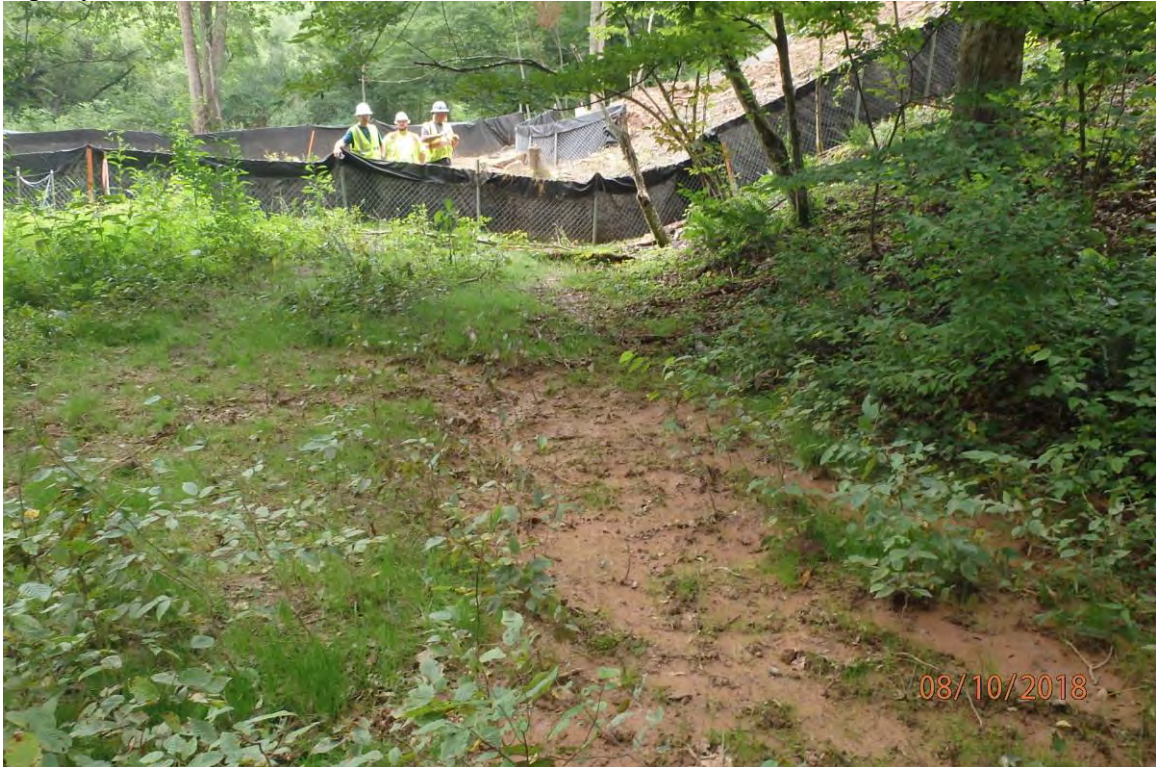
Sediment trail leading to Laurel Run (39° 01.043' X 80° 35.867') from the site as a result of perimeter controls that have been overwhelmed due to improperly installed water bars and being not properly operated. Deficiencies in site evaluation item numbers 6, 7, 14, 19, 20 & 21 pictured.
