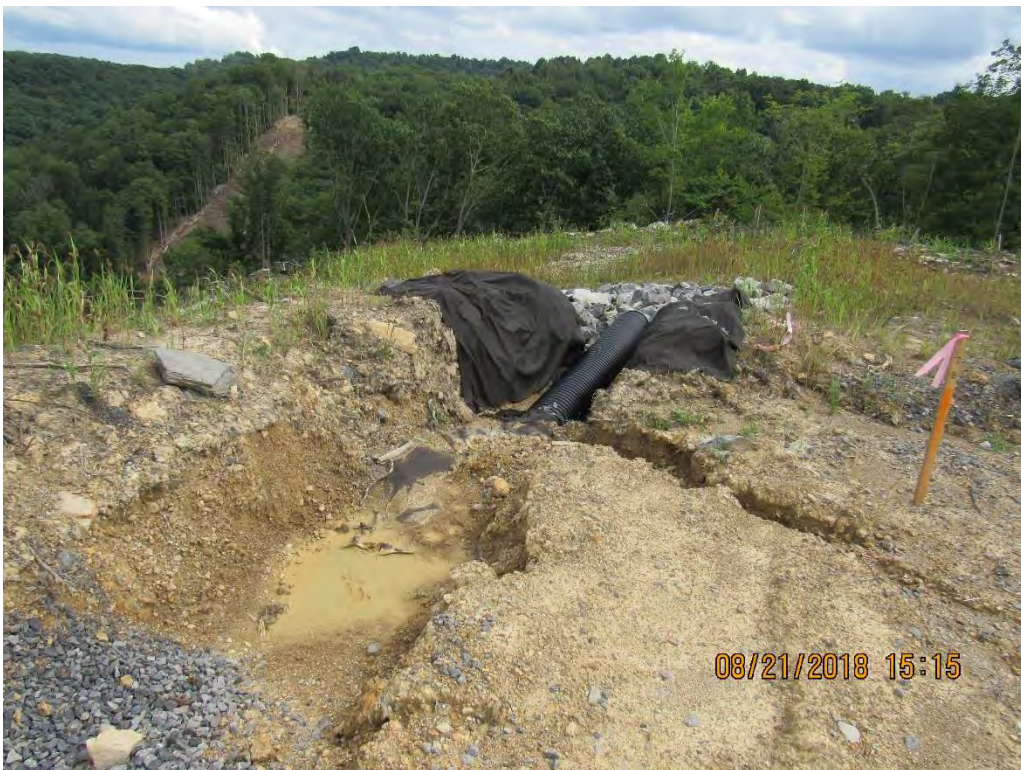
Photo 2: Unfinished underdrain installation.
