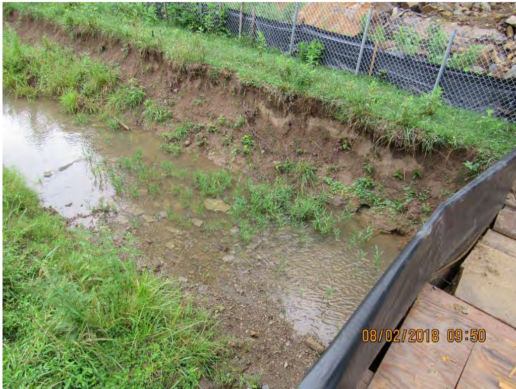
Photo 9: Upstream of bridge on east side of site below vertical mat rock barrier.
