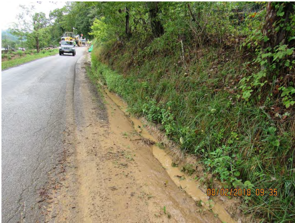
Photo 4: End of road side ditch prior to culvert diverting to laydown yard.
