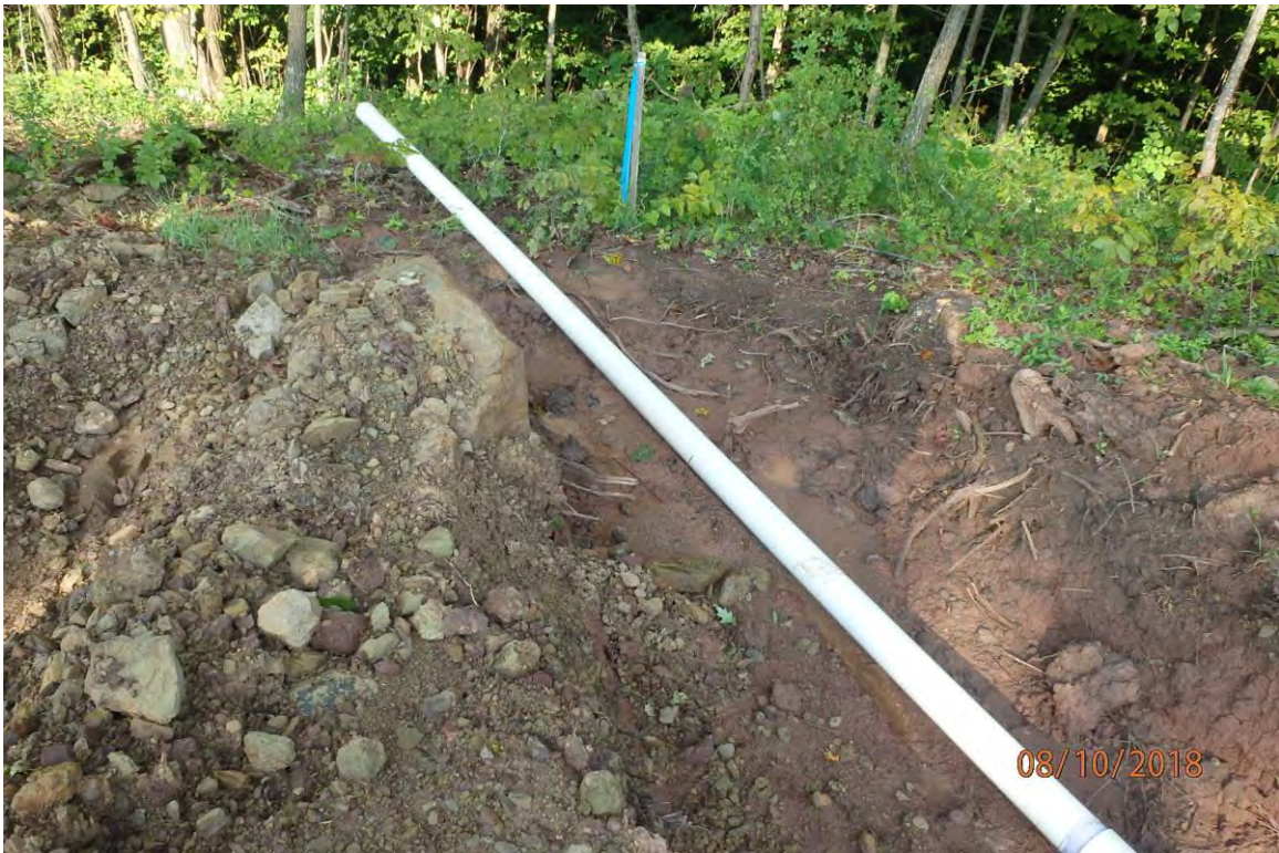
Water bar terminus BMPs that have been removed in the Meathouse Fork watershed due to trench plug drain installation that were not in place at the time of inspection.
