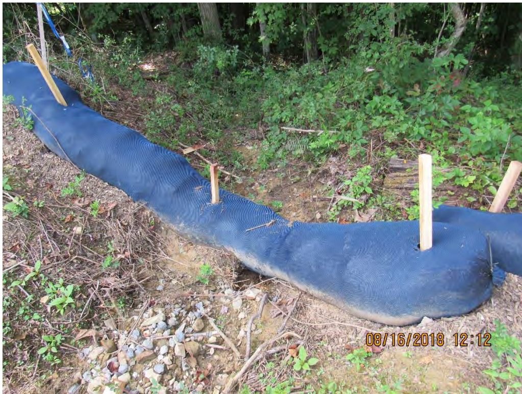
Photo 30: Perimeter controls failure downslope of SR culvert outlet allowing sediment laden water to leave site.
