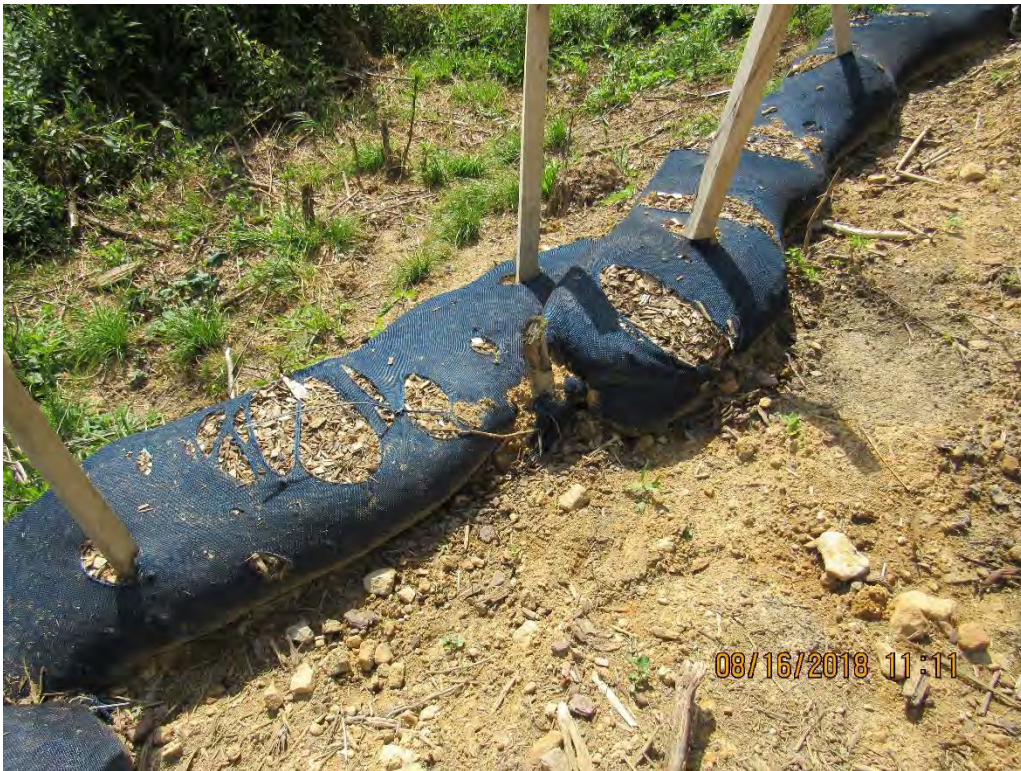
Photo 13: CFS needs maintenance near station 7232+00
