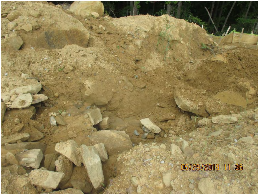
Waterbar outlet terminating onto slope at station No. 4027+00
