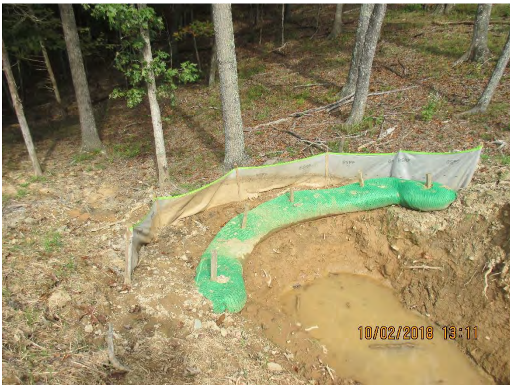
BMP outlet being overwhelmed near station number 9717+52.
