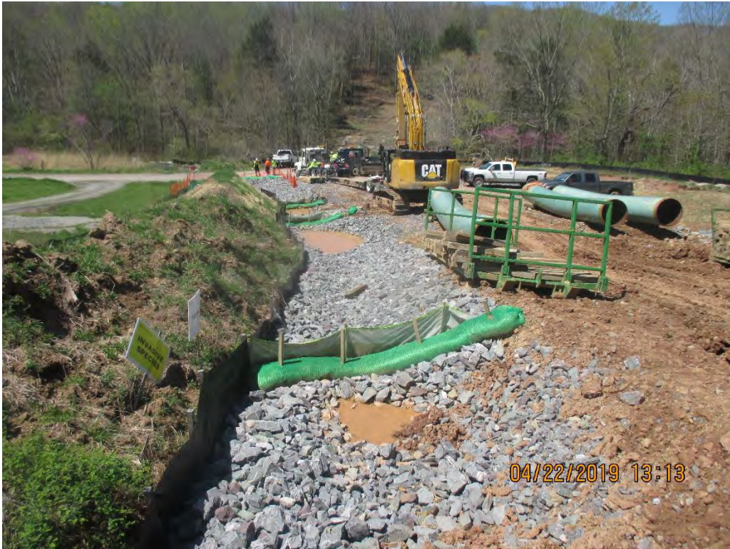
Controls on West side of LOD facing North at station #9004+00
