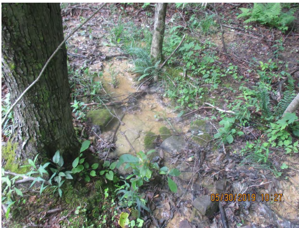
Sediment deposits past the LOD and controls at station No. 6474+16.
