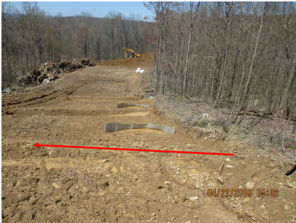
Waterbars terminating onto ROW at station #8633+71 facing North/Downslope. Arrow depicts Waterbar that was overwhelmed with sediment that impacted stream S-T35(A).
