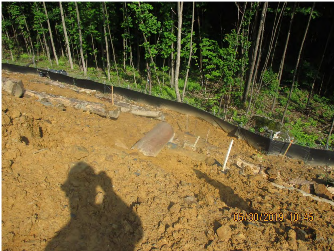
Pipe outlet below seep. Diversion not stabilized and No rip rap apron installed as required per SWPPP near station No. 6485+10. The inlet had been cut due to trench being dug.
