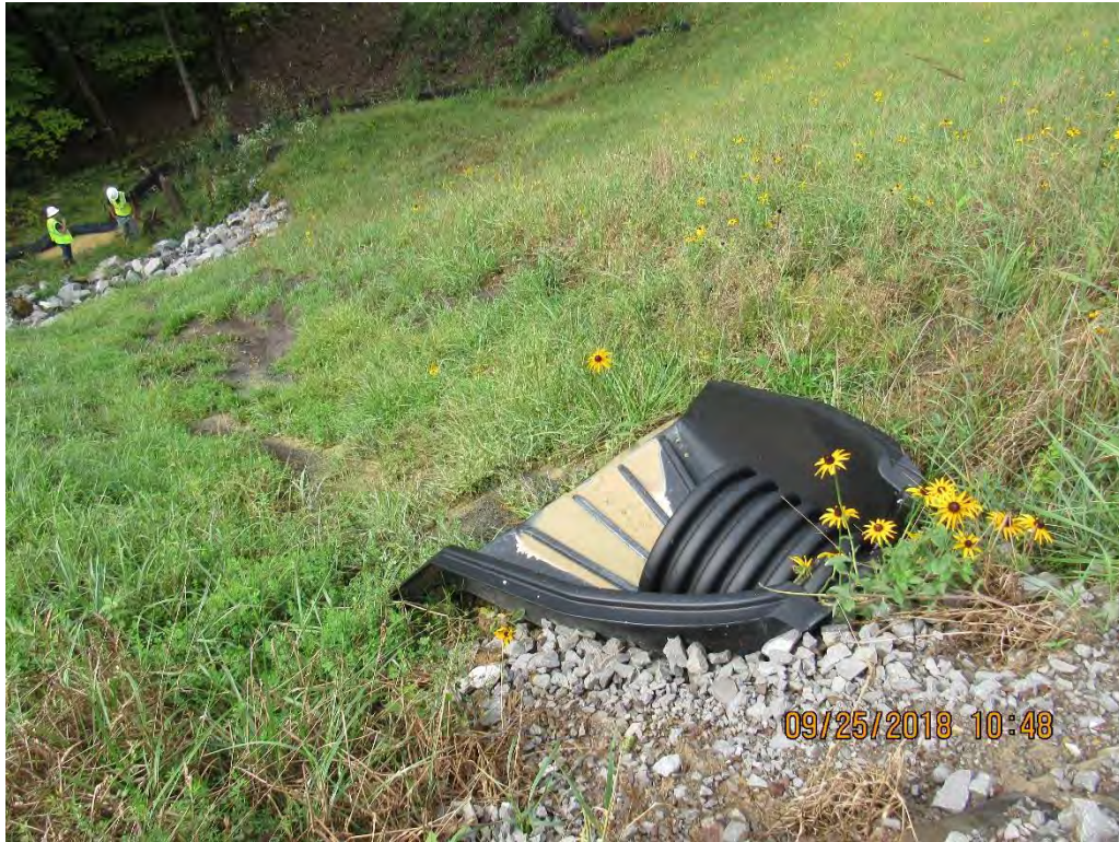
Photo 1: Station 550 outlet and sump at base of fill slope where perimeter controls failed allowing sediment laden water to leave site and create conditions not allowable in UNT of Little Kanawha.
