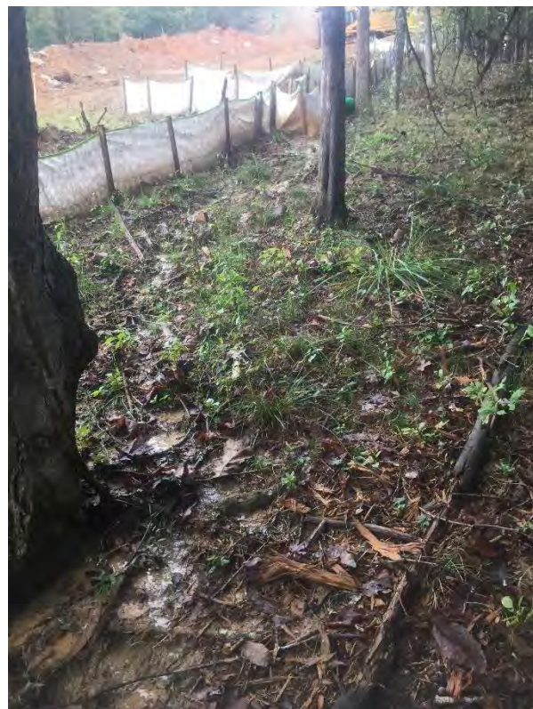
ROW near station numbers 9779+00 and 9778+00 where water bar outlets were being overwhelmed and SLW was passing through and under and being transported past LOD.
