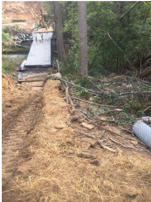
Facing Hans Creek near Station #9907+00. Super Silt fence located next to chain link had failed and sediment deposits were observed migrating towards Hans Creek.
