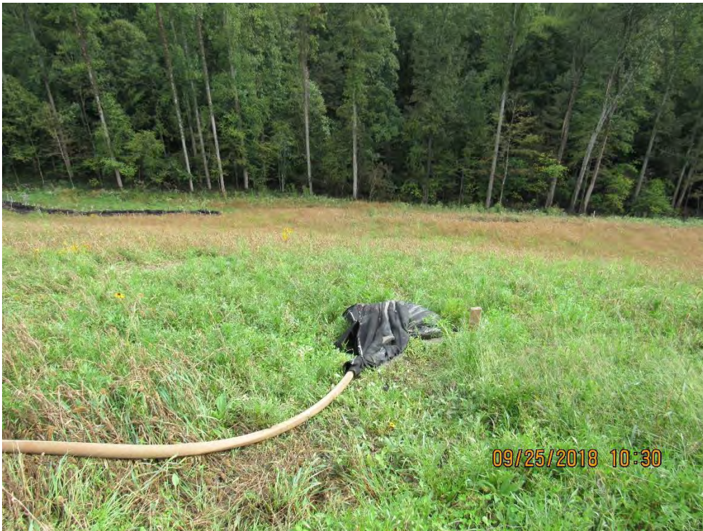
Photo 5: 2 of 3 improperly installed filter fabric bags still in use on north eastern side of site.
