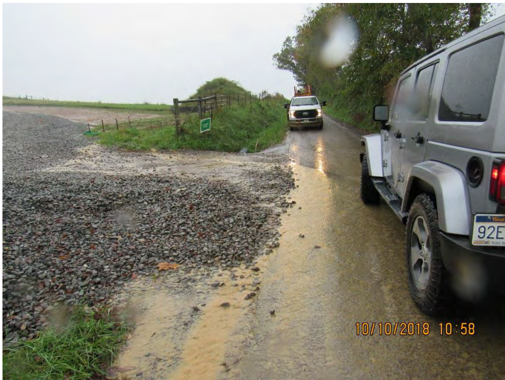
Photo 2: AR 210-sediment laden water leaving site entering county road- up gradient view.
