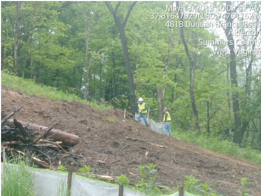
Complainant photo depicting MVP field staff installing outlet controls on Monday 5/13/19 at 10:09am.
