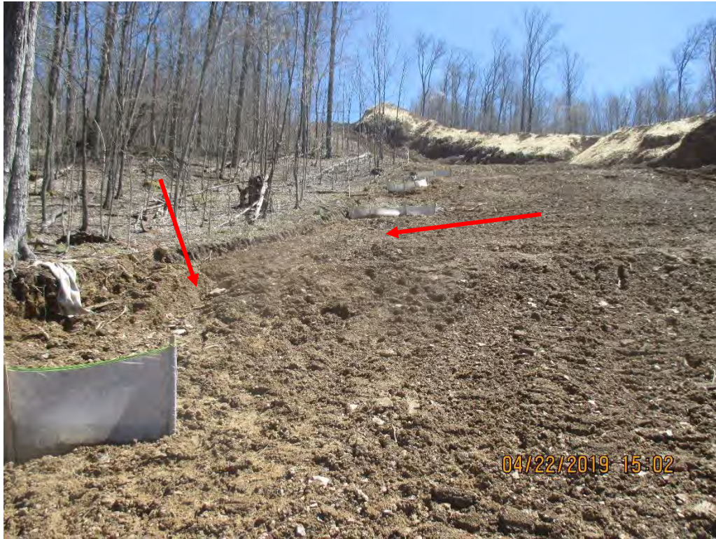
Facing upslope at station #8633+71. Arrow depicts where erosion is occurring between waterbars.
