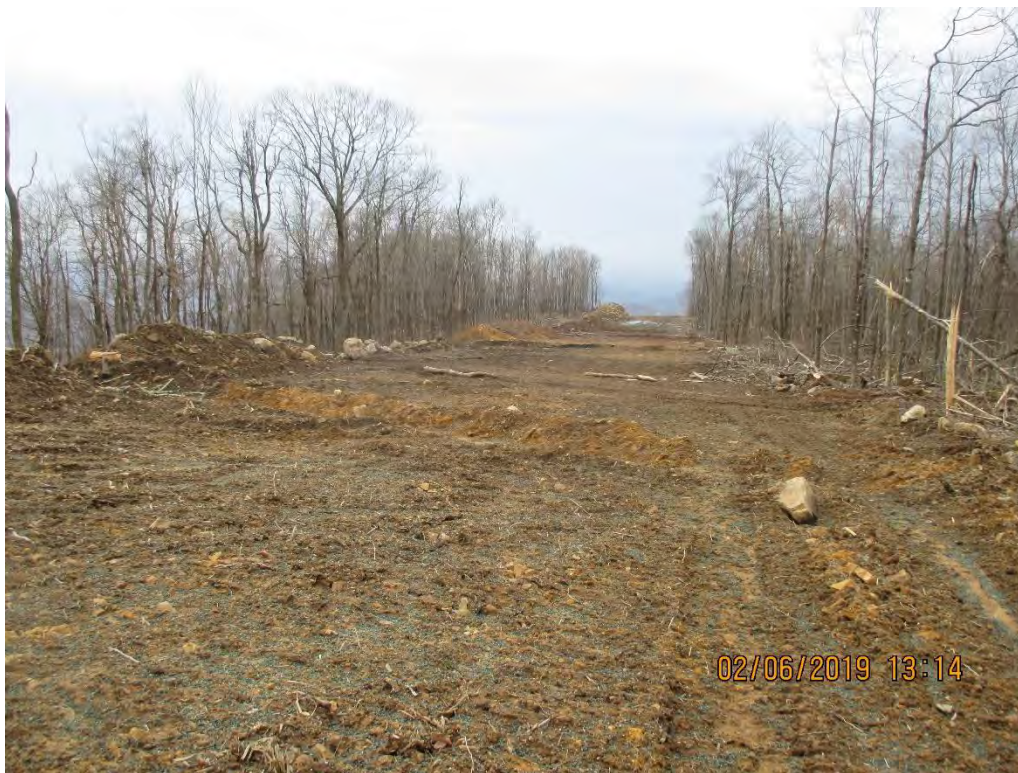
MVP ROW facing South at station number 8795+00. Waterbars in place per SWPPP.
