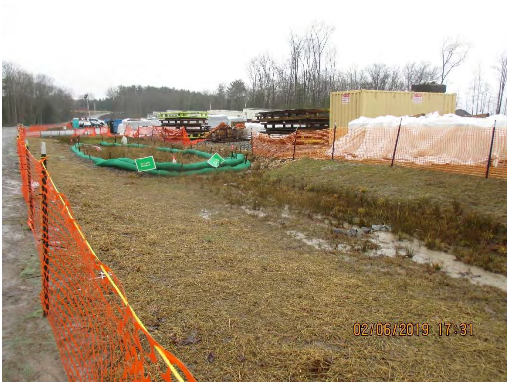
View facing towards wetland in drainage ditch. Sediment laden water (SLW) present in ditch and wetland.
