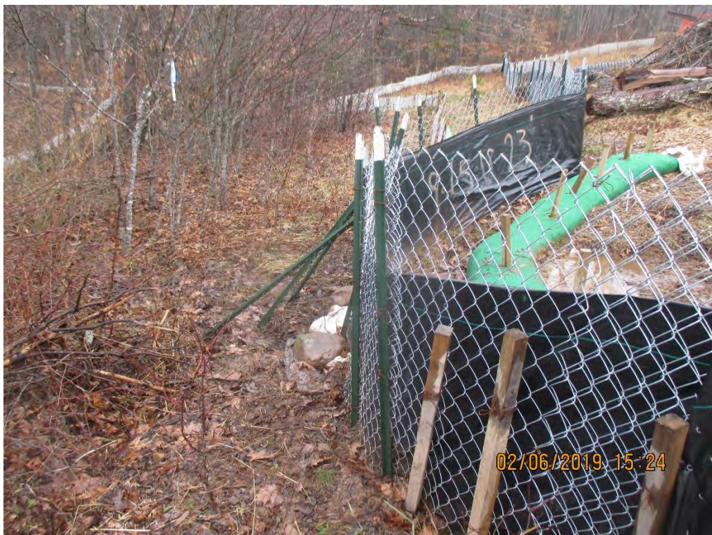
Super silt fence at end of controls near station #8986+00 Water running clear at time of inspection.
