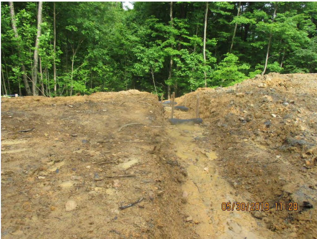
Seep running onto ROW via Waterbar above Stream S-N13. Diversion not stabilized near station No. 6940+00.
