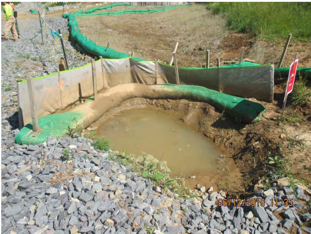
Controls added on edge of LOD to control run-on from adjacent property disturbance.
