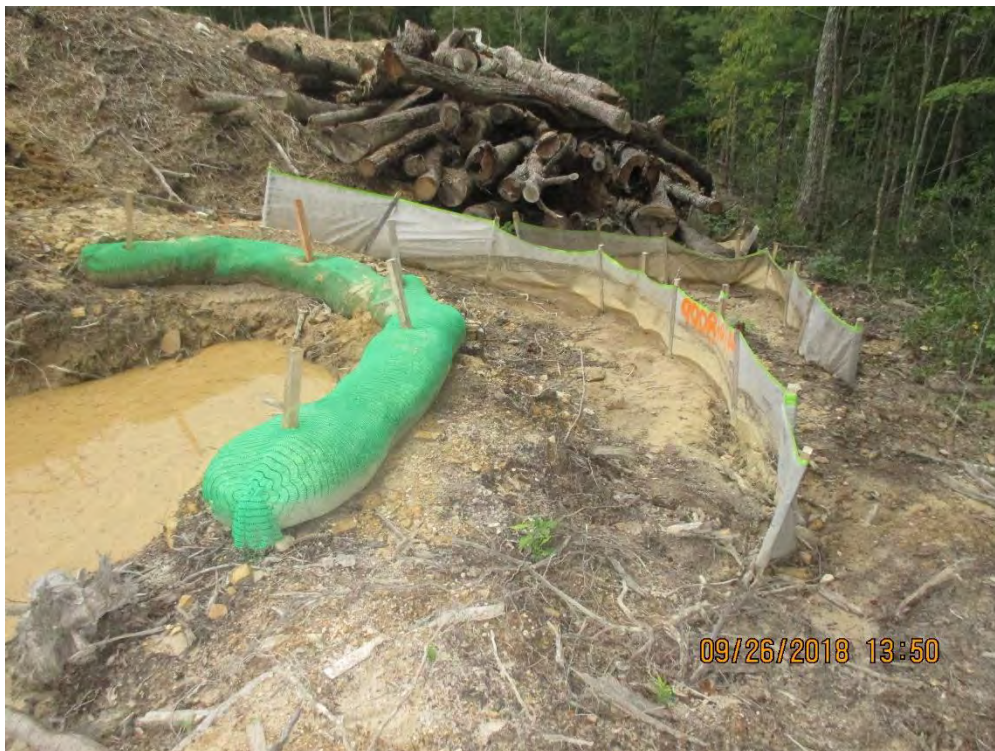
BMP at Station number 9908+00 being overwhelmed where off-site sediment deposits were present past the LOD.
