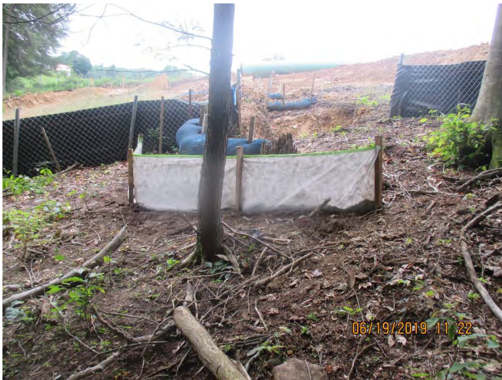
Waterbar Outlet with enhanced secondary controls added at Station No. 6587+00.
