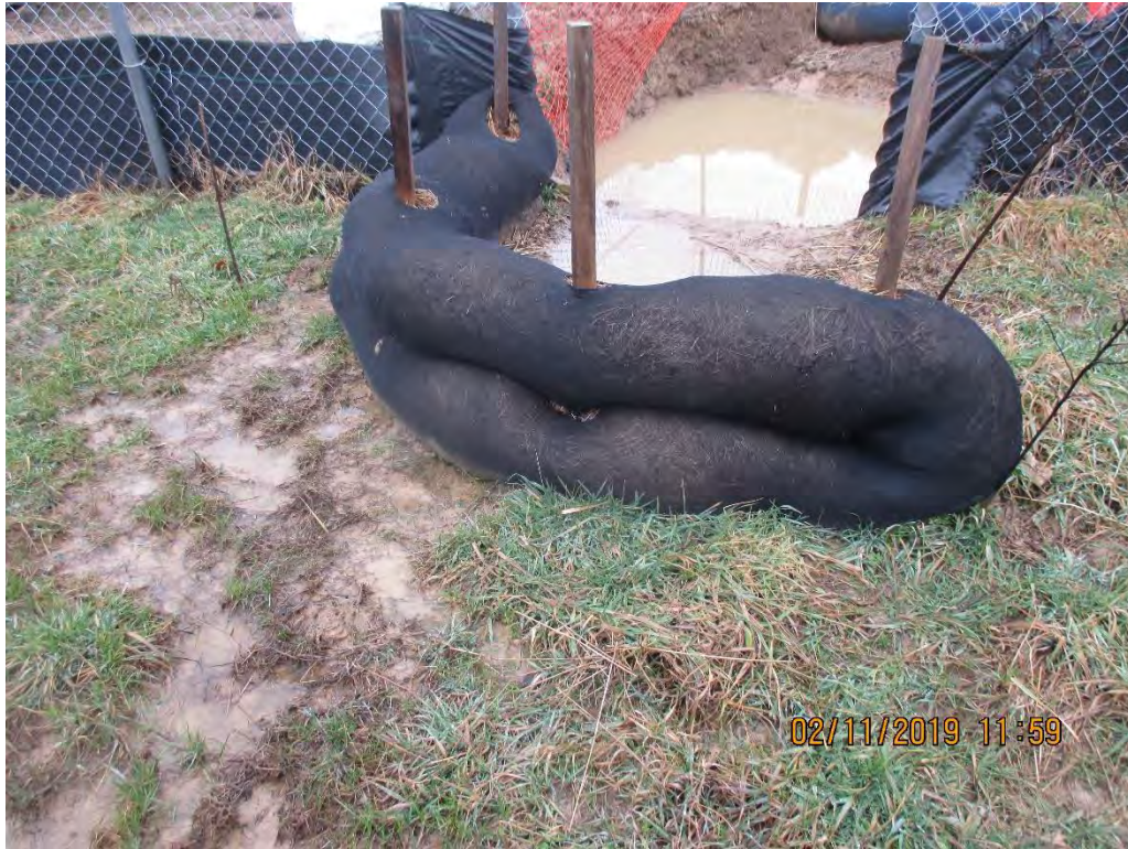
Waterbar terminus near station 5985+50, Sediment deposits and SLW present.
