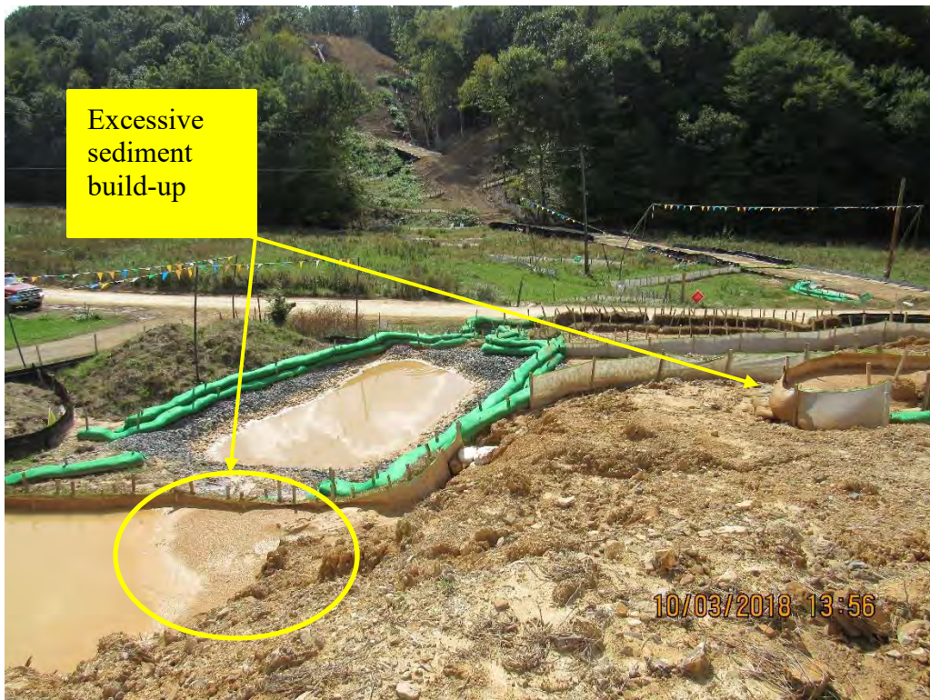
Photo 2: Unacceptable amount of sediment in sumps after maintenance performed at Painter's Run station 10270.
