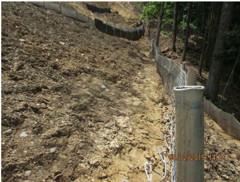
Controls below where dozer work was taking place. Sediment deposits observed below these controls at station No. 9780+00.
