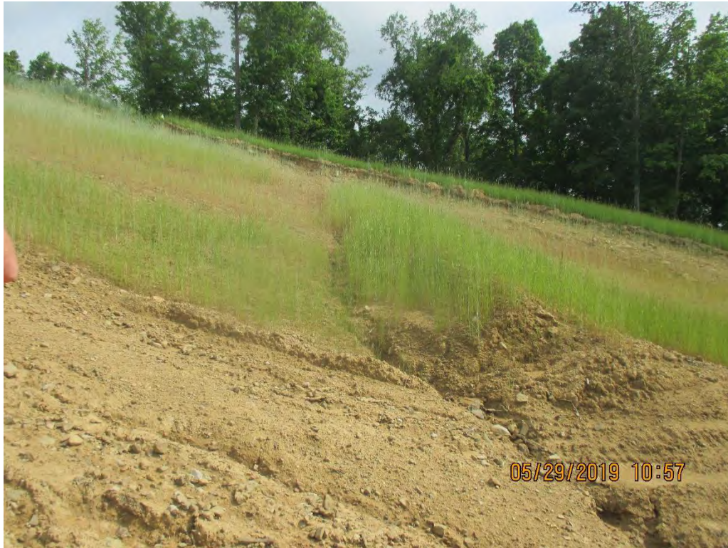
Facing towards cut in slope/ROW at station No. 4031+00. Waterbar had erosion present.
