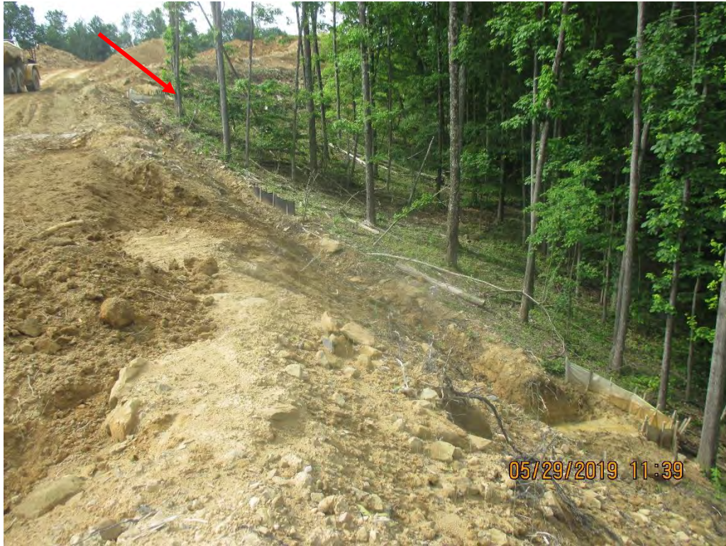
Facing upslope near station No. 4027+00. Arrow depicts Waterbar and where sediment deposits were observed. Diversion berm installed as perimeter control with multiple outlets present.
