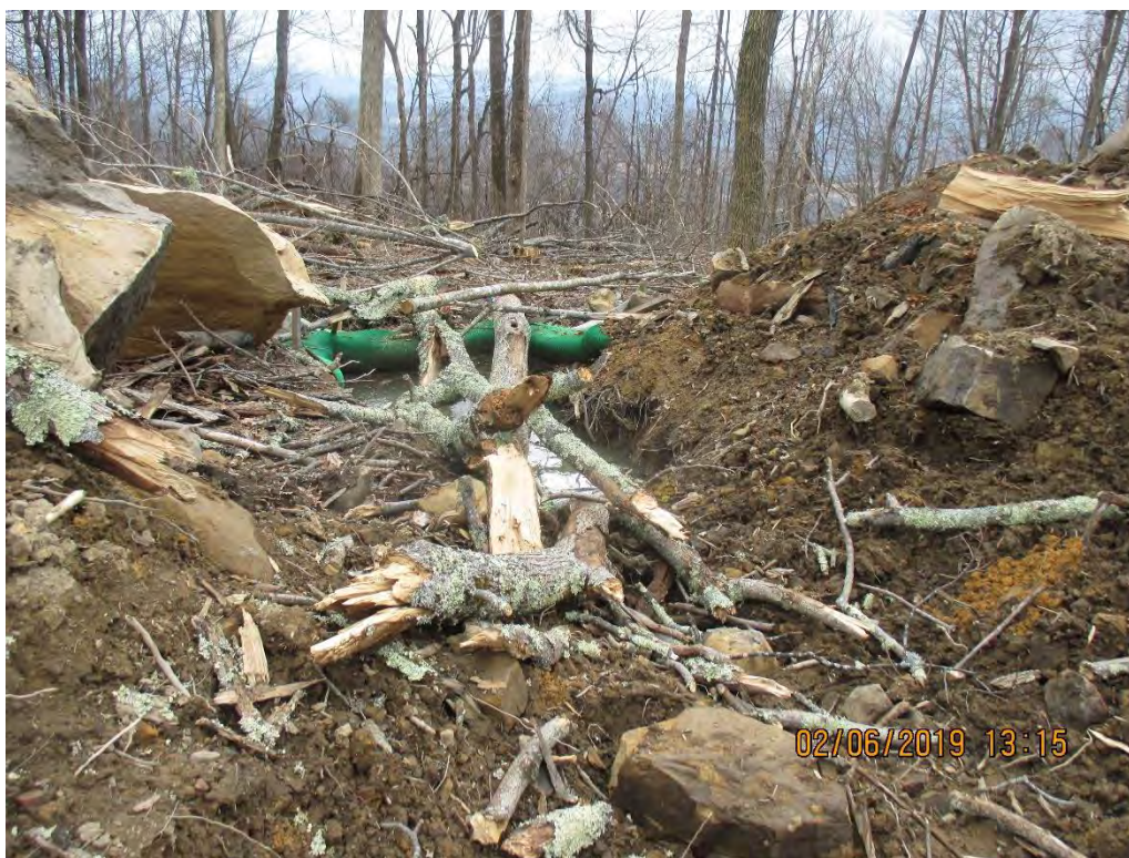
Waterbar outlet at station number 8795+00 with tree limbs present due to past ice storm.
