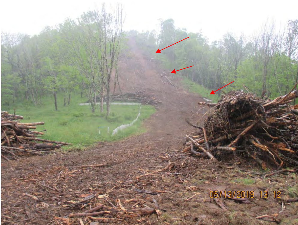
Facing upslope near station #8399+10. Controls were in place at time of inspection at Waterbar outlet per SWPPP. Arrows depict Waterbar outlets.
