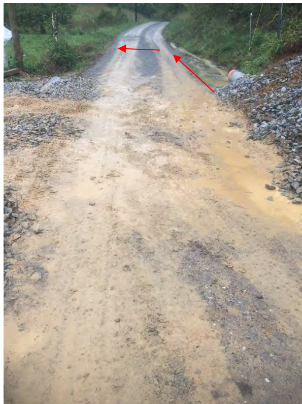
Photo depicting SLW flowing through culverted stream crossing and under road through culvert and into stream on other side of Ellison ridge road. Mud also present on road.
