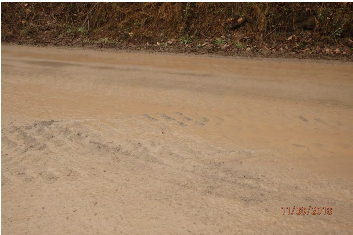
Access Road WV-HA - 29.5 off CR 50/5 showing the lack of an adequately stable construction entrance and the associated track out onto the public road.
