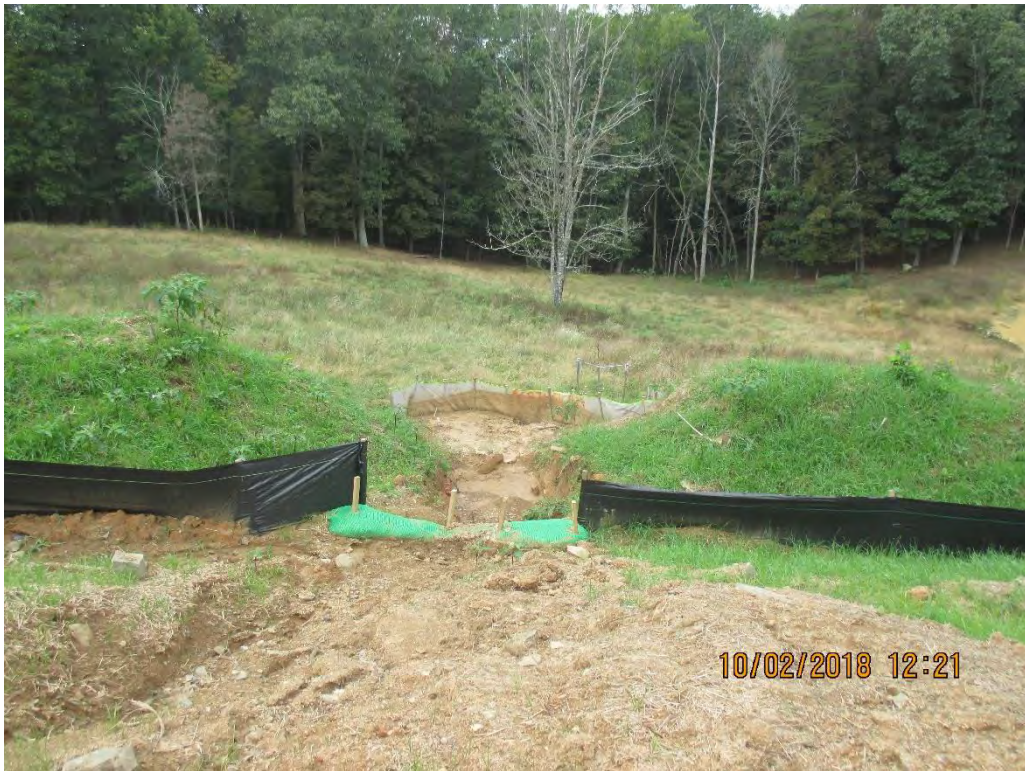
ROW near station #9687 where BMP is failing.
