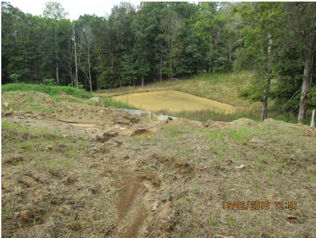
Gully erosion occurring near Station #9687 and flowing towards Pond (P-D2). BMP pictured was failing and off-site sediment deposits were present past the LOD.
