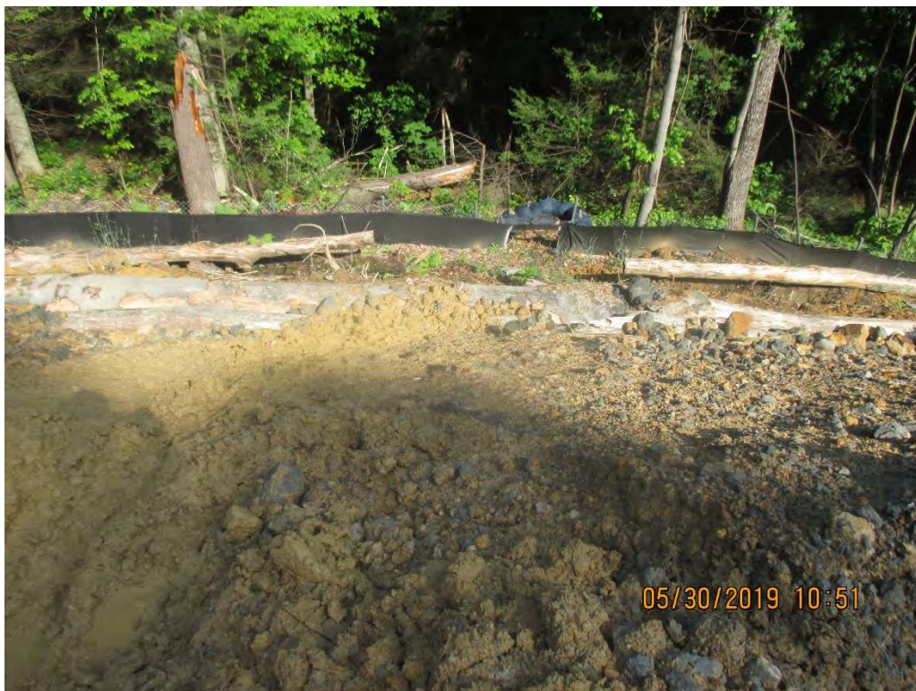
Waterbar outlet terminating onto slope at station No. 6485+10. Erosion present on slope above perimeter controls.
