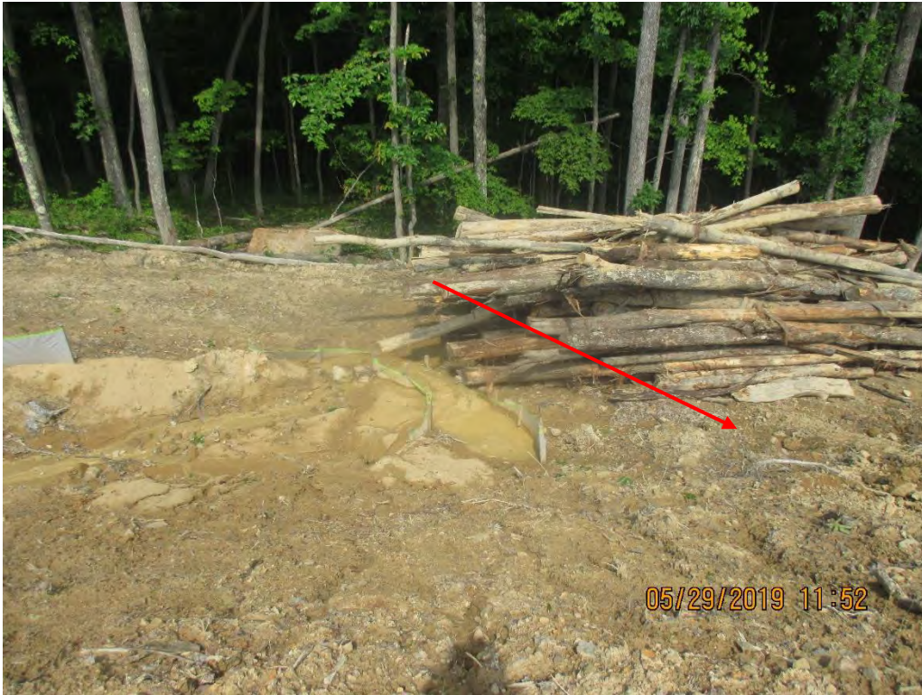
Below Waterbar outlet near station No. 4017+00. Evidence that sediment laden water flowed past LOD was observed. Arrow depicts where run-off was flowing.
