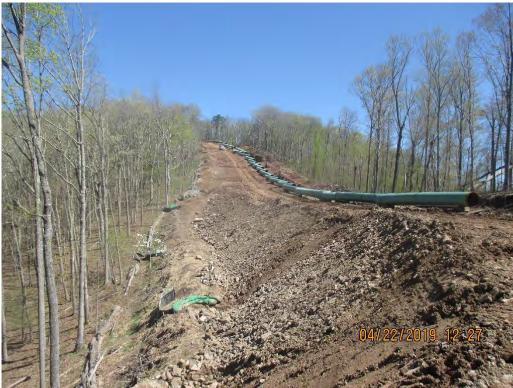
Near station #9015 facing North. Berm installed as perimeter control on downslope section of LOD.
