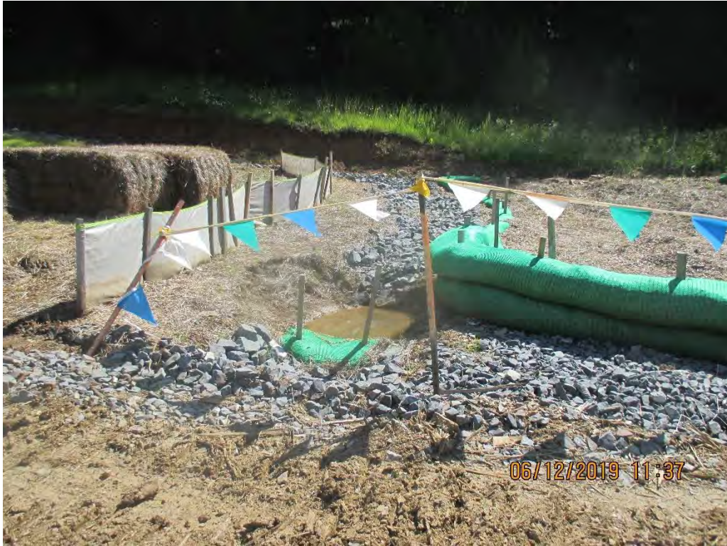
French drain installed at base of cut slope. Drain terminated into sump with controls and conveys under ROW to outlet that has sump present with controls.
