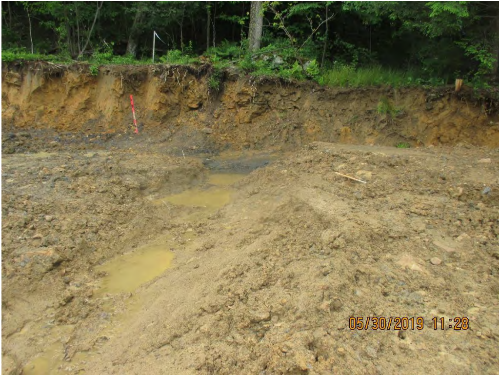
Seep running onto ROW above Stream S-N13. Diversion not stabilized near station No. 6940+00.
