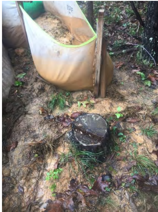
ROW near station numbers 9779+00 and 9778+00 where water bar outlets were being overwhelmed and SLW was passing through and under and being transported past LOD.
