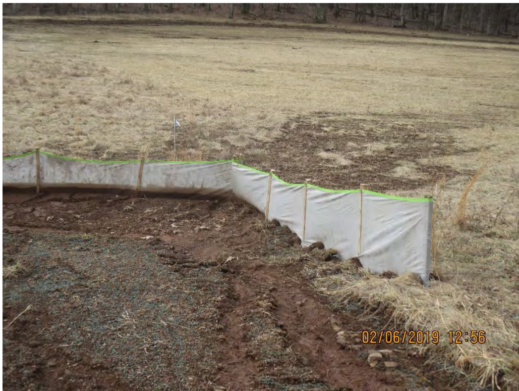
Waterbar termini at station #8780+00 facing South. Evidence of concentrated flow due to absence of vegetation past LOD.
