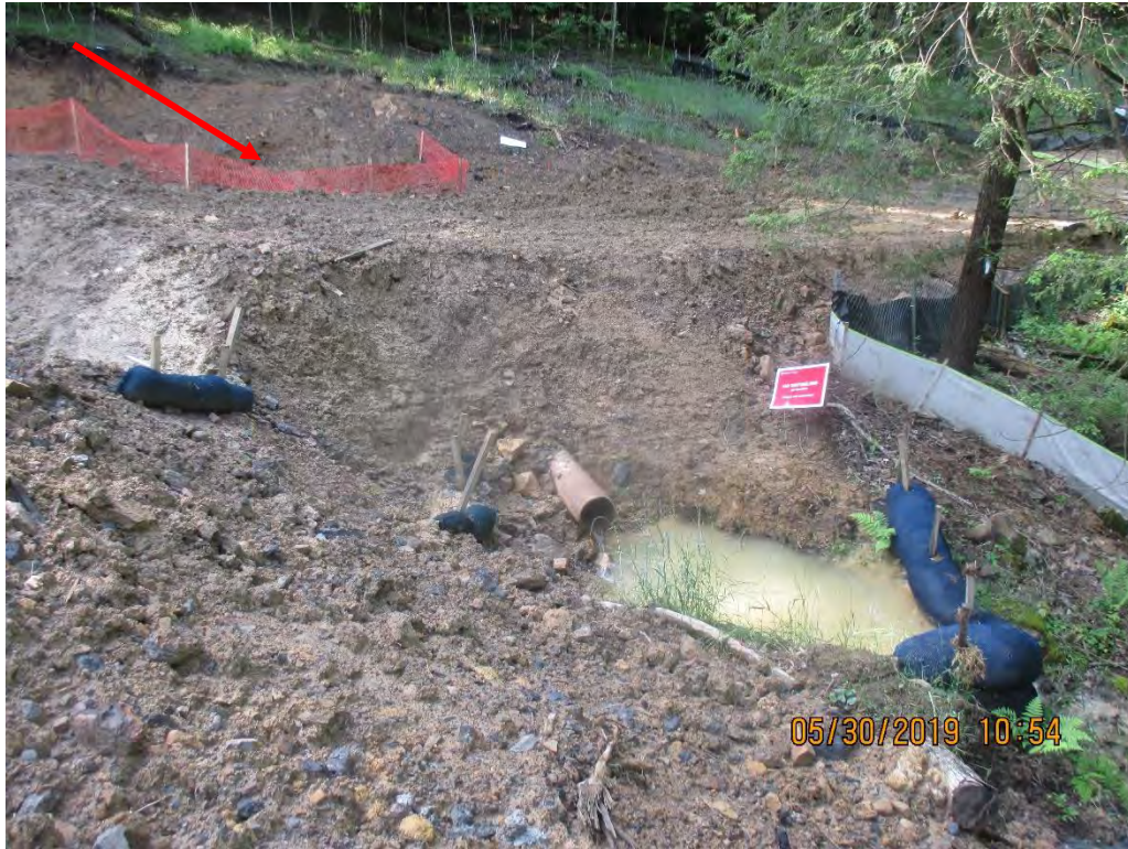
Sep drain outlet above Stream S-EE1. Clean water diversion not stabilized above or below inlet/outlet. Clean water was being conveyed approximately 15 foot across disturbed soil to a sump where the inlet was located. The topsoil pile around the inlet was eroding into the sump. Arrow depicts where inlet was located.
