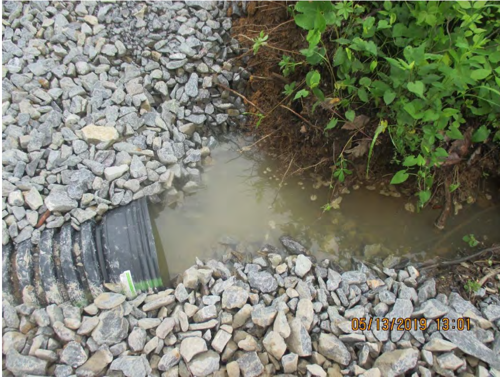
SLW present upslope of MVP ROW entrance entering installed culvert and conveying to ponded area in ditch line.
