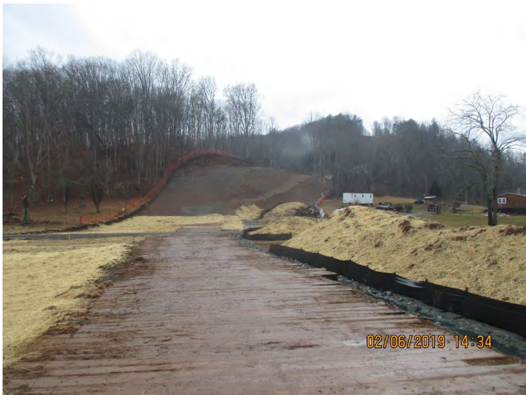
Boom Hollow Road (CR 6/2) Crossing near station number 8966+00 facing North at MVP ROW.
