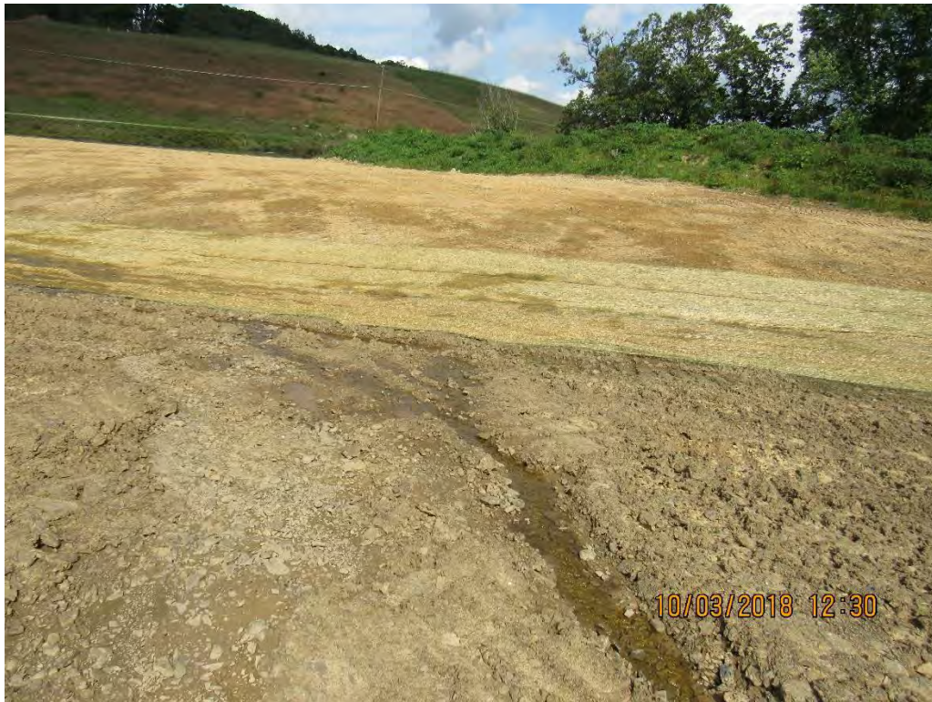
Photo 7: Run on water lacks established channel through site at Lindsie Methodist Church station 10116+49.
