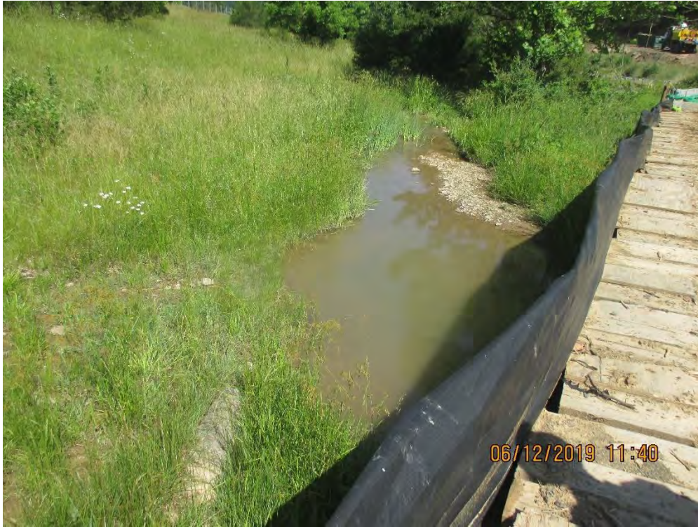
Anne's Branch crossing near station No. 9744+00 facing downstream. Past disturbance observed from land owner traffic across stream.
