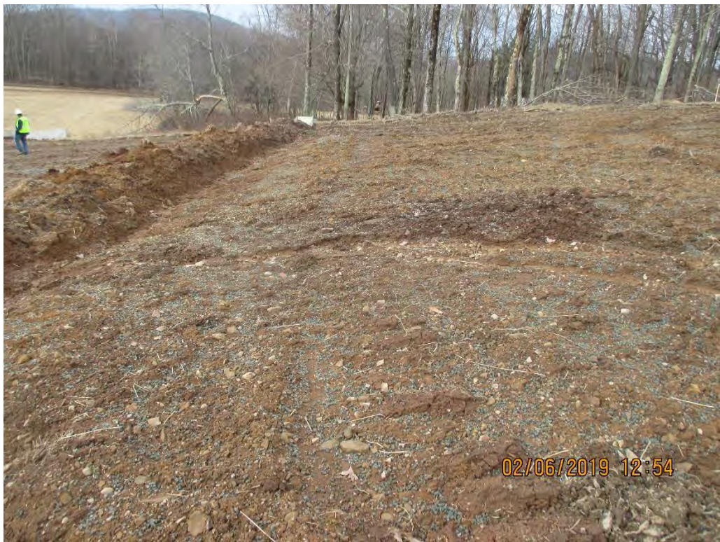
Facing West towards water bar terminus at station #8780+00. Rill erosion occurring between waterbars.
