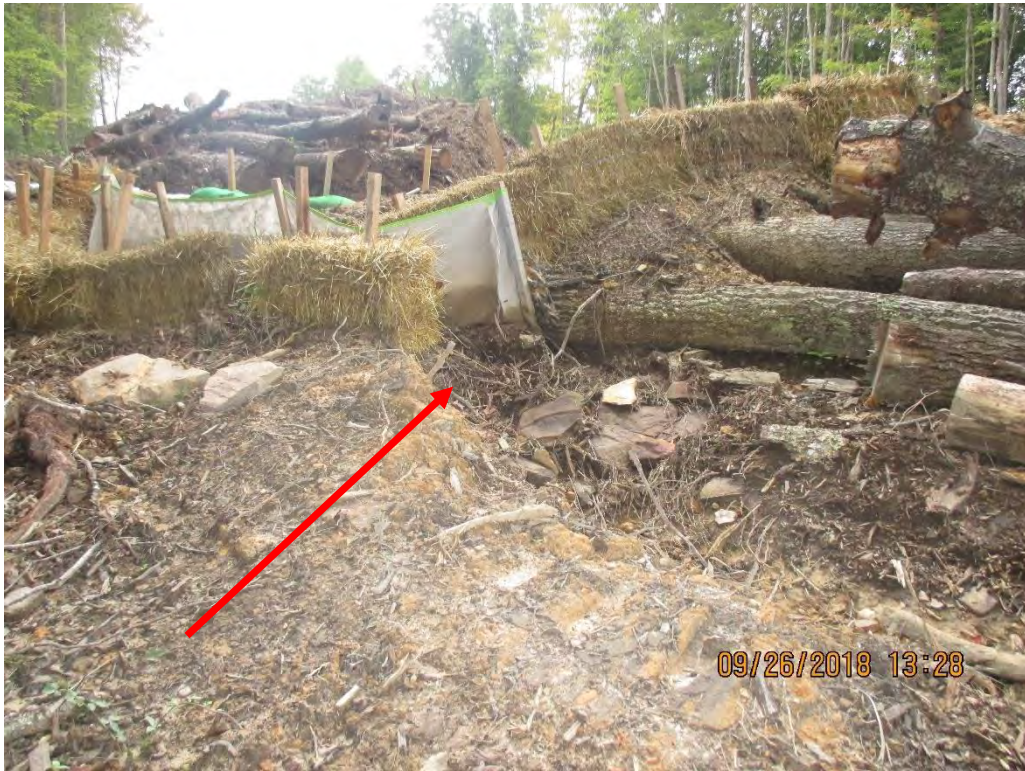
Arrow depicts where BMP was being undermined near Station number 9899+00.
