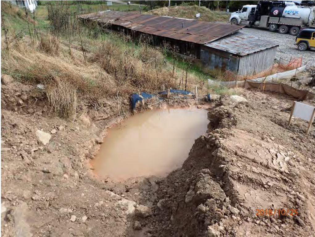
Overwhelmed sump near Sams Run.
