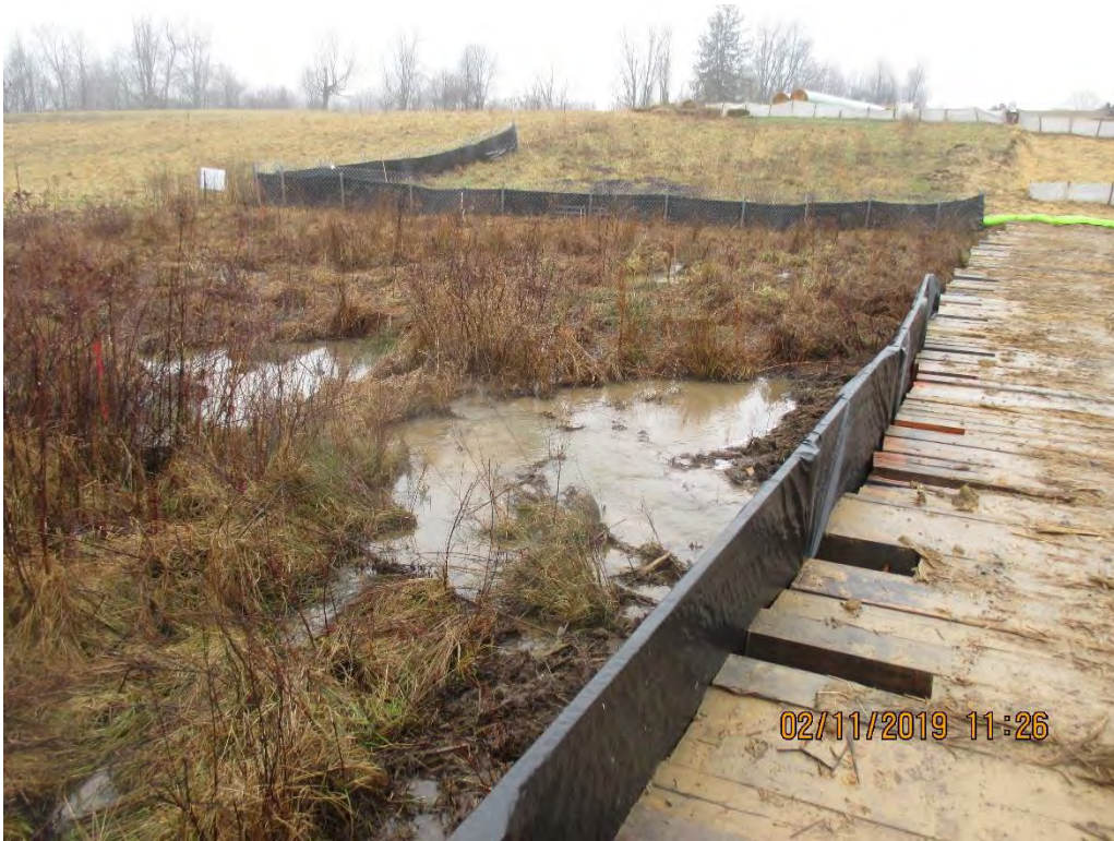
SLW present in Wetland W-B-26 at crossing facing West.
