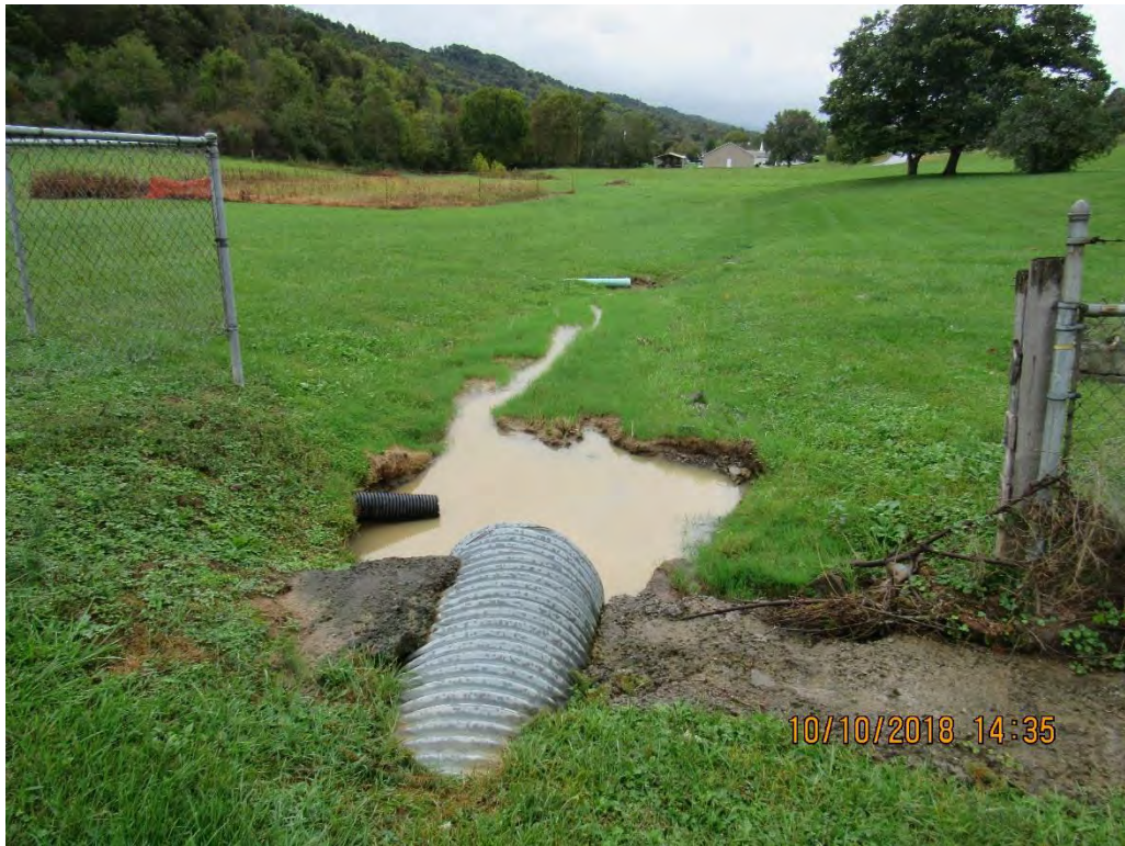
Photo 19: Culvert on west side of Lindside Methodist Church station 10116- unable to determine location of sediment.
