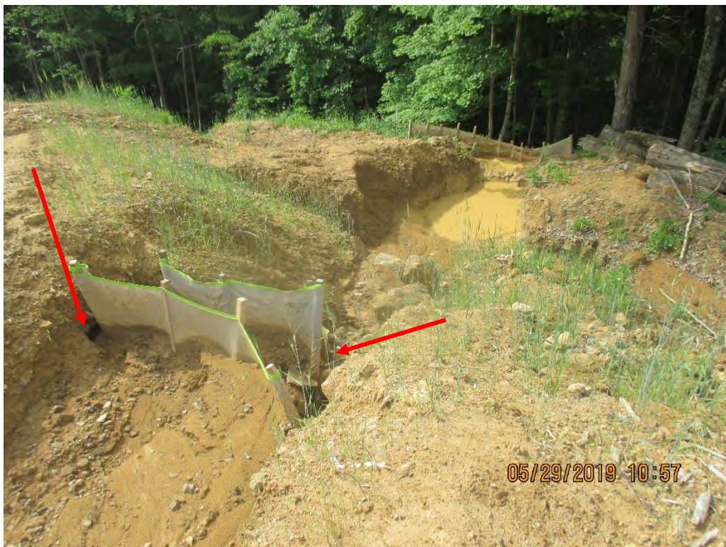
Waterbar outlet and diversion berm outlet at station No. 4031+00. Sediment was being deposited behind controls. Arrow depicts where runoff was flowing around controls.
