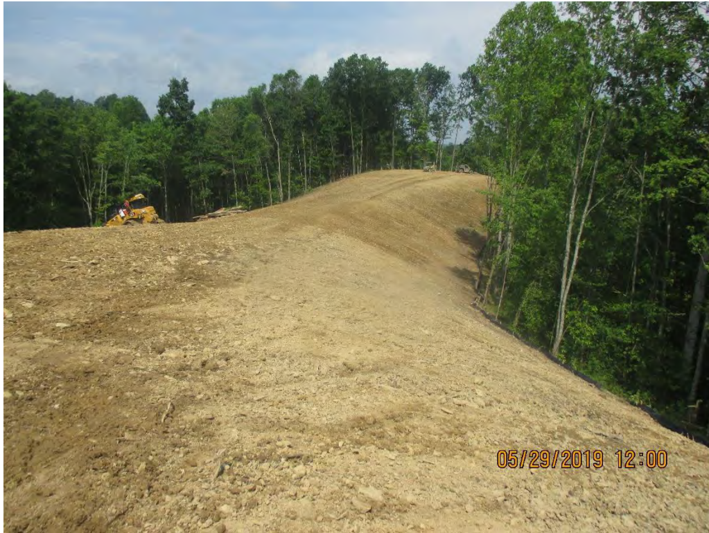
Facing South at station No. 4017+00. ROW was actively being restored to final grade.
