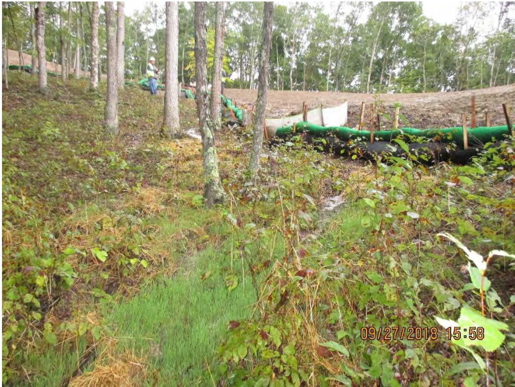
Areas near station number 9417+75 where water bar terminus being overwhelmed with SLW.
