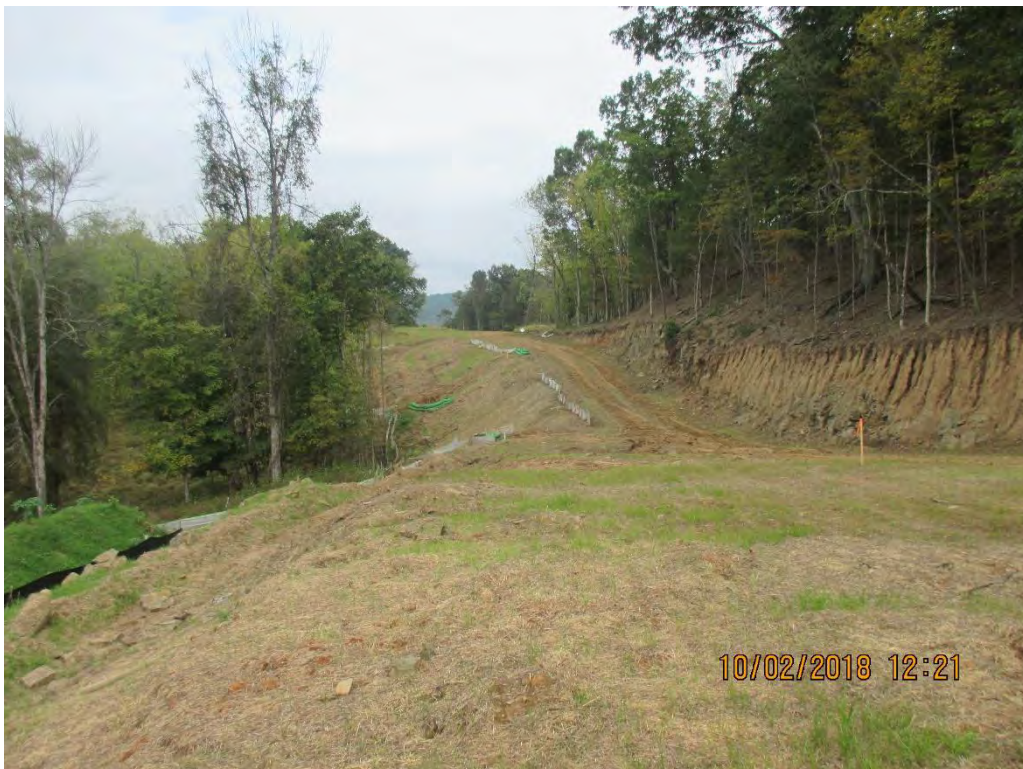
ROW near station #9687 where multiple BMP's are failing.
