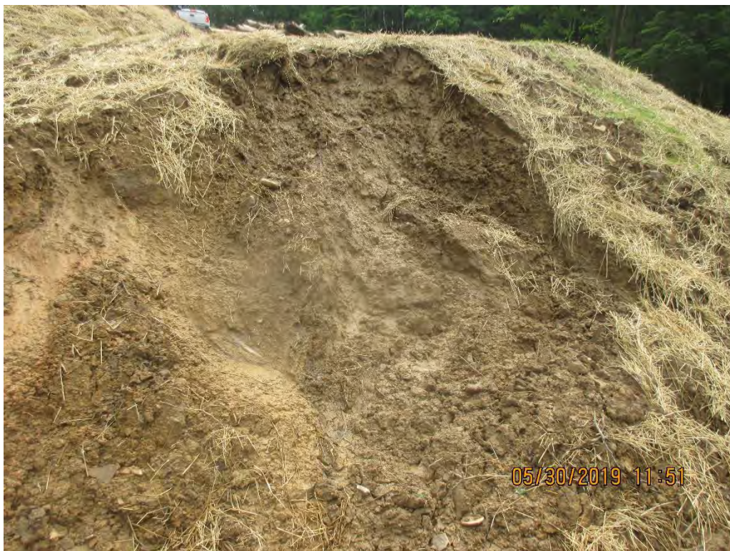
Topsoil pile slipping into Waterbar at station No. 6508+40.
