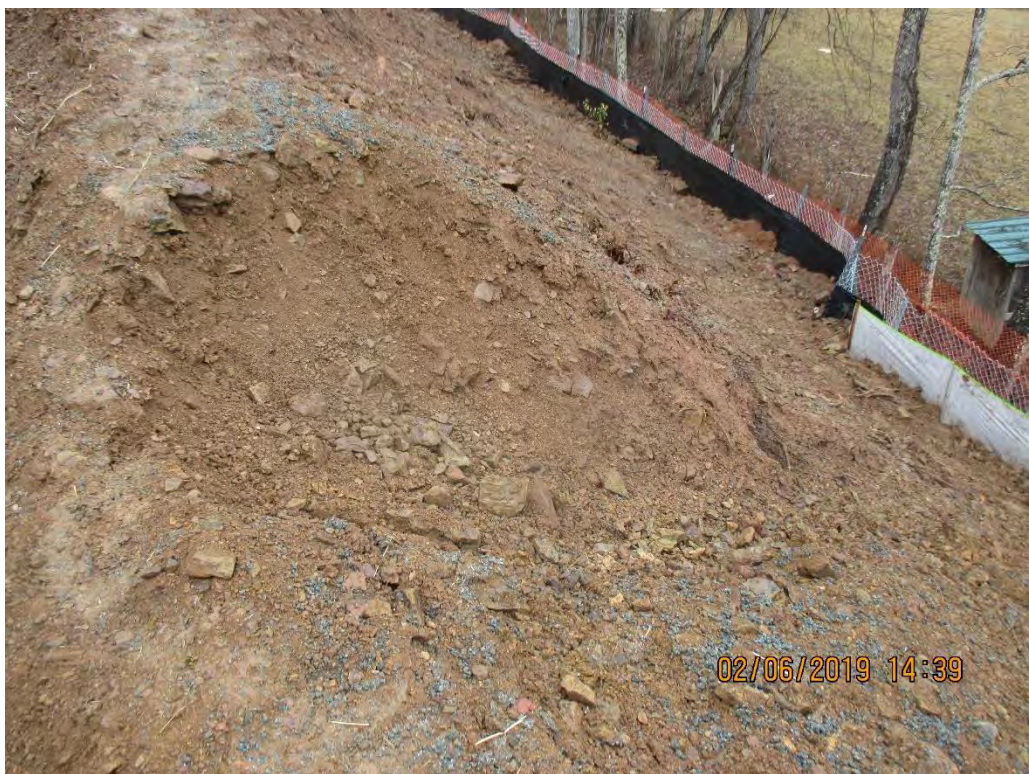
Small slip on side slope near station number 8966+00.
