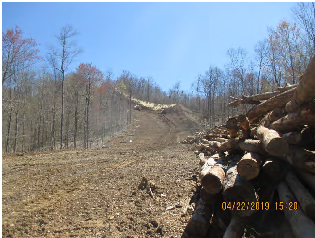
Facing South towards slope that had Waterbar failure near station #8628+00.
