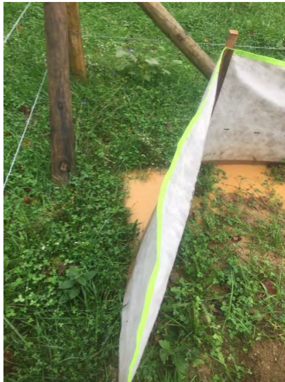
SLW flowing under and through BMP near station number 9784+00.
