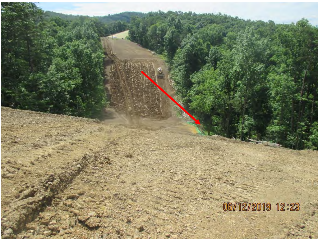
Facing South near station No. 9745+00 on North side slope. Arrow depicts location of Dargo silt fence.
