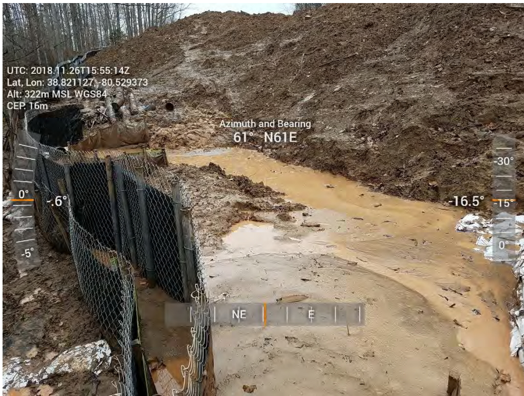
Photo 5: Temporary repairs installed prior to permanent repairs at reported slip. Photo supplied by EI Andy Pauley.
