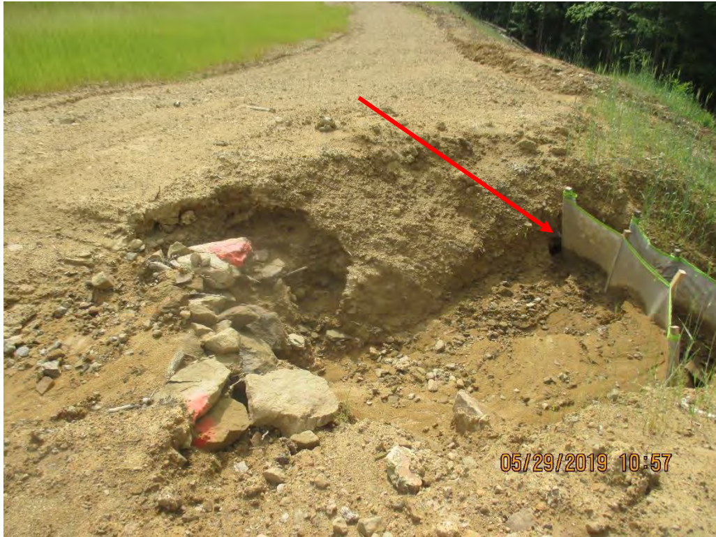
Waterbar outlet at station No. 4031+00. Arrow depicts where runoff was flowing around control and causing increased erosion.
