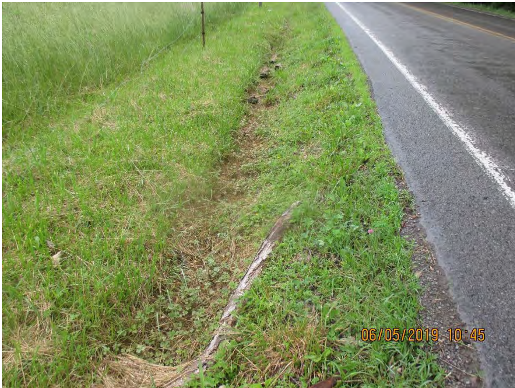
Upslope of culvert intake that conveys under route 82. No sediment deposits present at time of inspection.
