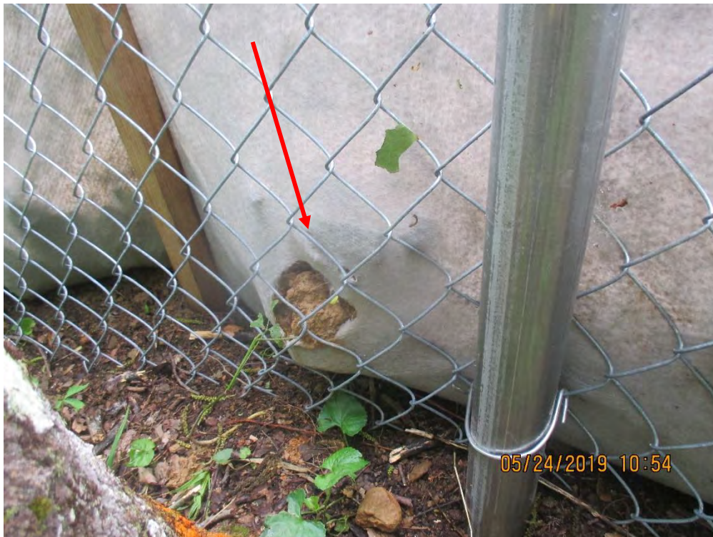
Near station No. 8410+00. Hole present in P1 silt fence due to material slipping into controls.
