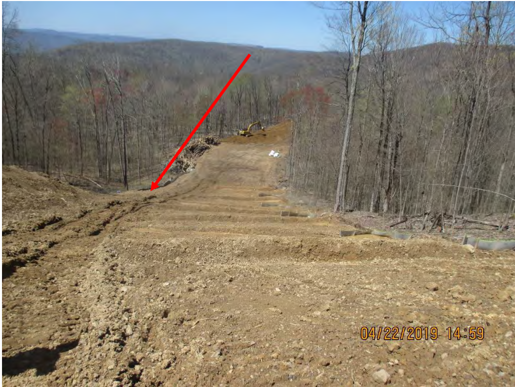
Standing above station #8633+71. Arrow depicts where Waterbar conveyed sediment into Stream S-T35(A).
