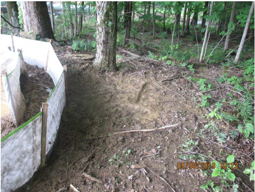
Facing downslope towards Stream S-N10. Scouring of vegetation and sediment deposits were observed below these controls.
