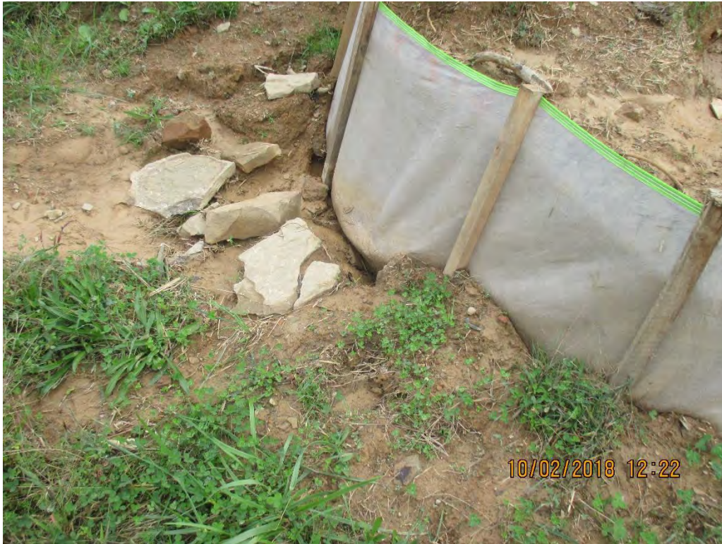
Above mentioned BMP being undercut from run-off.
