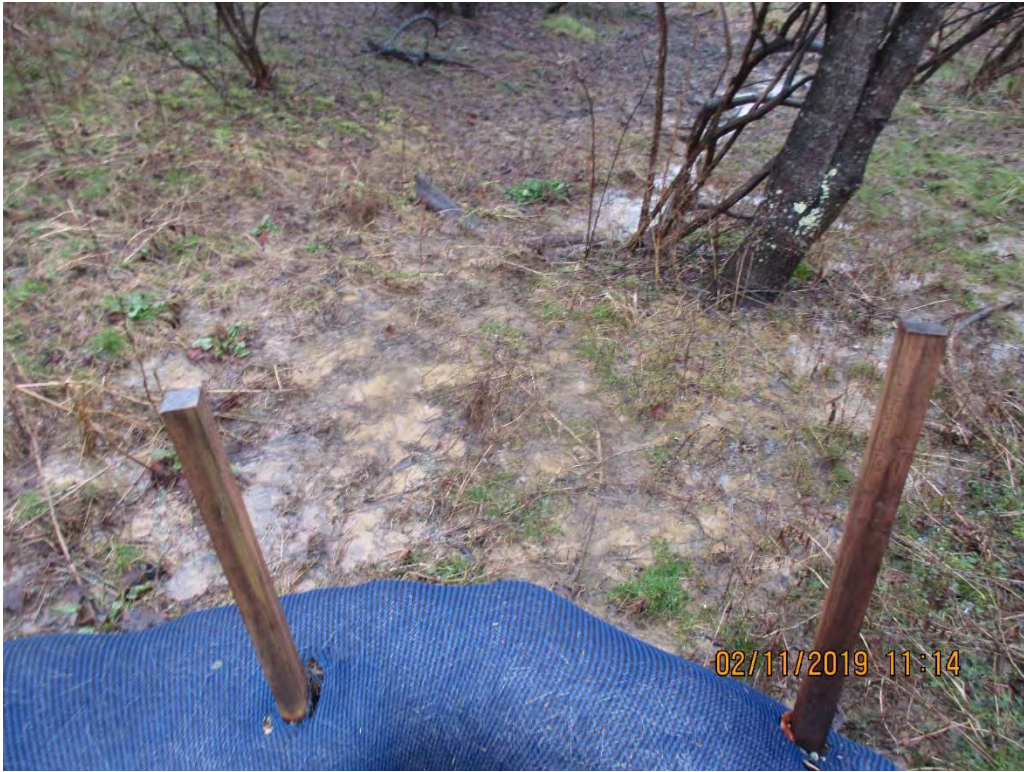
Evidence of sediment being deposited past LOD near station #6017+50
