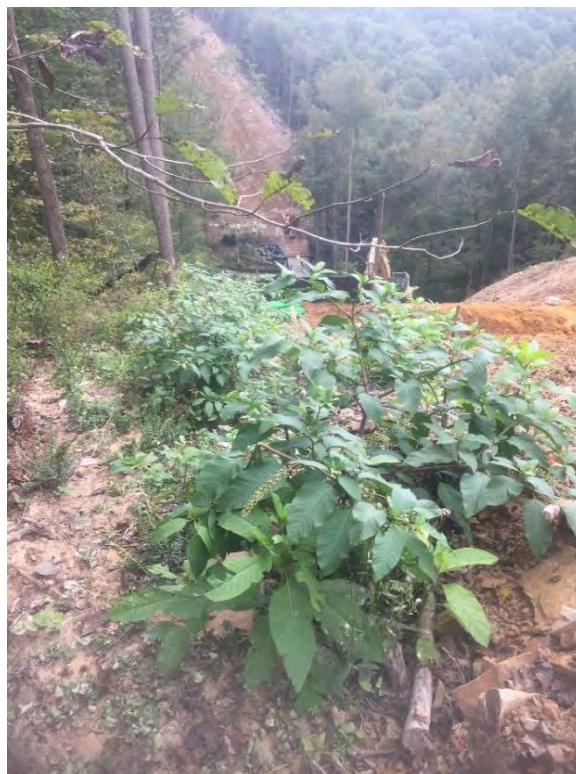
Near Station # 9911+00 where BMP was being overwhelmed and off-site sediment deposits were observed.
