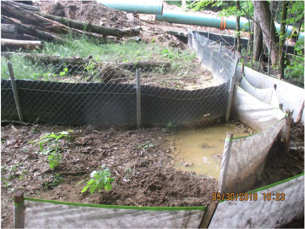
Controls at station No. 6474+16. Recent enhancement was observed.
