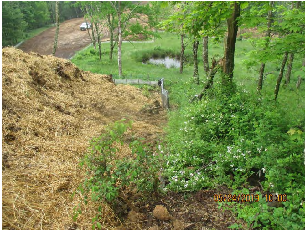
Facing downslope along MVP LOD near station No. 8387+96. Controls in place at edge of LOD approximately 75 feet downslope.
