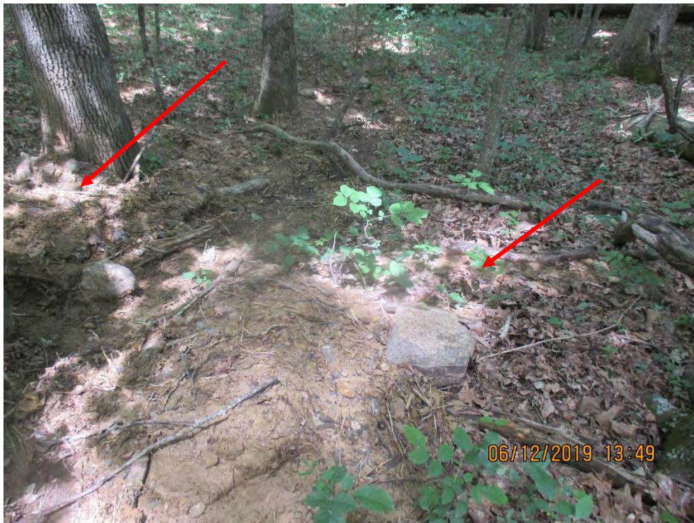
Sediment Deposits below and past controls/LOD at station No. 9780+00. Arrow depicts deposits.
