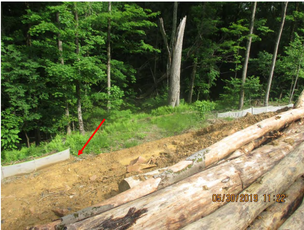
Station No. 6497+50. Perimeter controls not installed per SWPPP. Diversion berm installed however, arrow depicts section where sediment was being deposited against controls and not tied into berm.
