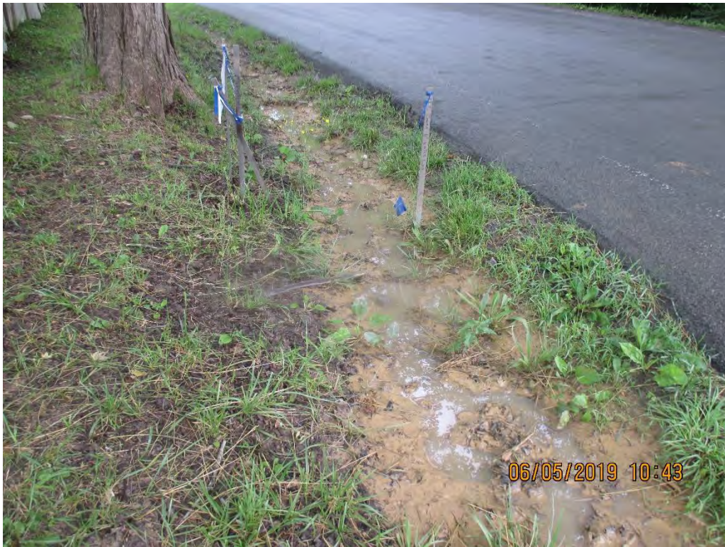
Sediment deposits and sediment laden water being conveyed past the LOD along Route 82.
