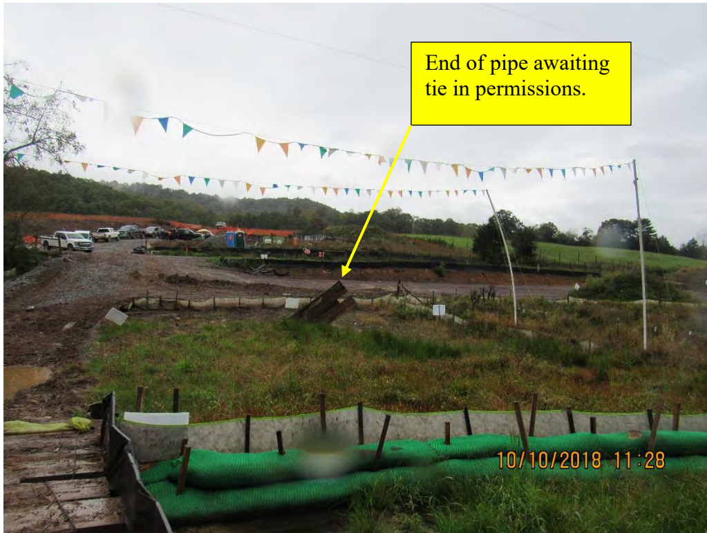
Photo 11: Wayside/Talcott station 9466 with matting indication end of pipe awaiting USACE permission for tie in.
