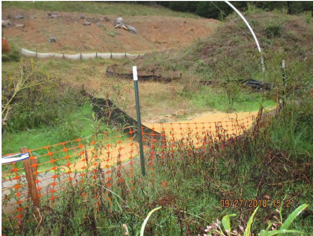
Lack of fill slope protection causing erosion and sediment laden water to accumulate and overwhelm BMP.
