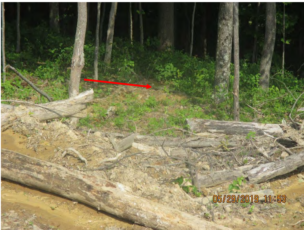
Below perimeter controls near station No. 4017+00. Sediment deposits were present past LOD.
