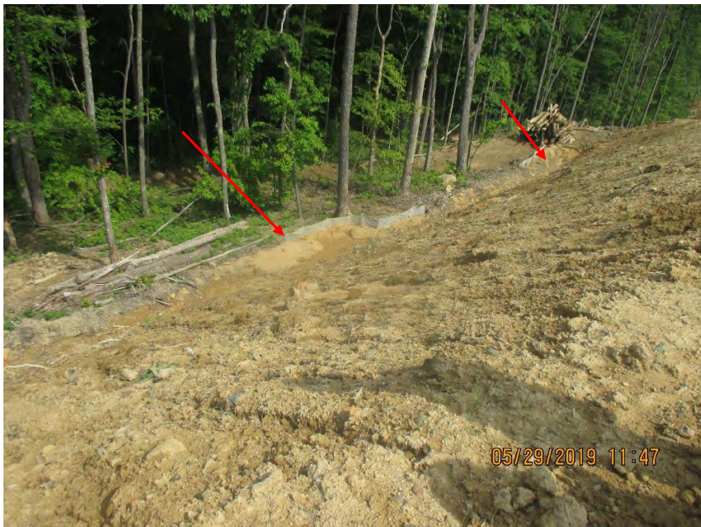
Erosion present on slope near Station No. 4017+00. Perimeter controls overwhelmed with sediment.
