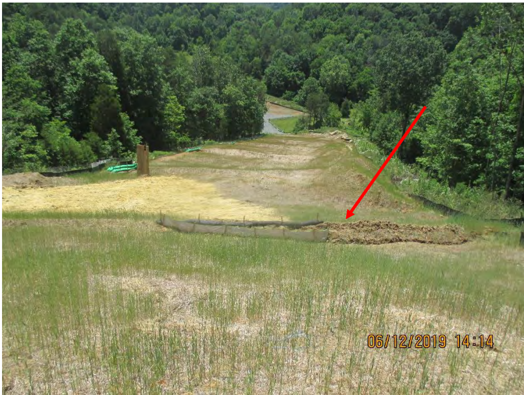
Facing South towards Ellison Ridge Road. Waterbar blow out and repair observed where AR-221 comes onto ROW.
