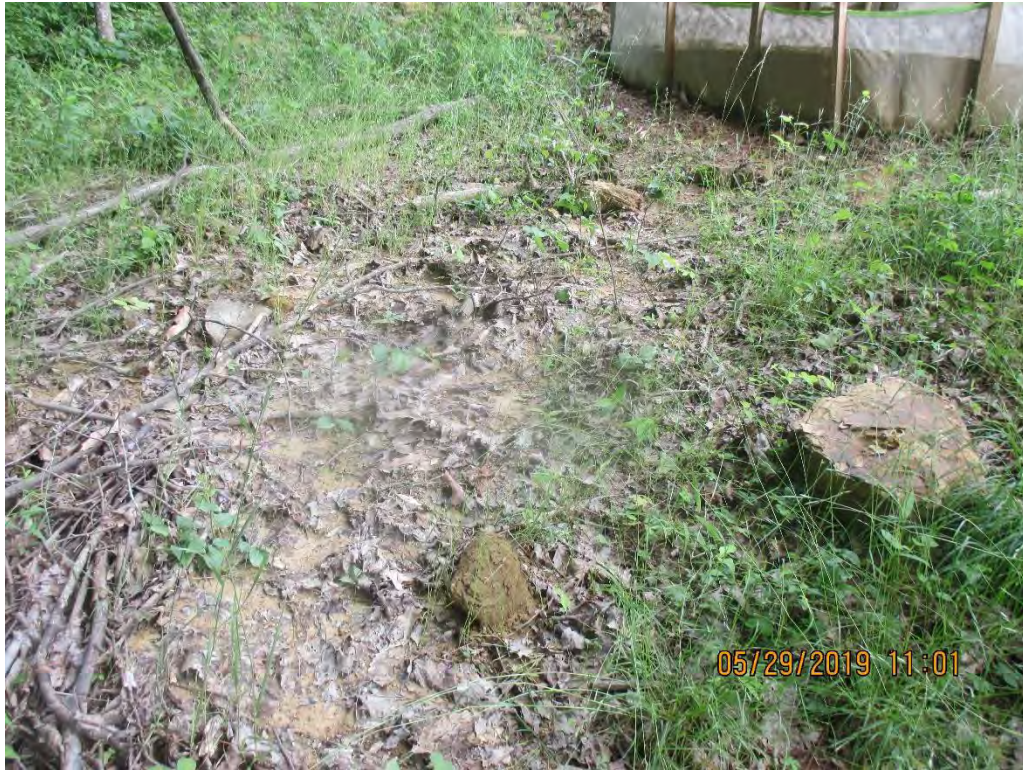
Standing below diversion berm outlet No. 2 near 4031+00. Scouring of vegetation present below control.
