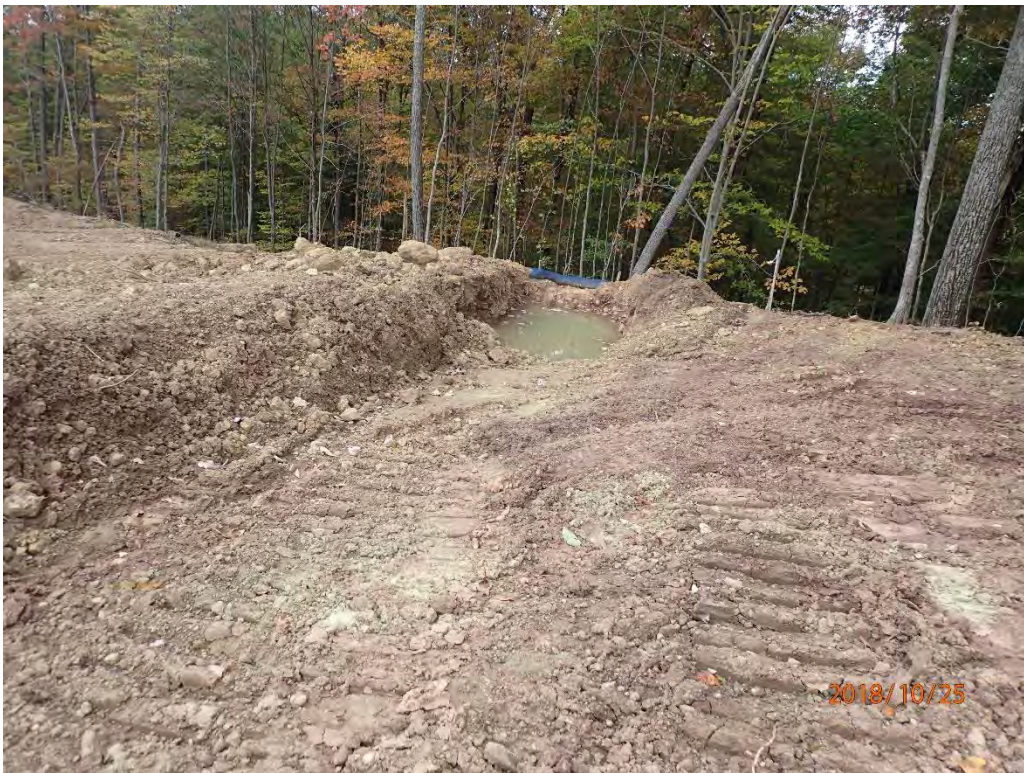
Sump at Station 286 in need of maintenance.
