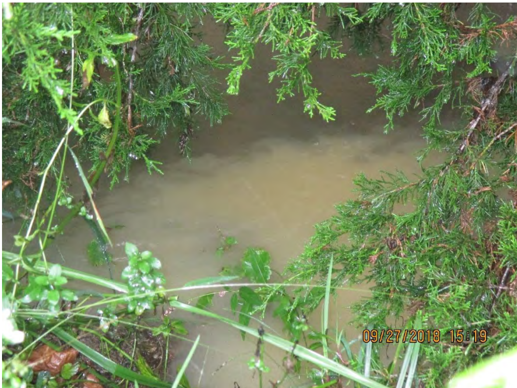
Sediment Laden water leaving project and entering stream (S-A60).
