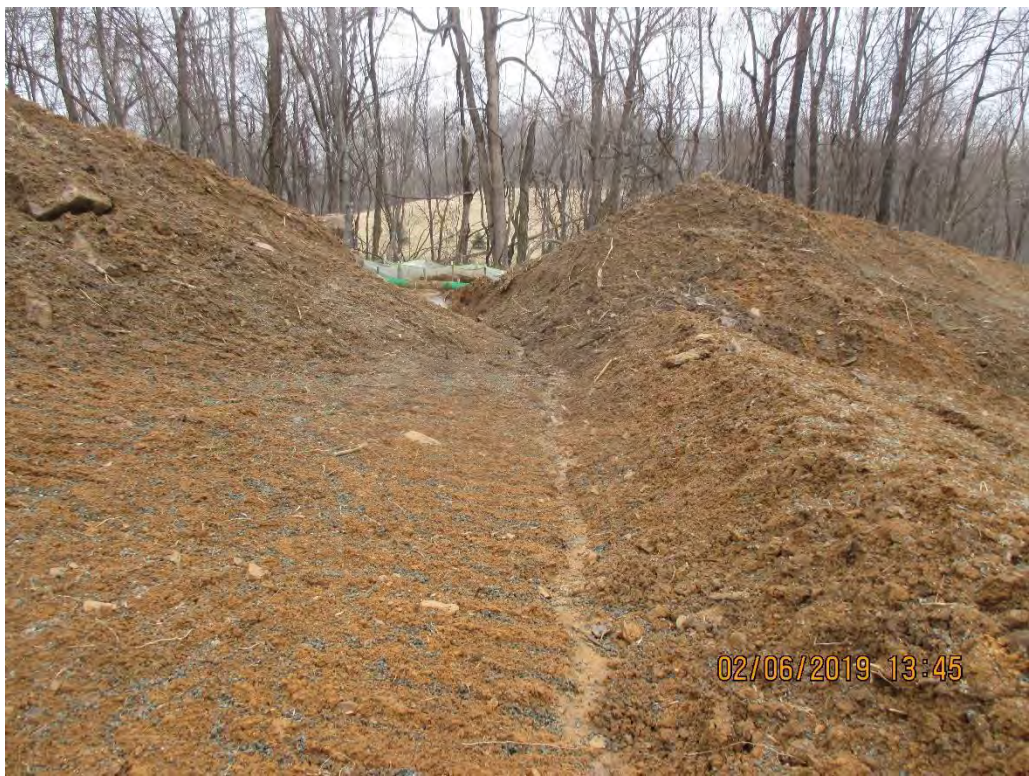
Waterbar outlet at station number 8816+00.
