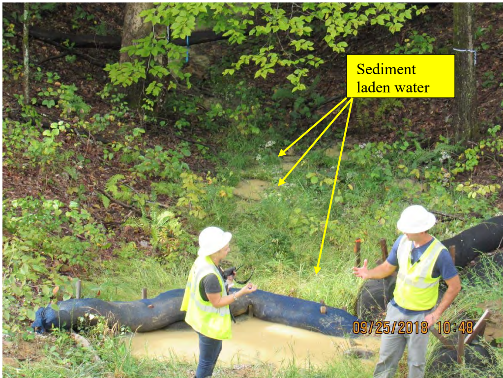
Photo 2: Station 550 sump at base of fill slope where perimeter controls failed and sediment laden water leaving site.
