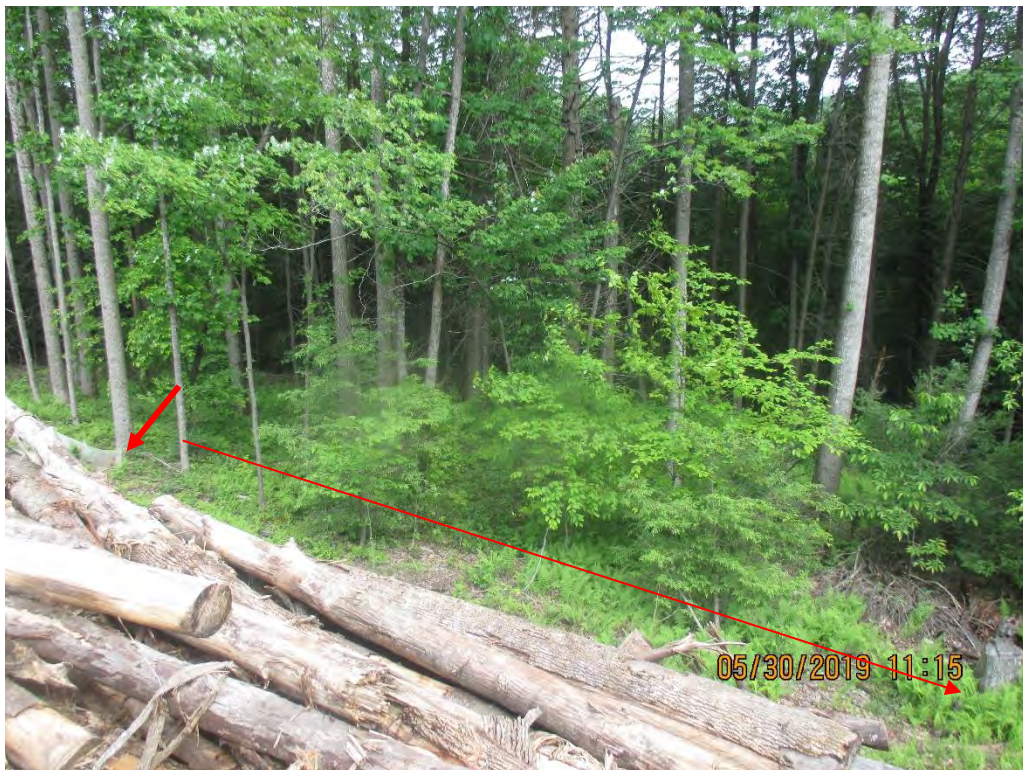
No perimeter control installed per SWPPP on downslope side of fill slope at station No. 6495+00.
