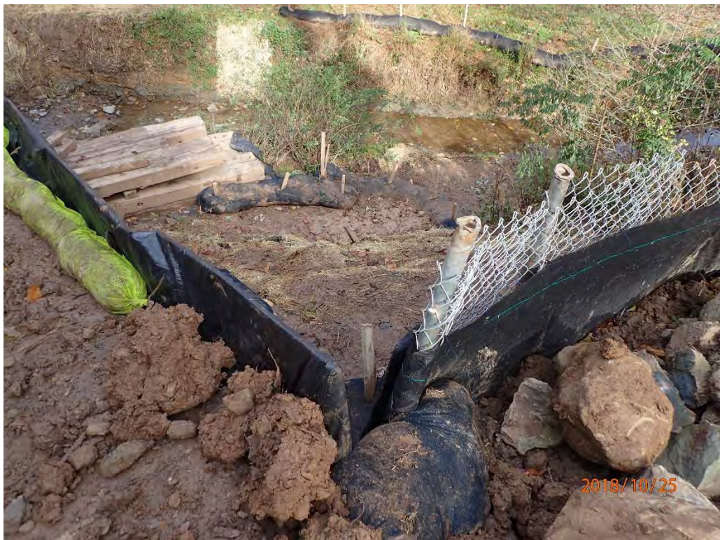
UNT of Mobley Run - There was sediment build up near the silt sock close to the stream. Contractors replaced the silt sock during the inspection.
