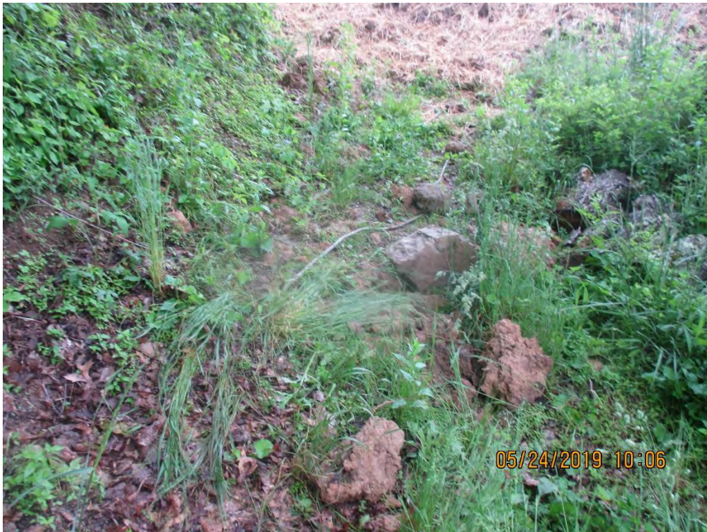
Facing towards MVP LOD near station No. 8387+96. Material had slipped from pile off ROW past LOD. No perimeter controls in place.
