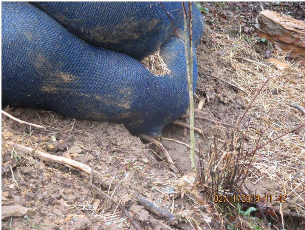
CFS at waterbar terminus near station 5999+50 showing signs of being undermined due to concentrated flow
