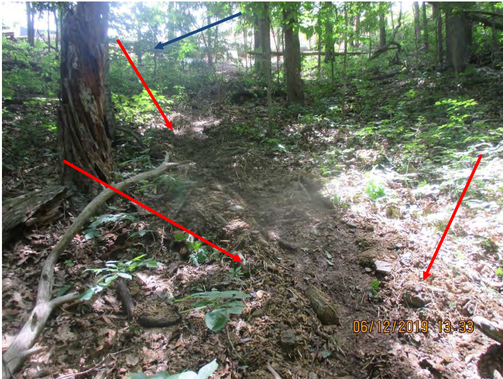
Scoring and sediment deposits below controls at station No. 9780+00. Red Arrow depicts deposits. Blue arrow depicts controls at edge of LOD.
