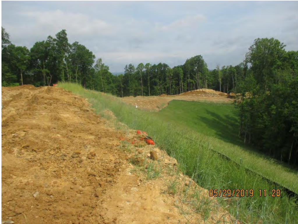
Standing at station #4031+00 facing South at MVP ROW and western edge of LOD.
