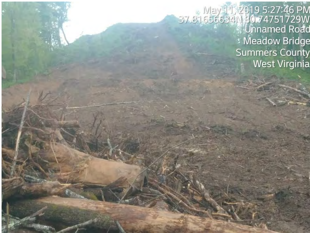
Photo of steep slope near station #8399+10 depicting no controls in place on 5/11/19 at 5:27pm
