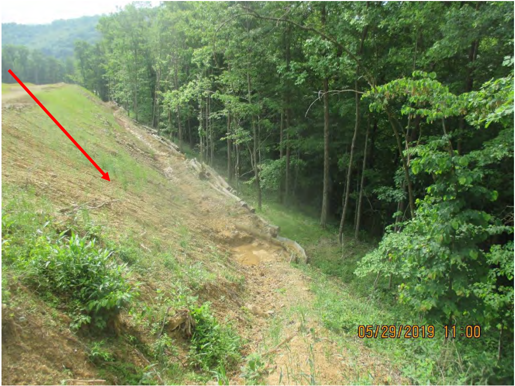
Near station No, 4031+00 facing downslope at diversion berm outlet No. 2. Arrow depicts Erosion present on fill slope.
