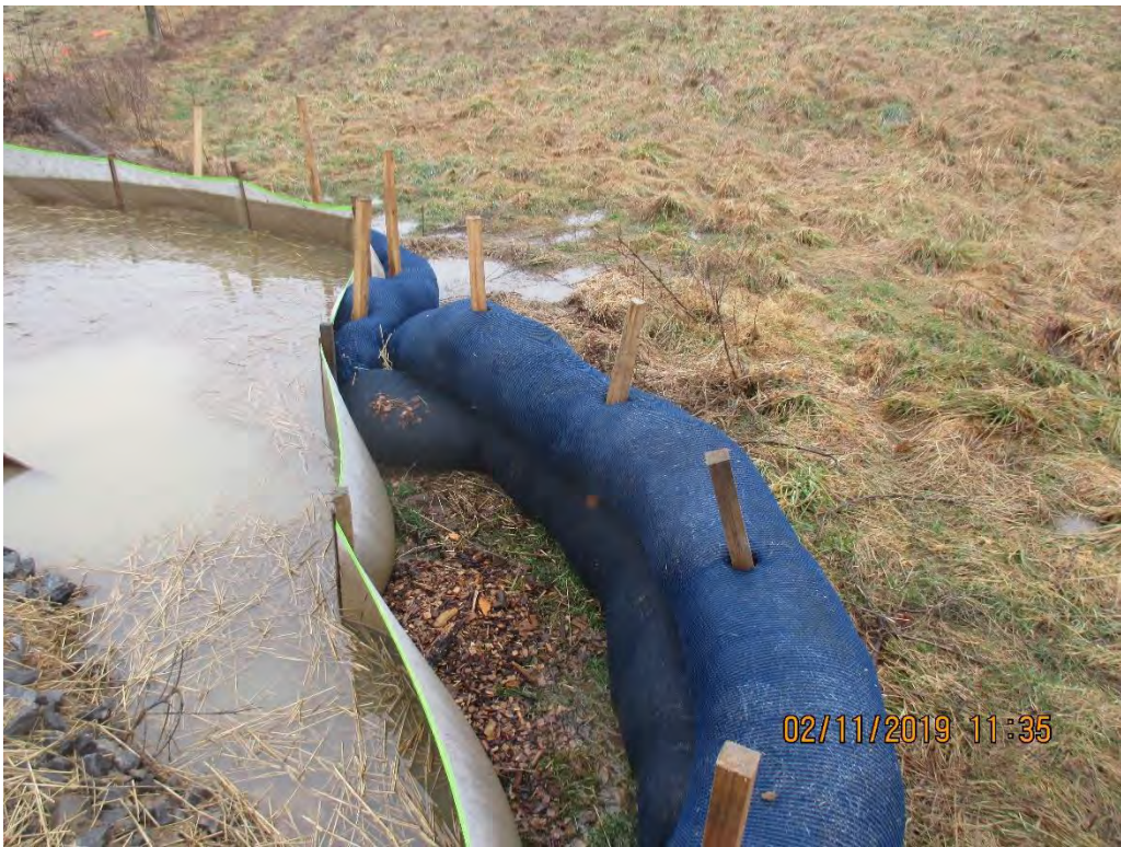
Culvert terminus on Access Road MVP-IN-141.01 opposite angle from backside of control
