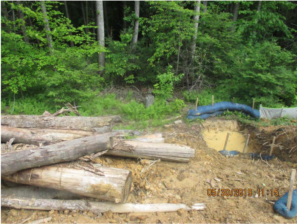
Same area near station No. 6495+00. Perimeter controls not extended per SWPPP into outlet controls.
