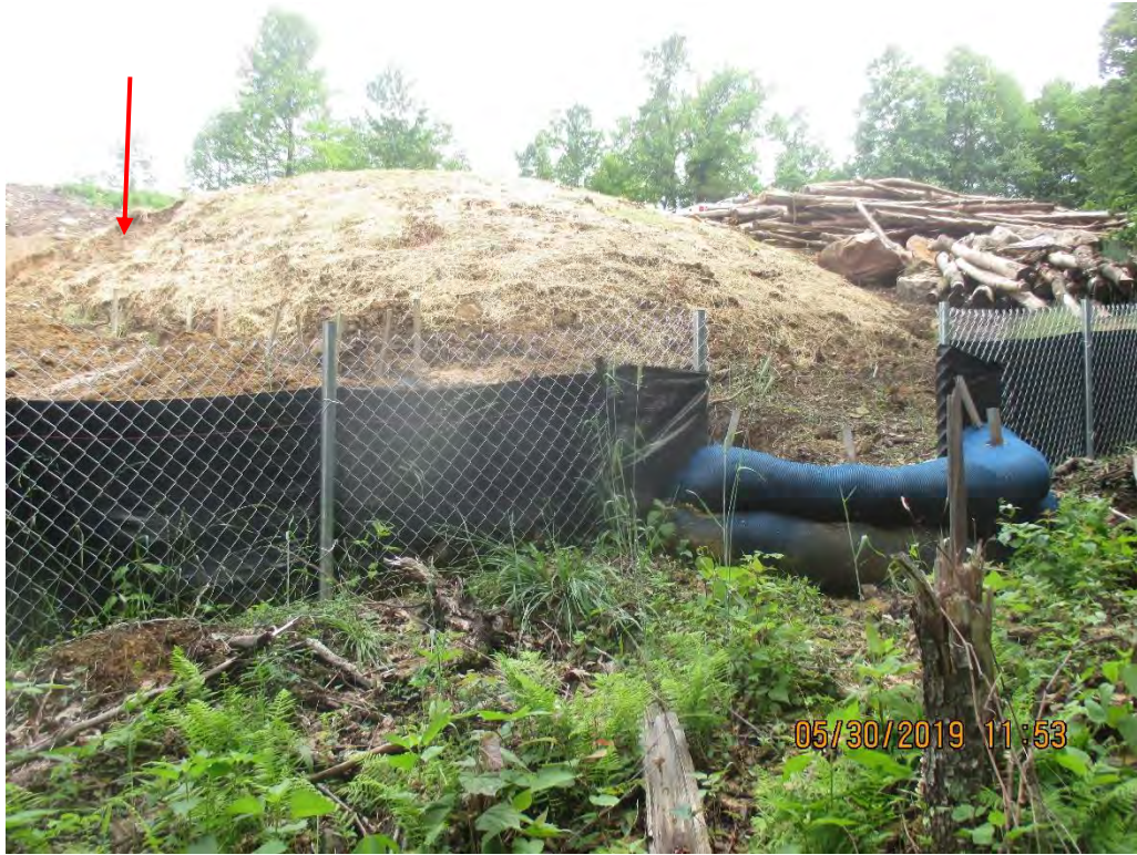
Facing upslope at Waterbar and topsoil pile at station No. 6508+30. Arrow depicts topsoil pile that is slipping into Waterbar.
