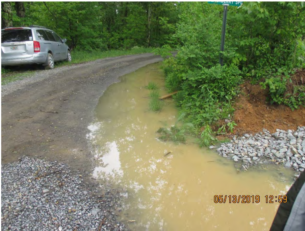
SLW ponding in ditch downslope of MVP ROW construction entrance.
