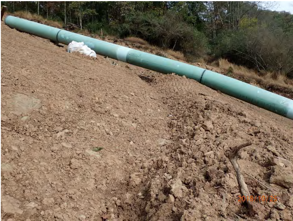
Damaged waterbar directly N of Sams Run.
