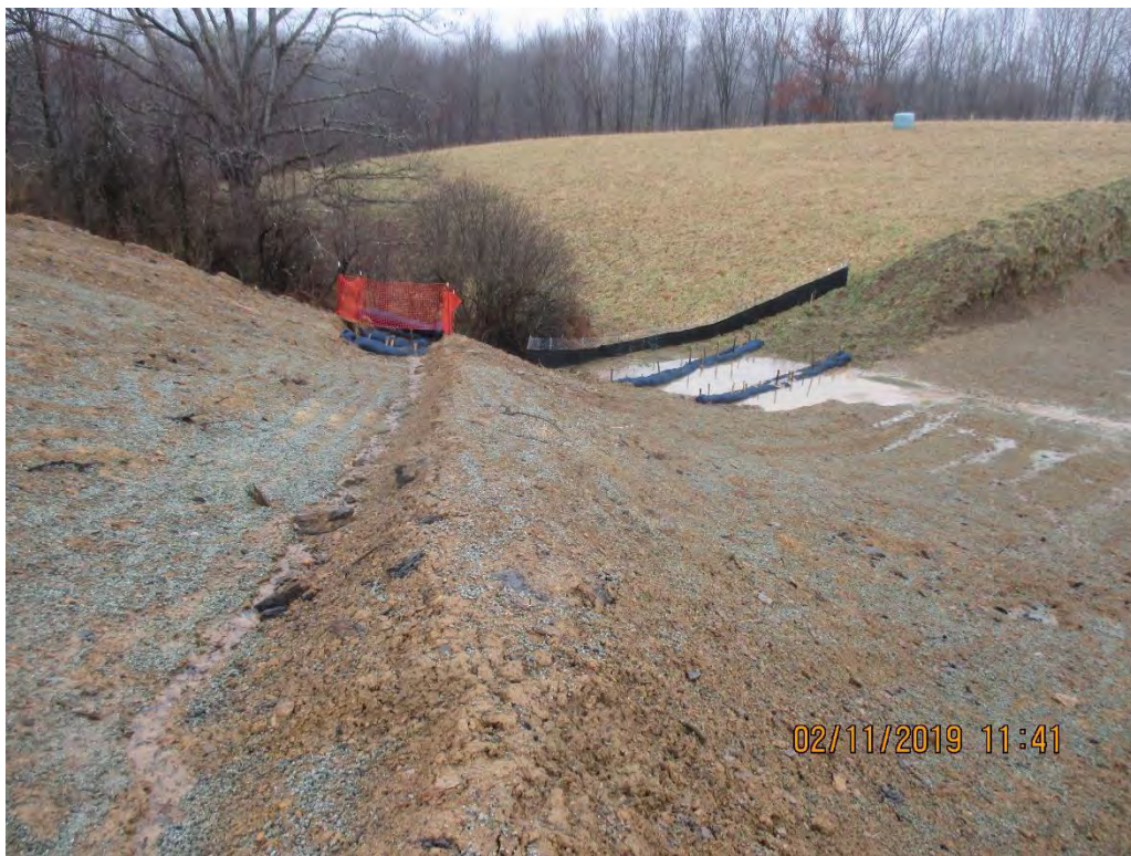
Waterbar terminus at station #5999+50 facing West
