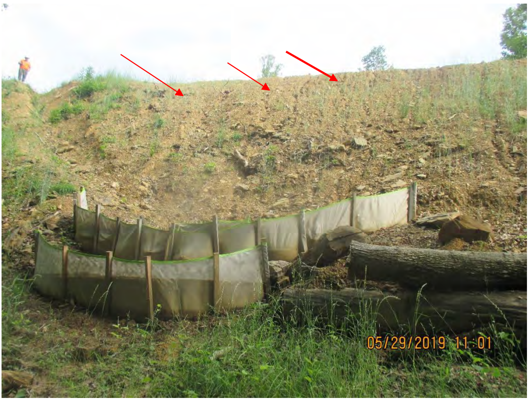
Facing upslope near station #4031+00 at diversion berm outlet No. 2. Waterbar was also terminating onto slope with no controls. Arrow depicts erosion on slope.
