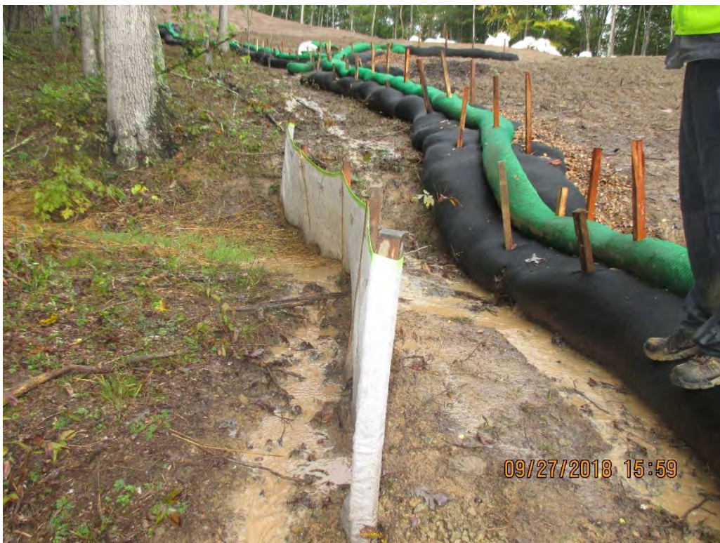
Areas near station number 9417+75 where water bar terminus being overwhelmed with SLW.
