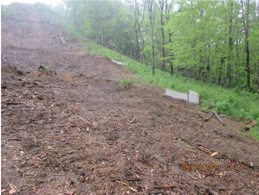
Facing upslope near station #8399+10. Controls were in place at time of inspection at Waterbar outlet per SWPPP.
