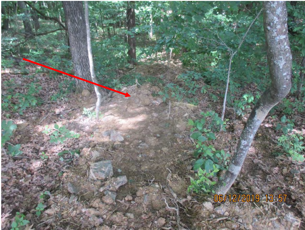
Below controls at station No. 9780+00 facing downslope at sediment deposits and scouring of leaf litter. Arrow depicts deposits.
