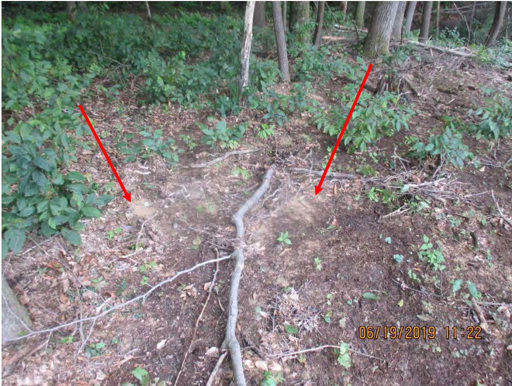
Downslope of Waterbar outlet controls at Station No. 6587+00. Arrow depicts Sediment Deposits.
