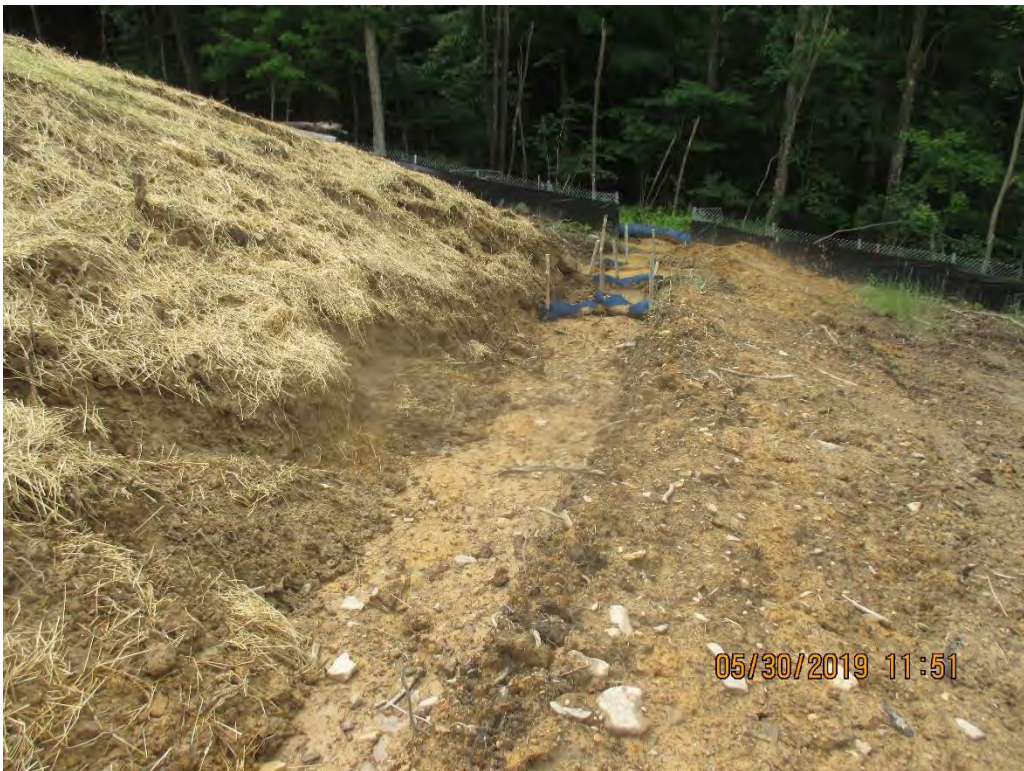
Waterbar with CFS checks installed and scouring topsoil pile below Deepwell road crossing at Station No. 6508+30.
