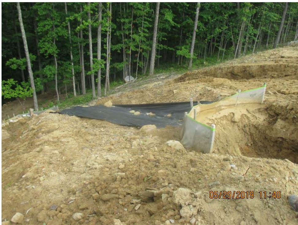
Waterbar outlet downslope of Station No. 4027+00. Waterbar terminating on slope. Fabric installed below control on slope above perimeter outlet.
