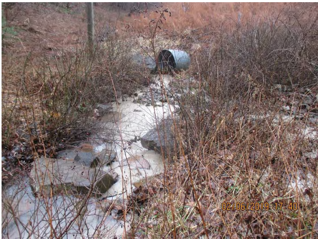
SLW entering UNT of Brammer Br. And traveling downstream towards larger culvert conveying under MVP construction yard entrance.
