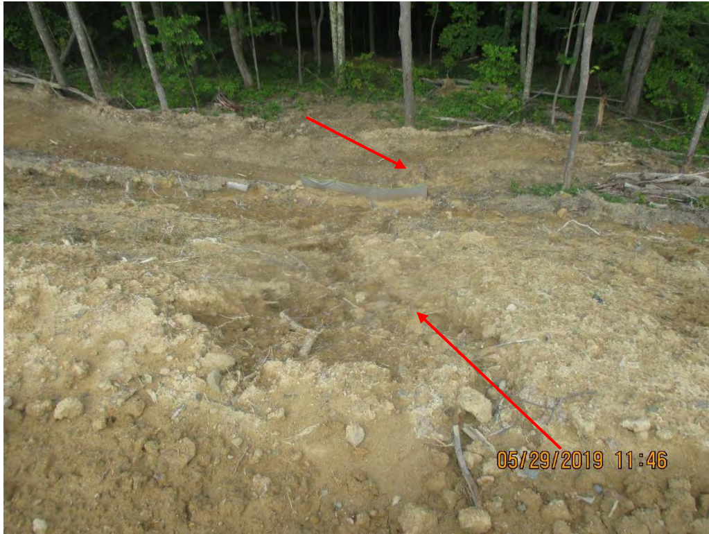
Standing near station 4027+00 facing downslope. Erosion present on fill slope. Perimeter control being overwhelmed with sediment. Evidence that Sediment laden water was observed due to deposits being present past controls. According to representative logging disturbance had taken place.
