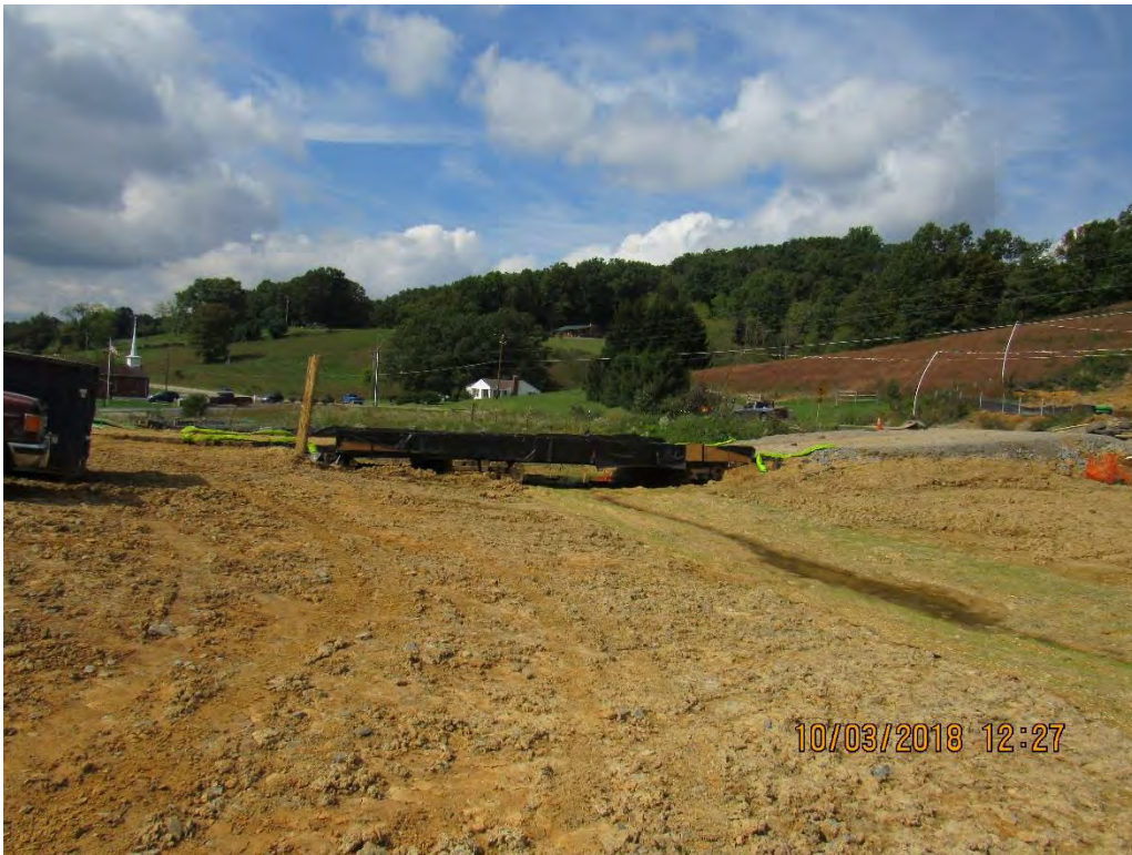
Photo 5: Bridge installed in established area of concern at Lindsie Methodist Church station 10116+49.
