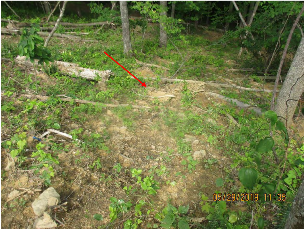
Sediment deposits present past LOD at station No. 4027+00 facing downslope of perimeter outlet.
