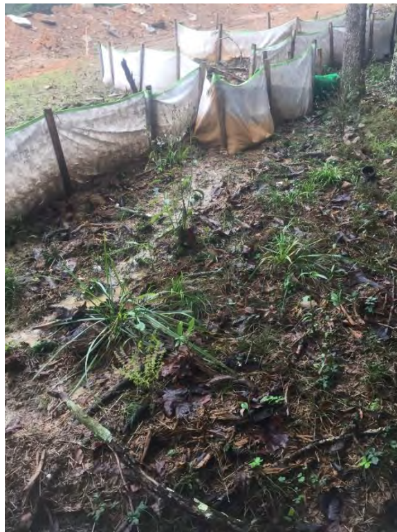
ROW near station numbers 9779+00 and 9778+00 where water bar outlets were being overwhelmed and SLW was passing through and under and being transported past LOD.
