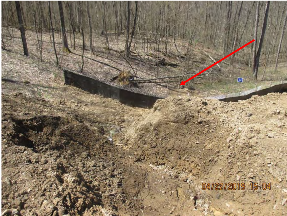
Stream S-T35(A) facing downslope Waterbar terminus at Station #8633+71. Waterbar appeared to be directed towards stream. Controls were buried in sediment where erosion was present. Super Silt was added after clean-up occurred. Arrow depicts Sediment deposits that were present in stream.
