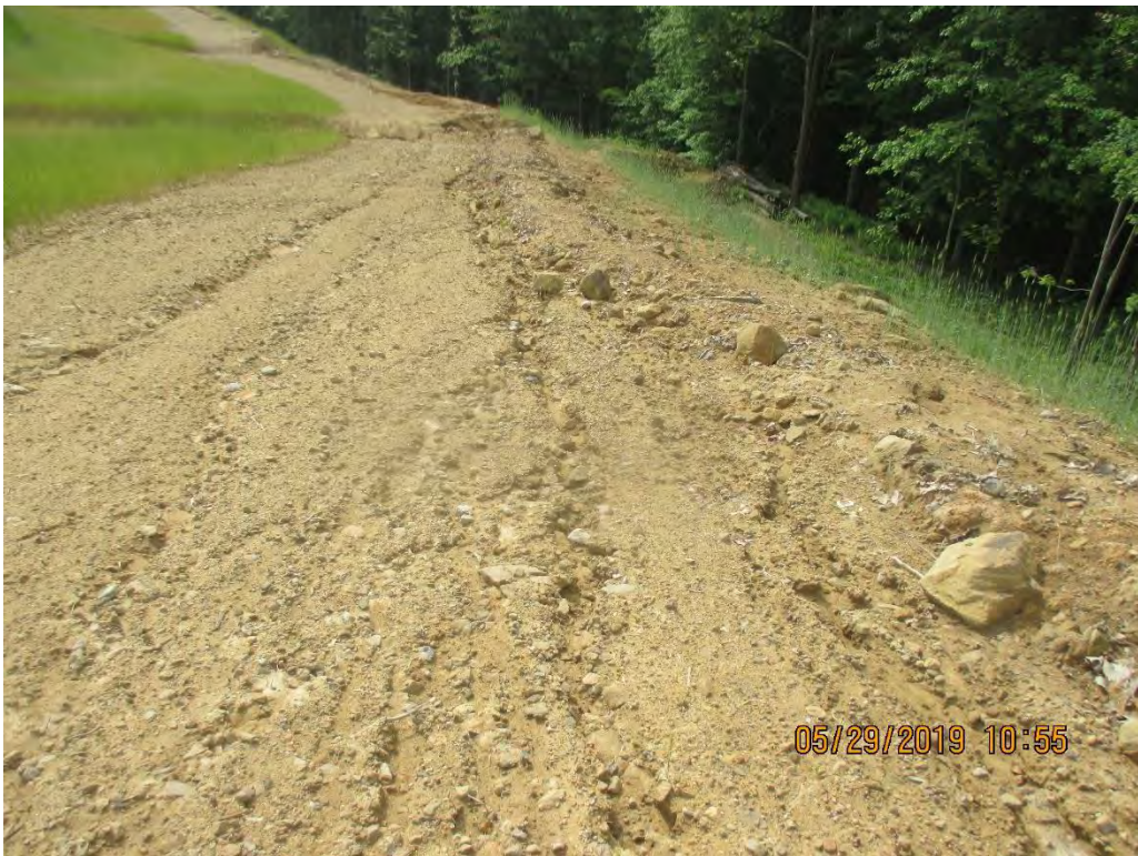
Near station No. 4031+00 facing downslope. Erosion present on ROW where grass hadn't germinated in travel lane.
