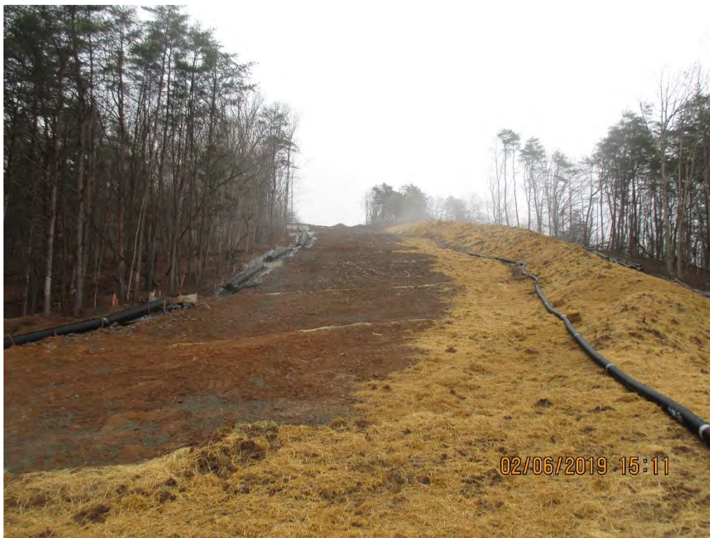
View of MVP ROW facing South at Access Road MVP-MLV-AR-20 near station #8986+00.
