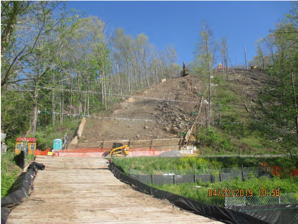
CR 12/3 crossing above greenbrier river at station #9049+93 facing North at MVP ROW
