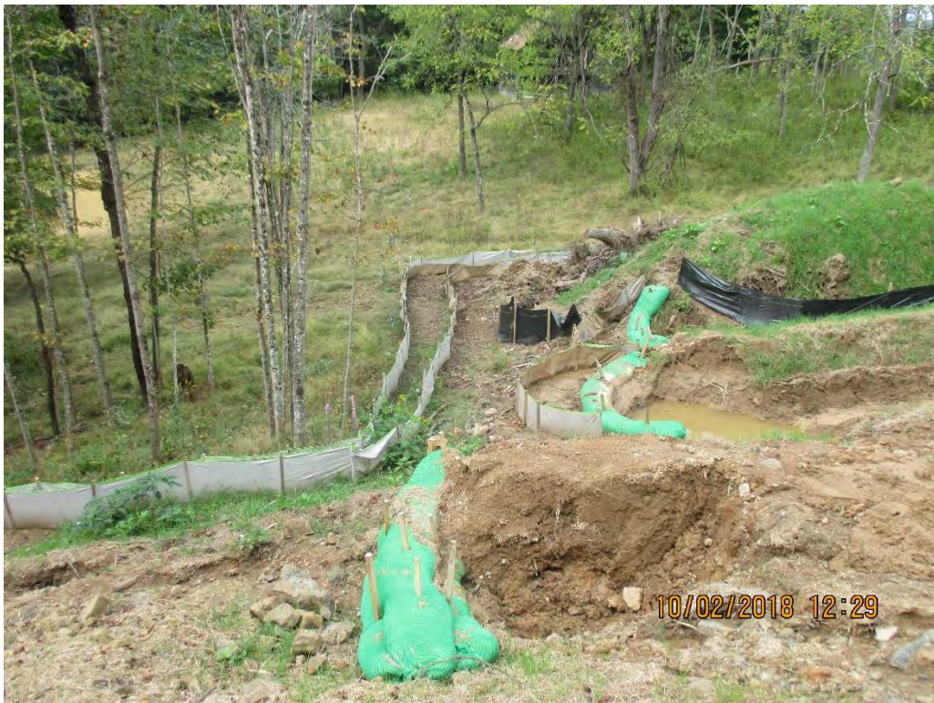
Overview of BMP's north of pond and near station # 9687.
