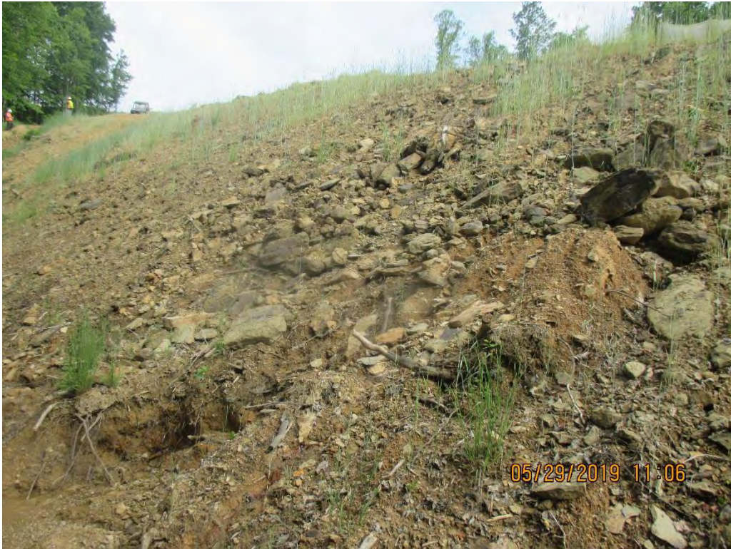
Fill slope with erosion present above diversion berm outlet No. 3.
