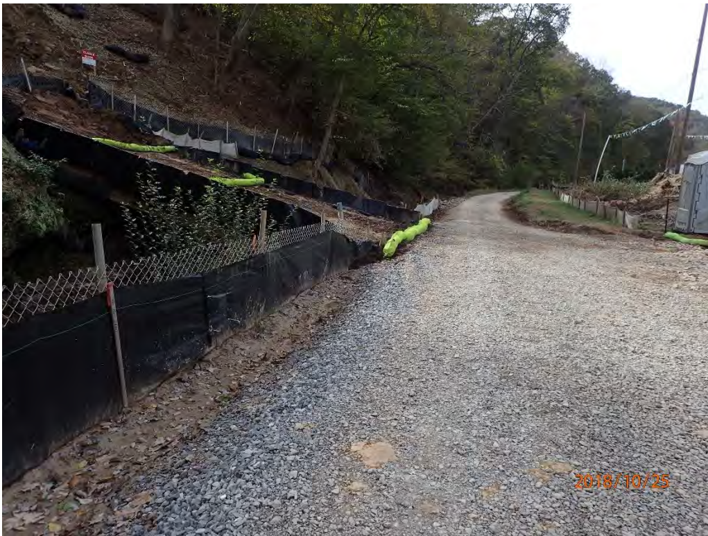
Sams Run Road re-graveled since last inspection.
