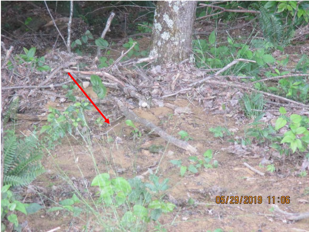
Downslope of diversion berm outlet No. 3. Sediment deposits present.
