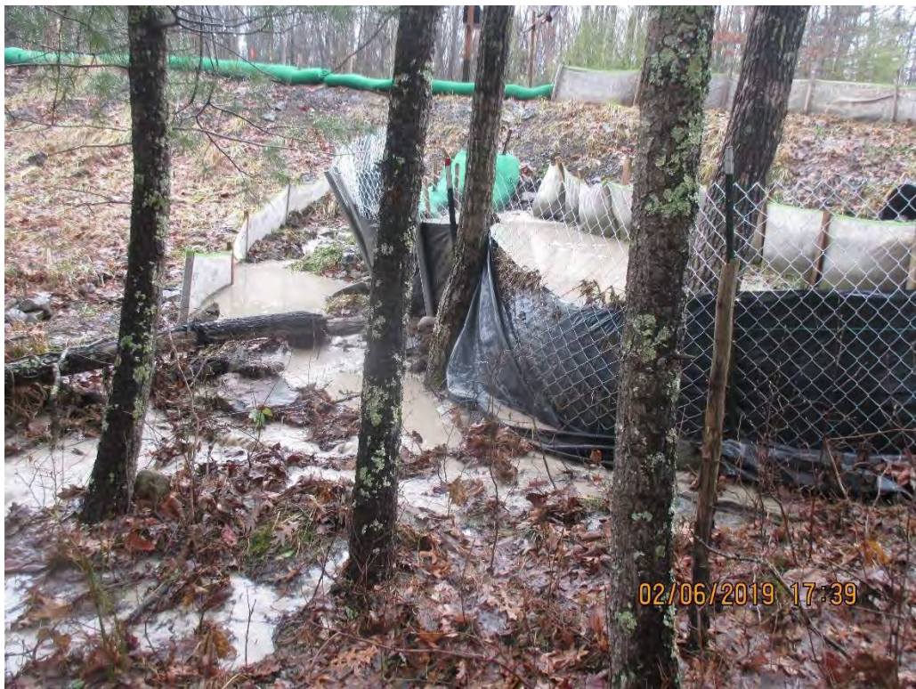
SLW flowing past controls and downslope to UNT of Brammer Branch. Backside of silt fence fallen over.
