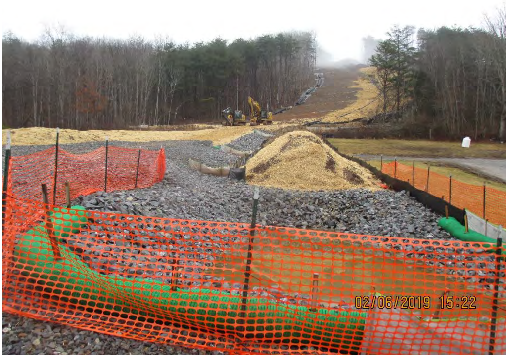
Pipe slope drain in background and rock lined channel terminating into large sump.
