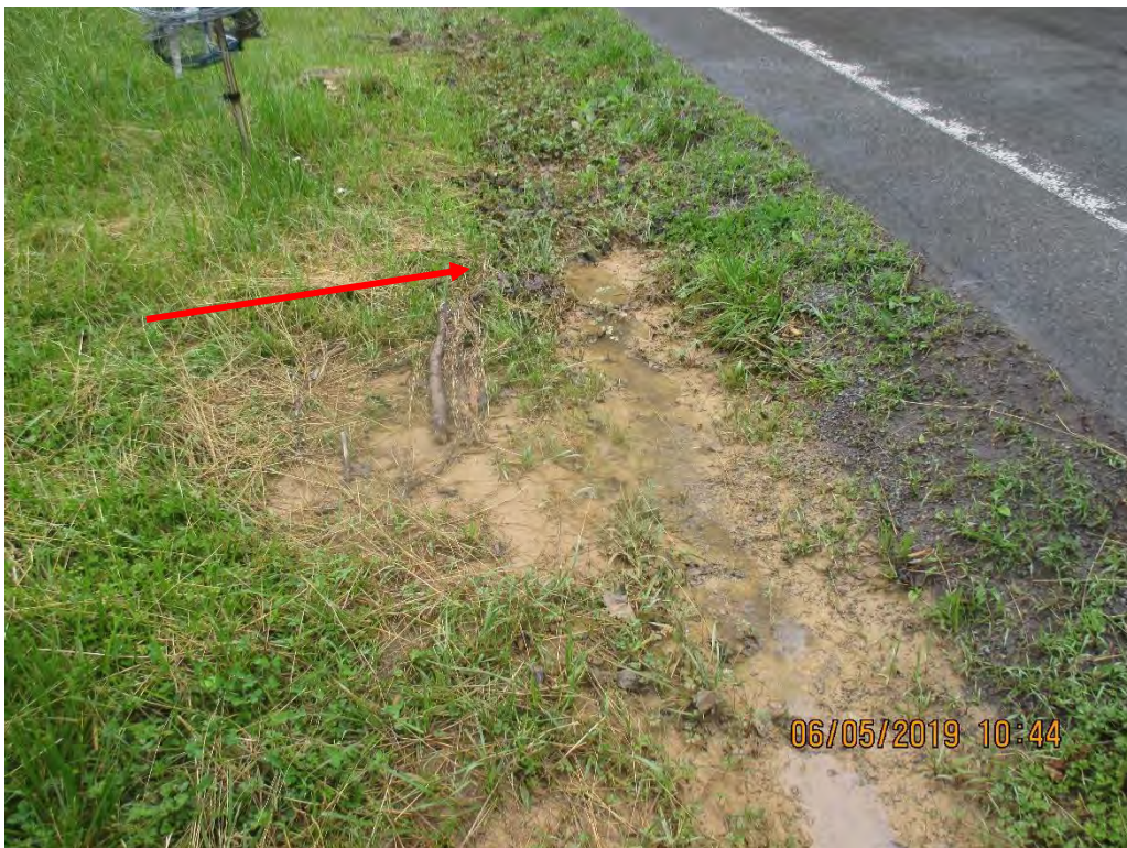
Sediment deposits in roadside ditch that parallels route 82. Arrow depicts culvert intake that conveys under route 82.
