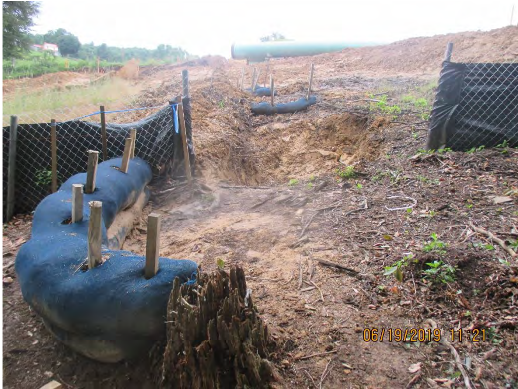
Waterbar Outlet and primary controls at Station No. 6587+00 facing towards Additional Workspace and CR 18.
