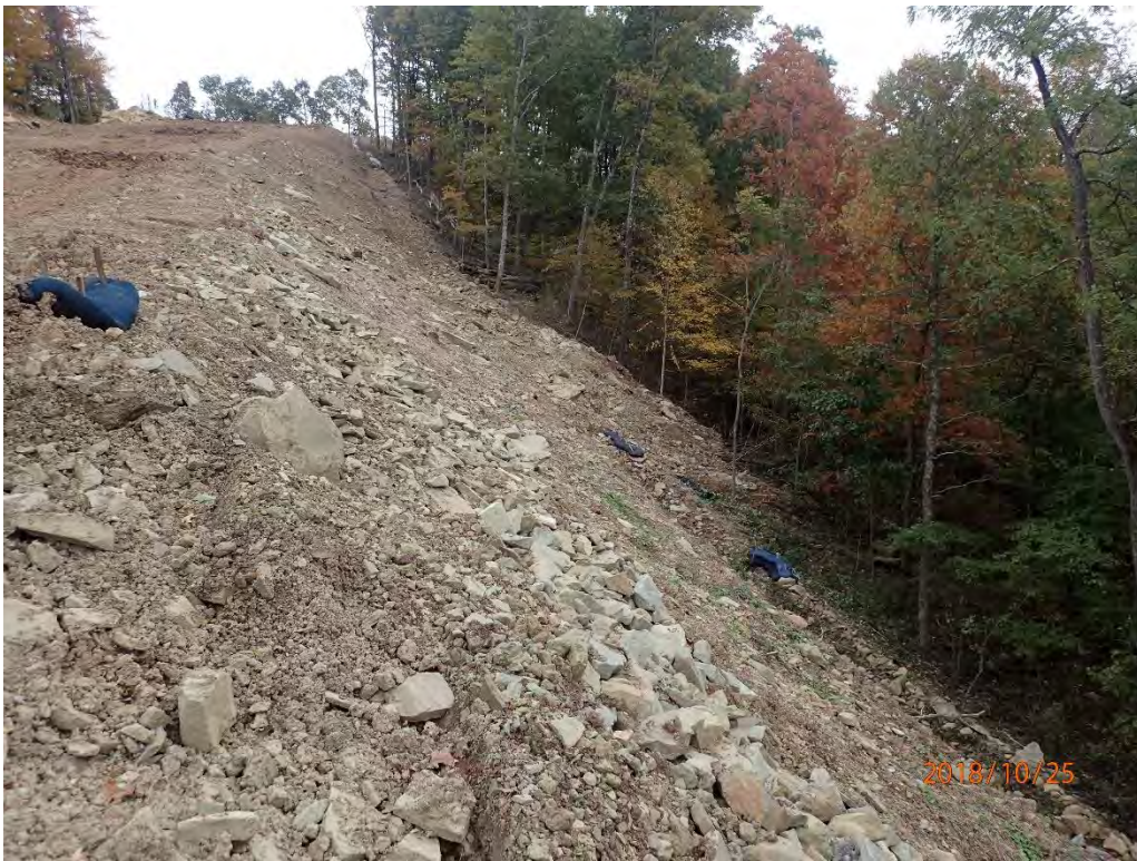
Slip at Station 489 entered the ditchline from a sideslope allowing sediment to leave the project ROW.
