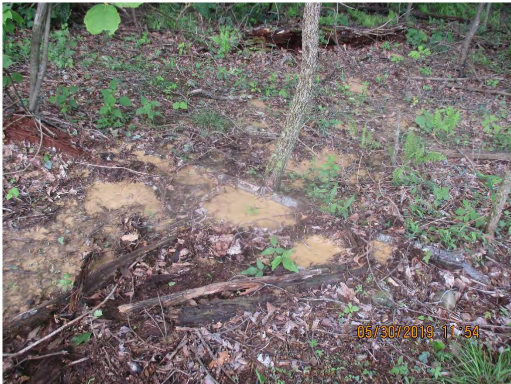
Sediment deposits observed past LOD and Controls below Waterbar and topsoil pile at station No. 6508+30.
