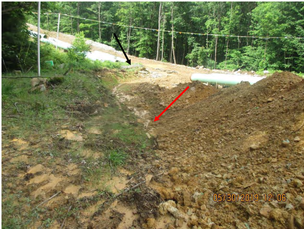
Sediment deposits and SLW traveling downslope at station No. 6510+40. Seep was present in cut next to topsoil pile. Channel wasn't stabilized and conveys to a sump with a slope drain that crosses ROW. Arrow depicts seep. Black arrow shows sump with slope drain inlet.
