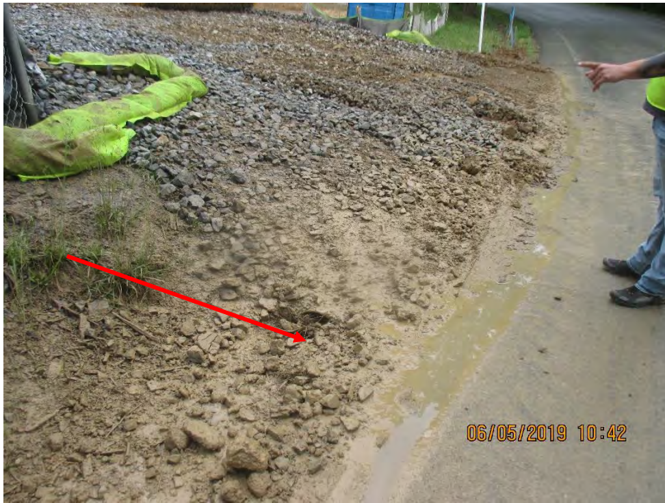
Construction entrance at the Route 82 crossing at station No. 5539+00. Arrow depicts culvert inlet.
