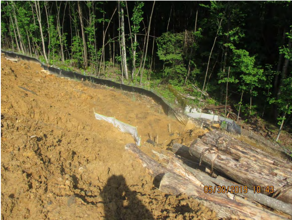
Slope below Waterbar terminus. Perimeter controls becoming overwhelmed with sediment.
