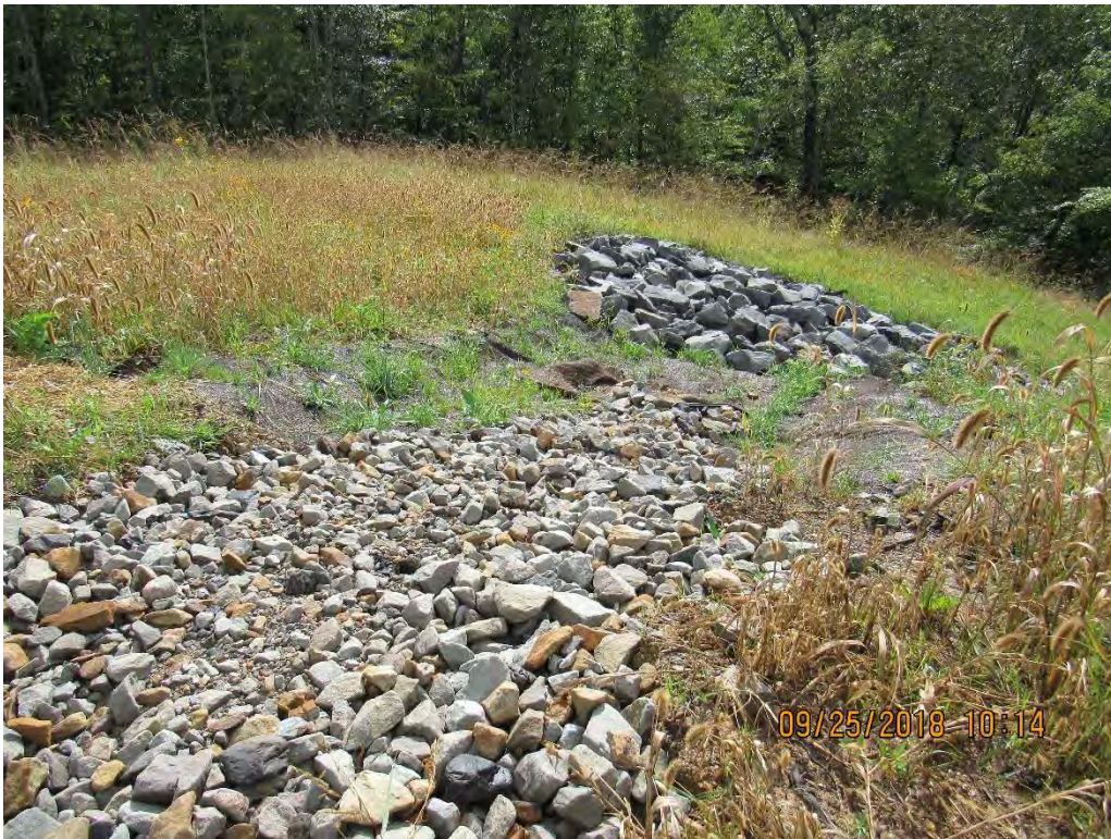
Photo 7: 1 of 2 covered underdrain outlets abating NOV# W18-52-007-CP.
