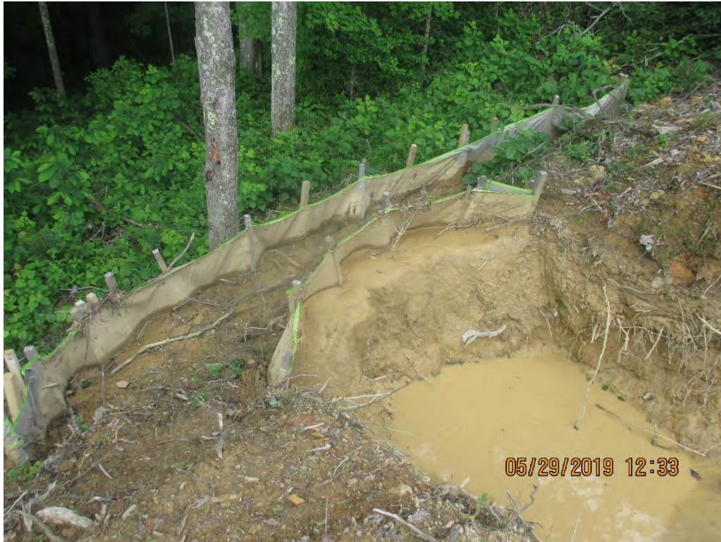
Below Waterbar outlet at station No. 3977+00 looking at perimeter outlet controls.
