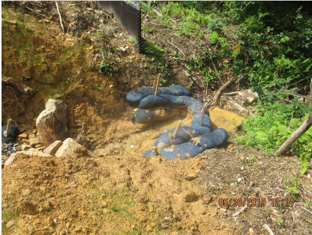
Below seep slope drain outlet. SLW and sediment overwhelming controls.
