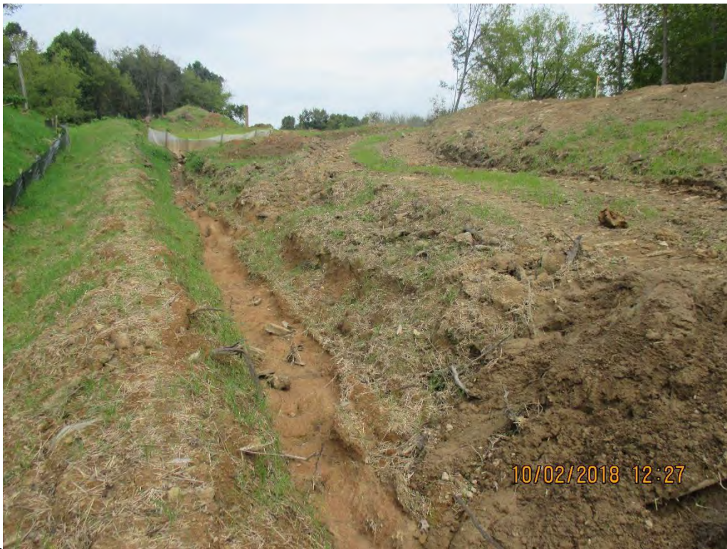
Un-stabilized channel flowing towards above mentioned BMP at station #9687.
