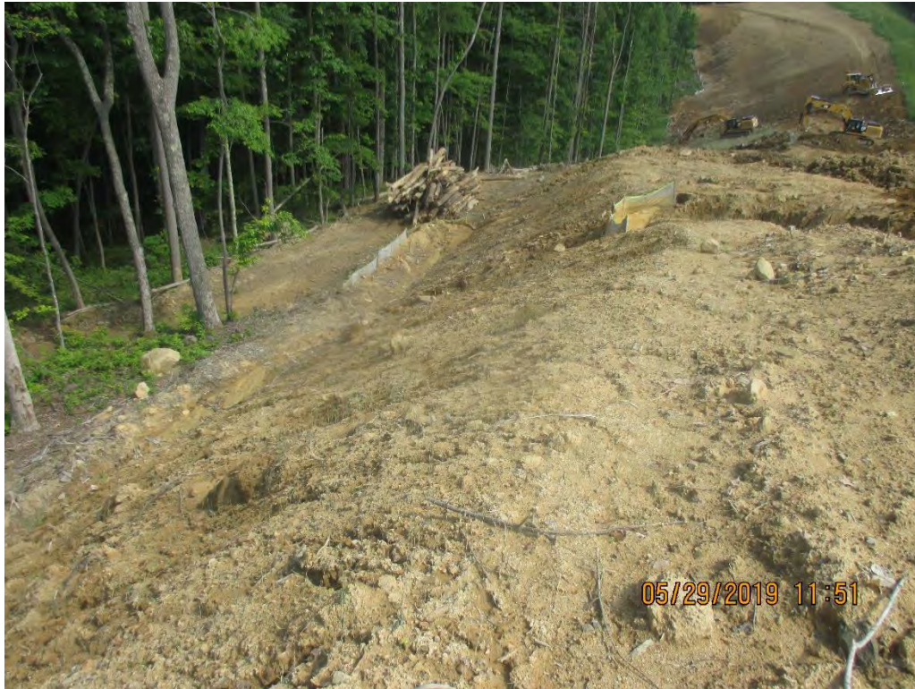
Near station No. 4017+00. Waterbar terminating onto slope.
