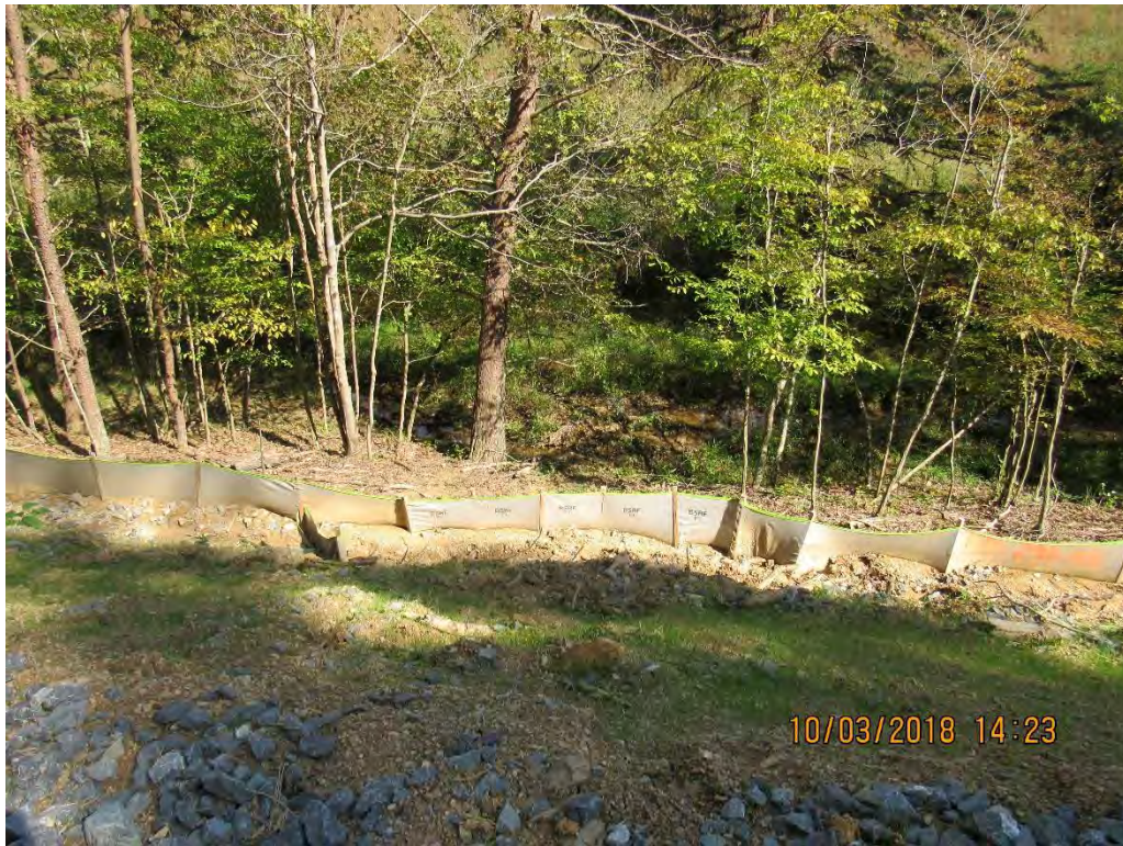
Photo 11: Repairs made to location of failure at Access Road 231.01 abating NOV# W18-52-009.
