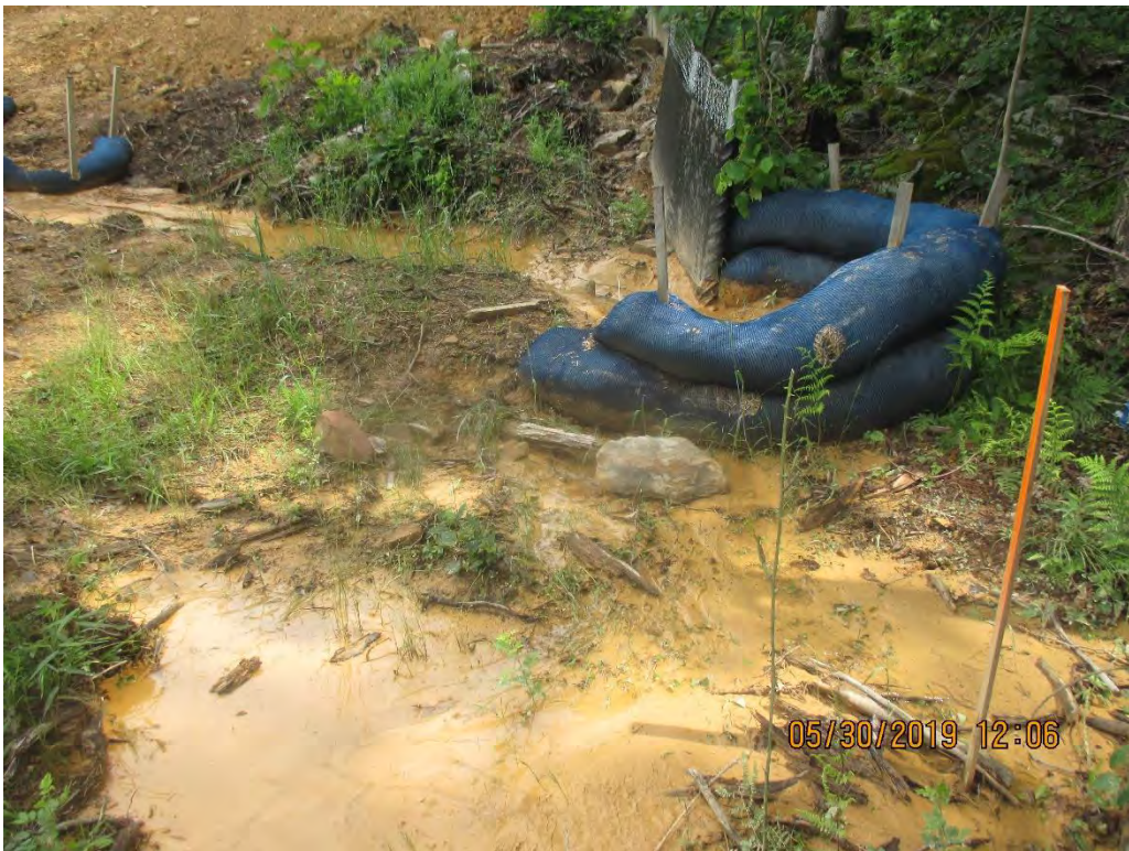
Waterbar outlet at station No. 6510+40 facing upslope. Sediment deposits were observed past LOD and conveying towards Wetland W-N18.
