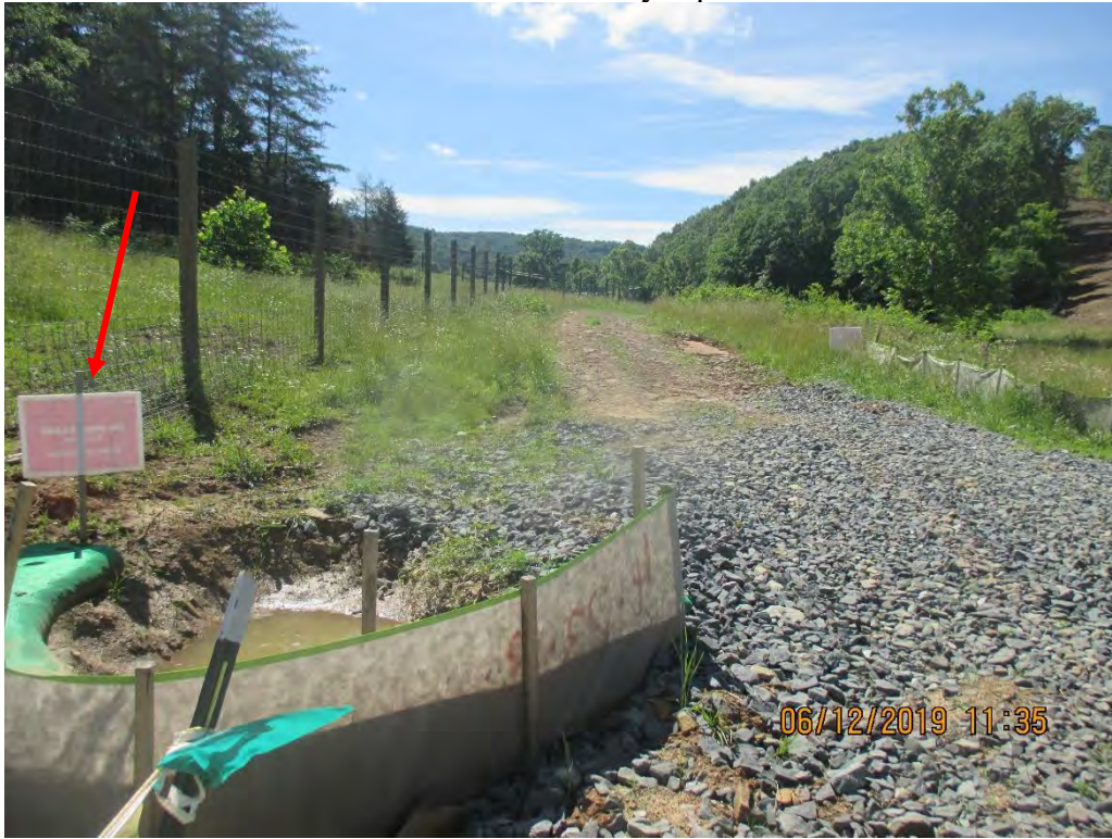
Above Anne's Branch crossing near station 9744+00. Facing upslope of MVP ROW. Erosion ongoing on road as well as slope above road. Arrow depicts LOD.
