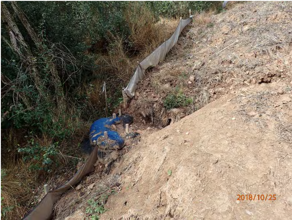
Overwhelmed sump near Sams Run.
