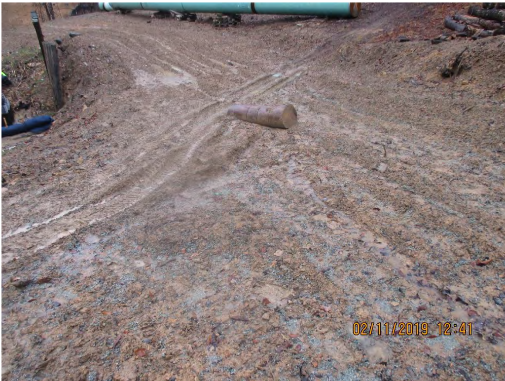
Disturbed slope upslope of Wetland Crossing W-IJ-55
