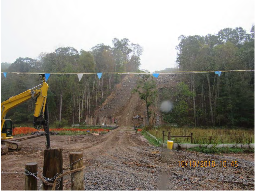
Photo 9: Keller's Creek road station 9127 with rough grade completed awaiting final grade and restoration.
