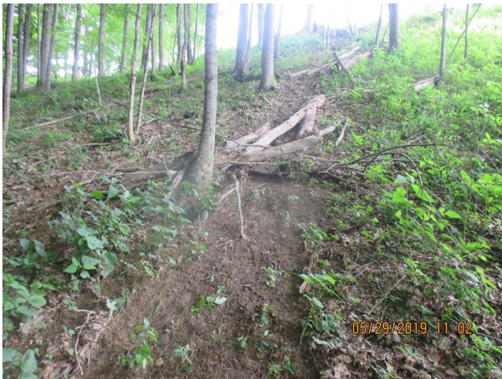
Standing further downslope below diversion berm outlet No. 2 near 4031+00. Scouring of vegetation present below control.
