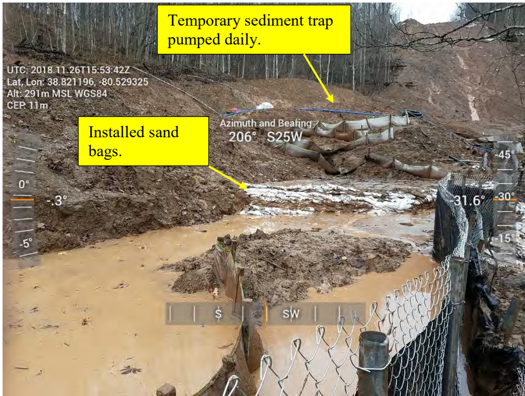
Photo 4: Temporary repairs installed prior to permanent repairs at reported slip. Photo supplied by EI Andy Pauley.
