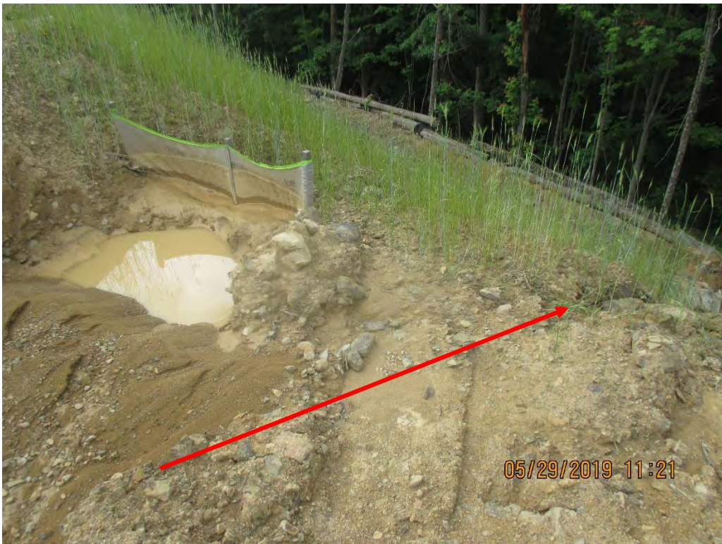
Waterbar outlet above diversion berm outlet No. 3. Sump full of sediment and evidence that concentrated flow on slope was observed due to controls not functioning as designed. Arrow depicts flow.
