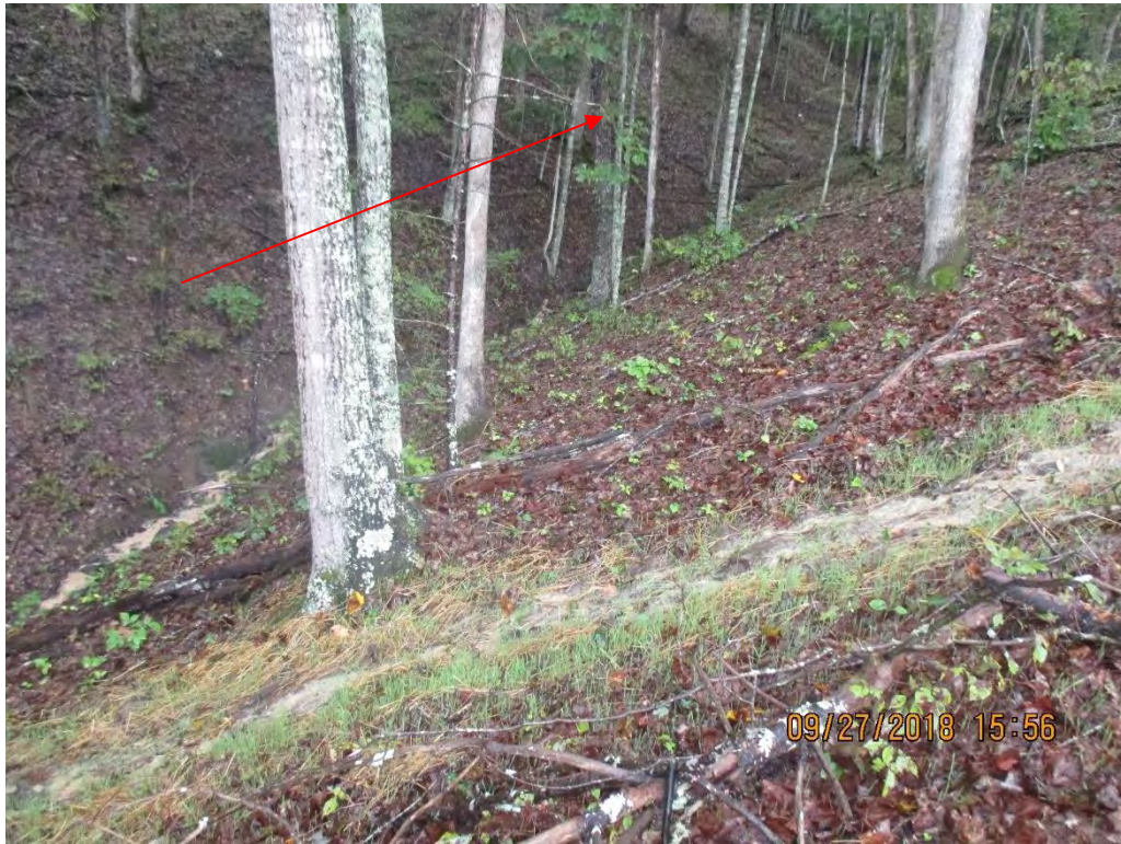
SLW being transported off ROW and past LOD into ephemeral streams near Station #9417+75. Red arrow depicts where ephemeral splits and goes upslope towards spring.
