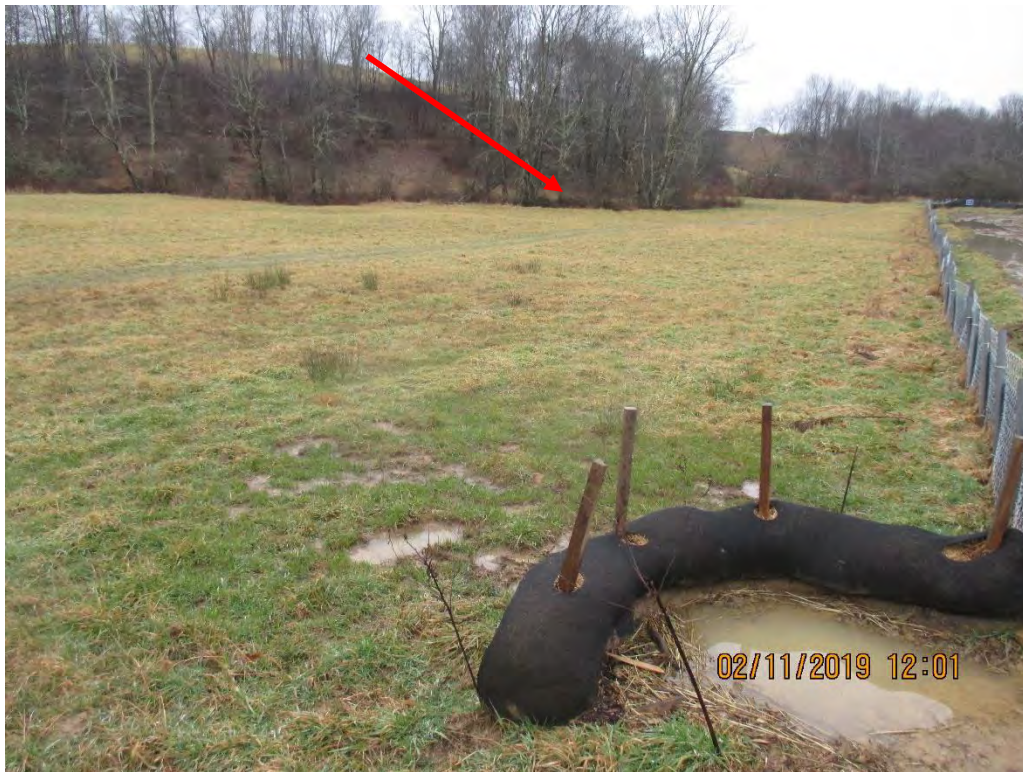
Waterbar terminus near station 5985+50, Sediment deposits and SLW present. Arrow depicts Stream S-B28
