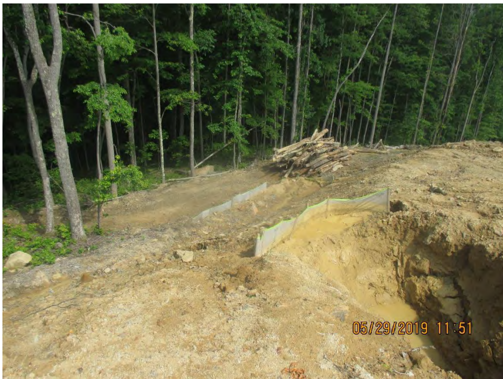
Below Waterbar outlet near station No. 4017+00. Evidence that sediment laden water flowed past LOD was observed.
