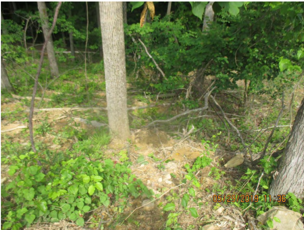
Sediment deposits present past LOD at station No. 4027+00 facing downslope of perimeter outlet.
