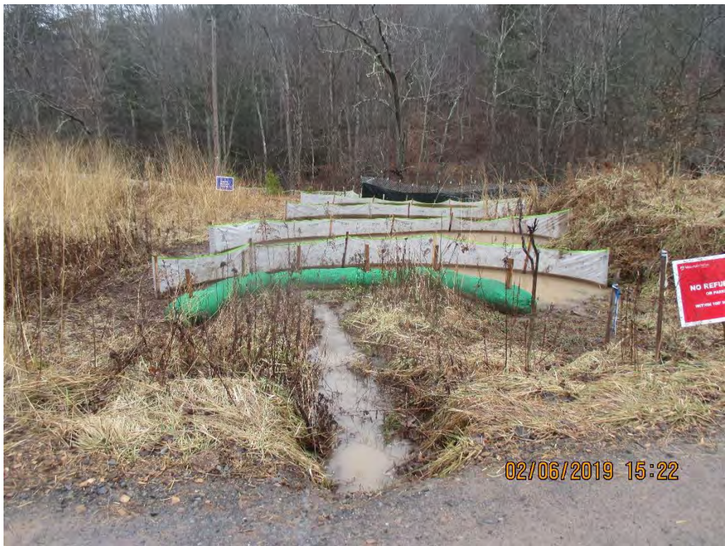
Culvert output on opposite side of access road conveying run-off through multiple controls near station #8986+00
