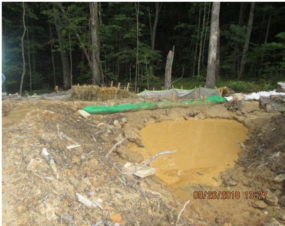
Waterbar terminus near being overwhelmed near Station #9899+00.
