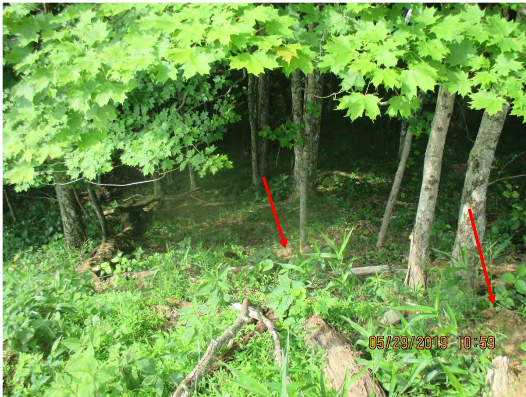
Downslope of Diversion berm outlet No. 1. Sediment deposits observed past LOD. Vegetation was also stained from SLW leaving site.
