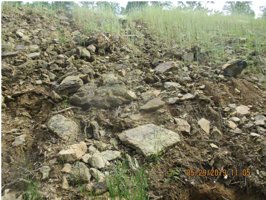
Fill slope with erosion present above diversion berm outlet No.3 near station No. 4031+00.
