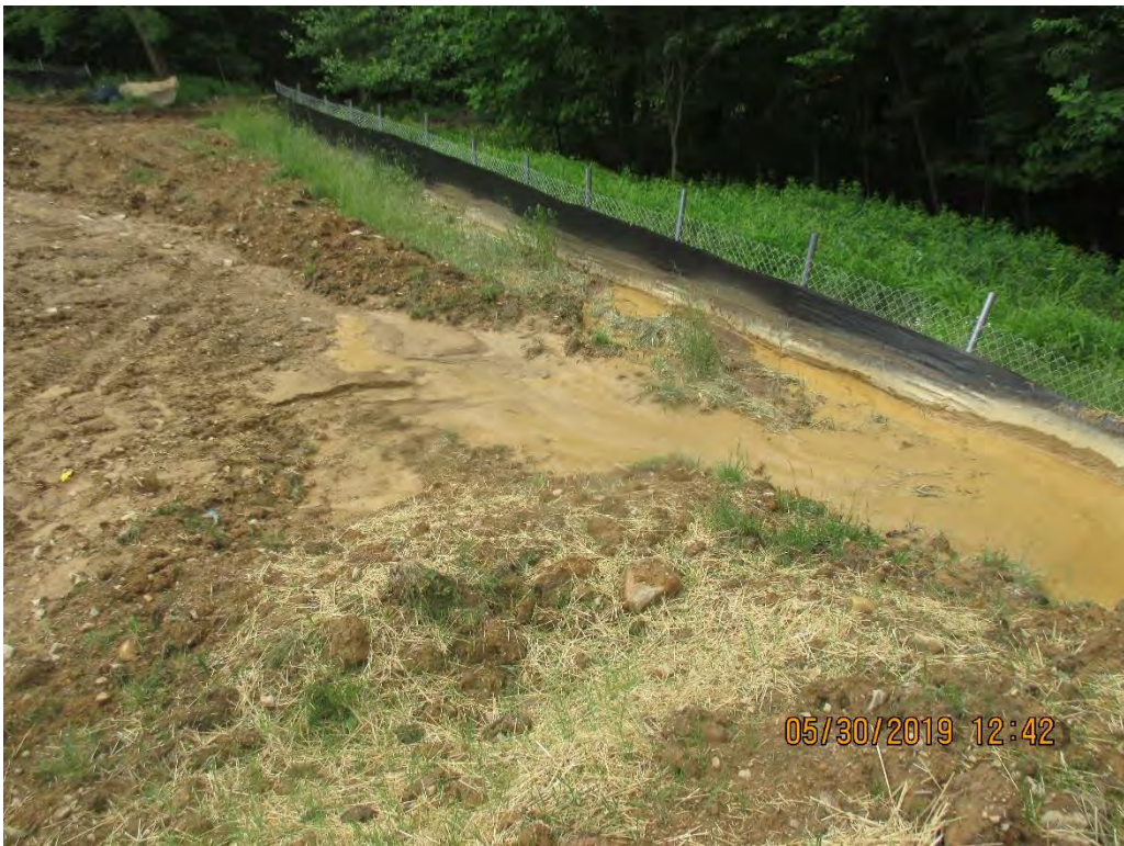
Erosion and sediment/SLW overwhelming perimeter controls at ATWS-22-7A at station No. 6514+60. Sediment deposits observed past controls and LOD.
