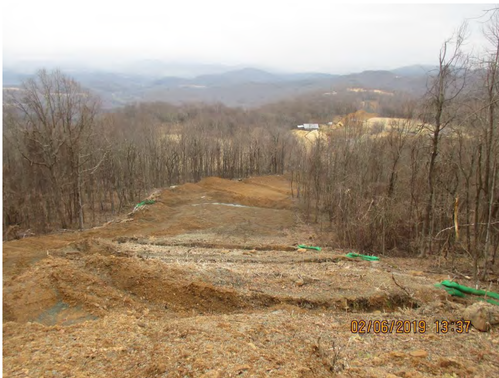
Standing at station 8809+20. Per SWPPP waterbar to be installed and not present.
