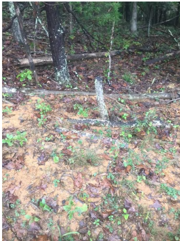
Off-site sediment deposits near station number 9779+00.
