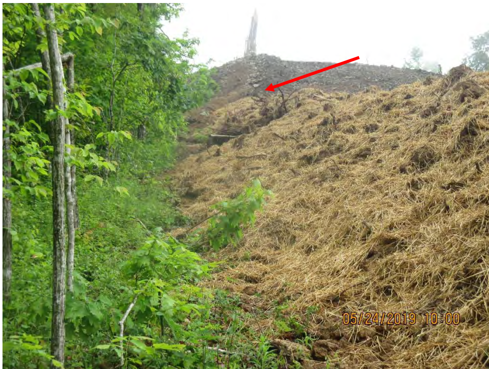
Facing upslope near station No. 8387+96. No perimeter controls in place approximately 150 feet upslope. Berm installed as perimeter controls half way upslope (see red arrow).
