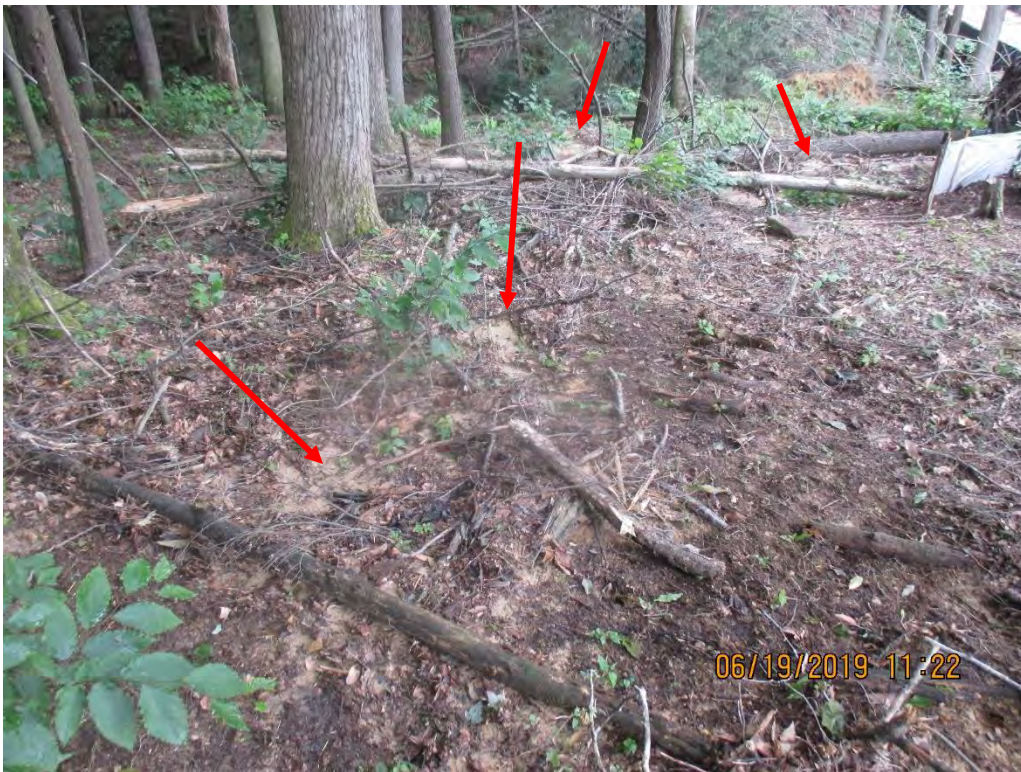
Downslope of Waterbar outlet controls at Station No. 6587+00. Arrow depicts Sediment Deposits.
