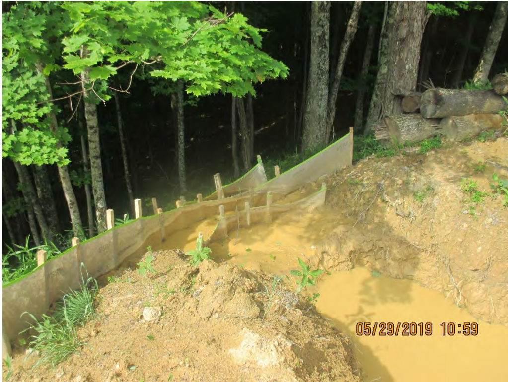
Diversion berm outlet No. 1 at station No. 4031+00. Controls in need of maintenance.
