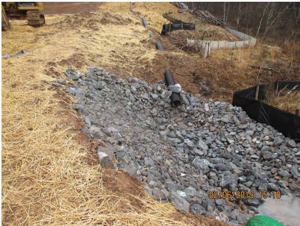
North side of ROW pipe slope drain outlet into rock lined channel on west side of slope.
