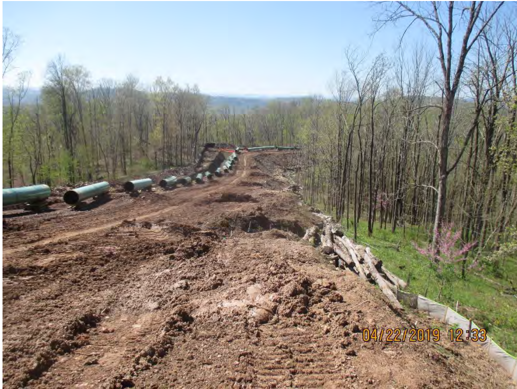
Near station #9015 facing South. Berm installed as perimeter control on downslope section of LOD
