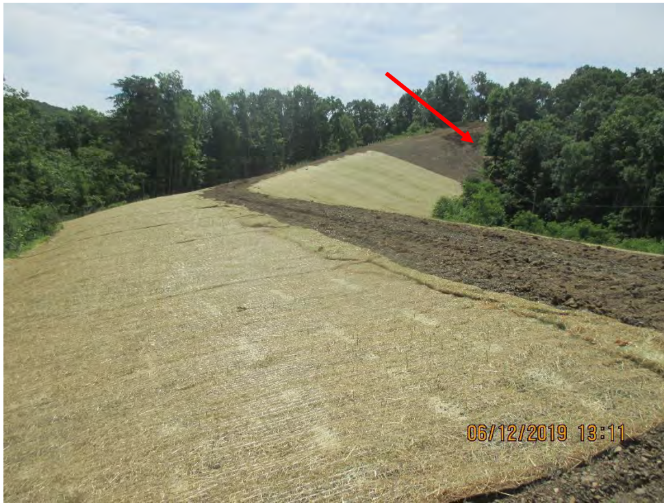
Upslope of Dargo silt fence. Facing South towards AR-221. Arrow depicts where dozer work was ongoing during inspection and controls needed maintenance.
