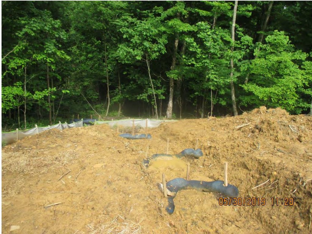
Seep running onto ROW via Waterbar above Stream S-N13. Diversion not stabilized near station No. 6940+00.
