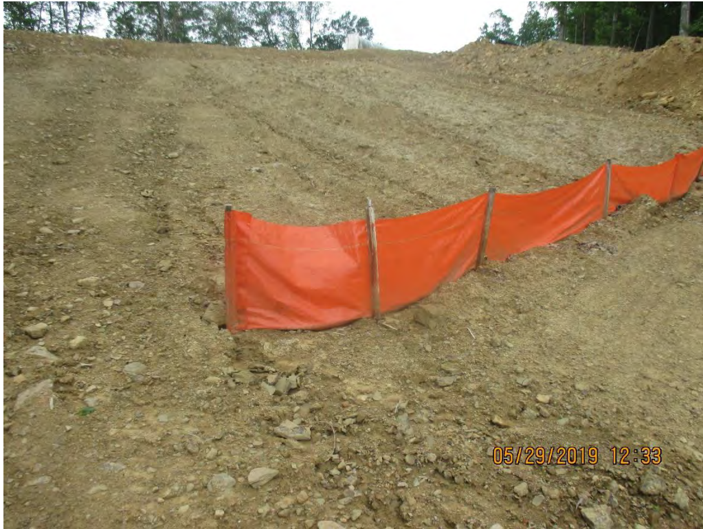
Sit fence installed above Waterbar at station No. 3977+00 facing upslope. Erosion present on slope.
