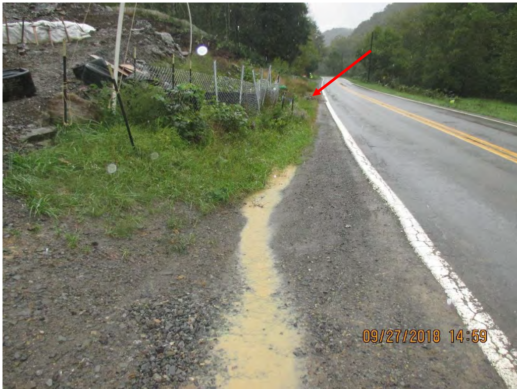
Sediment Laden water leaving ROW intercepted by ditch flowing towards Stream (S-A60). Arrow depicts where ditch connects to stream S-A60 and flows under road via culvert.
