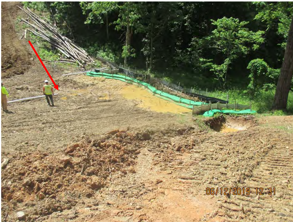
Dargo silt fence. Pipe slope drain terminating on ROW and not extended to edge of LOD. Arrow depicts slope drain outlet.
