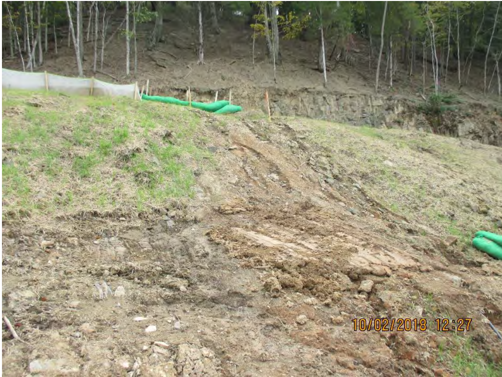
Lack of fill slope protection on opposite side of pond facing upslope near Station #9687.
