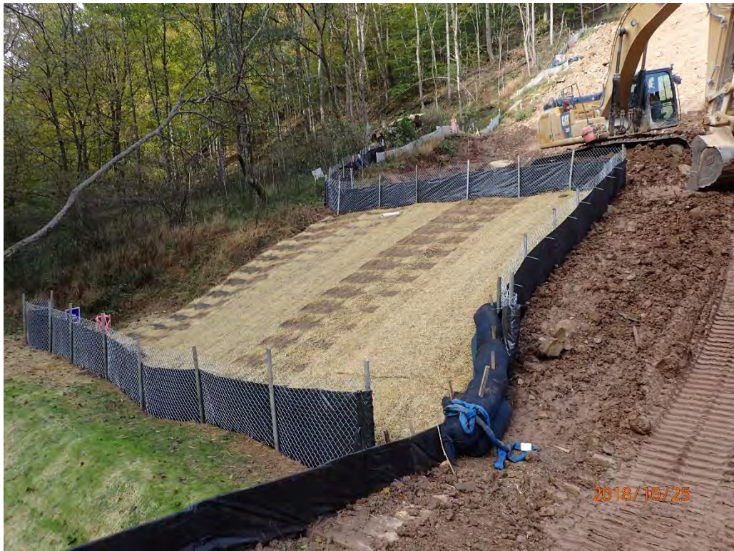
UNT to Mobley Run Slope had been restored since previous inspection where sediment had left the site and entered nearby stream.
