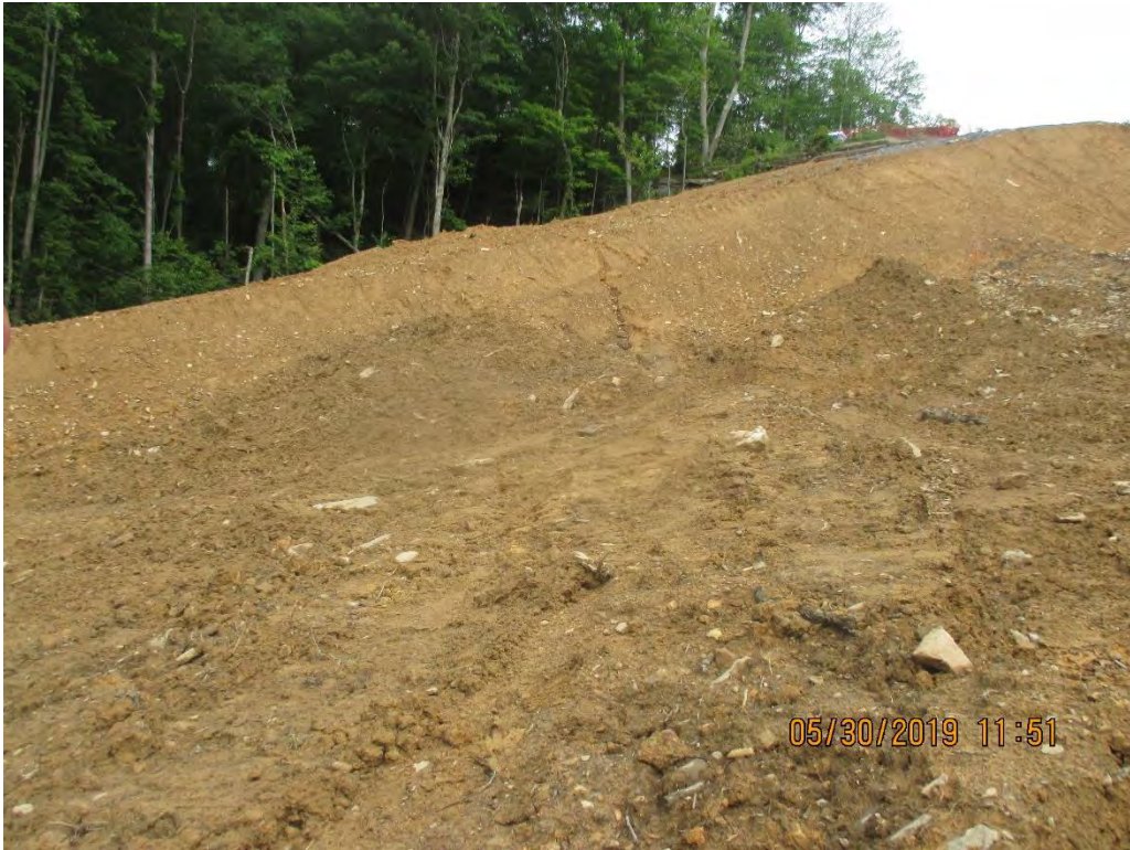
Facing upslope at Deepwell road construction entrance near station No. 6504+20. Erosion present on fill slope and ROW leading to Waterbar.
