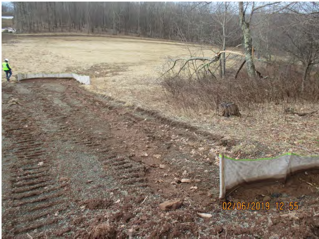
Waterbar termini at station #8780+00 facing South. Rill erosion occurring between controls.
