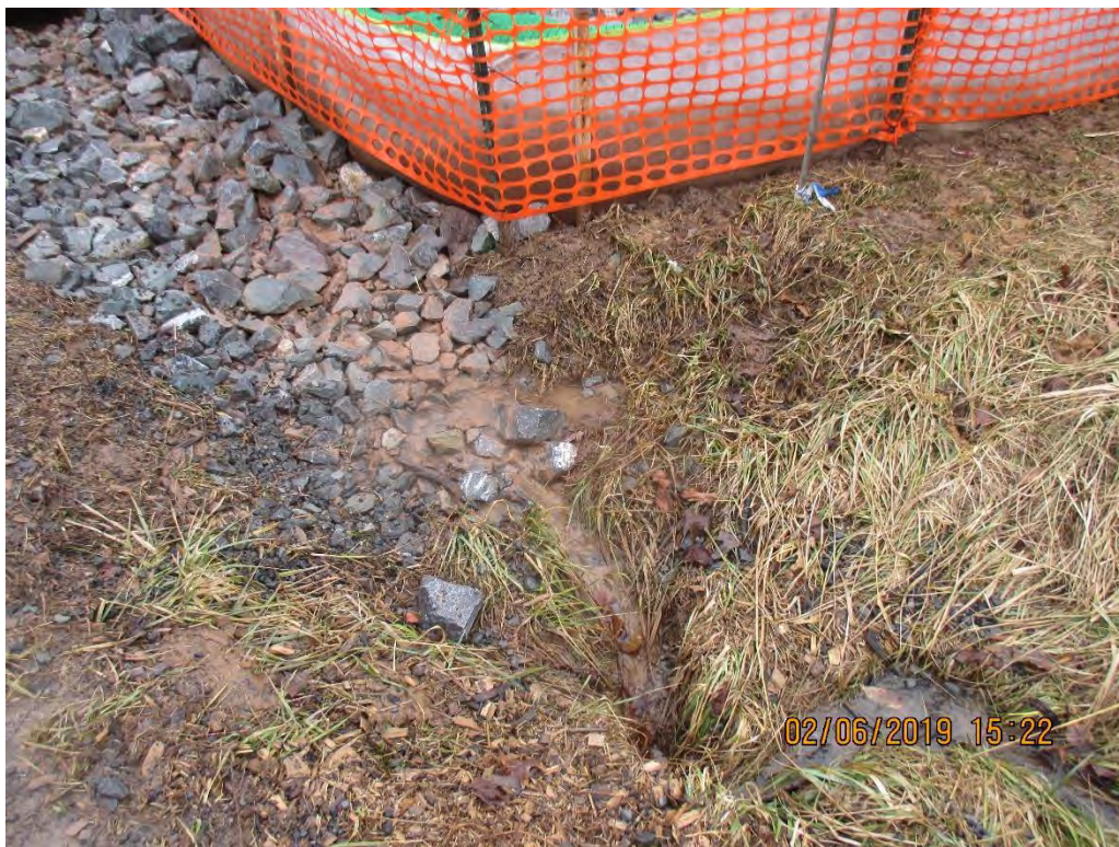
Culvert downslope of large sump transporting runoff under access road MVP-MLV-AR-20 near station #8986+00
