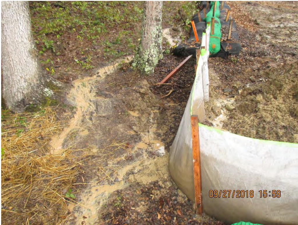
Areas near station number 9417+75 where water bar terminus being overwhelmed with SLW.
