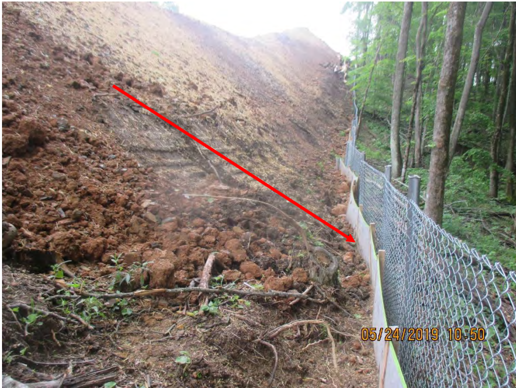
Near station No. 8419+00 facing South. Perimeter controls in place per SWPPP. Arrow depicts where material has slipped into P1 silt fence.
