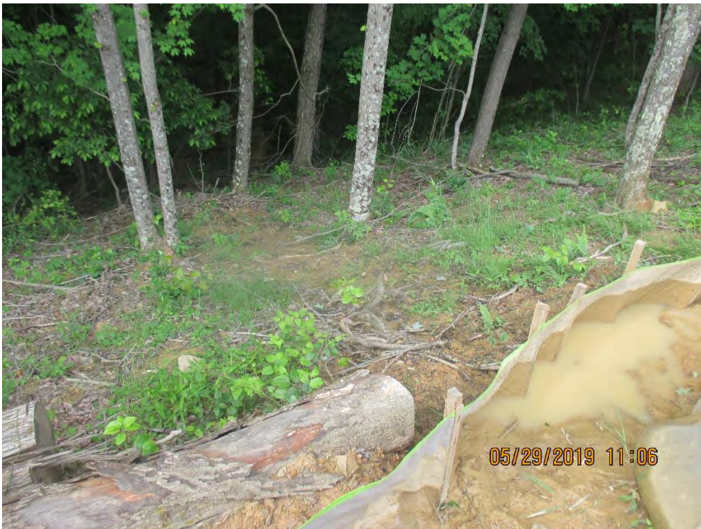
Downslope of diversion berm outlet No. 3 controls. Scouring of vegetation present with sediment deposits present past LOD.
