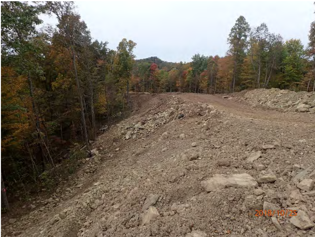
Slip at station 493 had entered the ditchline from a sideslope allowing sediment to leave the project ROW.
