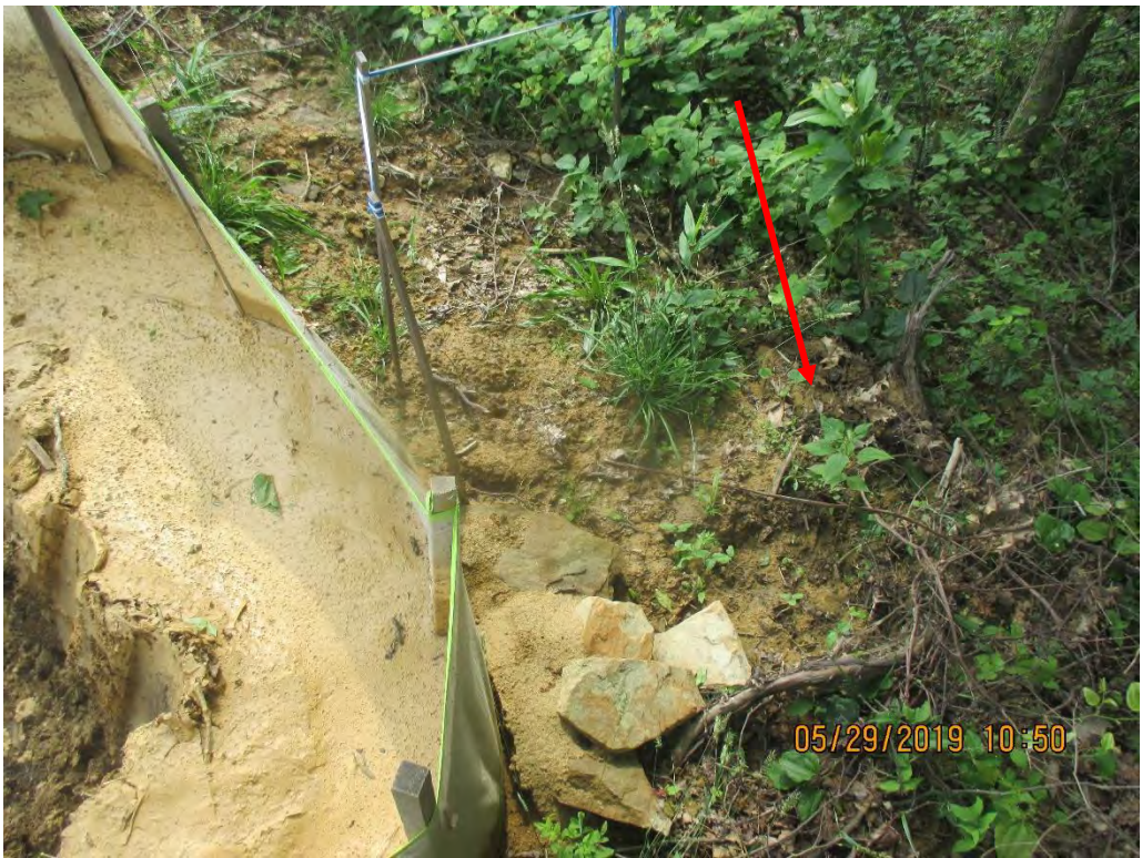
Waterbar outlet above fill slope at station no. 4031+00 facing downslope. Sediment deposits observed past LOD.
