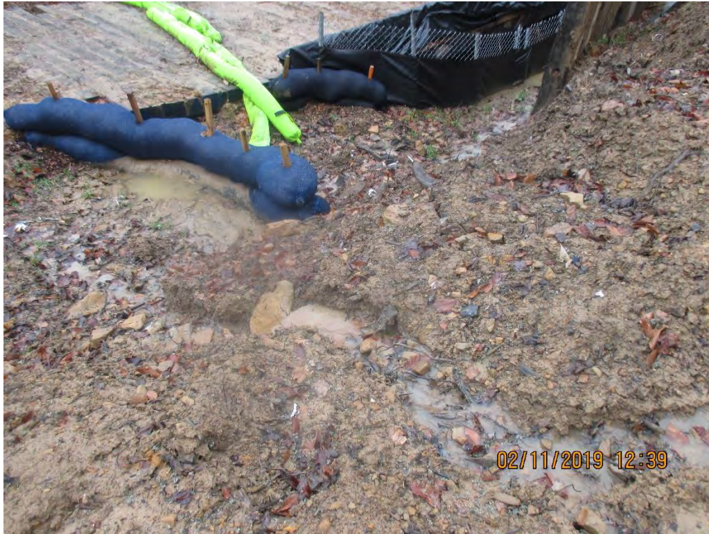
Erosion occurring due to runoff from ROW and being diverted to Wetland W-IJ-55
