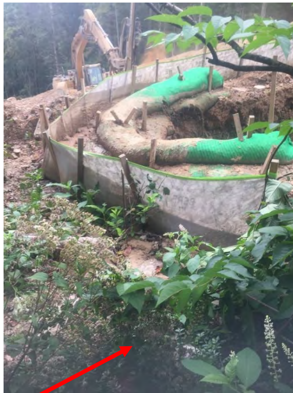
BMP near Station #9911+00 being overwhelmed and sediment flowing under and through control. Arrow depicts where SLW was leaving BMP.
