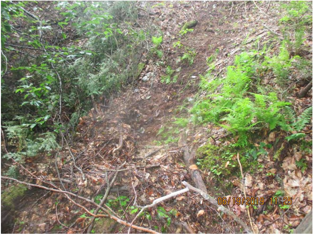
Scouring of stream bank below where sediment deposits were observed above Stream S-L38.
