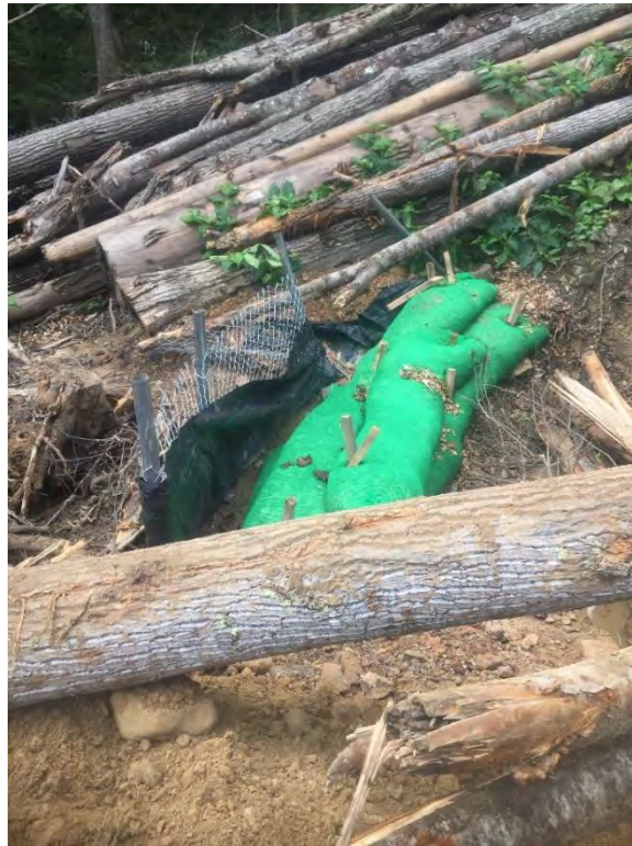
Area near station number 9907+00. Super silt fence had been undermined and damaged by logs
