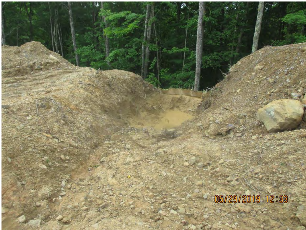
Waterbar outlet at station No. 3977+00.
