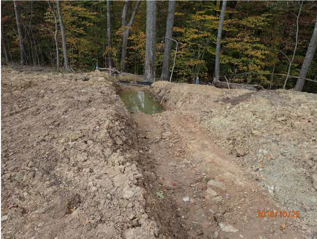
Sump at Station 290 in need of maintenance.
