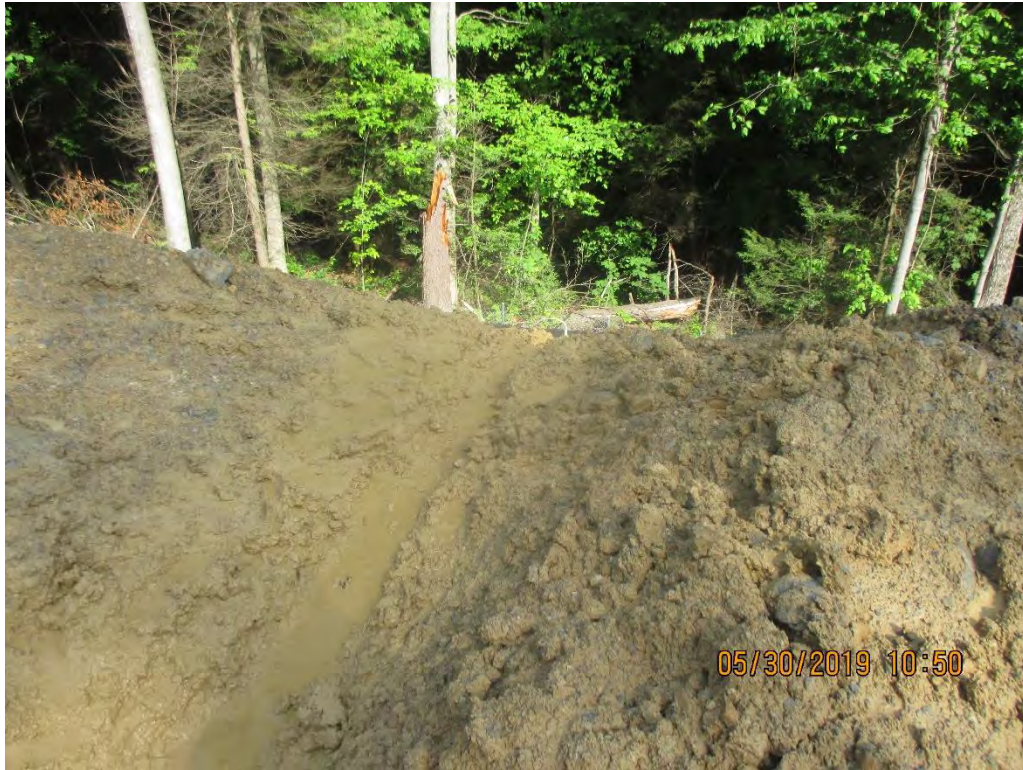
Waterbar outlet terminating onto slope at station No. 6485+10.
