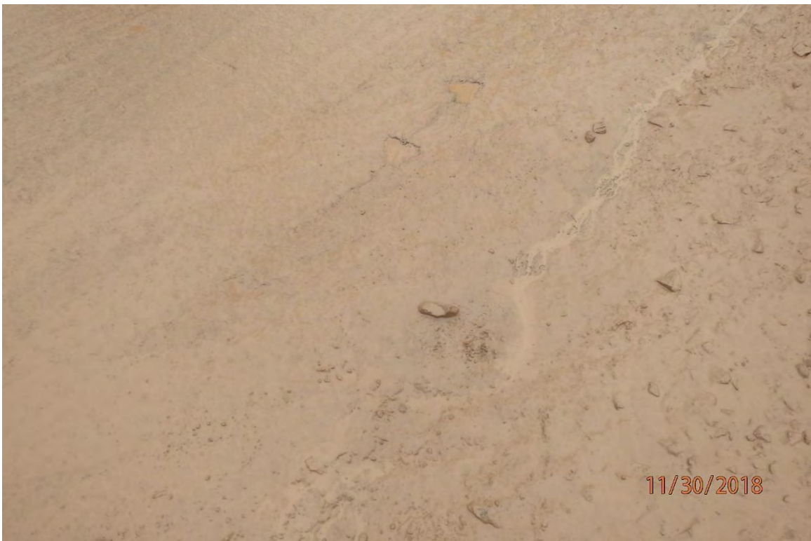
Access Road WV-HA – 31.1 off CR 50/4 showing the lack of an adequately stable construction entrance and the associated track out onto the public road.
