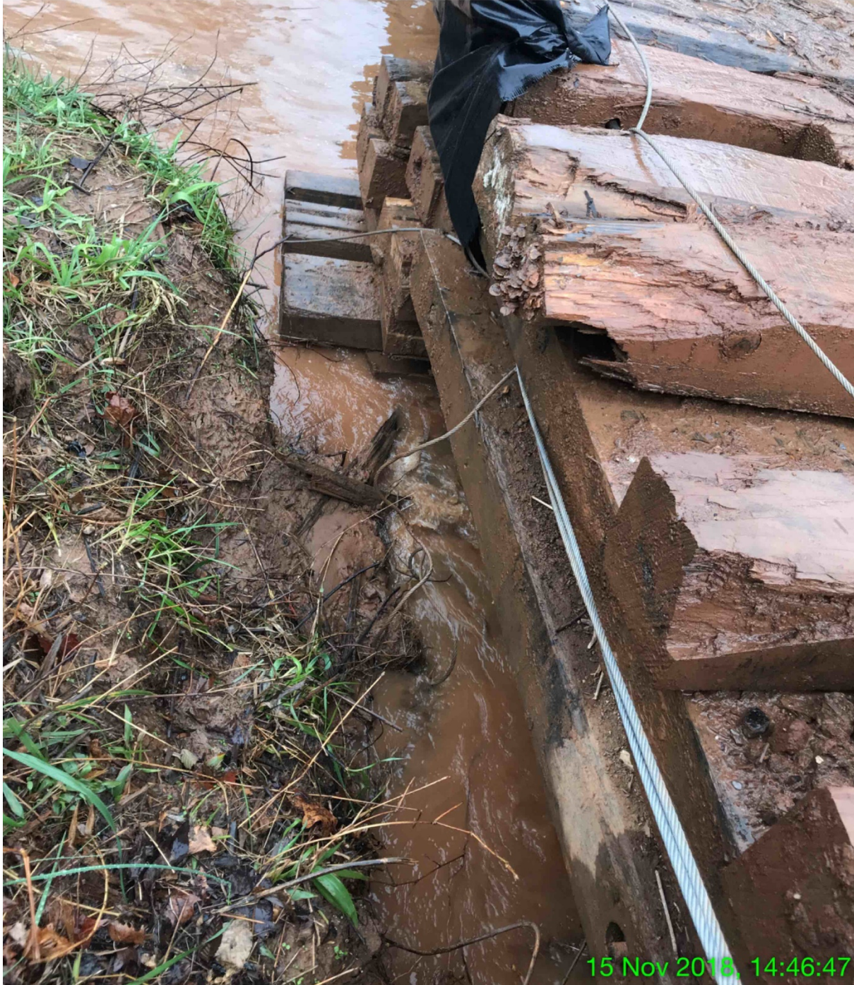
EXHIBIT J – The downstream side of the bridge over Little Creek. Muddy water flowing from the upstream side of the bridge, and under the bridge and into Little Creek with the creek almost full.
