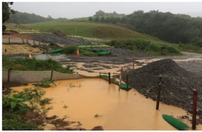
Ineffective silt fence and mulch socks allowing sediment to move into SGT.
