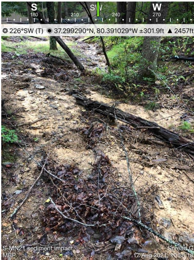
Figure 7 - Sediment deposited in UT to Mill Creek and on adjacent property, August 16, 2021, Action Log ID 5035, deadline to clean up extended while seeking landowner permission [report states impacts extend approx. 75 linear feet upstream and 100 linear feet downstream; landowner denied permission to access impacted areas; approx. 3 months later, inspector reported sediment deposits no longer visible.
