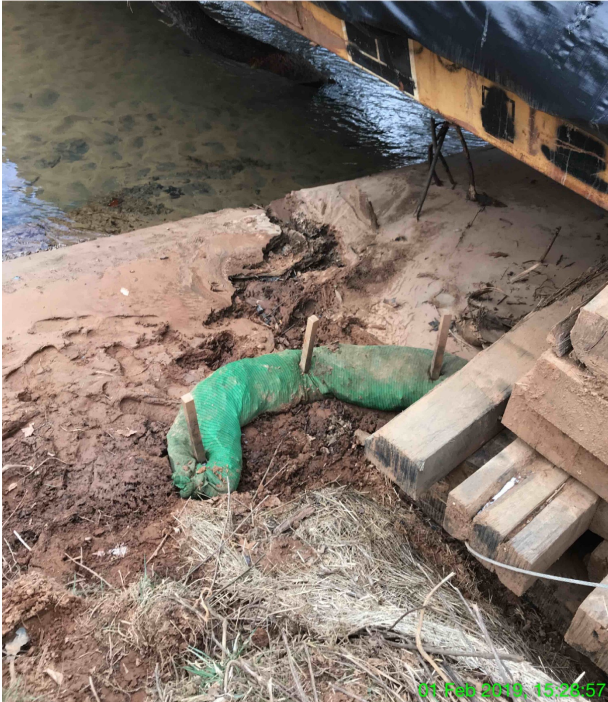
EXHIBIT K – The downstream side of the bridge over Little Creek which is the same location as Exhibit J above. The creek bottom which used to be rocky is covered in sediment. Sediment is piled on the banks. The erosion control sock had been recently installed when this photo was taken on February 1, 2019.
