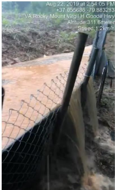
Figures 16 - 18 - August 22, 2019 Sediment-laden water flowing over, around, and through super silt fence and leaving the MVP ROW, several hundred feet upslope of the Blackwater River. Taken from a video accessible at Virginia Pipeline Violations Facebook page
