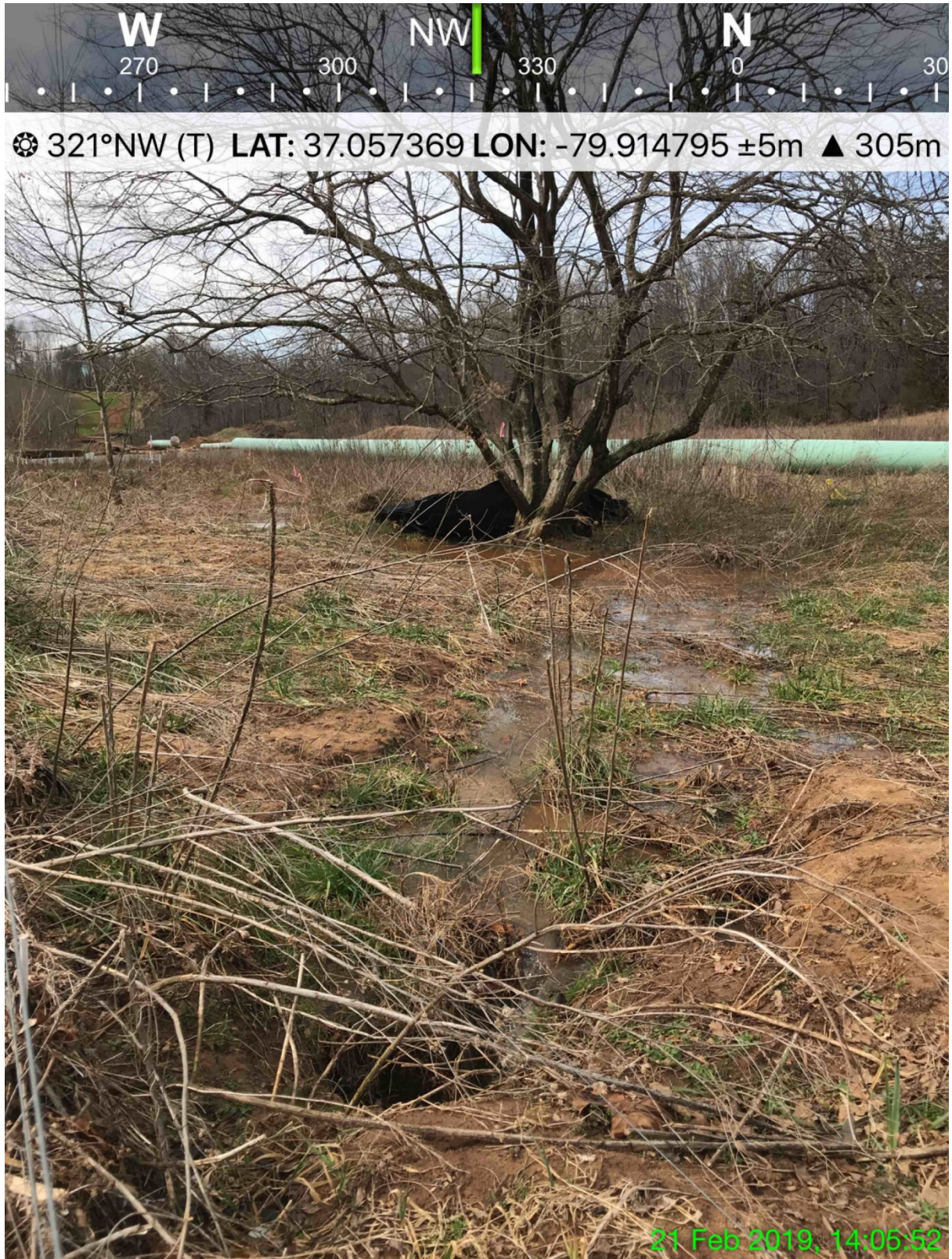
EXHIBIT D – Water flow from corridor toward Little Creek. The water that had been gushing from a hole is now eroding the creek bank.
