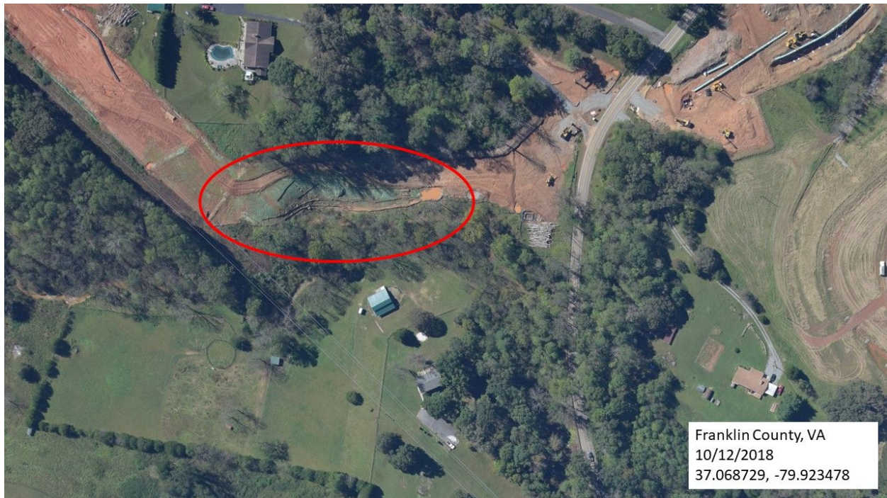
Figure 3: Image from 10/12/2018 shows E&S issues in area identified by red circle.
