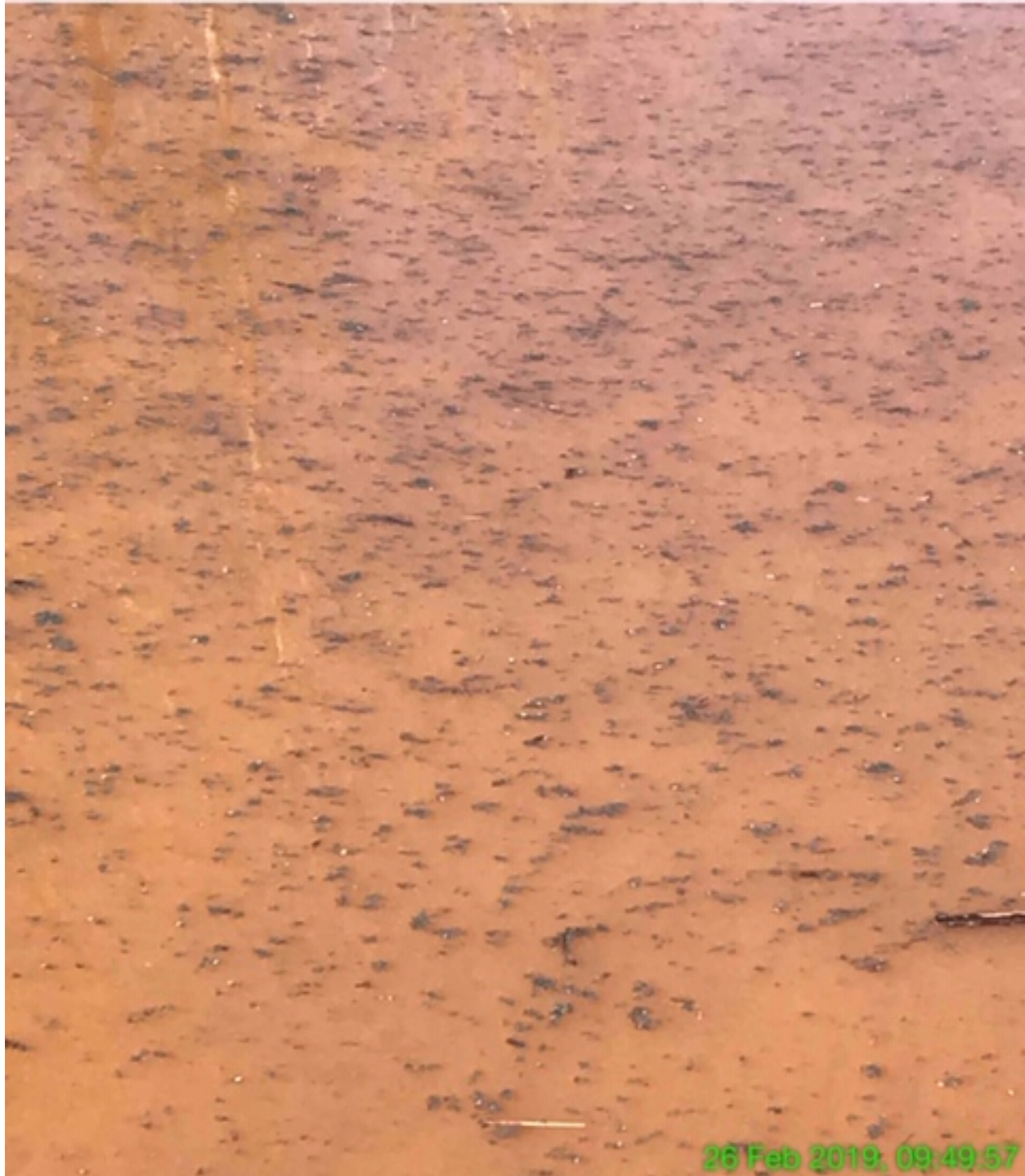
EXHIBIT V- Erosion control pellets dropped on the construction corridor where the stormwater has been ponding.
