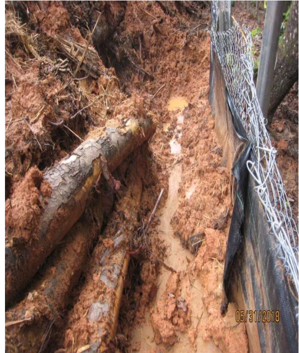
Sediment located on north side of SF
