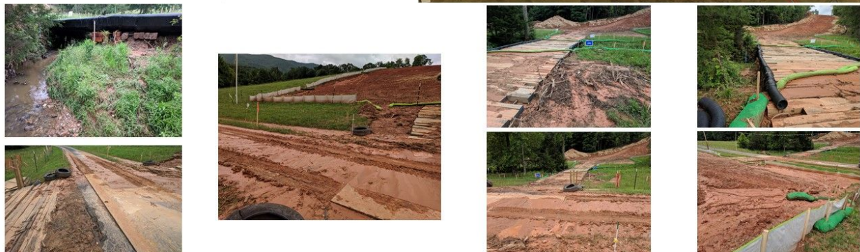
Figure 17: Potential violations reported May 28, 2018
