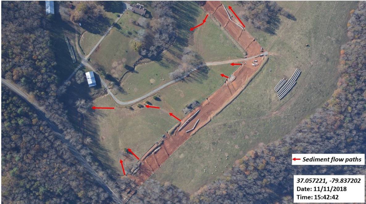
Figure 16: Flow paths where sediment leaves MVP construction ROW during rain events.
