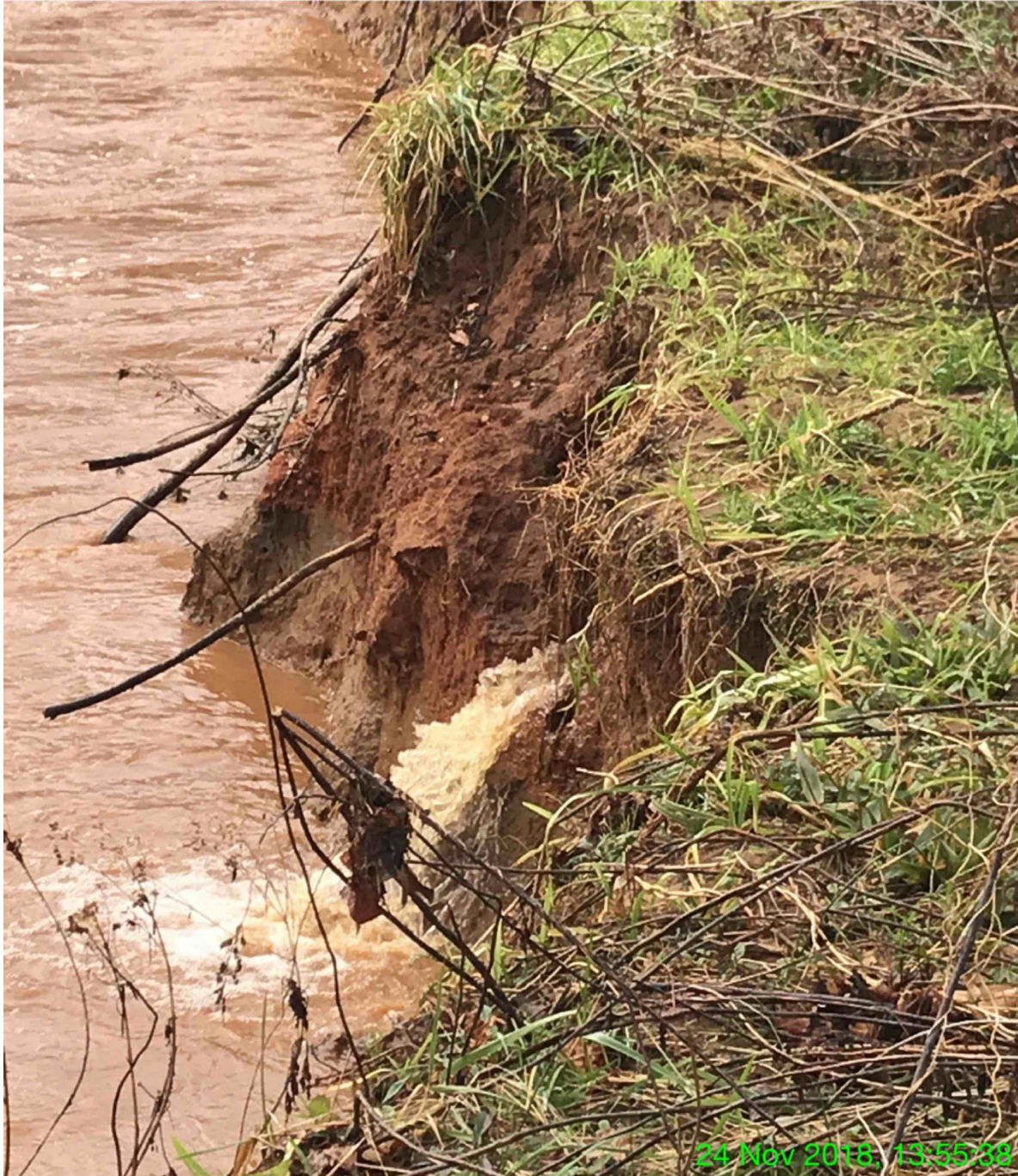
EXHIBIT A – Water gushing out of bank of Little Creek on Four Corners Farm, November 24, 2018. The gusher was discovered on November 15, 2018.
