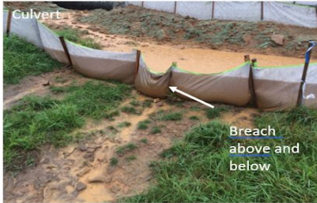
C. Another significant failure across the road. This one is pouring sediment off the LOD, into the stream and into SR 642 – SGT.
