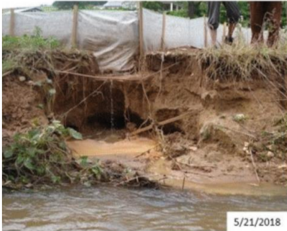
Figure 44 - A series of views of a collapsing stream bank on Teels Creek and Mountain Valley's attempts to repair the damage over several months in 2018. Source: Mountain Valley Watch Report, Appendix F to this report.
