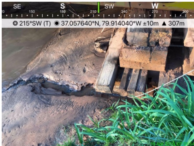
Exhibit LL – Sediment from ROW continuing to flow into Little Creek
