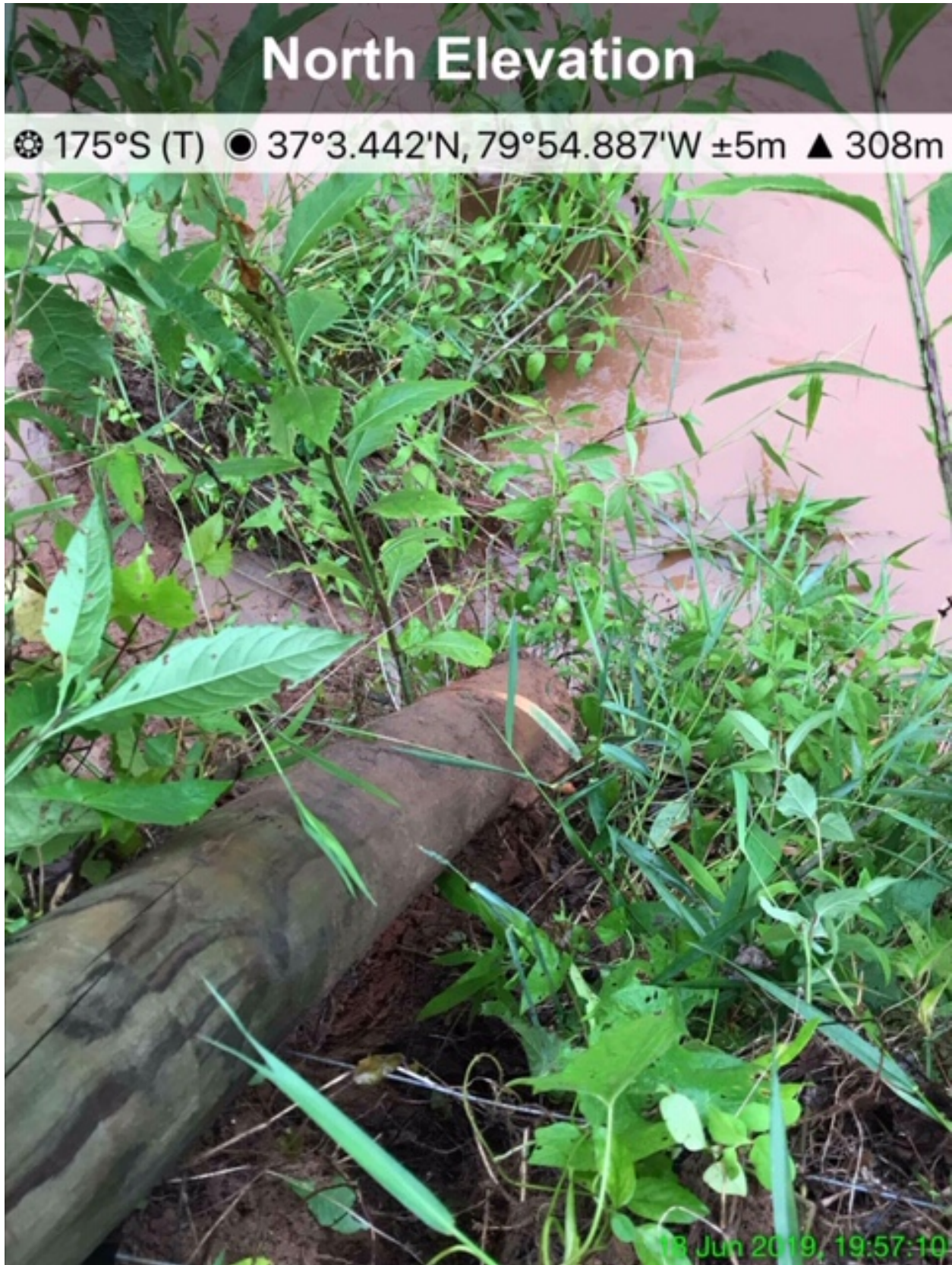
Exhibit OO – By June 18, 2019, the creek bank has eroded away from a fencepost that was at least six feet from the creek bank before construction started.
