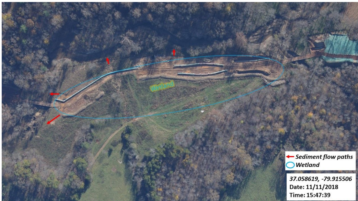
Figure 27: Trenching in a wetland; area is shown in ground photos below from table 1 & 2.
