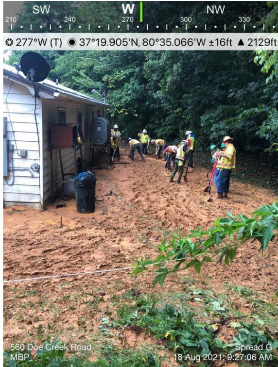
Figure 29 - Workers removing sediment from a landowner's property after the pollution "overwhelmed perimeter controls" at MVP sites. Action Log ID 5067. Source: MBP
