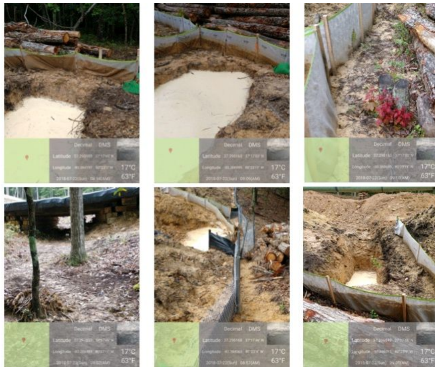
Figure 31: Photos from July 22, 2018 reported incident on Slayton property
