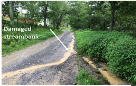
D. The ditch and culvert are still not stopping sediment flow down SGT. This photo at 7:12 am 05 Aug, over 24 hr after last significant rain on Thur , and before MVP Crews begin "cleanup". Why the strange diversion? This is where MVP traffic destroyed the stream bank.
