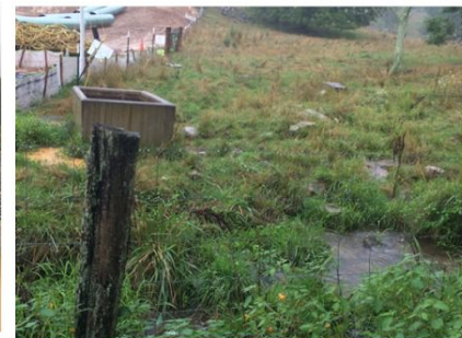
Stream coming from springs above the site is clear. Sediment above escaped the construction zone. Note position of cement water trough here and photo at left.
