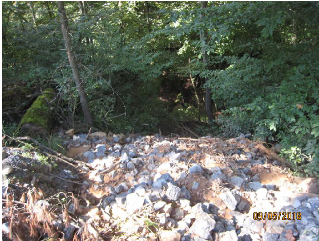
Photo 1: View from Access Road G/I 234 toward Kimballton Branch downslope of ESC failure Orientation: N/A
