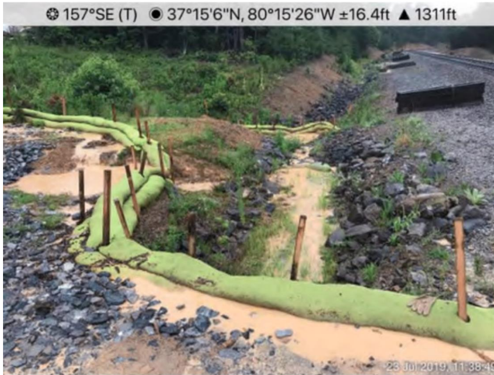
Figure 23 - Sediment-laden water undermining compost filters socks and discharging to a UT of Bradshaw Creek, July 23, 2019, DEQ Complaint inspection report, Source: DEQ [Bradshaw Creek is within the range of the Endangered Roanoke Logperch]
