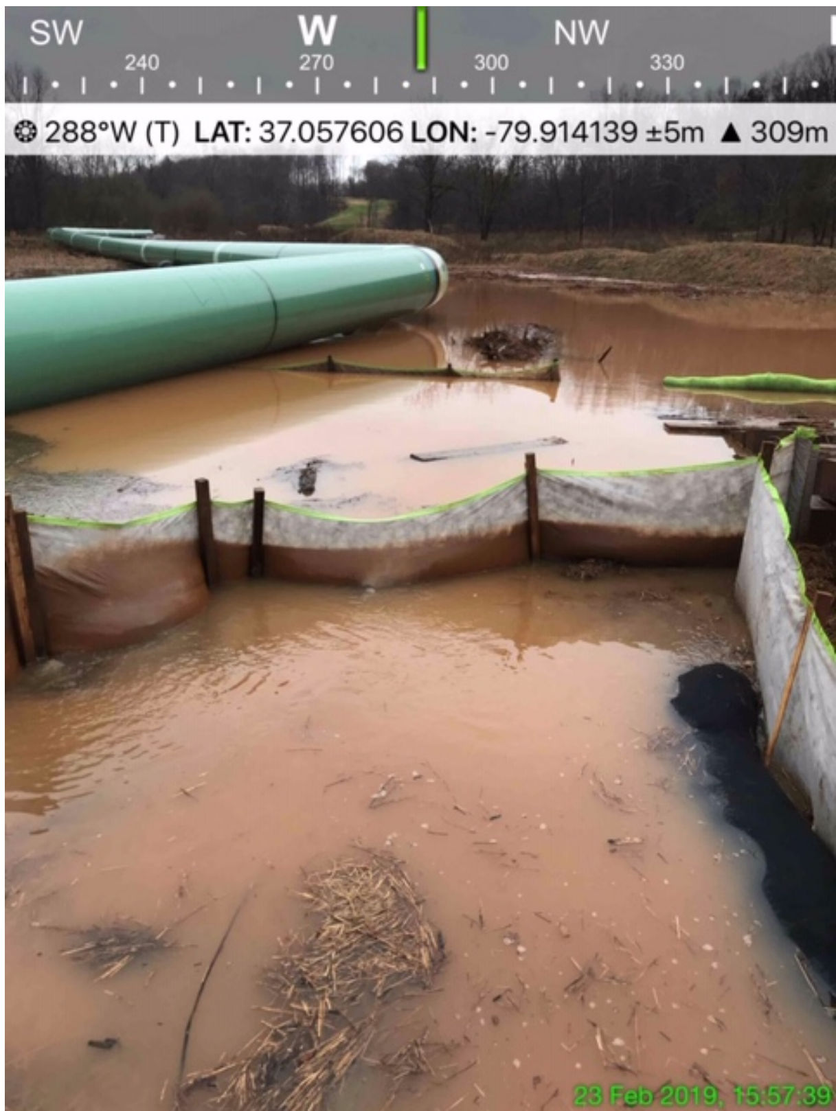
EXHIBIT M – The upstream side of the bridge over Little Creek on February 23, 2019. This is the same location as Exhibit I.
