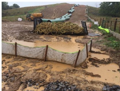
Silt fence in photo failed and has been “reconstructed”, but still actively failing. Standing in approximate centerline, looking eastward toward highly sloping double bench system, and away from SGT.
