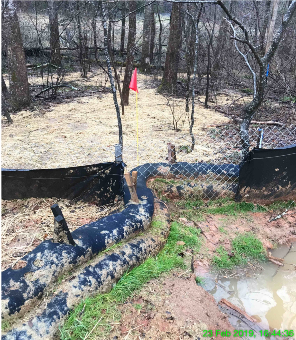
EXHIBIT N – Sediment-laden runoff has flowed from the construction corridor. MVP contractors have covered the sediment with straw. The photograph in Exhibit O shows what is typically found under the straw carpets.
