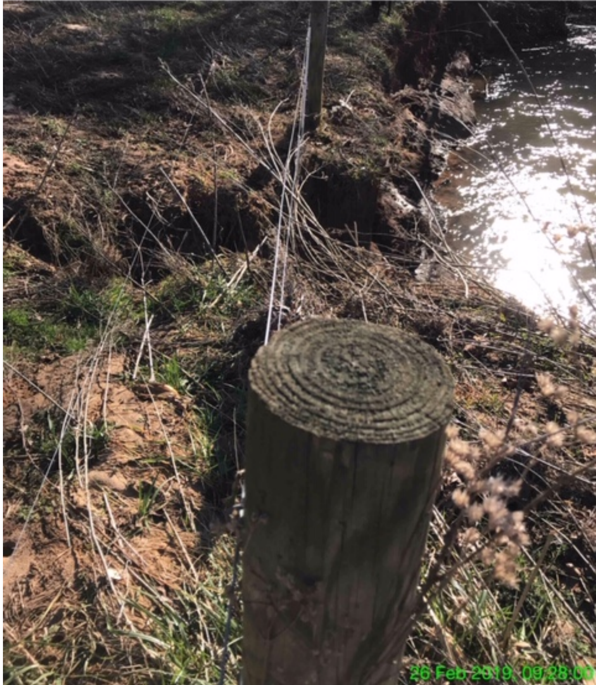
EXHIBIT G – The gusher had eroded to a full ditch that discharges sediment-laden runoff to Little Creek.
