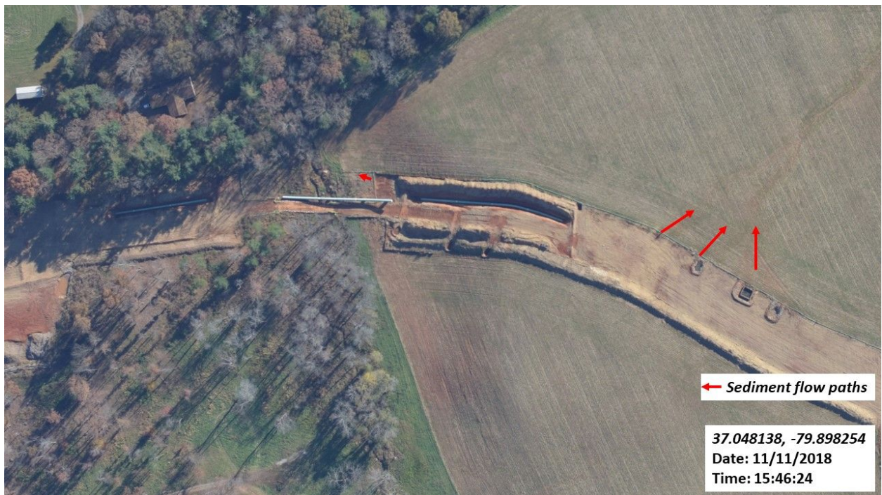
Figure 19: Sediment flowing into adjacent field.
