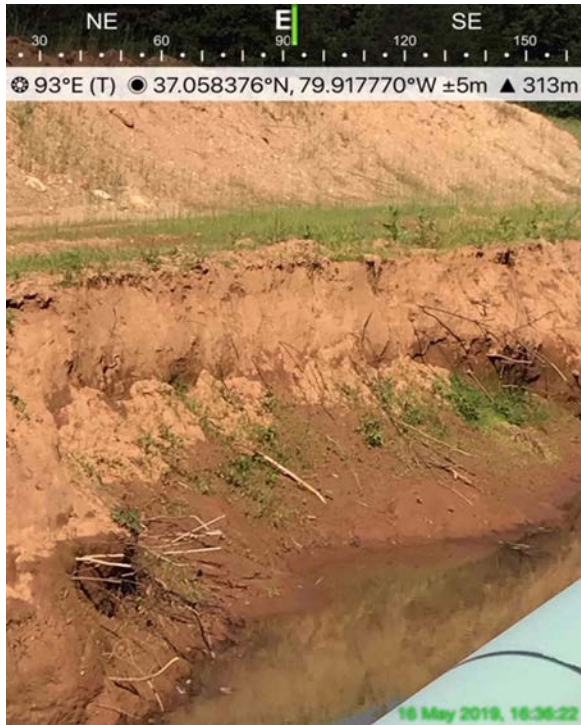
Exhibit HH- Sprouted grass and erosion along ROW
