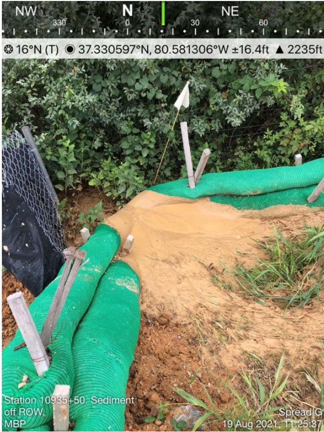
Figure 30 - Sediment overflowing compost filter socks, deposited off MVP ROW near UT to Doe Creek, August 19, 2021, Action Log ID 5081, Source: MBP
