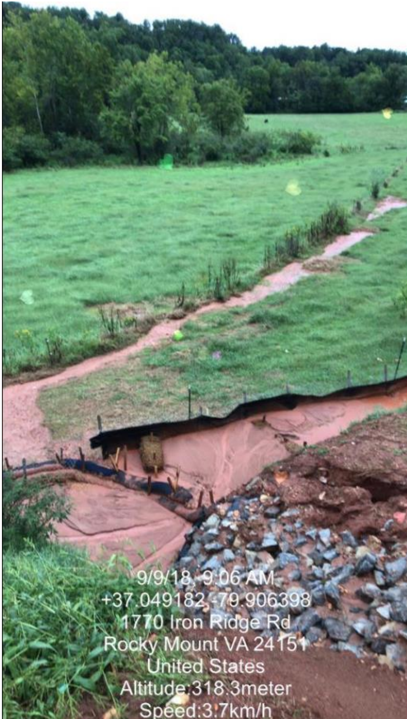
Figure 12 - Sediment off ROW near UT to Little Creek, September 9, 2018, Source: citizen observer, accessible at Virginia Pipeline Violations Facebook page
