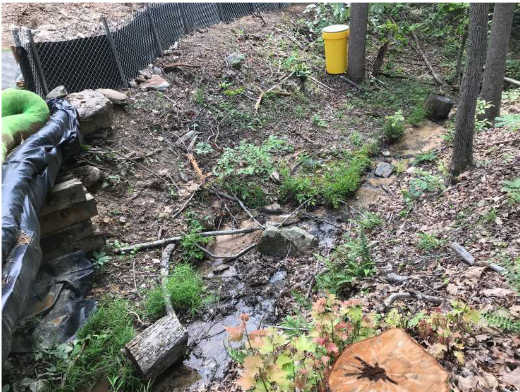
Photo 2: Sedimentation and woody debris downstream of bridge crossing Orientation: Downstream
