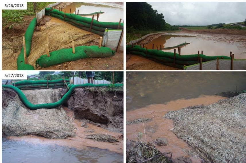
Figure 14: Potential violations reported - May 26 - 27, 2018
