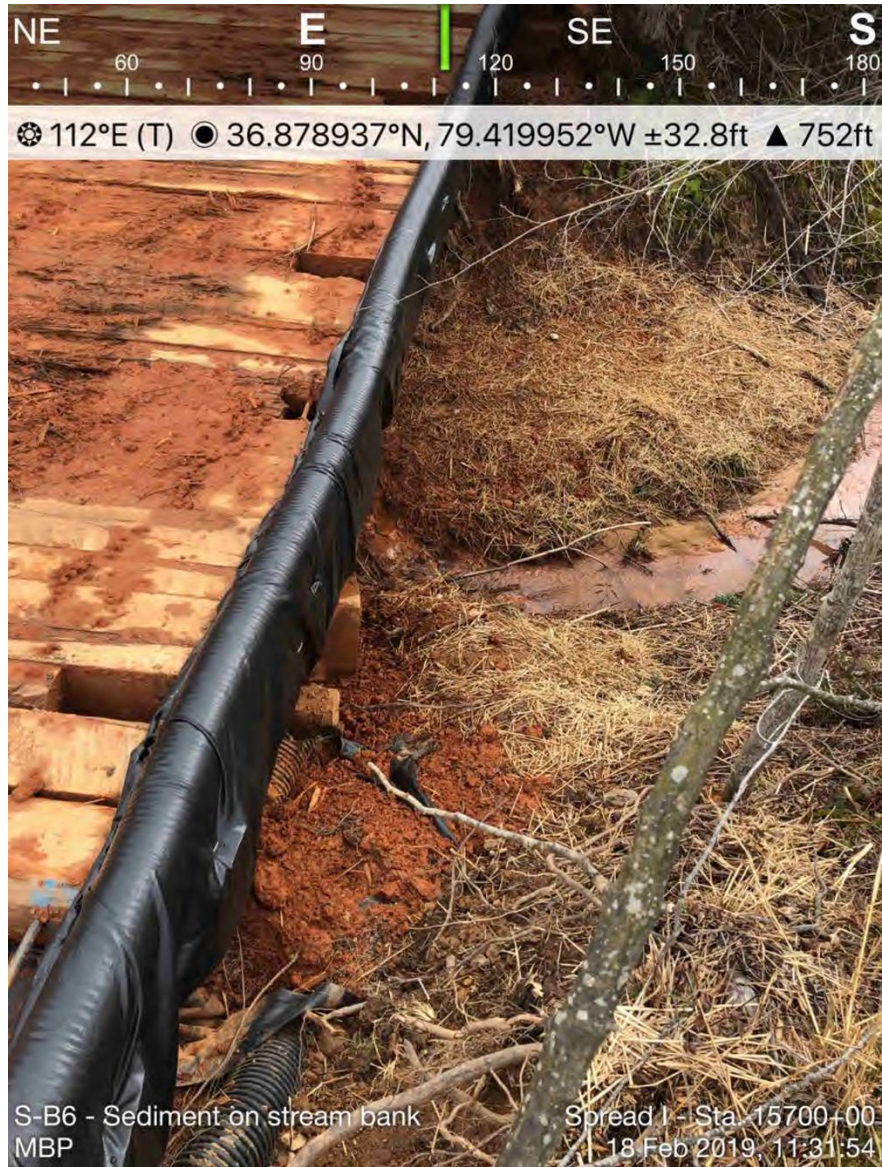
Figure 49 - Sediment deposited off ROW onto streambank at UT to Pole Bridge Branch, February 18, 2019, Action Log ID 1901, Source: MBP [deadline to remove extended "due to wet ROW," not removed until 6 days after deposited]
