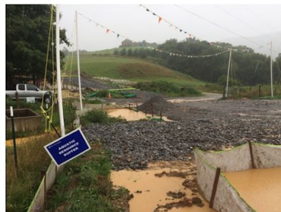
Looking westward toward SGT. Failed mulch socks and silt fencing. Note thick gravel layer placed to fill and hide pooling mud between silt fence and SGT, is not effective in slowing sediment loss. Besides BMP failure, sediments are clearly entering 1) an Aquatic Resource Buffer, 2) a State Road, 3) a
