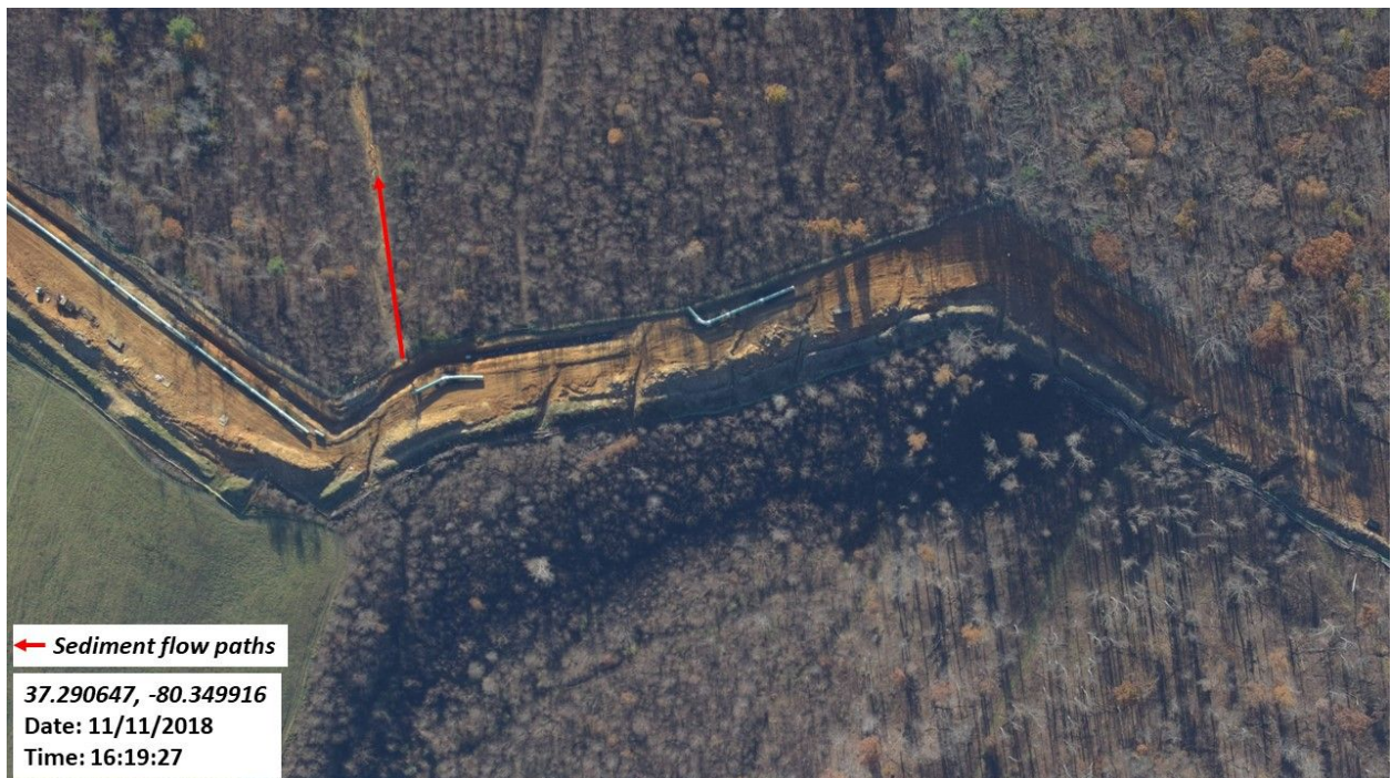
Figure 37: Sediment flowing into stream channel from right of way.
