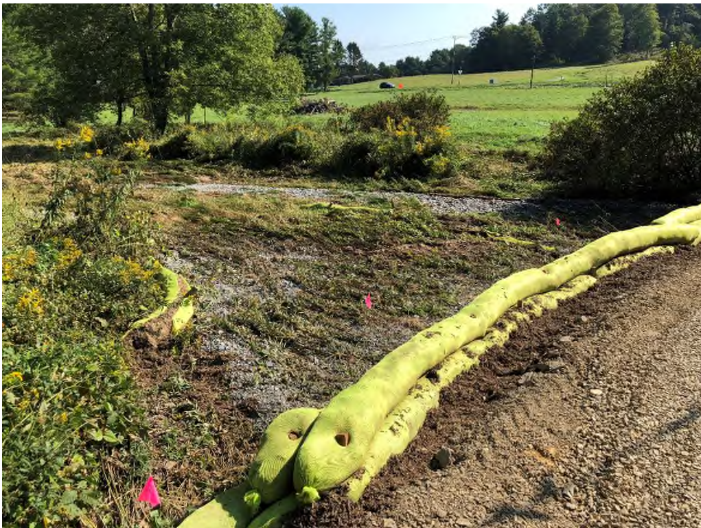
Photo 2: Gravel from Access Road 288 in Wetland IJ-10 due to ESC failure Orientation: N/A
