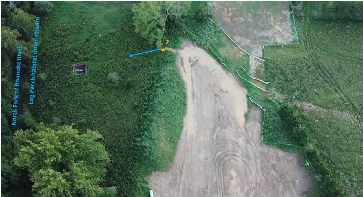
Figure 11: Location 2 is another location at this site where sediment laden stormwater continually flows into the North Fork of the Roanoke River during rain events.
