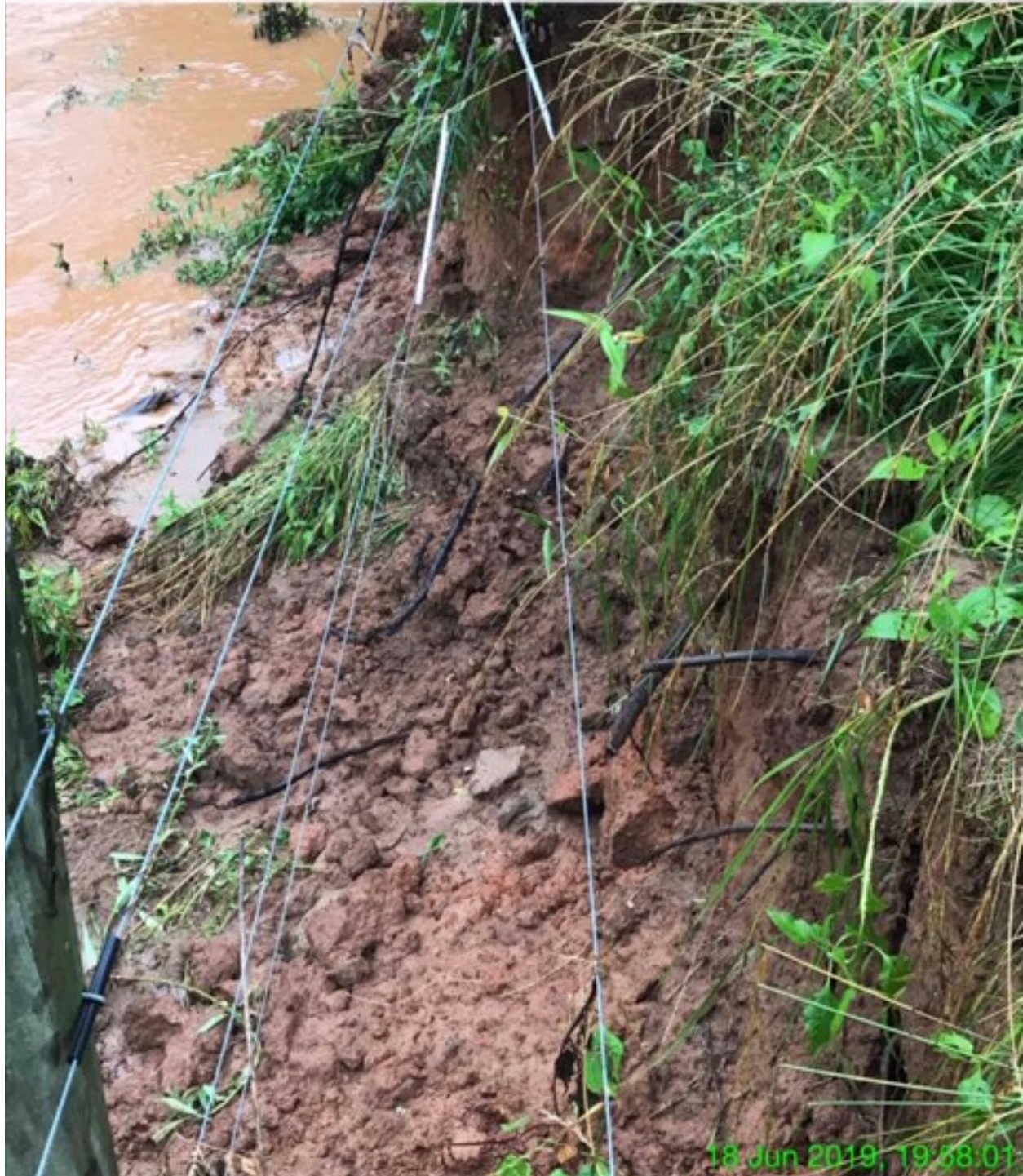
Exhibit PP – By June 18, 2019, the creek bank has eroded several feet beyond a fencepost that was at least six feet from the creek bank before construction started.
