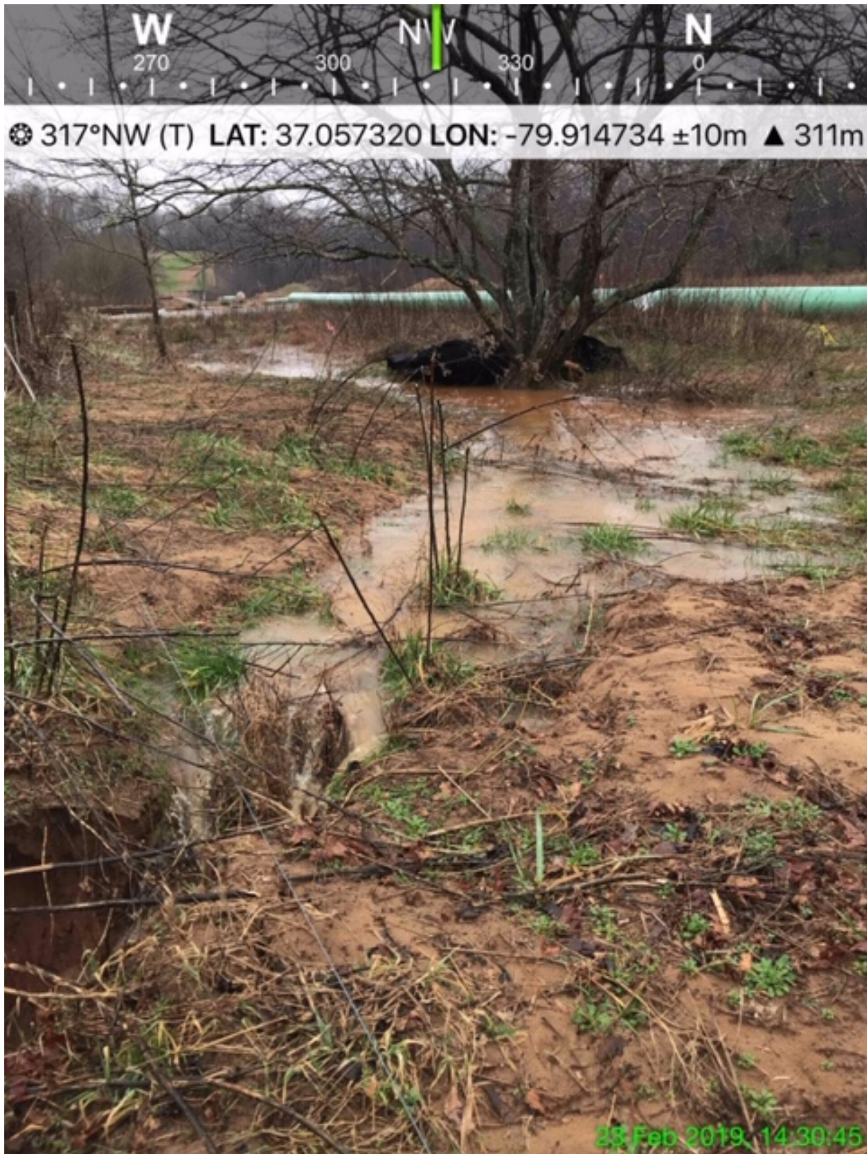
Exhibit E – Same location as in Exhibit D, two days later, after 2.5 inches of rain. The drainage into the creek is collapsing. The fence wire is visible on the left.
