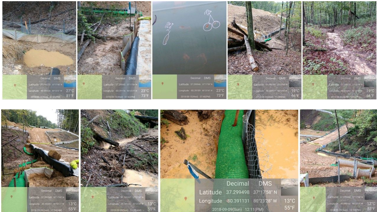
Figure 7: Ground images showing issues along the MVP construction LOD
