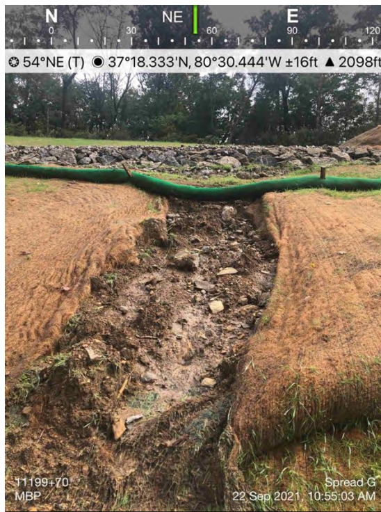
Figure 24 - Compost filter sock undermined near Sinking Creek, September 22, 2021, Action Log ID 5196, Source: MBP
