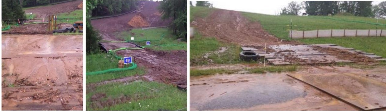
Figure 16: Potential violations reported May 18, 2018
