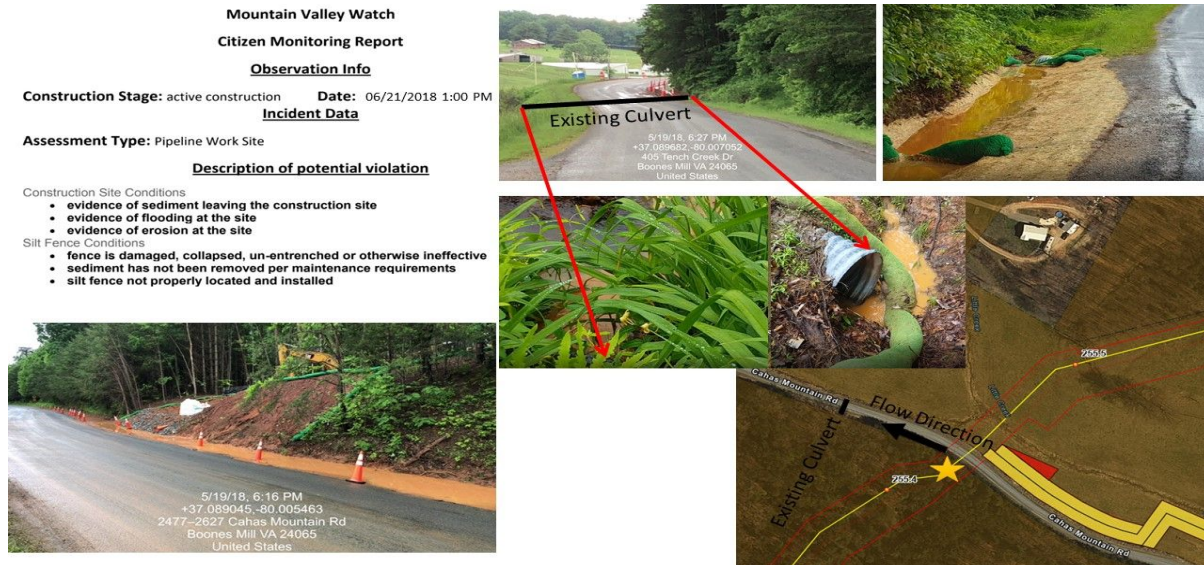
Figure 9: Cahas Mountain Road mudslide site showing location of sediment entry to Little Creek through an existing culvert beneath road.
