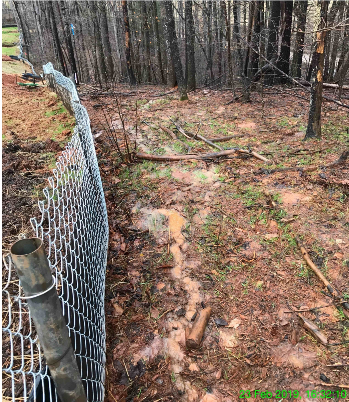
EXHIBIT T – Sediment-laden runoff flowing from the construction corridor.
