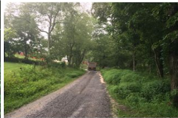
This is 05 Aug at 13:15 hr Friday. After crew departure, a gravel truck arrives and delivers a last load of gravel to the worksite. Note that the road is still receiving copious amounts of sediment and they enter the stream at the damaged streambank.
