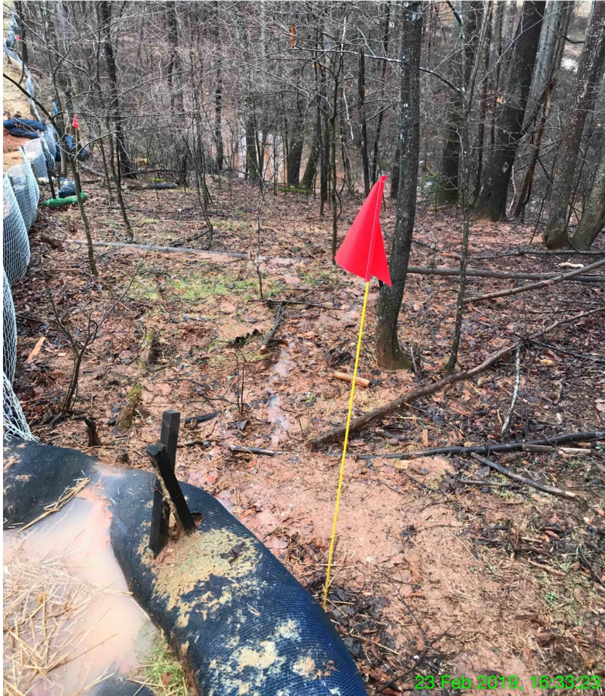
EXHIBIT S – Sediment-laden runoff has flowed from the construction corridor.
