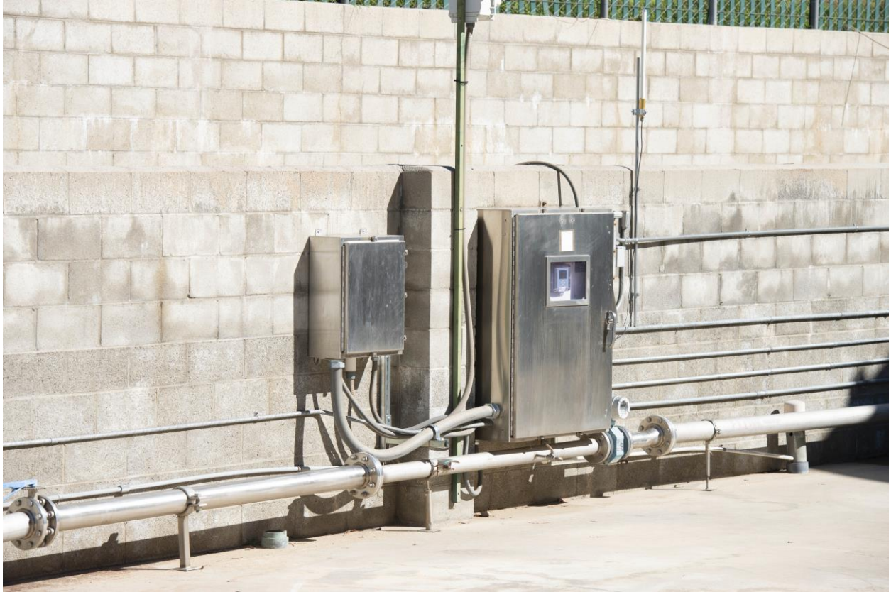
(c) the meters that measure the water flows
