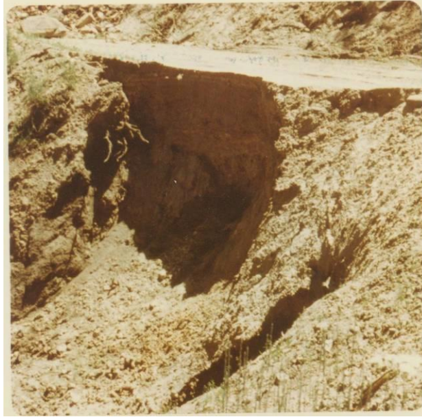
Poorly sorted fill materials and inadequate drainage result in failures as shown above.
