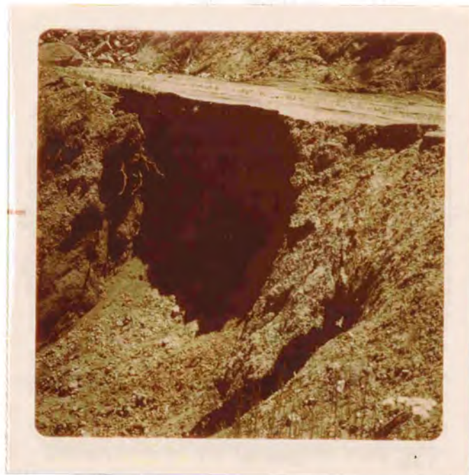
Poorly sorted fill materials and inadequate drainage result in failures as shown above.
