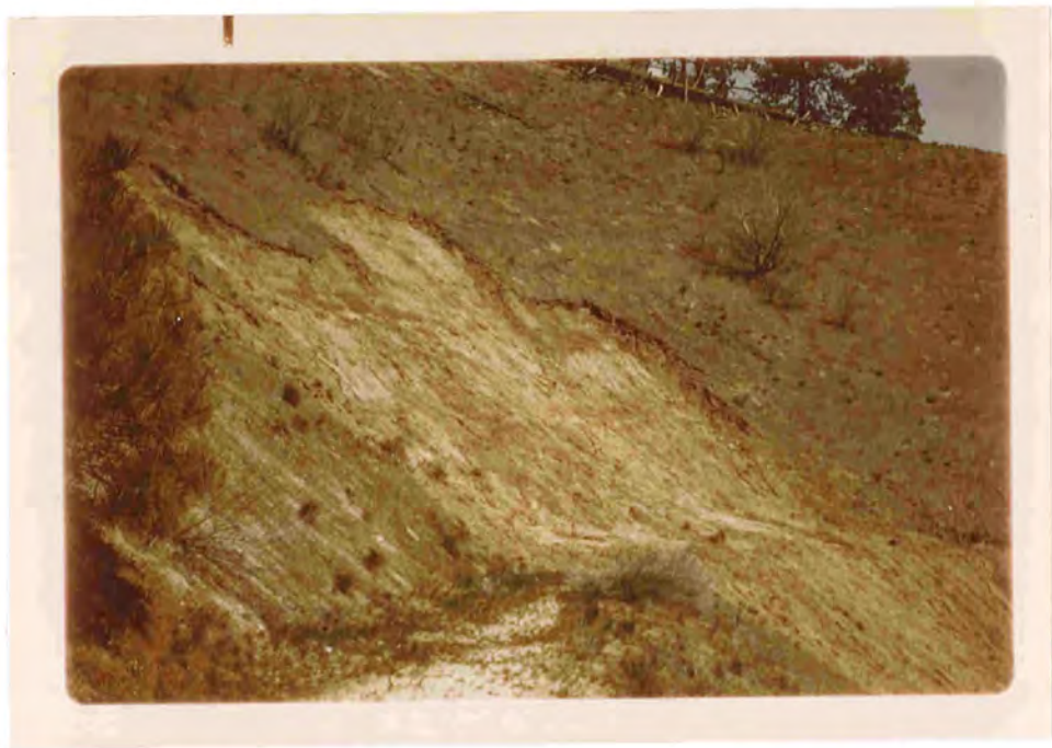
Mass failures can many times be related to soil and/or bedrock characteristics.
