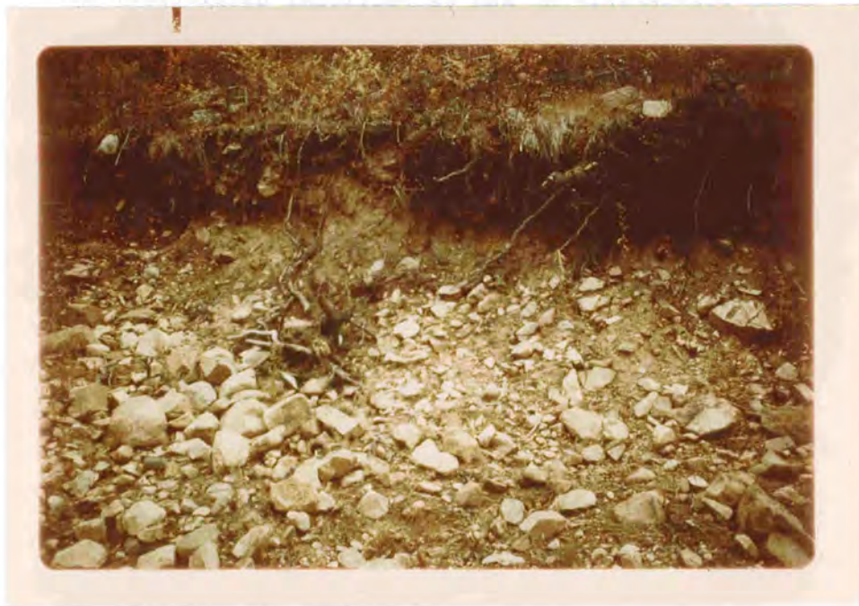
Competent rock fragments as shown in the above exposed profile aid the stability of cut slopes caused by road construction.
