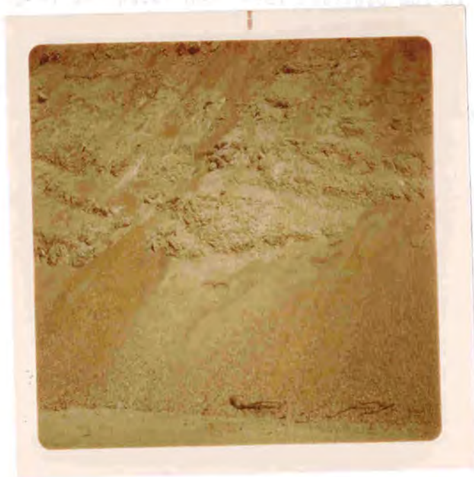
Soft granitic bedrock of a spalling nature causes road maintenance costs after a road is built.
