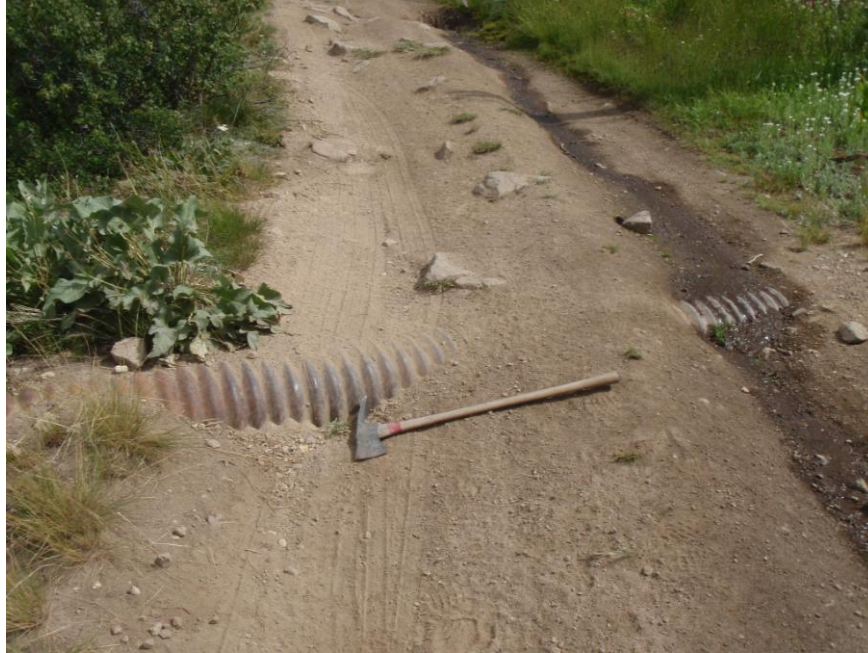
Photo 3. Photo of a road segment of NFSR 583 leading to Bear Valley Mountain Lookout. Although, this road delivers very little sediment, much of the road is badly eroded and yields high sediment production rates.
