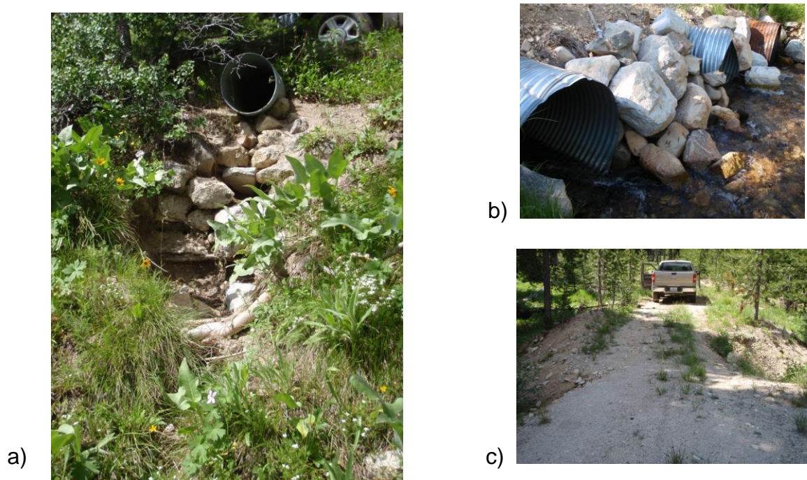
Photo 2. Photos of high delivery drain points. a) Gully at outlet of highest delivering drain point in the entire basin, located on NFSR 569. b) Sack Creek stream crossing on FR 582, one of top 24 highest delivering drain points in basin. c) Eroded and dilapidated stream crossing of Bearskin Creek on NFSR 563C1.
