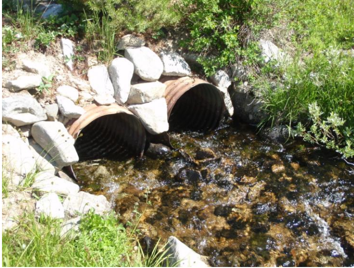
Photo 5. Many stream crossings such as this one have more than one pipe to prevent blockage or flow diversion. SBI figures do not account for the presence of multiple pipes which means some SBIs may predict higher risk than what actually exists.
