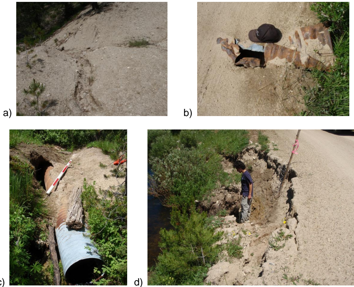
Photo 4. Examples of drain point condition problems including: a) erosion at a broad based dip, b) a rusted and damaged ditch relief culvert, c) a stream crossing with flow around and possibly over the pipe, and d) a non-engineered feature where the stream is cutting into the road fill material.
