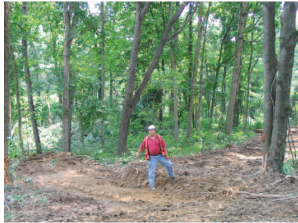
Fig. 16.6 Water bar constructed on a modern skid trail following guidelines developed in the Fernow Experimental Forest in the 1950s. (Source: http://www.muskingumtrees.com/water-bar.jpg )
