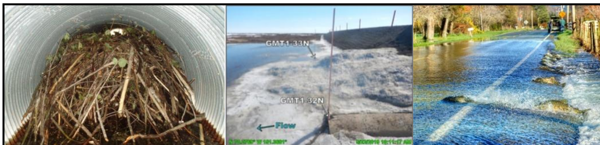
Figure 4. Examples of common causes of culvert blockages: beaver activity (left), ice on Alaska’s North Slope (middle), and flooding (right). Images from lizottesolutions.com, Michael Baker International 2019, and thirstontalk.com.
