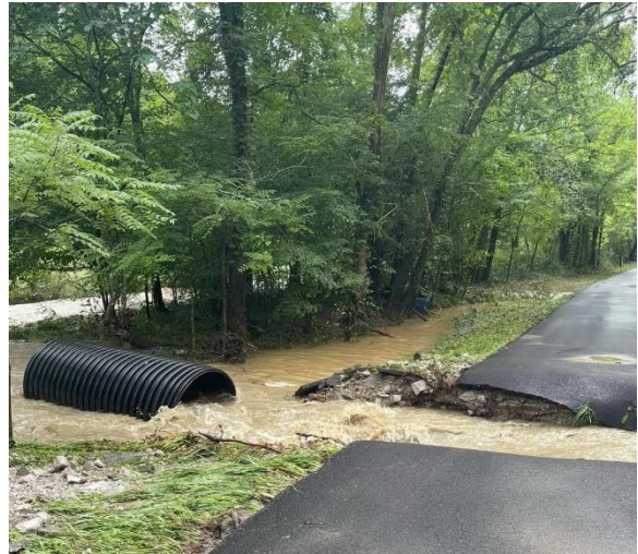
Little Wolf Creek Road washed out in the July 2022 mega flood. Photo by Sue Moses, used with permission.
