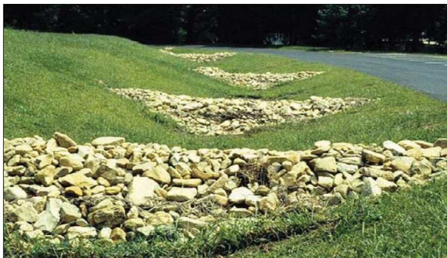
Figure 11.—A series of rock check dams in a grassed swale to create storage potential within the swale. Photo by Virginia Department of Conservation and Recreation (1999), used with permission.
