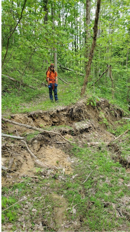
Figure 16. Slump along the Red Bird Crest Trail in the Mosely Fork area
