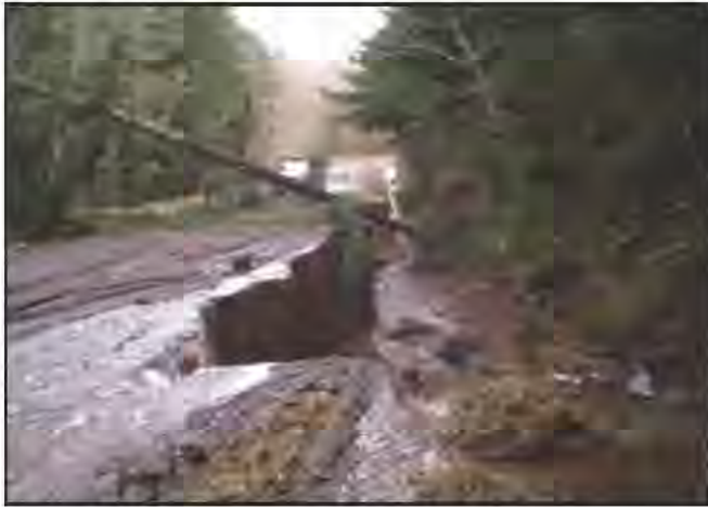
Figure 4.12—Ditch scour along an Olympic National Forest road. Changes in hydrology and physical watershed processes with climate change will likely increase the incidences of culvert capacity being exceeded, fill slope failures, and development of first-order channels that can affect roads and related structures. (Photo courtesy of USDA Forest Service, Olympic National Forest.)
