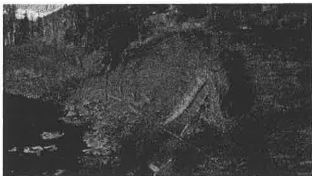
Sept 2012 Eroding road bank Sweetwater Valley
