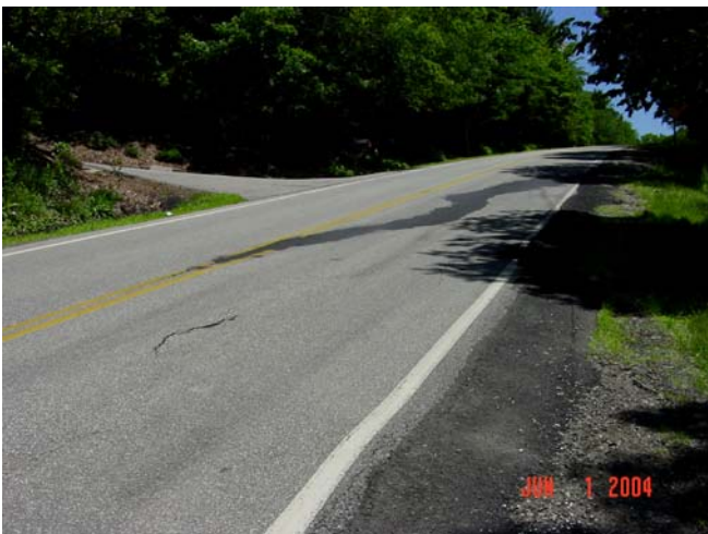
Fig. 17 Highland road fill before stabilization with launched soil nails, Summit County, Ohio. Note asphalt patch preserving evidence of incipient fill failure. Photo: Weber et al. 2005
