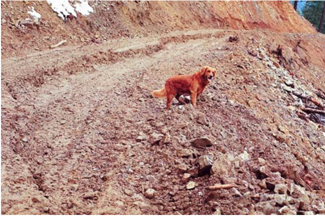
Fig. 14 Slump in road fill on logging road in Klamath National Forest, California
