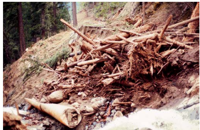
Fig. 8 Stream crossing fill failure initiates debris flow. Note broken culvert plugged with bed load (Klamath National Forest, California)
