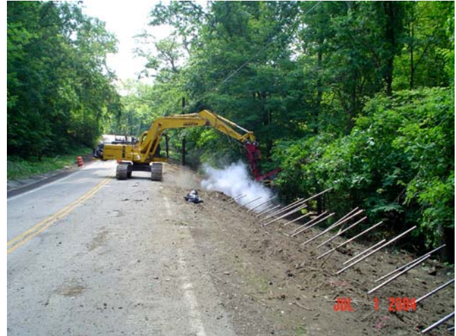
Fig. 18 Highland road fill after stabilization with launched soil nails, Summit County, Ohio. Photo: Weber et al. 2005
