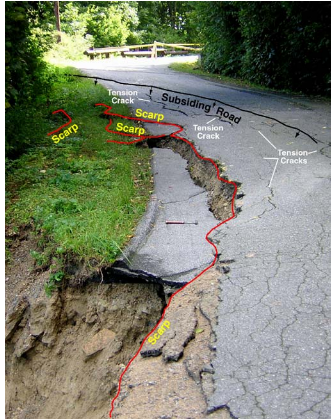
Fig. 15 Warnings signs of unstable fill (subsidence, tension cracks, scarps). Lower left corner of photo shows major scarp of road-fill failure that mobilized into a debris flow from heavy rain remnants of Hurricane Francis in 2004 in Bear Rock Estates subdivision, Henderson County, North Carolina. Photo: North Carolina Geological Survey
