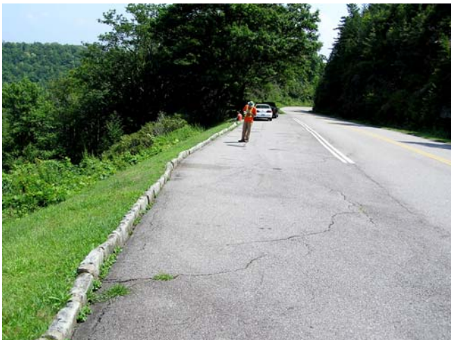
Fig. 19 Grass in cracks and curb separation in scenic overlook (fill) on steep slope on Blue Ridge Parkway in North Carolina: signs of long-term movement of fill appropriate for hazard/risk analysis and monitoring
