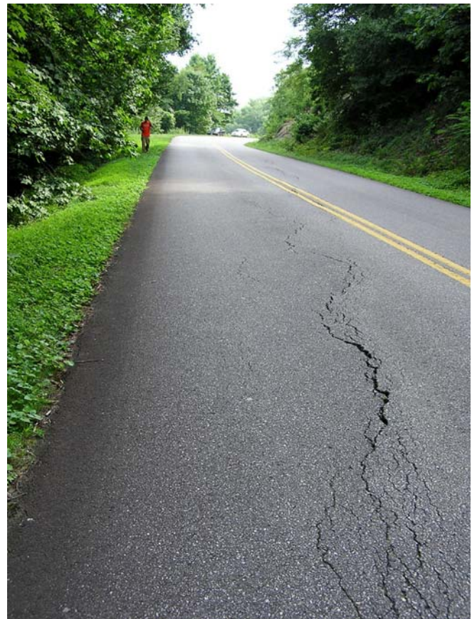
Fig. 9 Arc-shaped tension cracks in road fill on Blue Ridge Parkway near Mount Mitchell, North Carolina (August 1, 2005)
