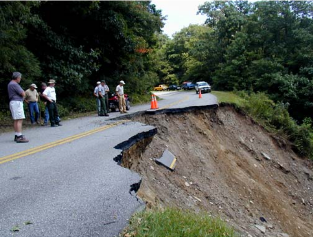
Fig. 4 Blue Ridge Parkway (Milepost 348) fill-slope failure that initiated Bear Drive Branch debris flow on Pisgah National Forest, North Carolina (Hurricane Frances, September 2004)
