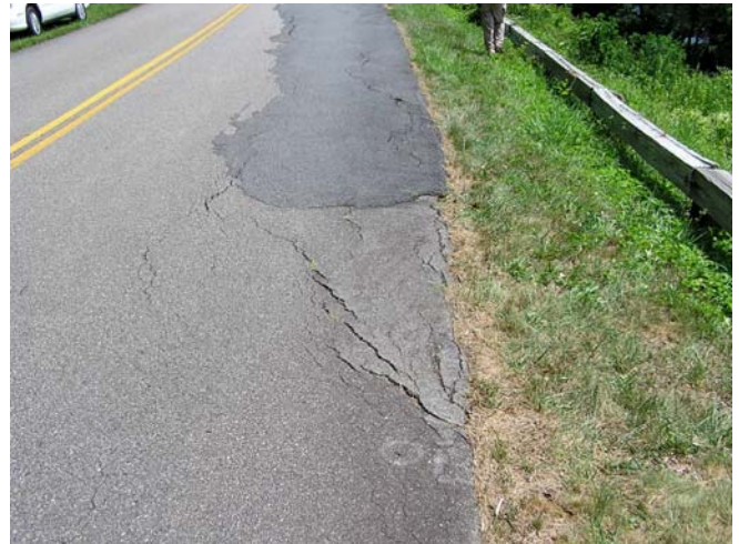
Fig. 12 Incremental failure evidence with asphalt patching in road fill on Blue Ridge Parkway north of Mount Mitchell, North Carolina (August 2, 2005)
