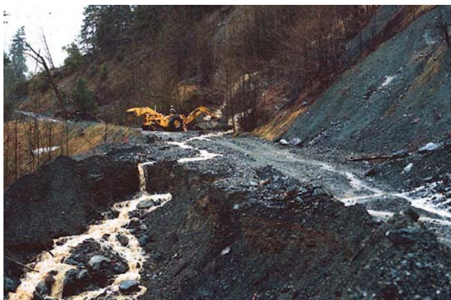
Fig. 16 Plugged culvert creates two fill-slope debris-flow hazards: (1) a temporary dam at the plugged culvert, and (2) overflow leading to failure of another fill. Road in Klamath National Forest, California
