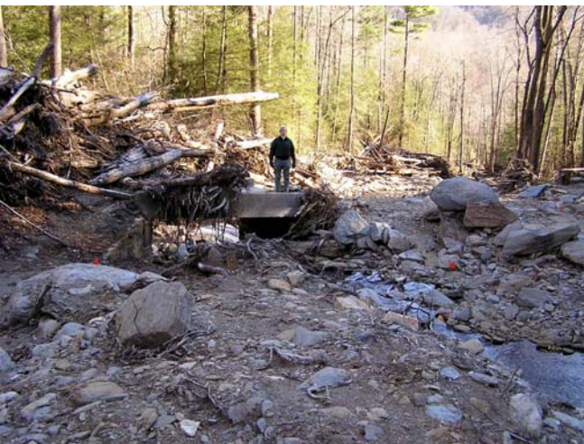
Fig. 5 Impact of September 8, 2004 debris flow at Curtis Creek road more than 2 km downslope from initiation site at Blue Ridge Parkway fill-slope failure (Milepost 348). View downstream to bridge crossing of Bear Drive Branch on Pisgah National Forest, North Carolina
