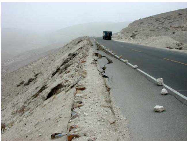
Fig. 20 Partial failure of fill slope on Pan American highway near the town of Tambillo, Peru, June 23, 2001 earthquake damage (Wartman et al. 2003). Photo: US National Science Foundation-sponsored geotechnical reconnaissance team
