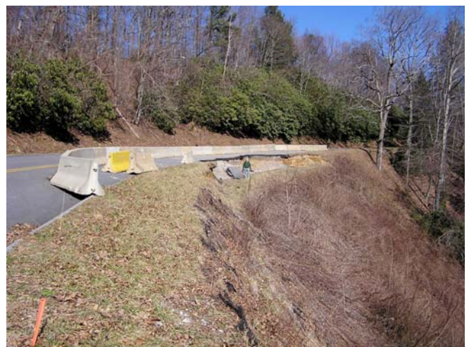
Fig. 13 Slump in road fill on Blue Ridge Parkway (MP345) north of Mount Mitchell, North Carolina (January, 2005). For scale, note person standing below road
