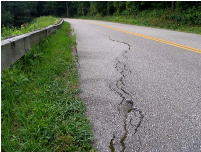
Fig. 10 Arc-shaped tension cracks in road fill on Blue Ridge Parkway south of Linville Falls, North Carolina (August 3, 2005). Photo: Scott Eaton and Bob Sas
