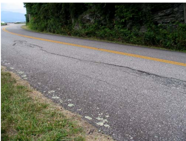
Fig. 11 Graben in road fill on Blue Ridge Parkway south of Linville Falls, North Carolina (August 3, 2005). Photo: Scott Eaton and Bob Sas
