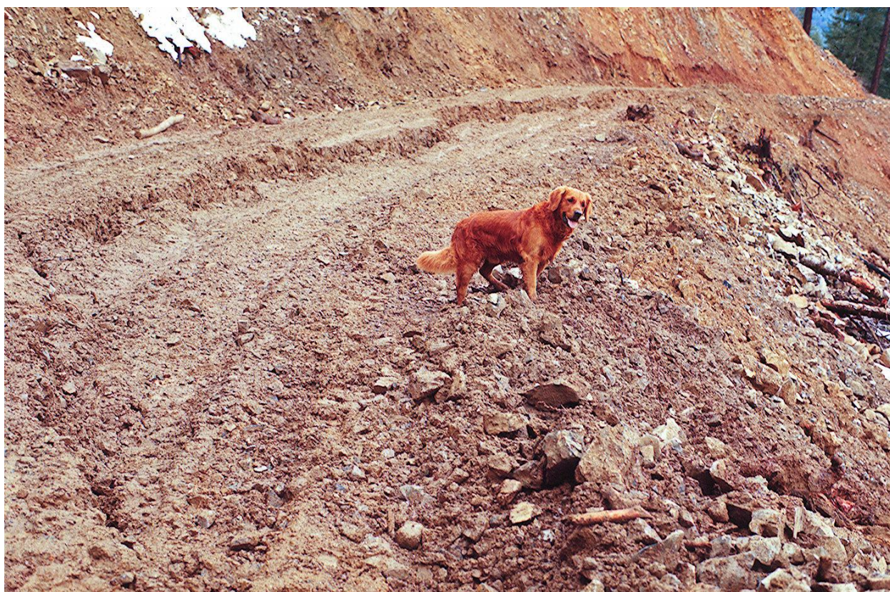
Figure 3 - Example of landslide hazard caused by progressive failure of road fill. Adding more fill to level up the road surface would increase the hazard and may lead to total failure of the fill and a debris flow that could gouge a path of destruction for hundreds or thousands of feet downslope.
