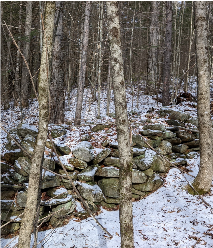
Vulnerable stone wall, Charleston Rd. Piermont, 2022
