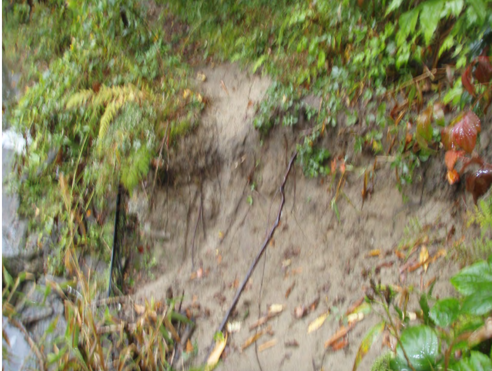
Boater Created Erosion Site B-5 @ 35 02 51.54 N 83 07 14.52 W on Sept. 25, 2015.
