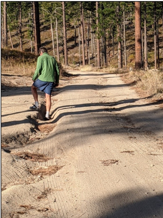
Figure 3 – Lack of BMP maintenance
