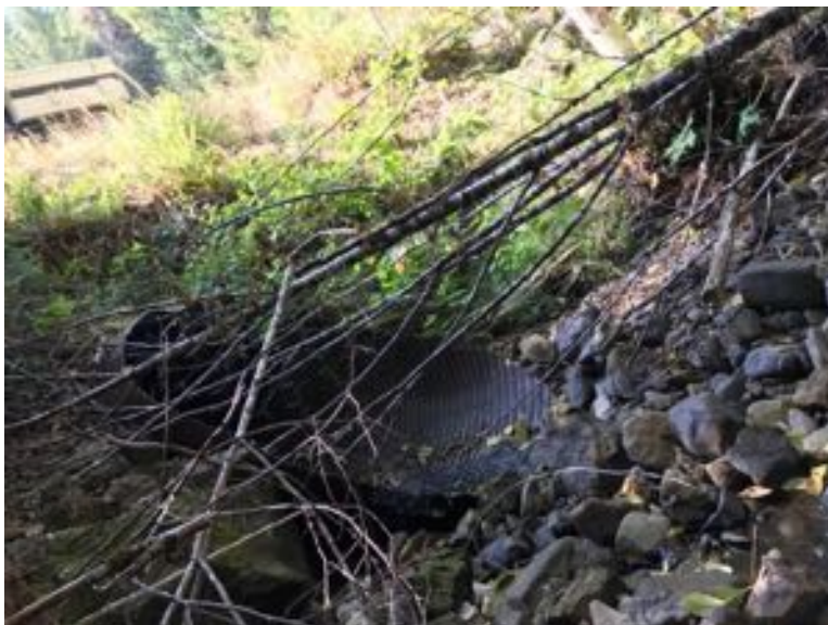
Figure 3: Elk Creek culvert- undersized at FSR1131101
