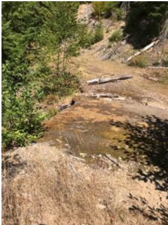
Figure 5: FSR1131101 at Unit 14. Asphalt spillover.
