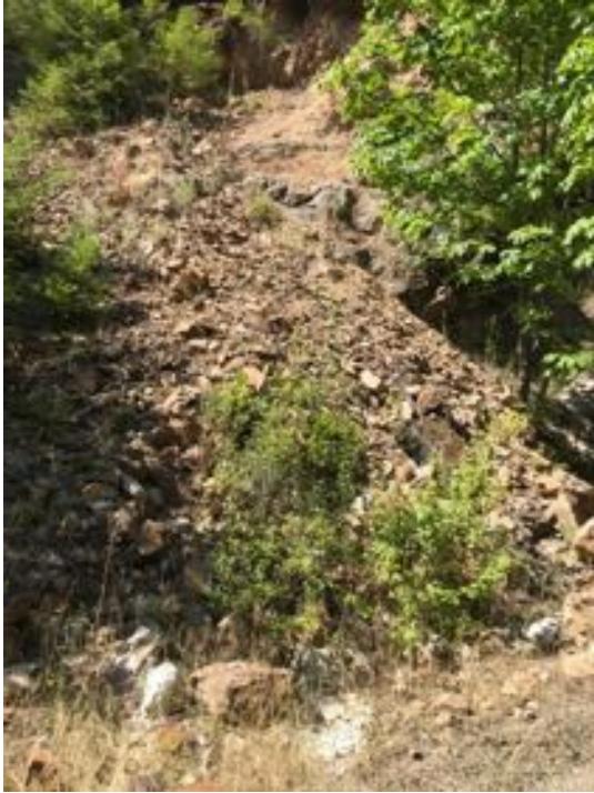
Figure 7: FSR1131108 along Unit 7. Small rockfall
