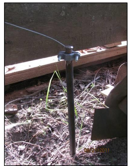
Grounding rod photo courtesy of Gillian Sanders
