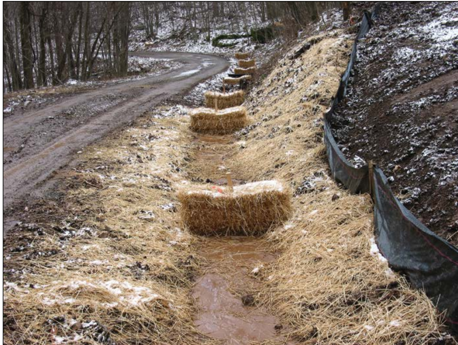
Straw bales installed in a ditch line to slow drainage and capture sediment, and straw mulch and silt fence on a cutbank used to control erosion after construction of an access road to a natural gas well pad. (Photo by U.S. Forest Service, Northern Research Station.)
