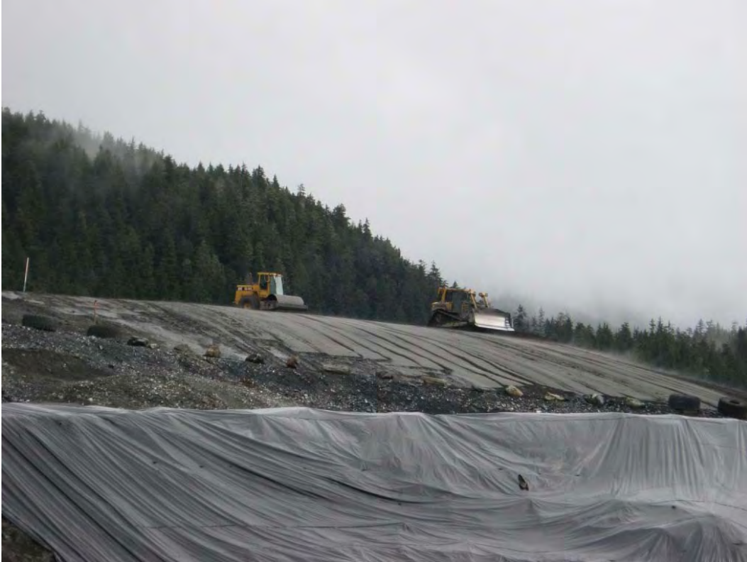
Photo 5: After spreading, the tailings are compacted with a self propelled, vibrating drum compactor
