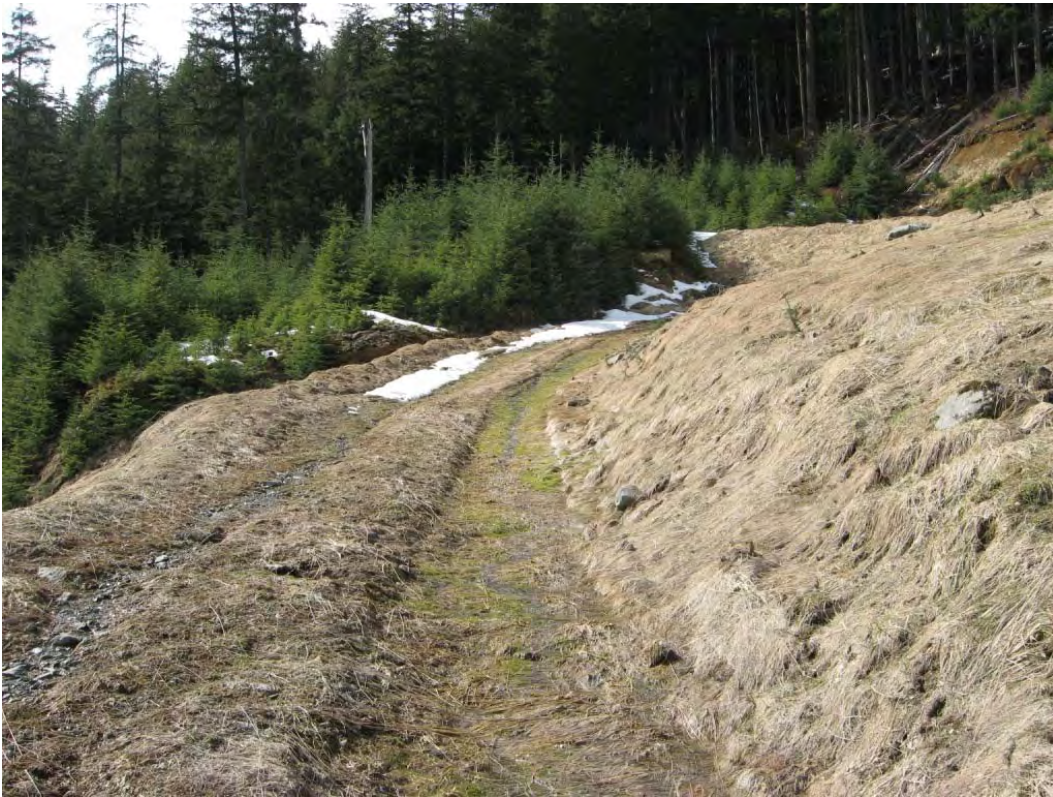
Photo 15: Access ramp across the front of the reclaimed and revegetated production rock at Pit 405
