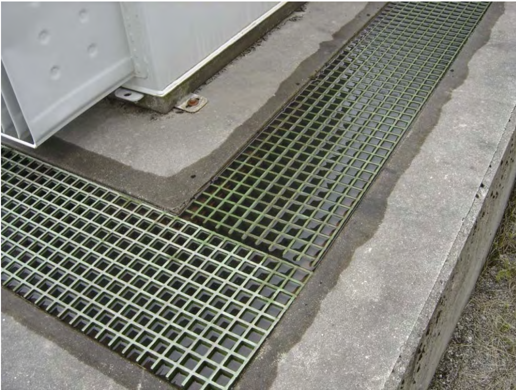
Photo 3: Transformer Secondary Containment
