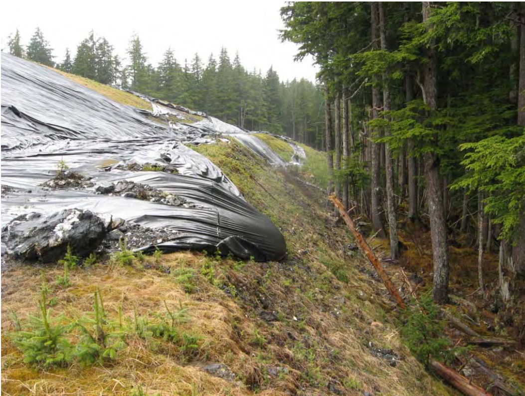
Photo 14: Part of Site E has been covered by a geomembrane to reduce infiltration in the short term
