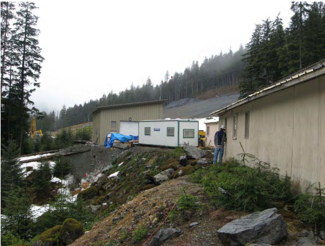
Photo 12: Side view, looking west at mine buildings which have been constructed on fill within Site C, part of Site C has no production rock
