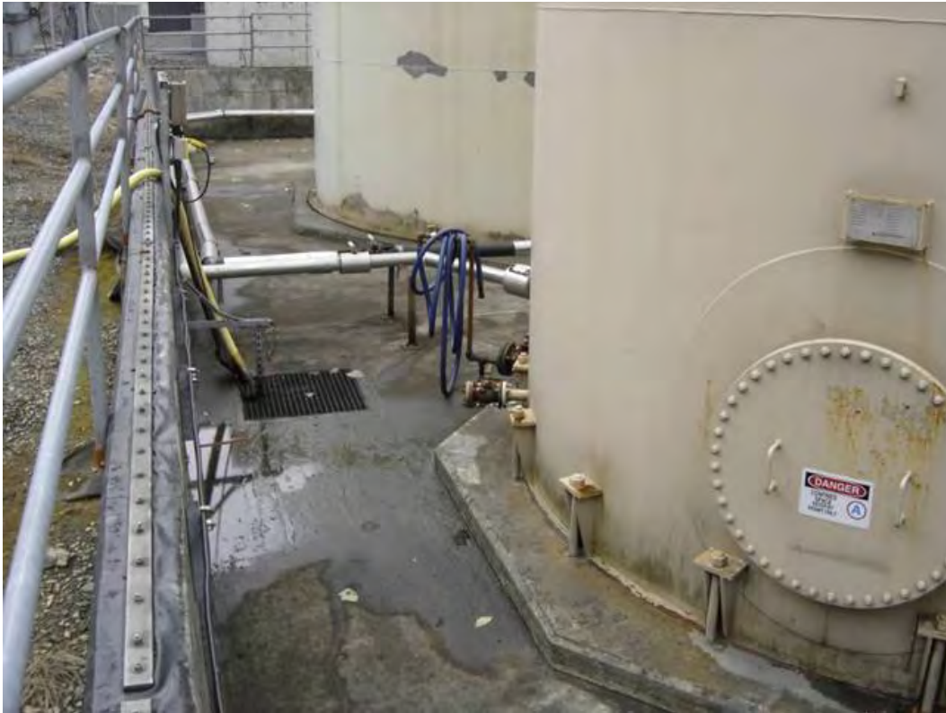
Photo 29: Secondary Containment for Fuel Storage at 920 Area
