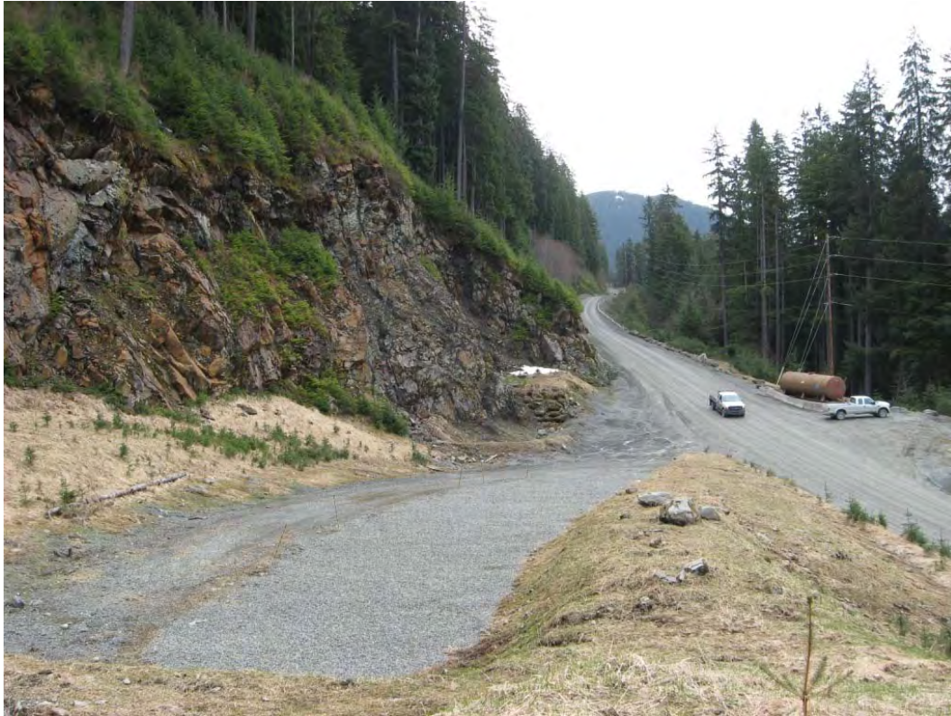
Photo 19: Looking down the access ramp that overlies reclaimed and revegetated production rock in Pit 174
