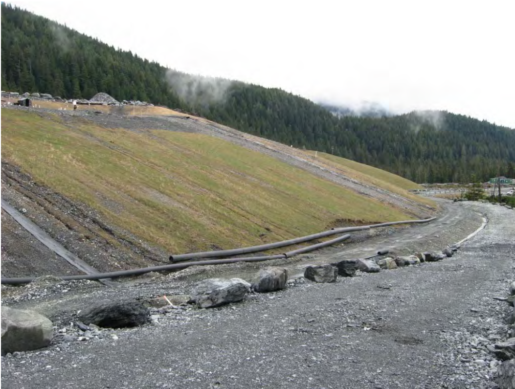
Photo 6: A revegetated slope, with a granular toe buttress, on the west side of the Tailings Disposal Facility
