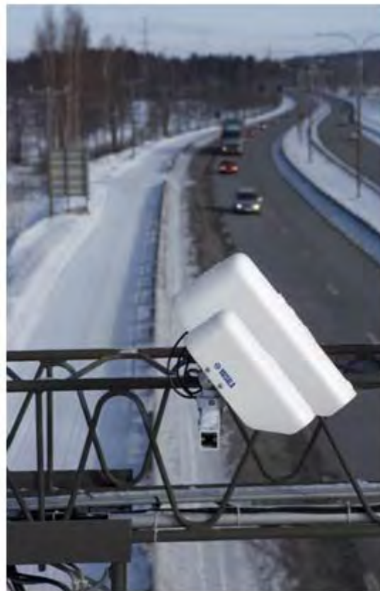
FIGURE 2 Nonintrusive sensors mounted on an overhead gantry.
